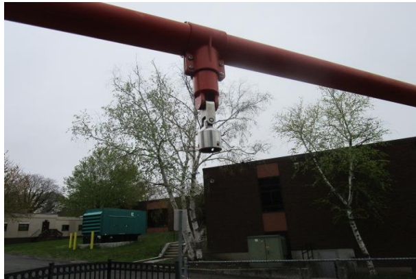
7ft. Tire Swing (Landscape) - Tire Swing seat is missing - MAINTENANCE
