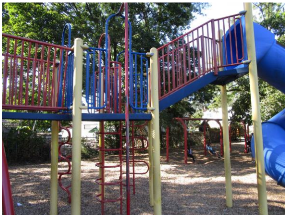
Climbing Pole - Slightly loose at top bracket - MAINTENANCE
