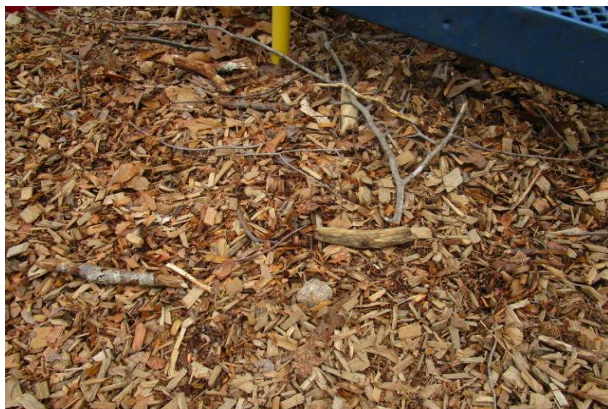
Surfacing - Rocks & debris in use zone - MAINTENANCE
