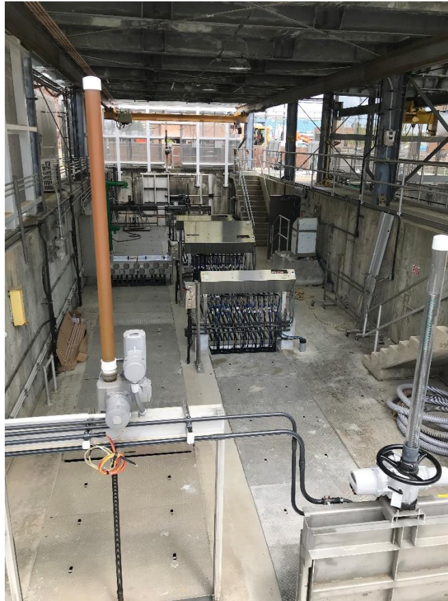
Wedeco system removed. TROJAN system in Channel 2
