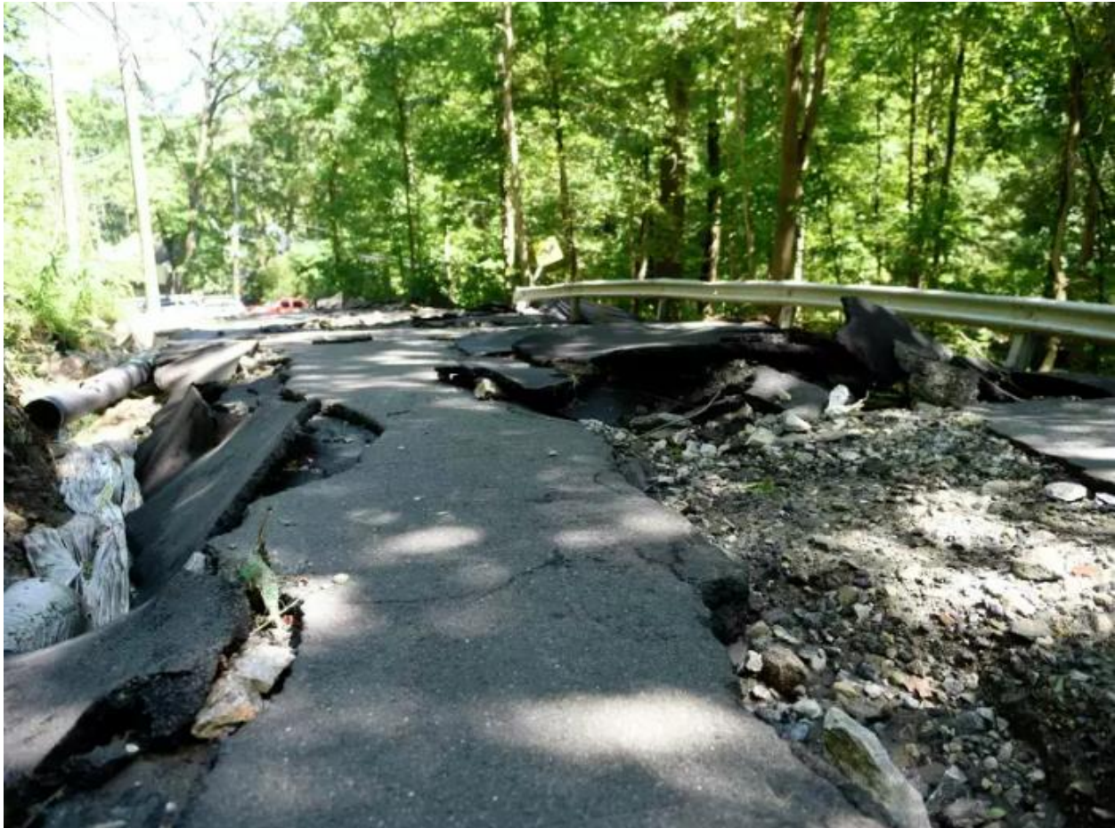
Figure 6 - Part of Farms Road, under construction at the time, collapsed and was washed away by Ida.
