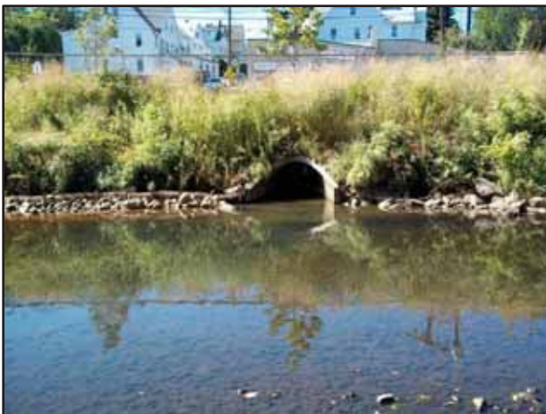
Photo 5. Outfall DIS 26/SON 008 drains to the Rippowam River.
