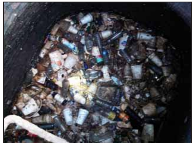
Photo 4. View of a storm manhole in Cummings Park that has accumulated a significant amount of garbage. .
