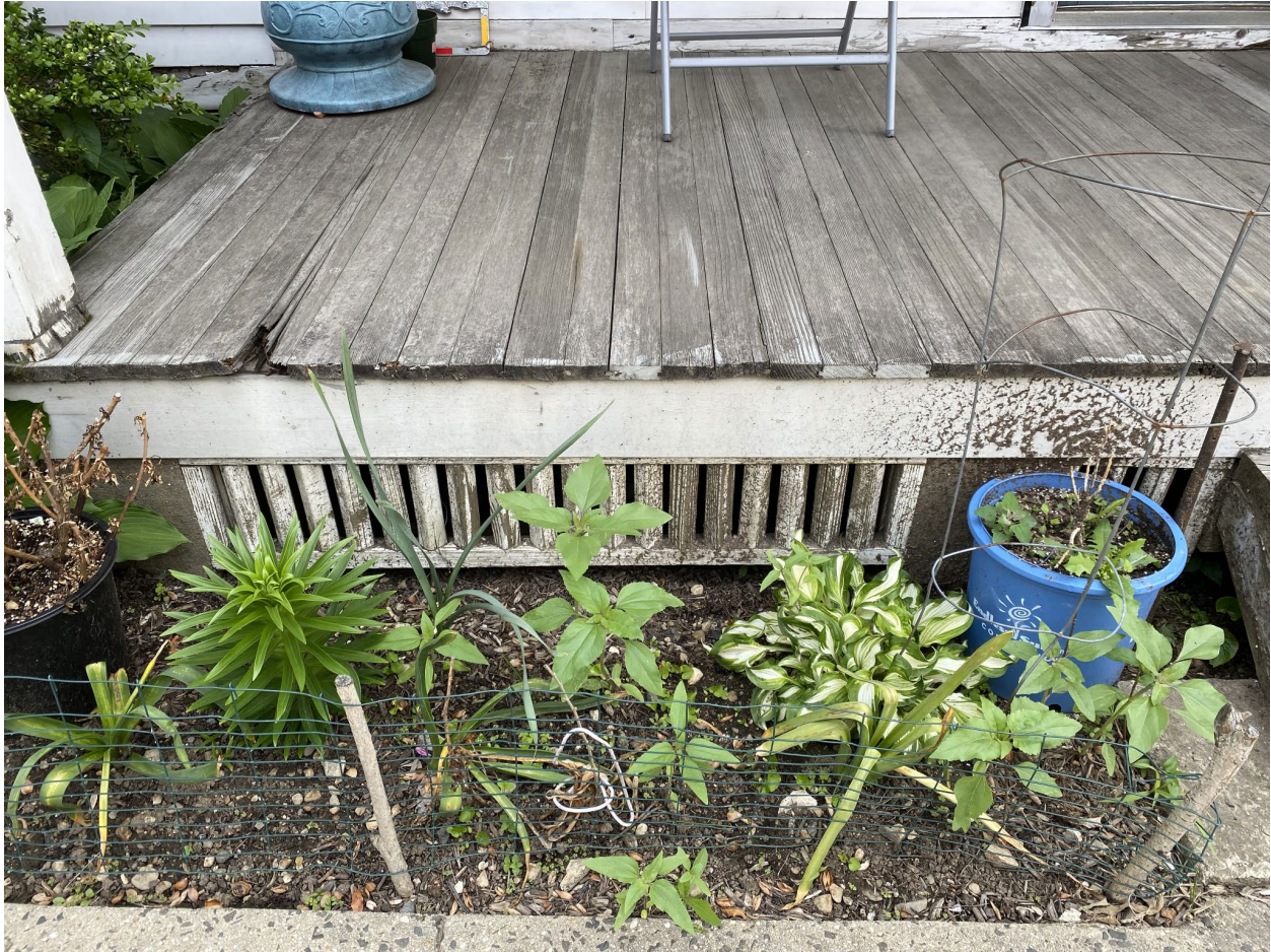
Fig. 6 Intact original decorative features such as this trelliswork under the front porches will be preserved and restored.
