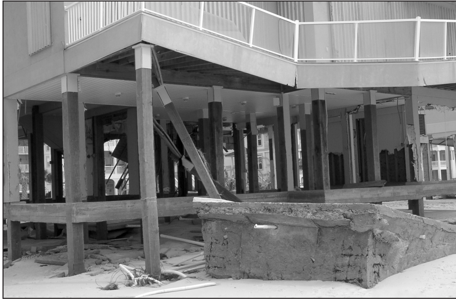
Figure 18. Movement of a spa likely caused failure of two piles supporting an elevated deck.
