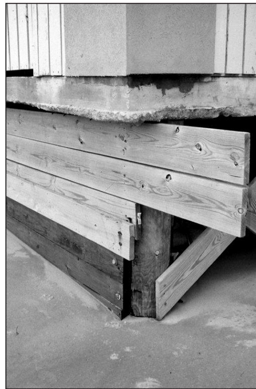
Figure 15. Shore-parallel timbers attached to a pile foundation were intended to act as a bulkhead, but constitute an obstruction and are prohibited.
