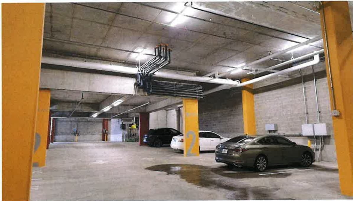
Figure 8- Level 3 – Parking Garage – Leaks at pipe penetrations near pool
