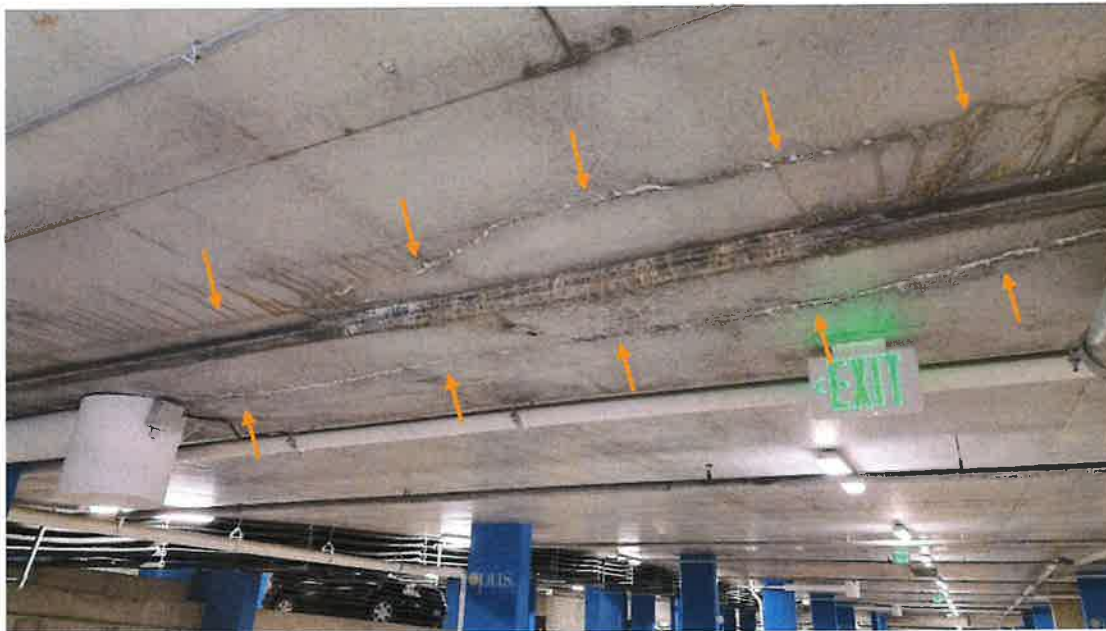
Figure 6- Level 1 - Parking Garage - Shrinkage cracks
