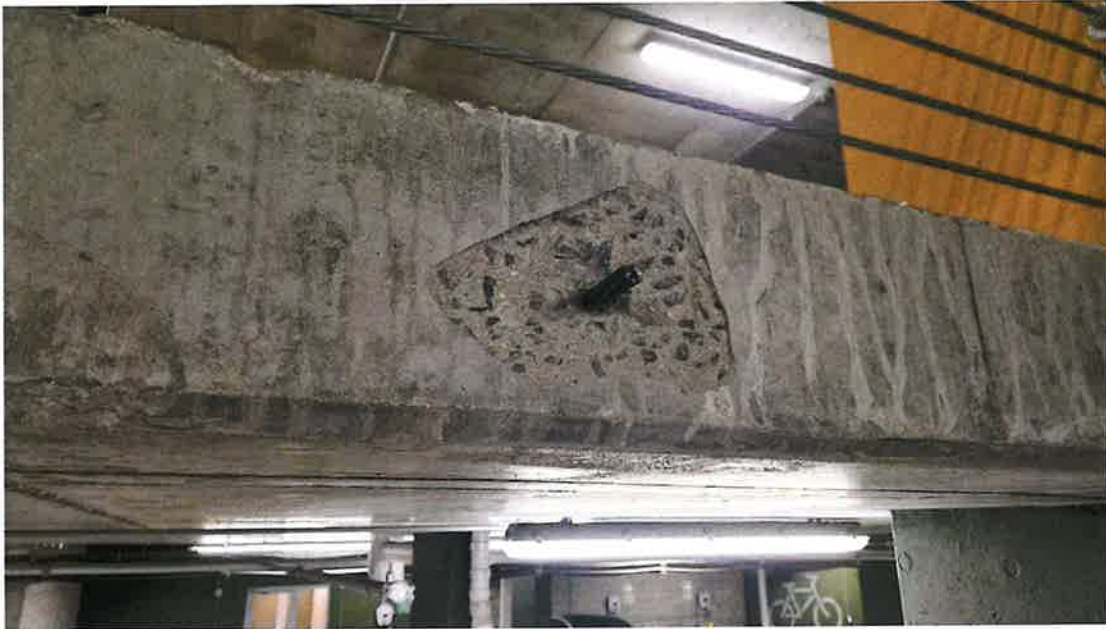
Figure 7- Level 2 - Parking Garage – Broken PT strand
