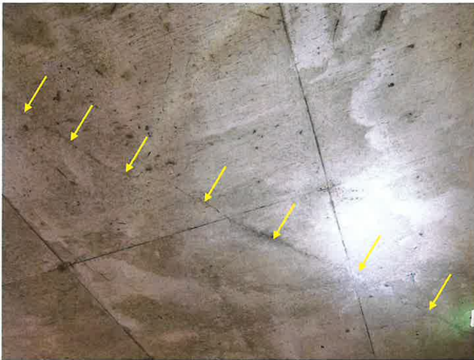
Figure 7- Hairline Shrinkage Cracks
