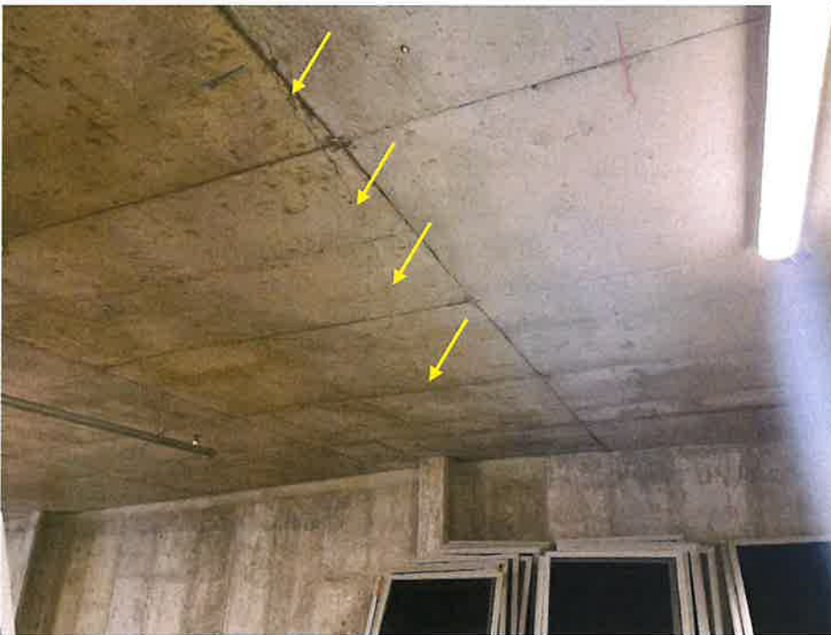
Figure 8- Hairline Shrinkage Cracks
