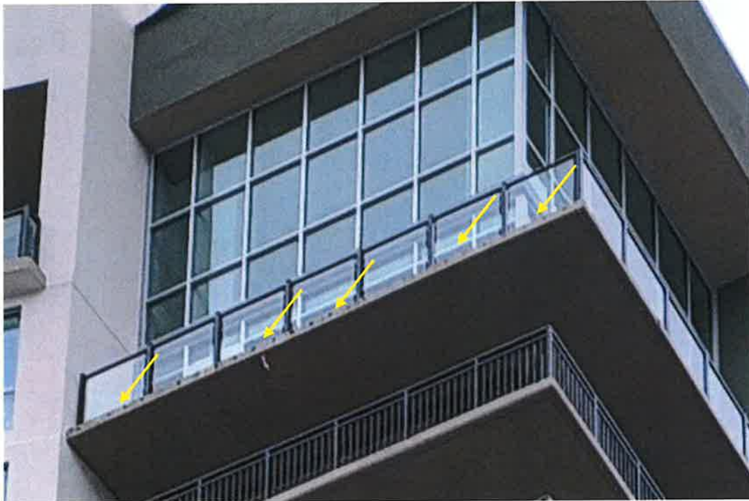
Figure 30- Possible Missing Grout at End Anchorages
