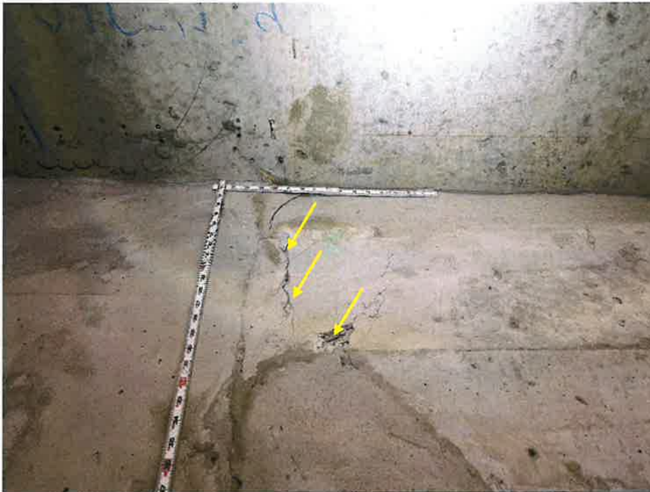
Figure 11- Cracking/Delamination at Beam to Column Connection
