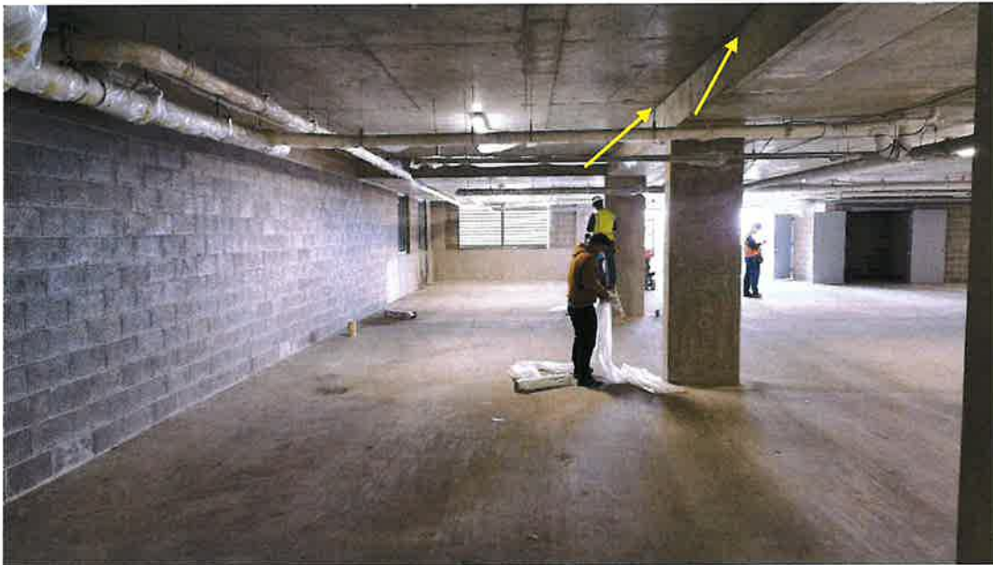
Figure 18- Step in 4 th Floor Terrace Level Slab
