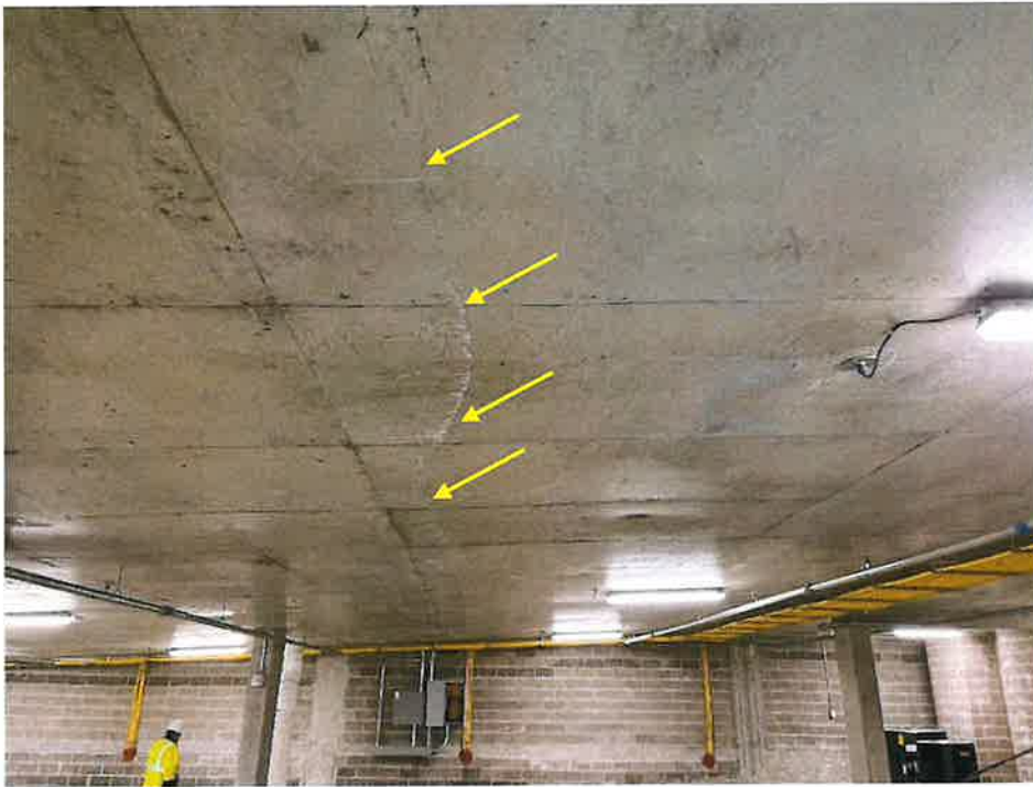
Figure 13- Shrinkage Crack with Efflorescence
