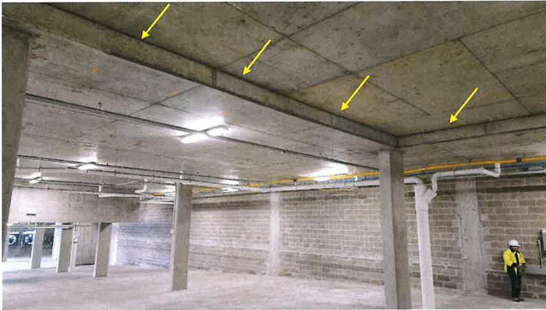
Figure 17- Step in 4 th Floor Terrace Level Slab
