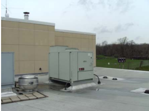
Photo #97: Rooftop air-cooled condensing unit at New AgriScience Building
