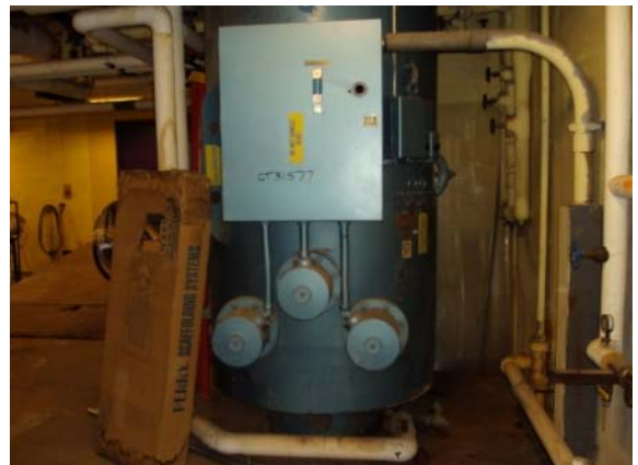
Photo #102: Domestic electric water heater at main mechanical room
