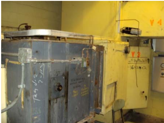
Photo #87: Air Handling Unit (V-3 & V-4)
