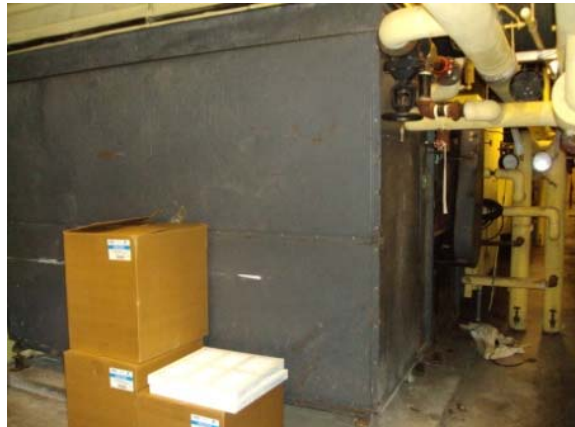
Photo #88: Air Handling Unit (V-7)
