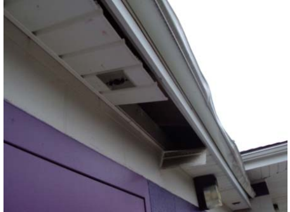
Photo #164: Damaged gutter and soffit
