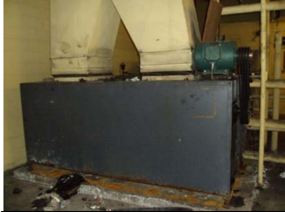
Photo #86: Air Handling Unit (AC-8)
