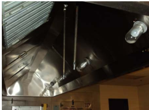
Photo #144: Exhaust hood with fire suppression above fryer
