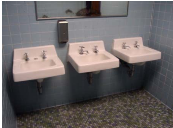
Photo #106: Common area restroom lavatory sinks
