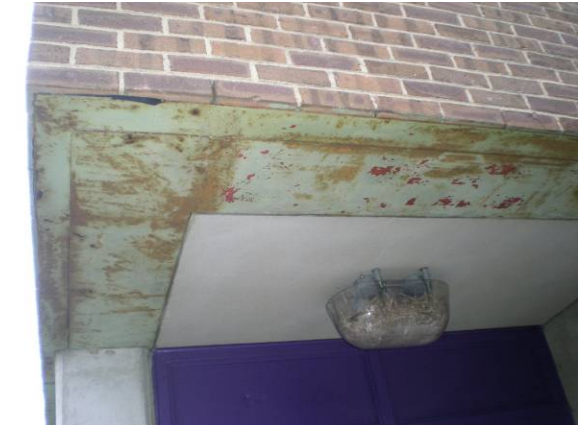
Photo #190: Steel lintel beginning to rust
