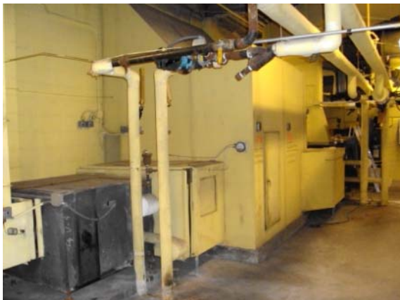
Photo #89: Air Handling Unit (V-9 & V-10)
