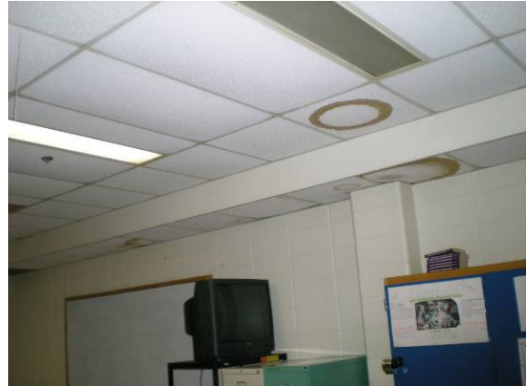
Photo #230: Leaks in classroom 435
