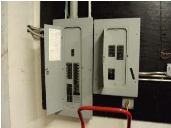
Photo #117: Main electrical switchgear at Old AgriScience Building
