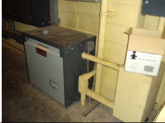
Photo #121: Step-down transformer
