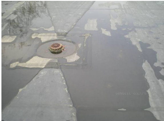
Photo #196: Large area of ponding at clogged roof drain
