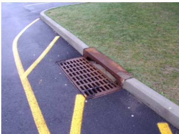
Photo #27: Drainage inlet at hard surface
