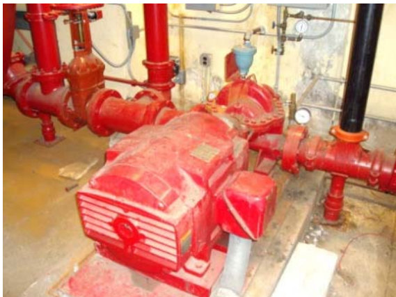
Photo #143: 1,000 GPM Fire pump
