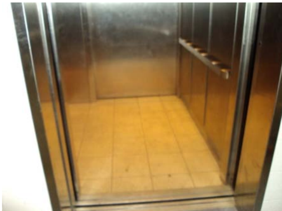
Photo #135: Elevator cab interior at New AgriScience Building
