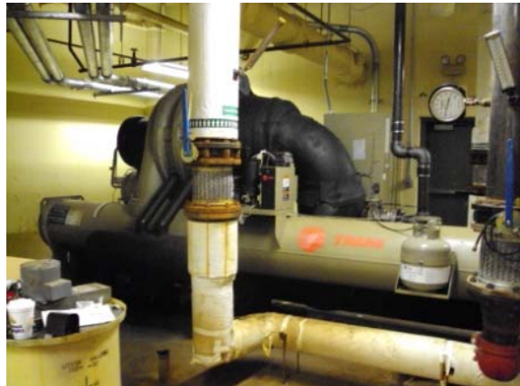
Photo #94: Chiller at basement mechanical room
