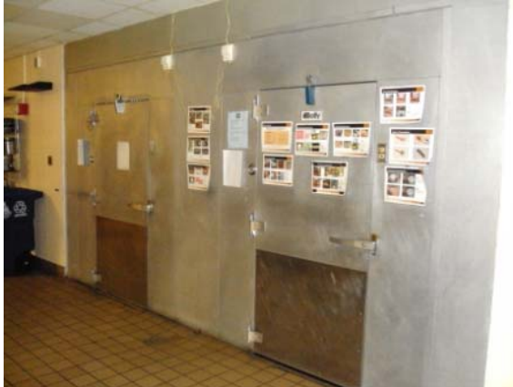
Photo #157: Walk in refrigerator and freezer
