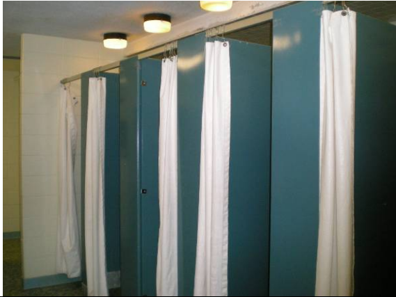
Photo #217: Showers in locker room off pool
