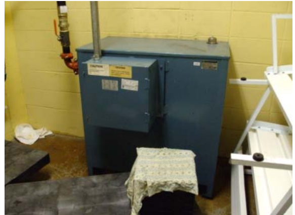
Photo #134: Hydraulic elevator machinery at main building
