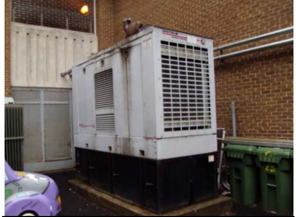
Photo #128: Generator for main building
