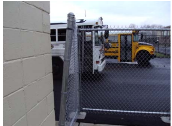
Photo #40: Damaged fence pole adjacent to Old AgriScience Building
