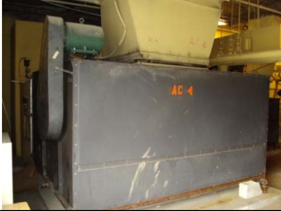
Photo #85: Air Handling Unit (AC-4)
