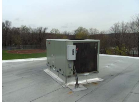
Photo #98: Rooftop air-cooled condensing unit at New AgriScience Building
