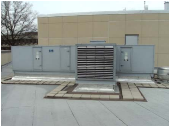
Photo #99: RTU-1 at New AgriScience Building
