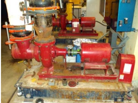
Photo #79: Hot water circulating pumps at main building
