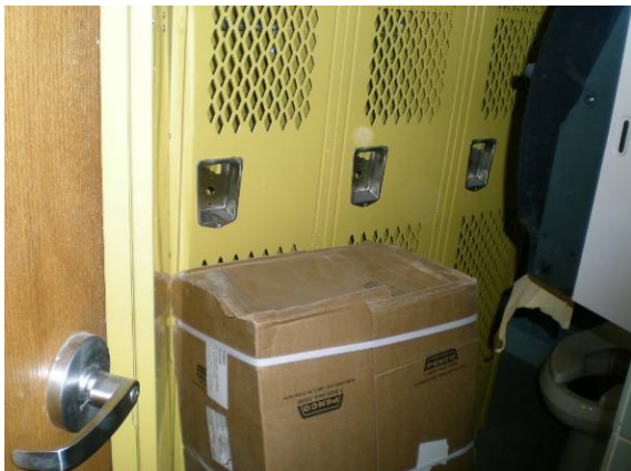
Photo #233: ADA shower/restroom in new gym locker room used for storage
