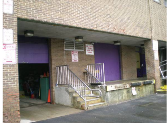
Photo #182: Loading dock damage at brick overhead
