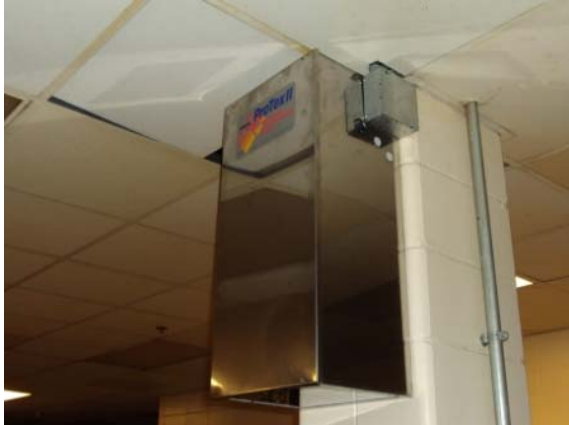
Photo #145: Fire suppression equipment for kitchen hood
