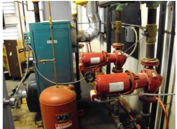
Photo #76: Heating boiler, circulator pumps and expansion tank at Old AgriScience Building
