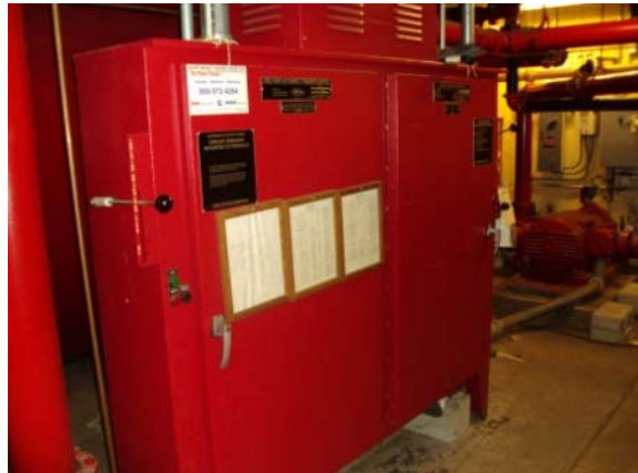
Photo #142: Fire pump controller
