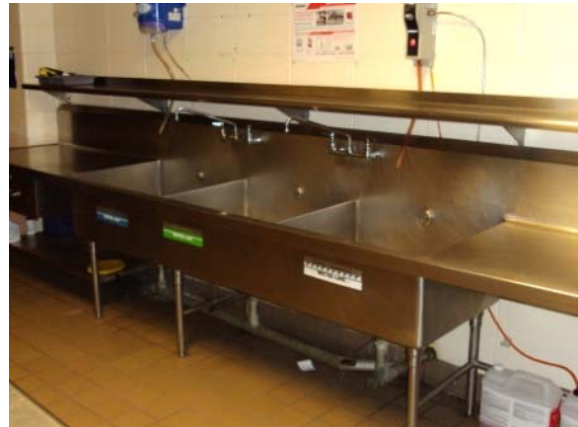
Photo #160: 3-Compartment sink in kitchen
