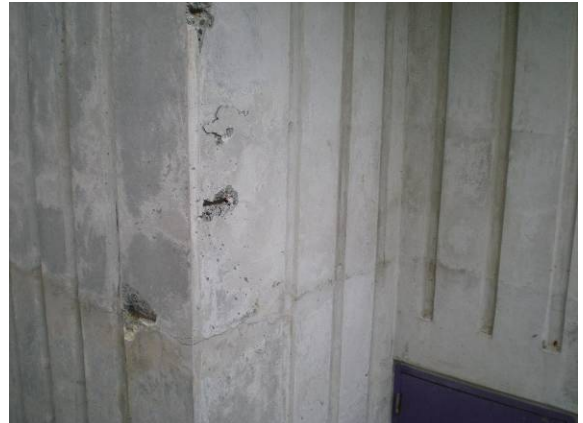
Photo #172: Concrete foundation wall with failing patches, exposed steel rebar and severe spalling
