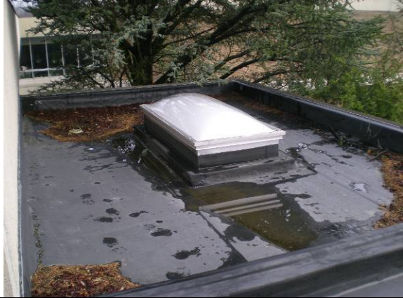
Photo #194: Clogged roof drain and ponding at small roof section at NE corner of Raynor (B) Wing
