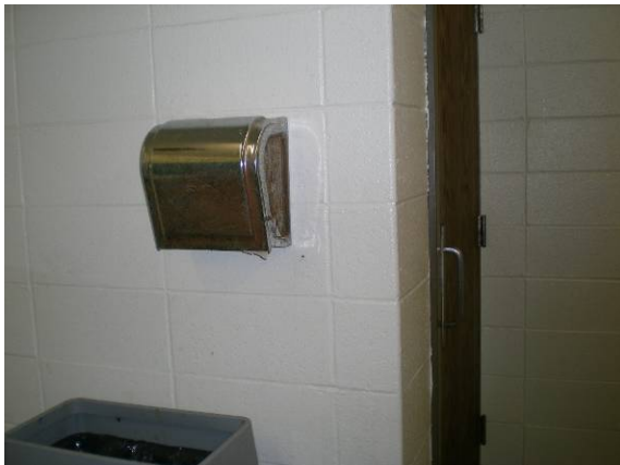
Photo #219: Paper towel dispenser requiring replacement due to twisting mechanism
