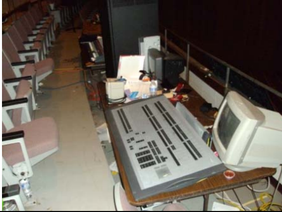
Photo #127: Auditorium audio controls
