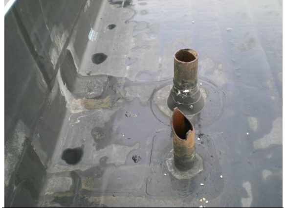
Photo #266: Close up of roof vent damage at old AgriScience Building
