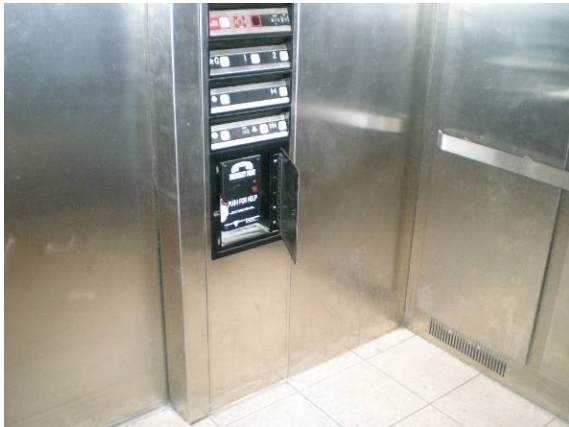
Photo #257: Elevator control panel
