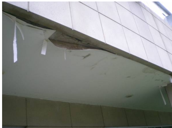
Photo #240: Peeling soffit at New AgriScience
