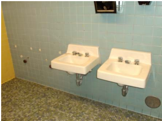
Photo #107: Common area restroom lavatory sinks with two missing sinks
