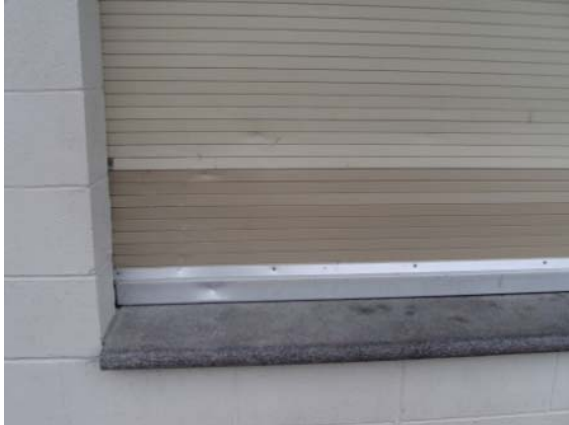
Photo #163: Damaged roll-up door
