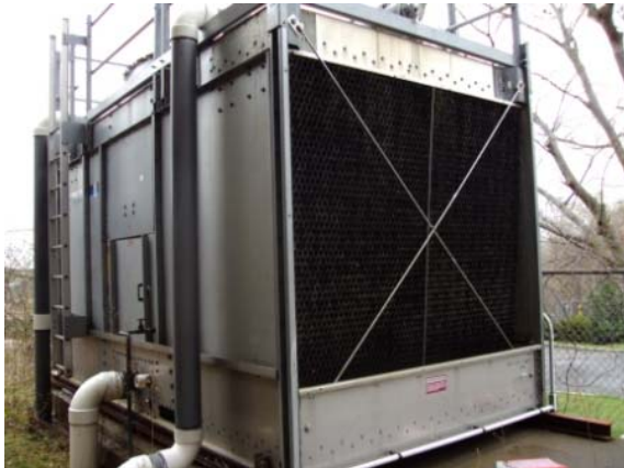
Photo #93: Cooling tower at east side of building
