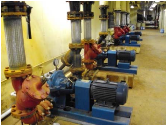
Photo #95: Chilled water circulating pumps at basement mechanical room
