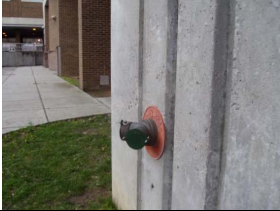
Photo #151: Siamese connection at front of building
