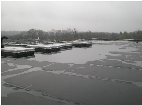
Photo #198: Large area of ponding at auditorium roof smoke evacuation hatches
