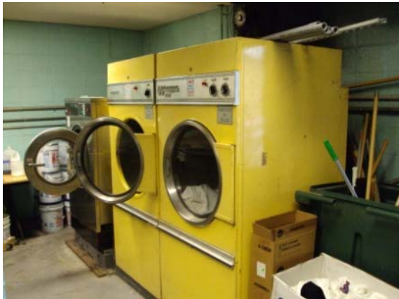
Photo #153: Commercial washer and dryers adjacent to rear loading dock
