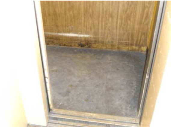
Photo #133: Elevator cab interior at main building
