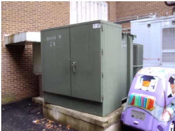
Photo #119: Pad-mounted transformer at rear of main building
