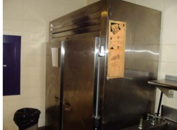
Photo #158: Refrigeration unit in kitchen
