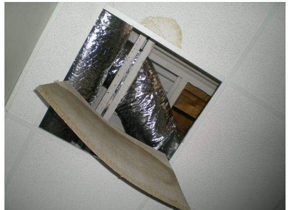
Photo #268: Leak at old skylight locations
