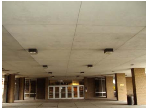
Photo #34: Surface-mounted light fixtures at covered walkways
