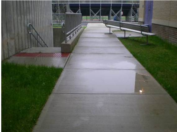
Photo #175: Ponding along walkway between old gym and new gym
