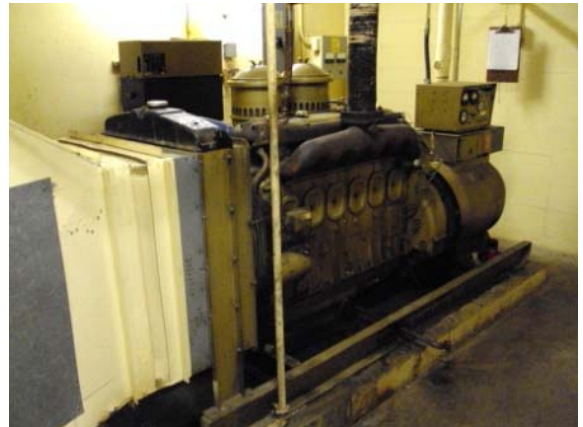
Photo #130: Generator for auditorium
