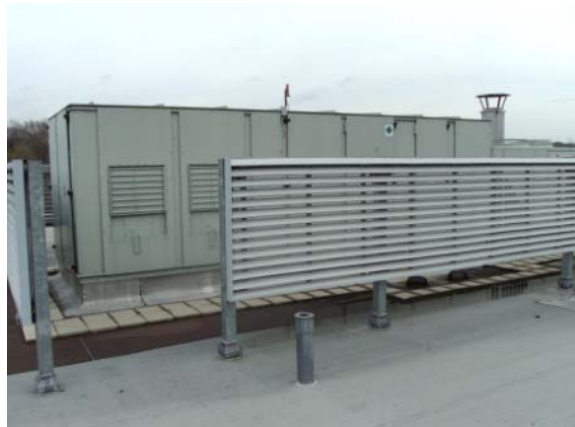
Photo #96: Rooftop air-cooled condensing unit at New AgriScience Building
