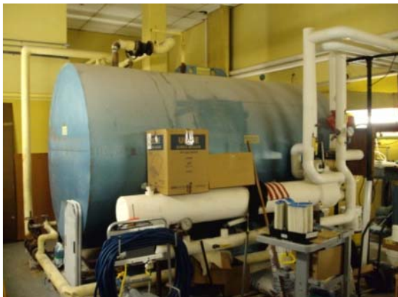
Photo #101: Domestic electric water heater and heat exchanger at pool filter room
