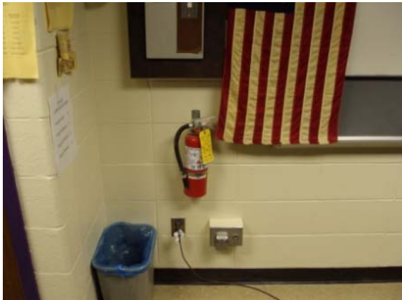
Photo #147: Fire extinguisher in classroom
