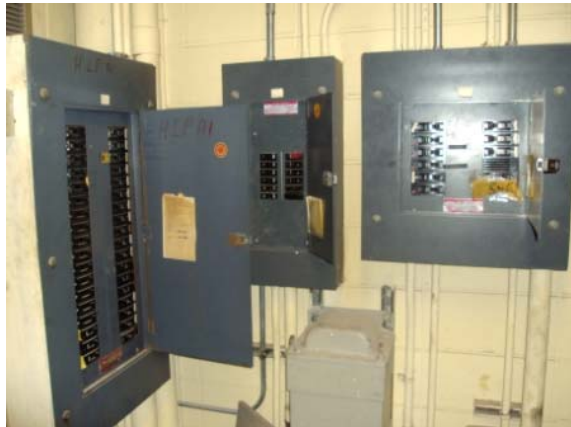
Photo #123: Electrical panels
