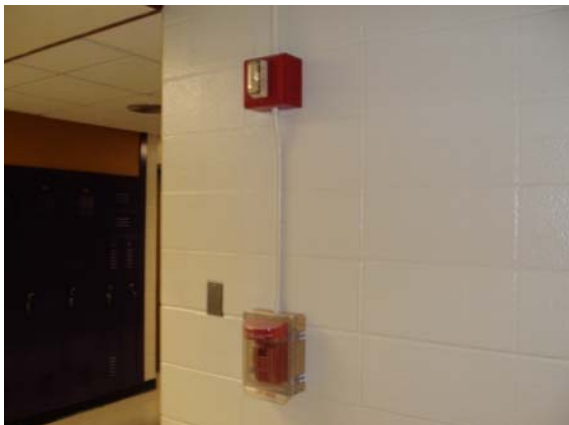
Photo #149: Common area fire pull station and strobe alarm
