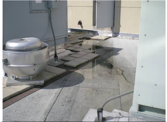
Photo #248: Ponding at entrance to roof of new AgriScience Building
