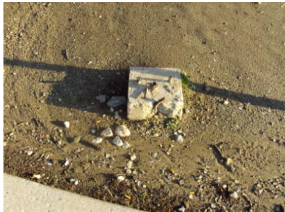
Photo #36: Abandoned pole light concrete base at front sidewalk
