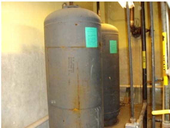
Photo #77: Expansion tanks at main building
