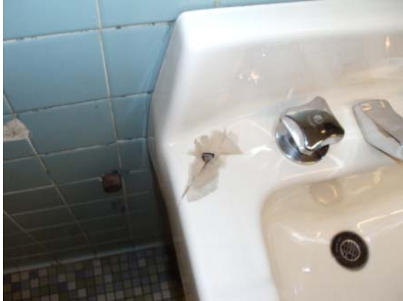
Photo #109: Common area restroom with broken lavatory sink
