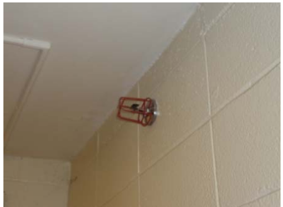
Photo #150: Fire sprinkler head
