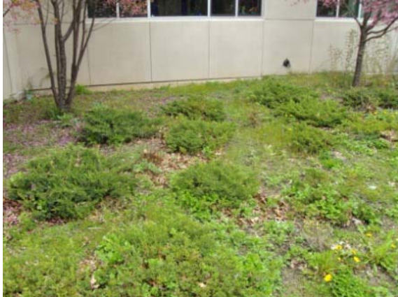
Photo #25: Landscaping sloped towards foundation wall at New AgriScience Building
