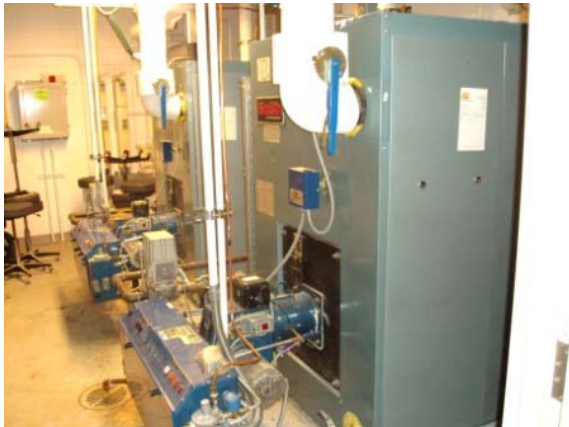
Photo #75: Heating boilers at New AgriScience Building (greenhouse mechanical room)
