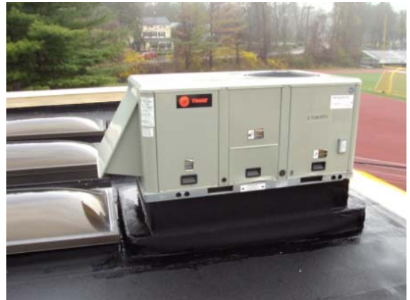
Photo #72: Rooftop package unit at Old AgriScience Building
