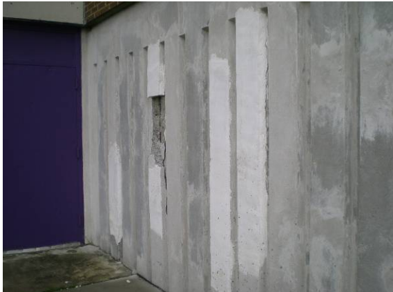
Photo #171: Concrete foundation wall with failing patches, exposed steel rebar and severe spalling
