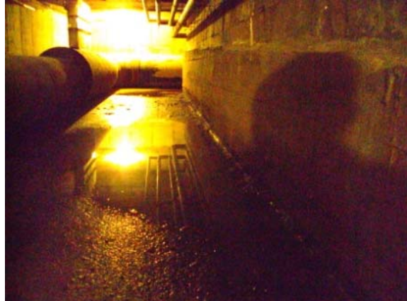
Photo #26: Water in tunnel below pool from overflowing sump pump basin, due to non-operational sump pump
