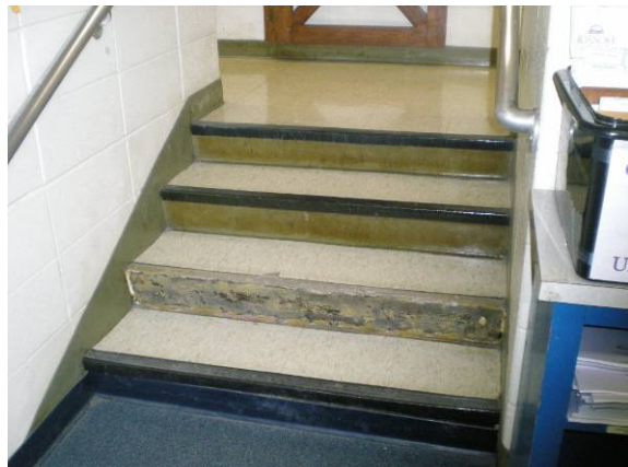
Photo #204: Finishes in guidance center – missing stair riser nosing and vinyl surface
