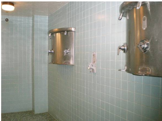
Photo #221: Shower controls in Boys' Locker room for pool too high and require twisting
