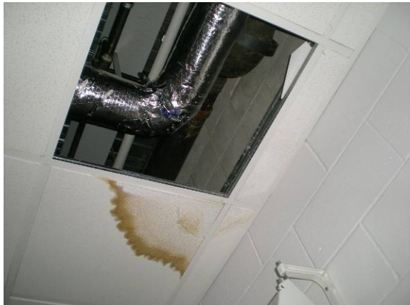
Photo #258: Leak in classroom #12
