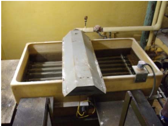
Photo #69: Pool filtration equipment
