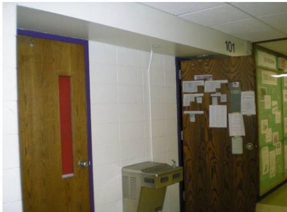
Photo #208: Protruding drinking fountain and knob handle hardware at classroom
