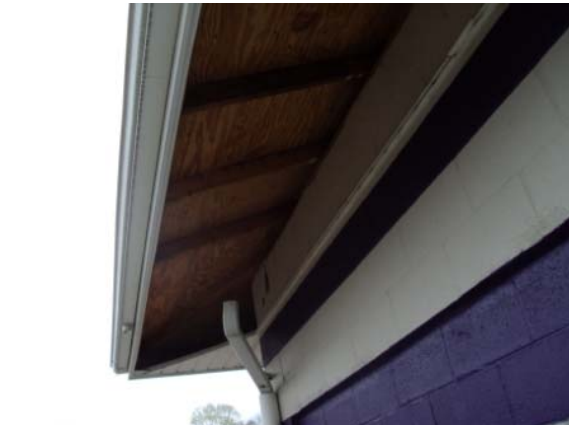
Photo #165: Unattached downspout and missing soffit
