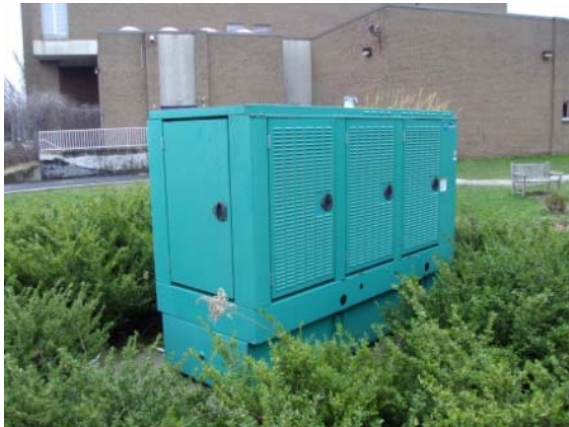
Photo #129: Generator for New AgriScience Building
