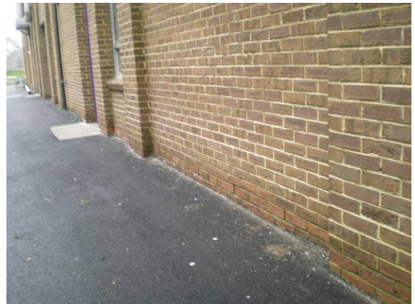
Photo #184: Worn mortar along base of wall perimeter including perimeter of old gym area, loading dock and audit.
