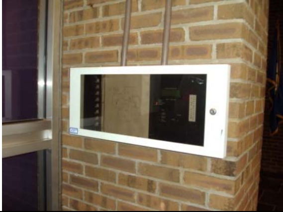
Photo #139: Annunciator panel at lobby
