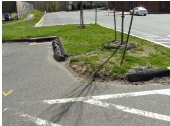
Photo #24: Deteriorated and displaced asphalt curbing adjacent to baseball field
