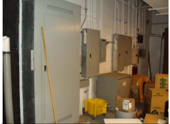
Photo #116: Main electrical switchgear at New AgriScience Building
