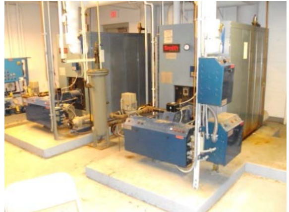
Photo #74: Heating boilers at New AgriScience Building (main mechanical room)
