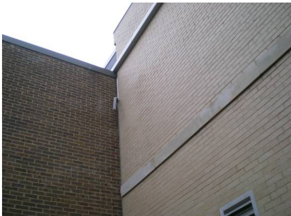
Photo #173: Loose gasket at joint of 9 th grade wing and original building
