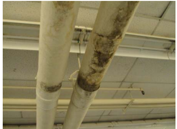
Photo #112: Suspect mold on pipe insulation at weight room #1
