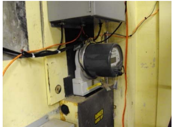
Photo #118: Main electric meter at main building basement adjacent interior vault
