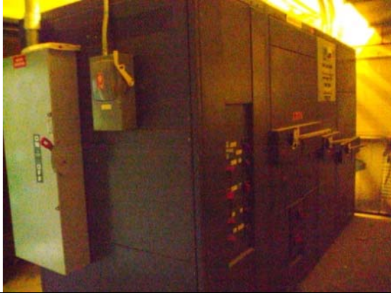
Photo #115: Main electrical switchgear at main building
