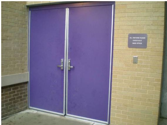
Photo #177: One of a few pairs of doors that do not close properly
