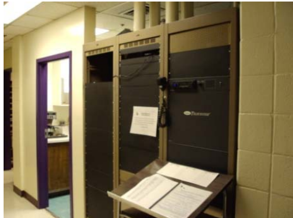
Photo #124: School PA system equipment at office
