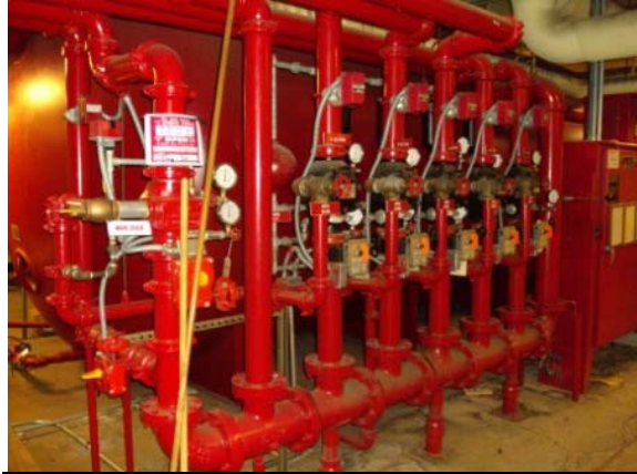
Photo #140: Main fire suppression system risers at main mechanical room
