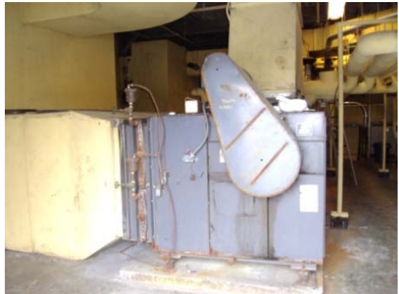
Photo #84: Air Handling Unit (AC-1)
