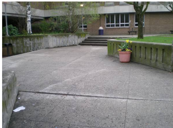
Photo #180: Potential tripping condition in courtyard with vertically displaced concrete
