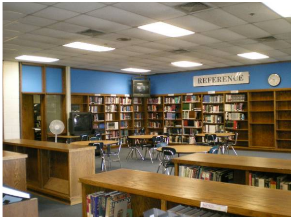
Photo #226: Cupping acoustic tiles in Media Center
