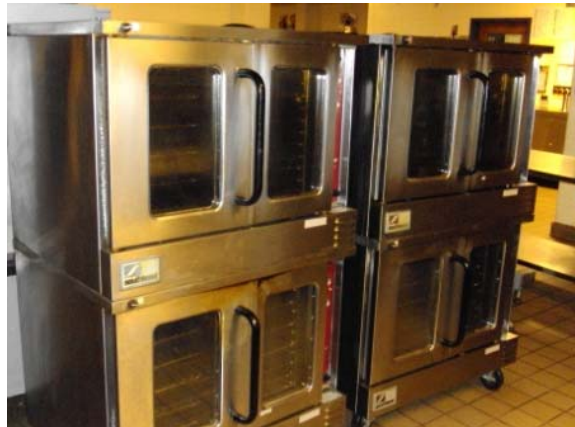
Photo #154: Kitchen ovens
