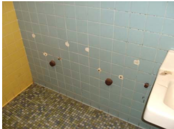
Photo #108: Common area restroom missing two lavatory sinks
