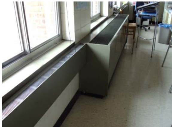
Photo #90: Classroom floor-mount unit ventilator and cabinet radiant heater
