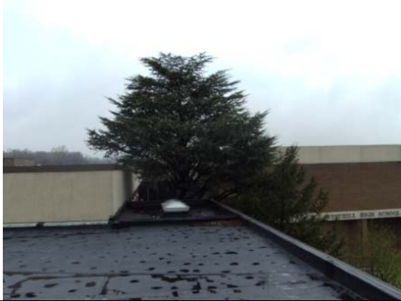
Photo #31: Overgrown tree at front of building
