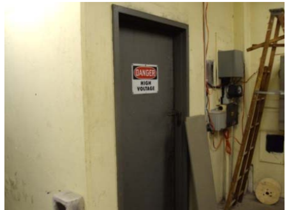
Photo #120: Interior vault at basement mechanical room
