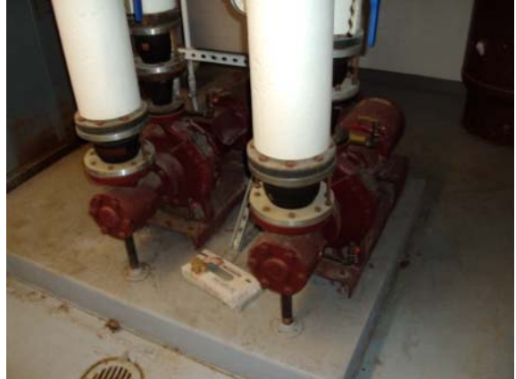
Photo #80: Hot water circulating pumps at New AgriScience Building
