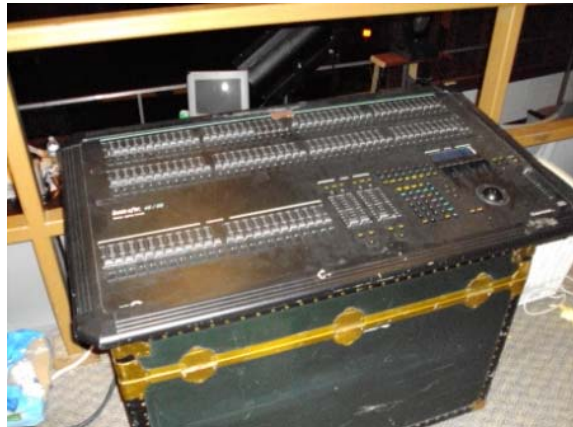
Photo #126: Auditorium light controls
