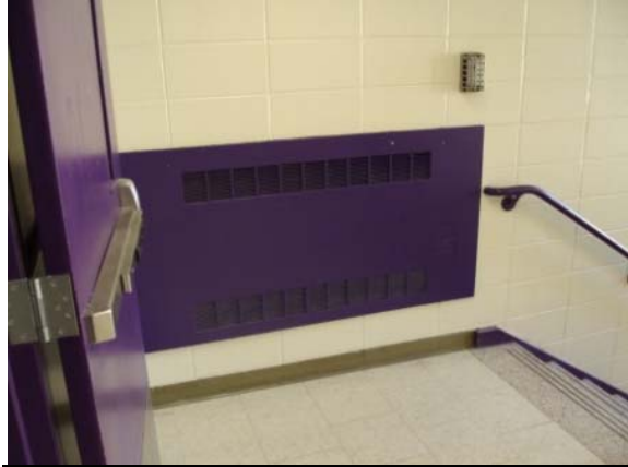
Photo #92: Recessed cabinet-mounted radiant heat unit at stairs
