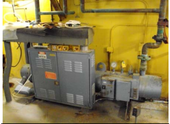
Photo #68: Pool electric heater
