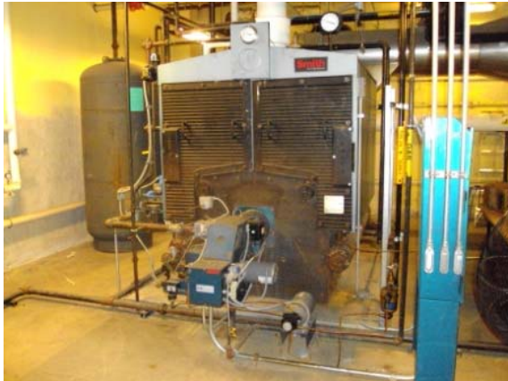
Photo #73: Heating boilers at main building (1 of 4)
