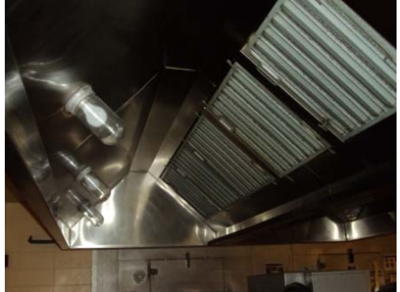
Photo #146: Missing sprinkler heads above portion of kitchen hood
