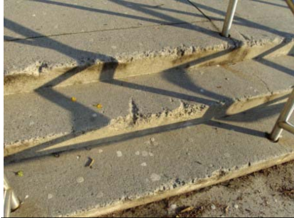
Photo #20: Damaged concrete steps
