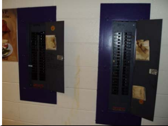
Photo #122: Electrical panels at main kitchen
