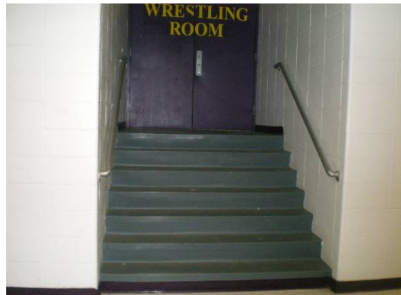
Photo #234: No ADA access to wrestling room
