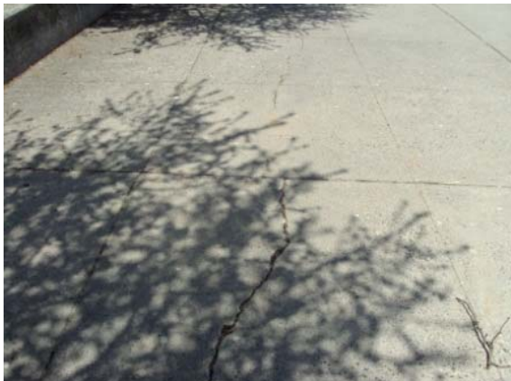
Photo #17: Cracking at concrete sidewalk at front of building
