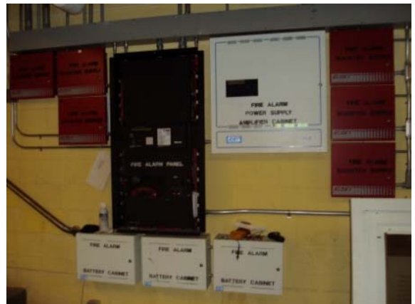
Photo #138: Central fire alarm panel at main mechanical room
