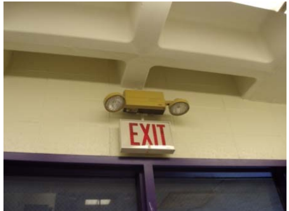
Photo #148: Illuminated exit sign and emergency lights
