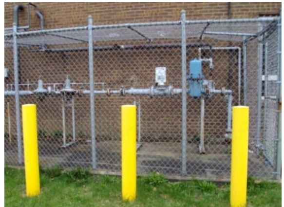
Photo #114: Enclosed and protected gas metering
