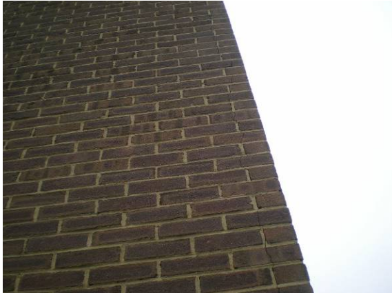
Photo #187: Minor cracking of brick veneer at corner
