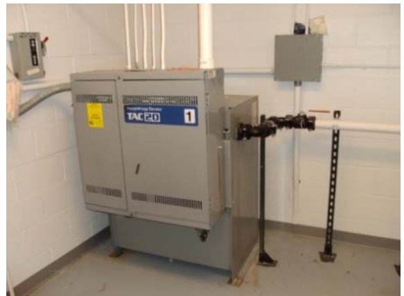
Photo #136: Hydraulic elevator machinery New AgriScience Building
