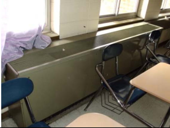
Photo #91: Classroom floor-mount unit ventilator
