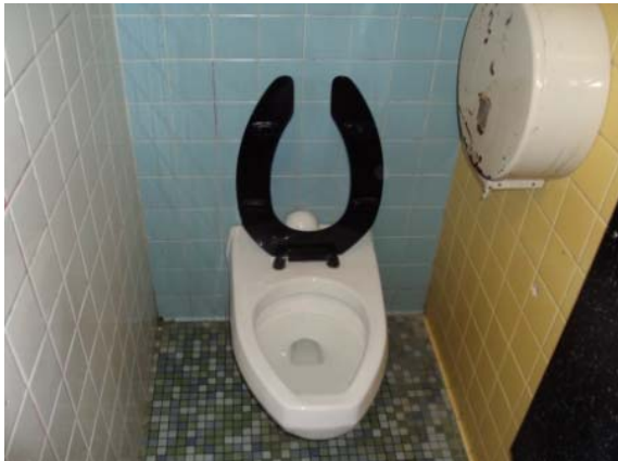
Photo #111: Wall-mounted toilet at common area restroom
