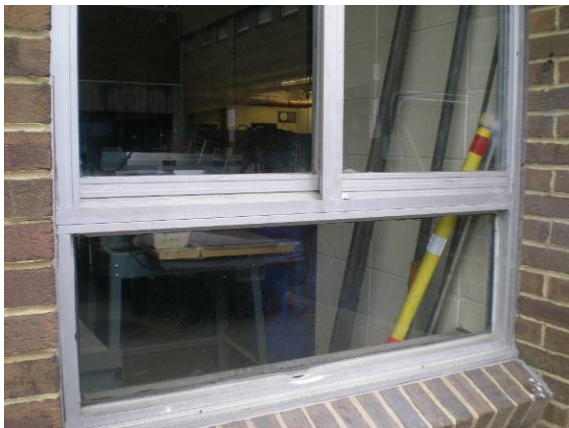
Photo #185: Single paned sliding window with damaged frame
