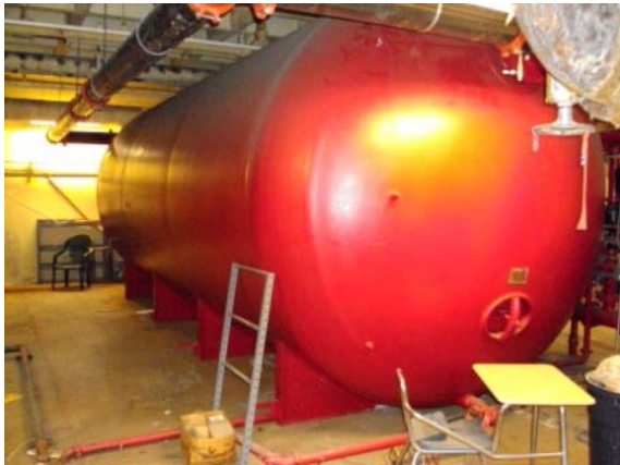
Photo #141: Water storage for fire suppression system
