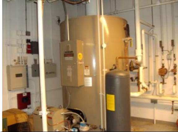
Photo #104: Domestic water heater at New AgriScience Building
