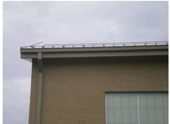
Photo #192: Damaged snow guard over new gym entrance – overall design of snow guard does not work
