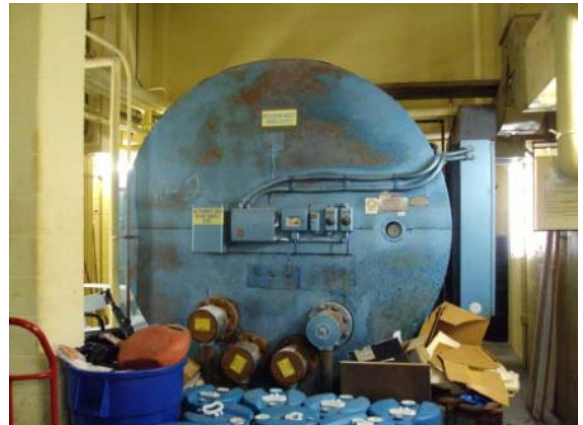
Photo #100: Domestic electric water heater at pool filter room
