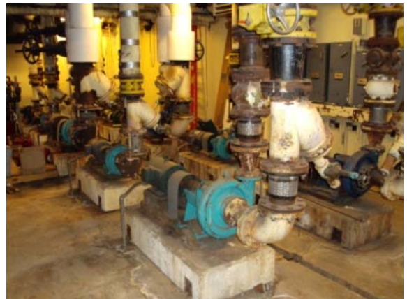
Photo #78: Hot water circulating pumps at main building
