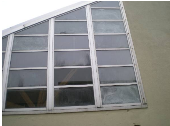
Photo #262: Close up of window damage
