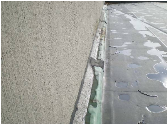
Photo #195: Roof flashing improperly shaped to hold water
