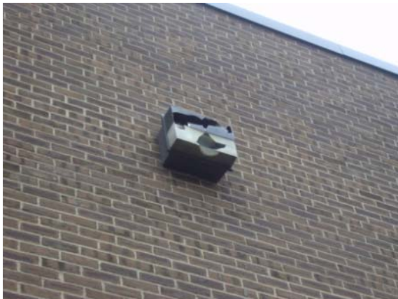
Photo #35: Damage building-mounted wall light at west side elevation of the building
