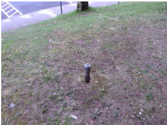
Photo #131: Buried UST fuel oil storage tank for auditorium generator
