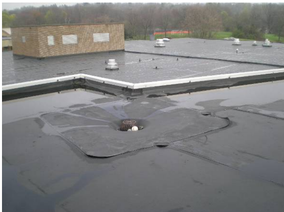
Photo #197: Failing roof patches and ponding areas not sloped to existing drains
