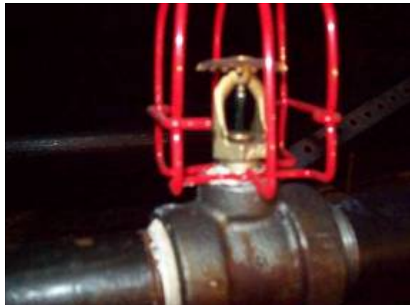
Photo #126: Fire sprinkler piping and head
