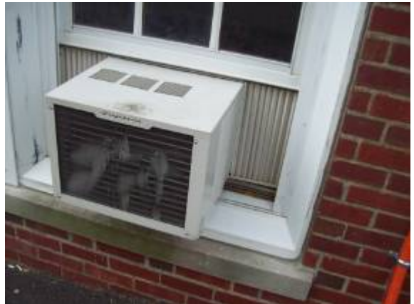
Photo #70: Typical window air conditioning unit
