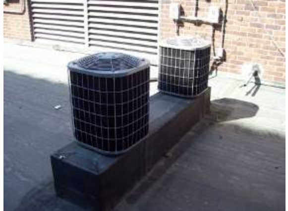
Photo #68: Small roof-mounted condensing units
