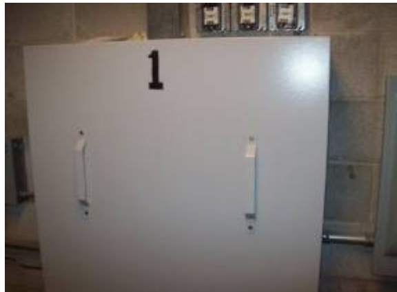
Photo #114: Elevator 3 control unit
