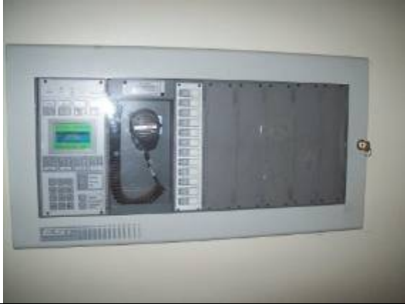
Photo #127: Fire alarm annunciator panel
