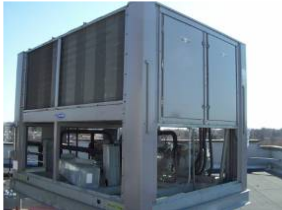
Photo #52: Condensing unit for cafeteria
