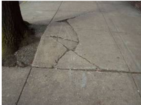
Photo #16: Sidewalk damage near gymnasium
