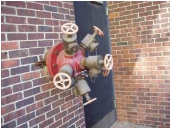
Photo #123: Fire department hose connection
