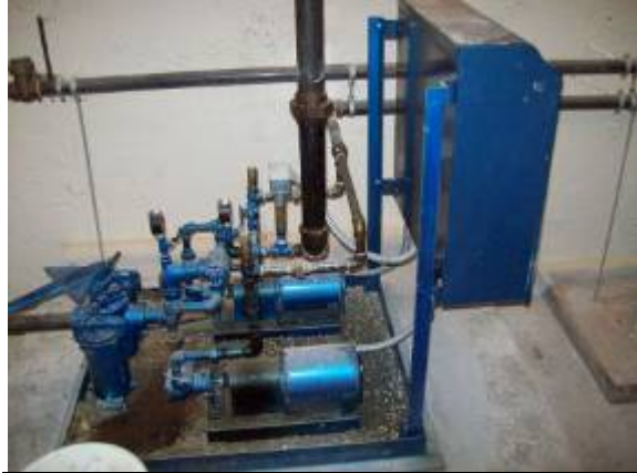
Photo #44: Fuel oil pump set
