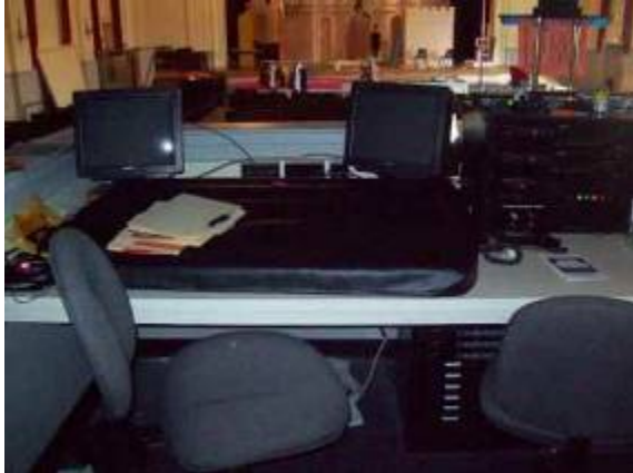
Photo #97: Auditorium lighting and sound control booth
