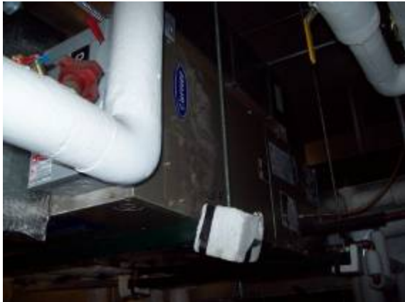
Photo #65: Typical split system air handling unit
