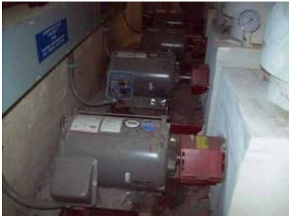
Photo #45: Circulating pumps
