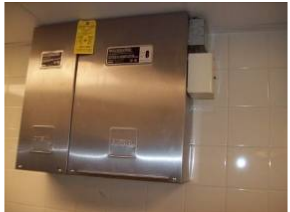
Photo #132: Ansul tanks in kitchen
