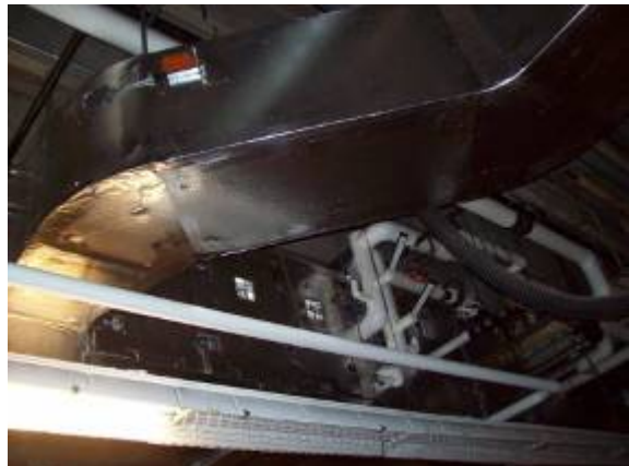
Photo #60: Air handling unit for Choral Room
