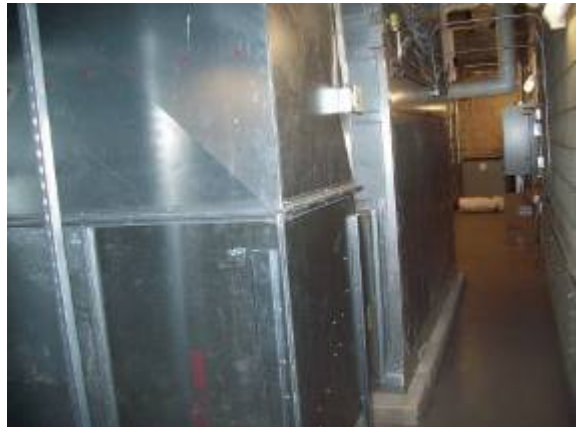
Photo #58: Air handling unit for gymnasium (1 of 2)
