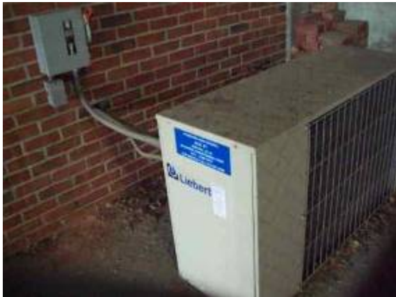
Photo #69: Liebert condensing unit for computer room
