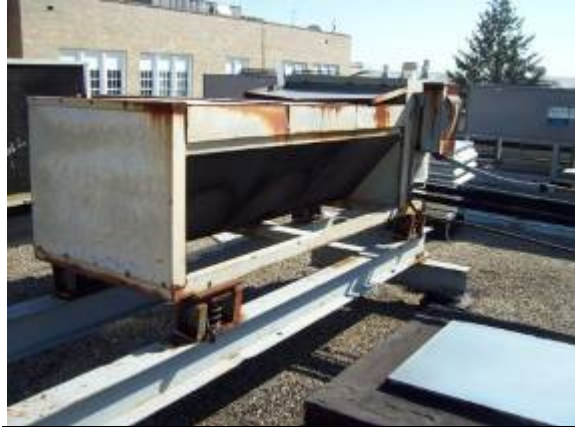
Photo #74: Condensing unit for Guidance Office
