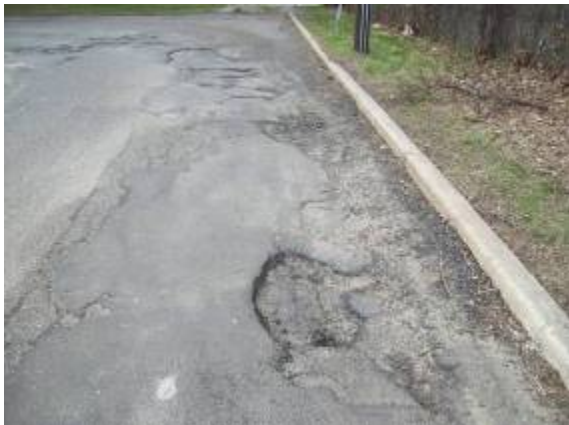
Photo #11: Typical asphalt damage
