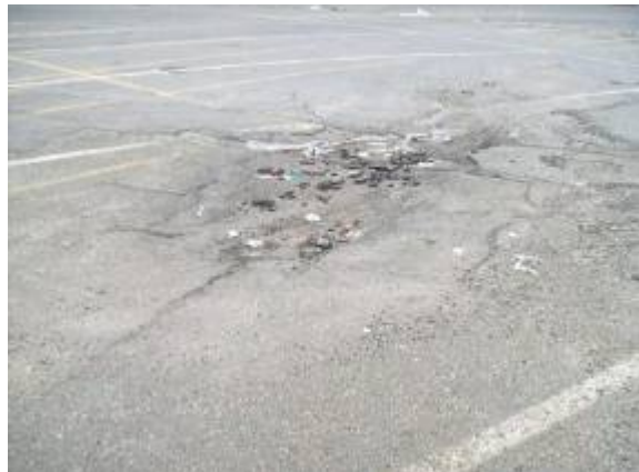
Photo #12: Typical asphalt damage
