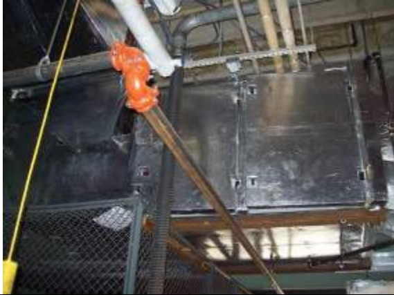
Photo #61: Air handling unit for Auto Mechanic Room
