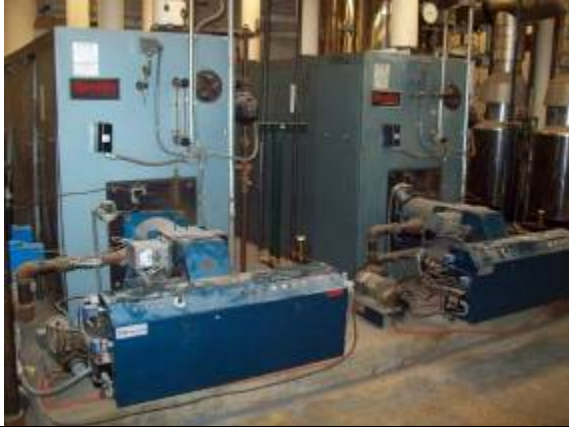
Photo #43: Boilers (2 of 4)
