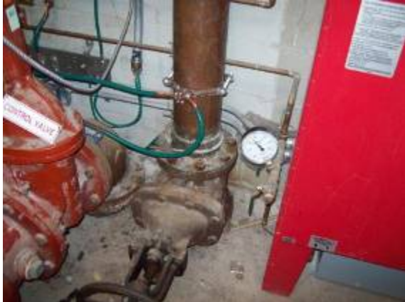
Photo #79: Incoming domestic water service
