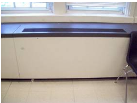
Photo #47: Typical unit ventilator for classroom
