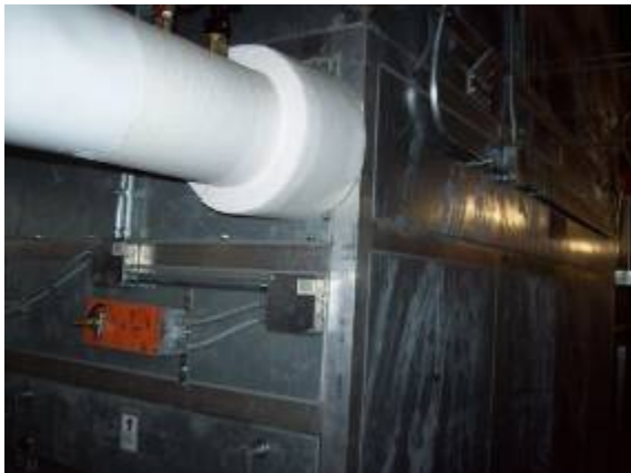
Photo #59: Air handling unit for gymnasium (2 of 2)
