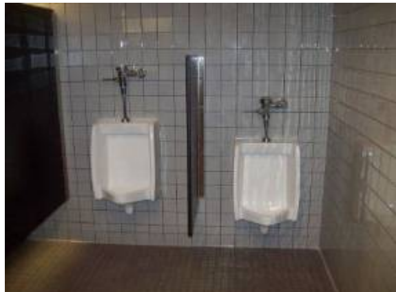
Photo #84: Restroom fixtures – urinals
