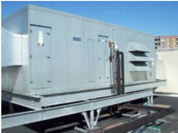
Photo #51: Ventilation unit for cafeteria
