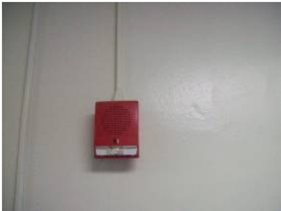
Photo #131: Fire alarm horn with strobe light
