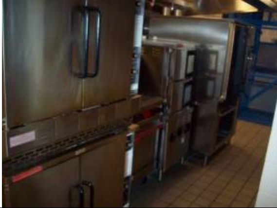
Photo #133: Kitchen equipment – Ovens
