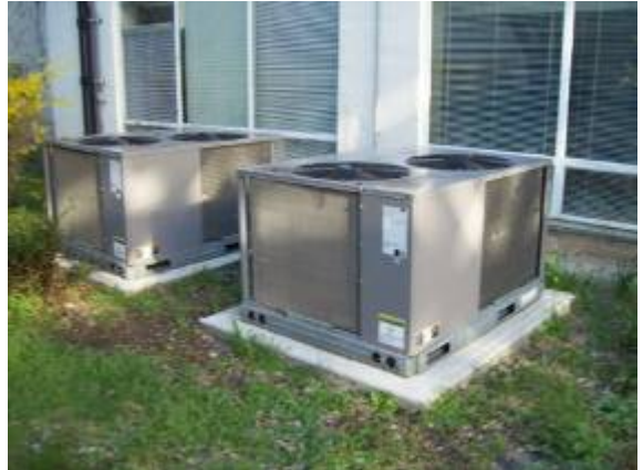
Photo #64: Typical pad-mounted condensing unit
