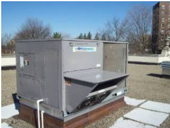
Photo #71: Rooftop unit for Large Group Instructional area
