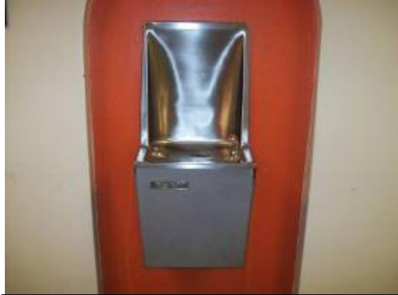
Photo #86: Plumbing fixtures – drinking fountain
