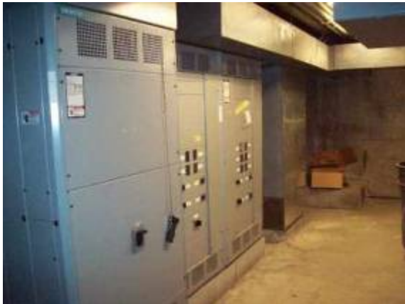
Photo #87: Main electrical switchgear
