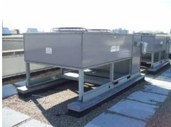
Photo #54: Condensing units for cafeteria
