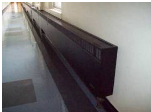
Photo #48: Wall mounted radiant heat unit for corridor
