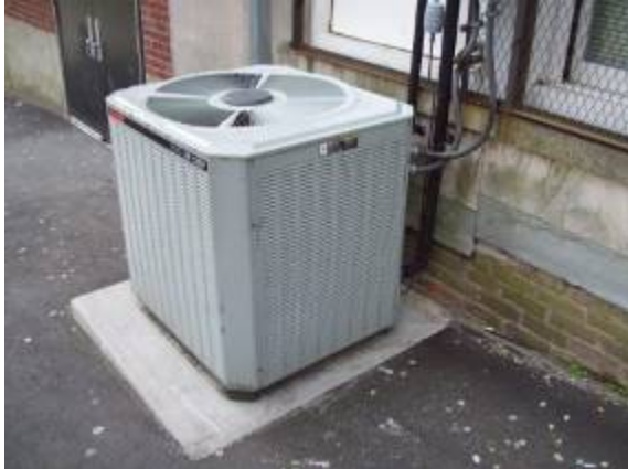
Photo #67: Typical pad-mounted condensing unit
