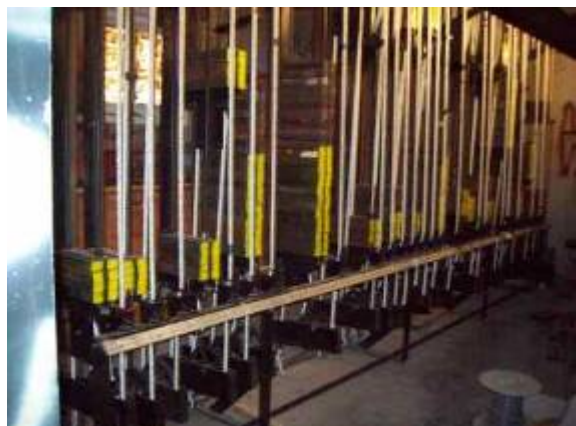
Photo #102: Stage rigging system
