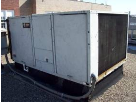
Photo #73: Rooftop unit for Guidance Office
