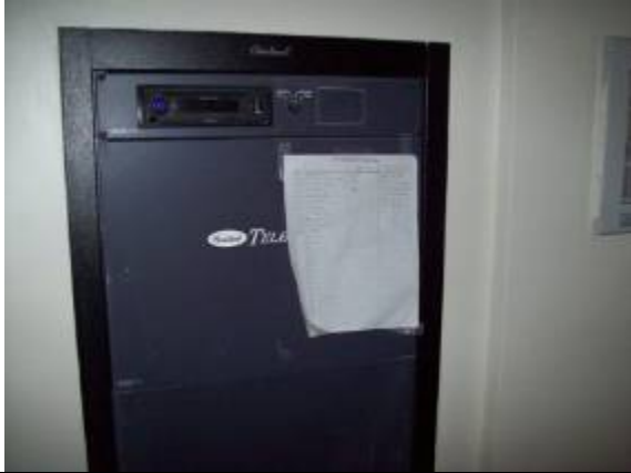
Photo #91: PA system control panel
