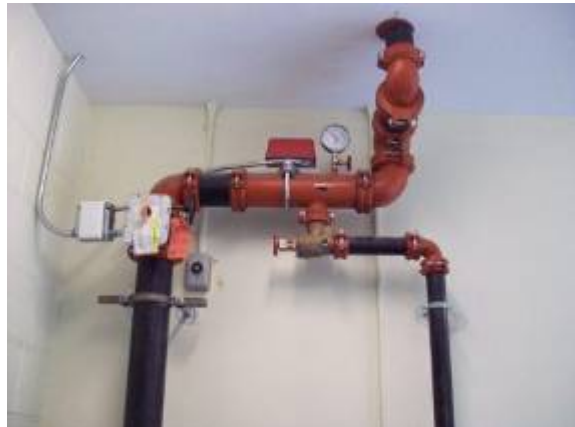
Photo #124: Fire sprinkler riser and test valves
