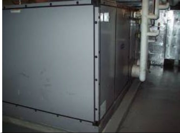
Photo #56: Air handling unit for Level F
