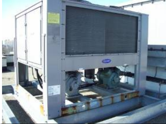
Photo #50: Condensing unit for auditorium
