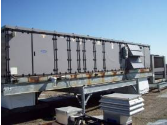
Photo #49: Air handling unit for auditorium
