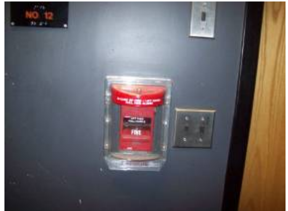
Photo #130: Fire alarm pull station
