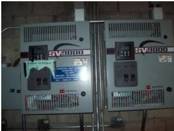
Photo #77: VFD controllers for air handling units
