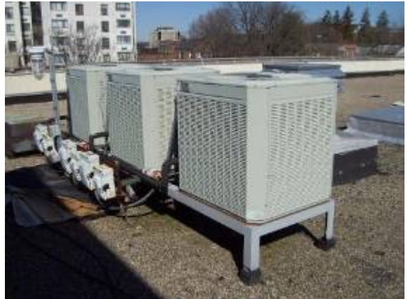
Photo #66: Typical roof-mounted condensing units
