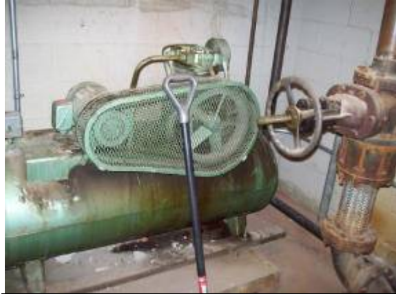
Photo #122: Air compressor for dry system section
