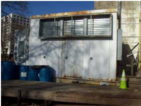
Photo #89: Generator enclosure
