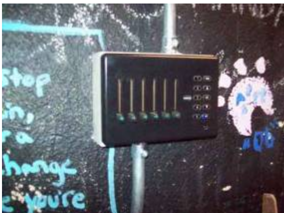
Photo #101: Stage lighting control
