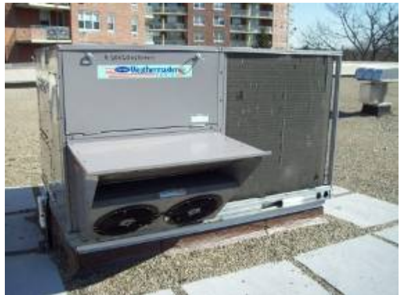
Photo #72: Rooftop unit for Administrative Offices
