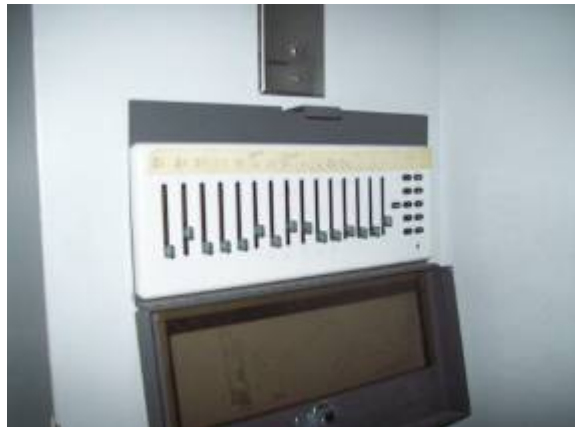
Photo #96: Advanced lighting control panel
