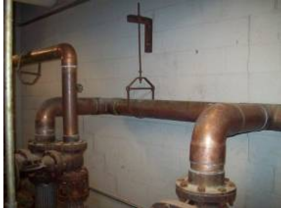
Photo #80: Domestic water distribution lines
