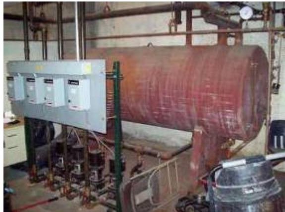
Photo #46: Condensate return system
