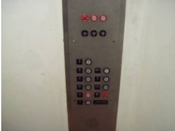
Photo #109: Elevator 2 control panel
