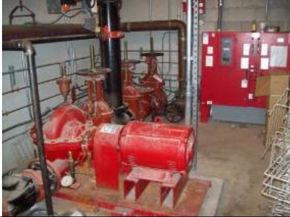
Photo #121: Fire pump and controller
