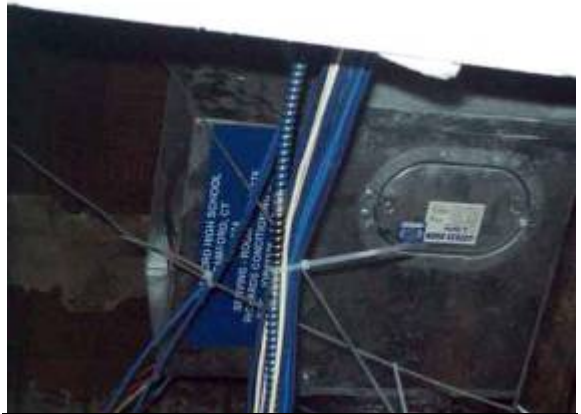
Photo #62: Typical VAV terminal
