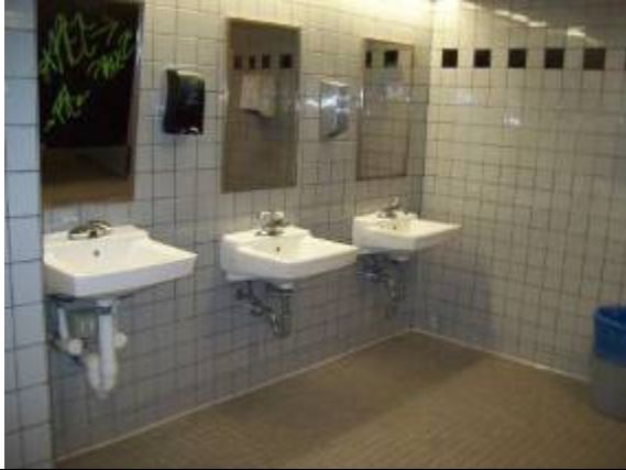
Photo #85: Restroom fixtures – lavatories
