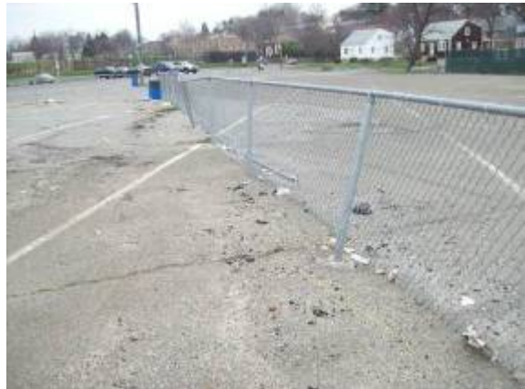
Photo #34: Damaged fencing in student parking lot
