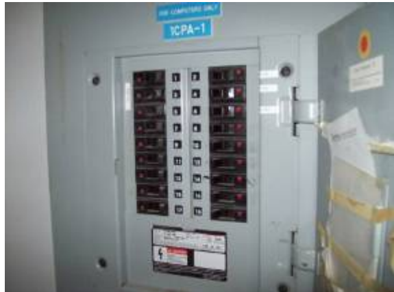
Photo #88: Typical breaker panel
