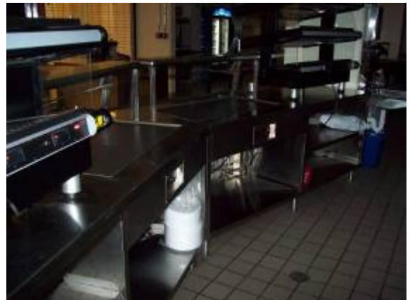
Photo #138: Kitchen equipment – Serving line
