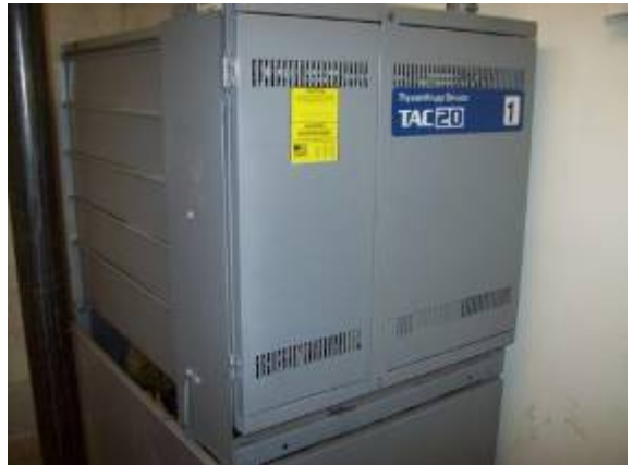
Photo #106: Elevator 1 hydraulic equipment
