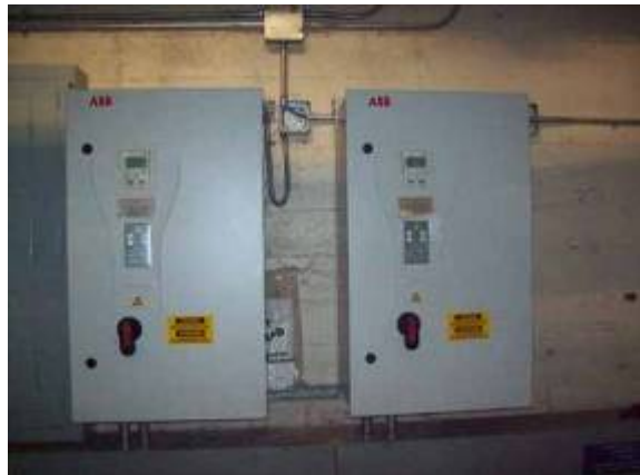
Photo #78: VFD controllers for circulating pumps
