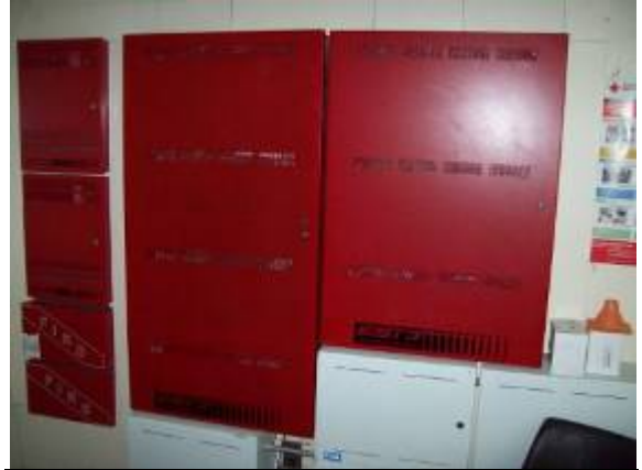
Photo #128: Fire alarm power and communicator panels
