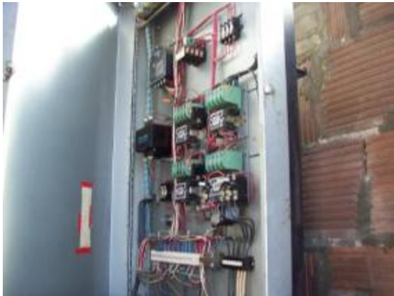
Photo #117: Elevator 4 control unit
