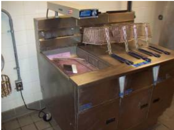
Photo #135: Kitchen equipment – Fryer
