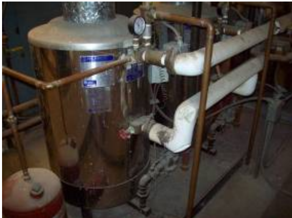
Photo #81: Domestic water boilers
