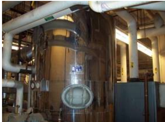
Photo #82: Domestic hot water storage tank
