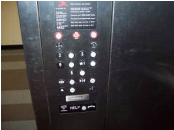
Photo #105: Elevator 1 control panel
