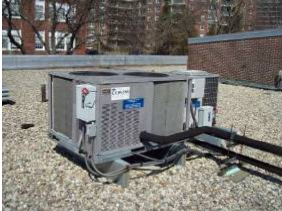
Photo #63: Typical roof-mounted condensing unit
