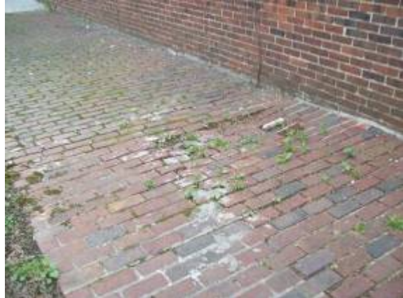
Photo #20: Damaged brick pavers
