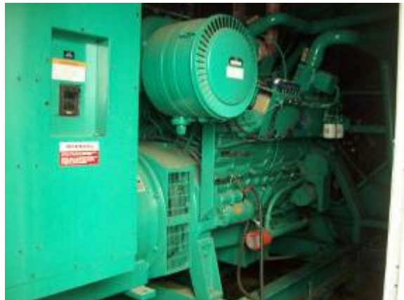
Photo #90: Emergency generator
