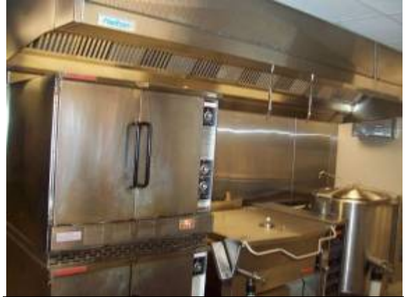
Photo #134: Kitchen equipment – Ovens and range
