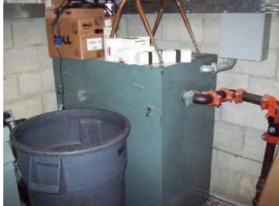
Photo #110: Elevator 2 hydraulic equipment
