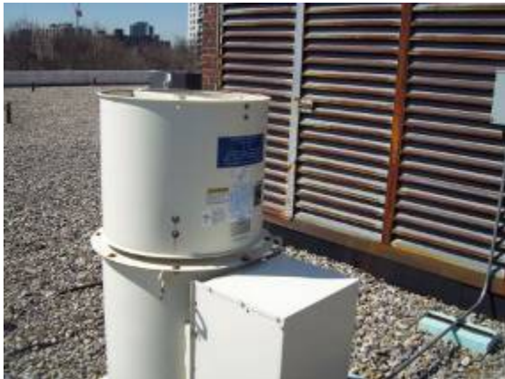
Photo #75: Typical roof-mounted exhaust fan
