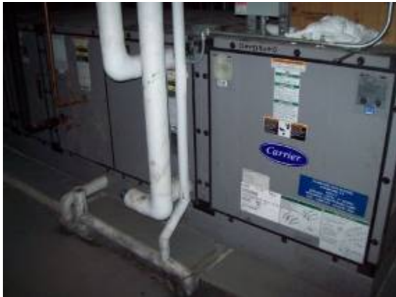
Photo #57: Air handling unit for Band Room
