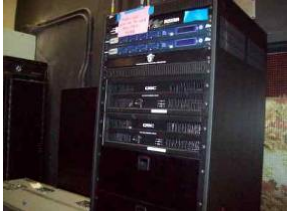
Photo #98: Auditorium sound system
