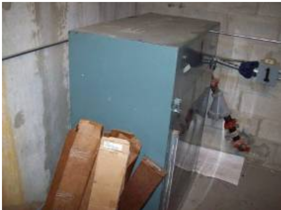
Photo #113: Elevator 3 hydraulic equipment
