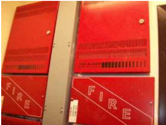
Photo #129: Fire alarm booster panels
