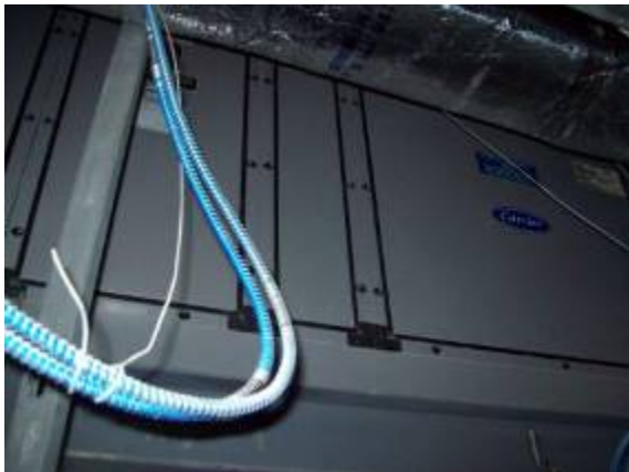
Photo #53: Air handling unit for cafeteria
