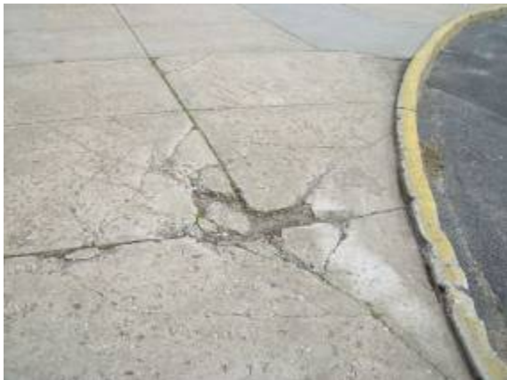
Photo #17: Sidewalk damage near gymnasium entrance
