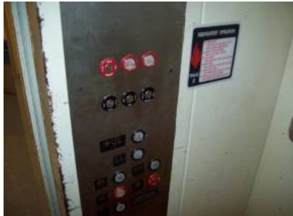
Photo #112: Elevator 3 control panel
