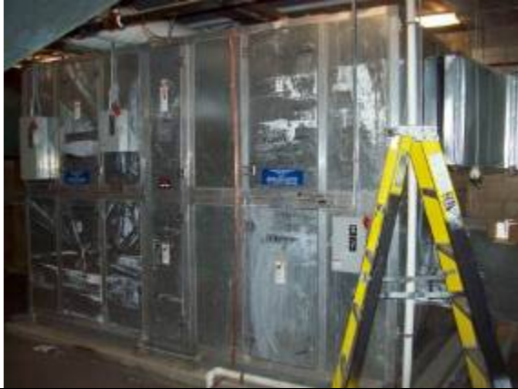
Photo #55: Air handling unit for Locker Rooms
