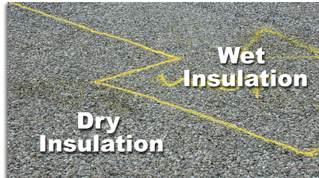
Control image, wet sections marked for removal
