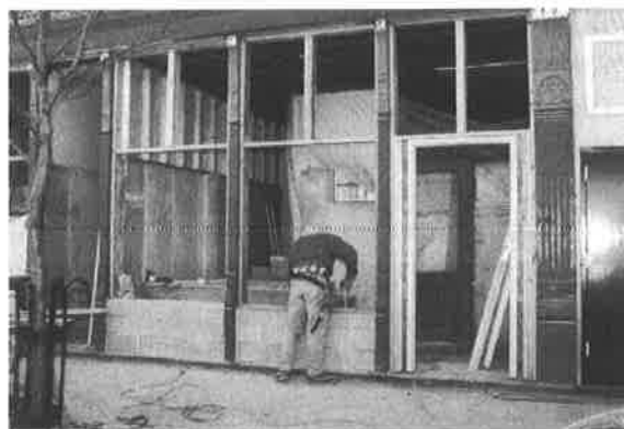
Floodproofing the vestibule of a storefront
