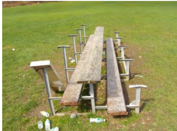
Photo #150: Bleacher at soccer field (damaged and missing seats)
