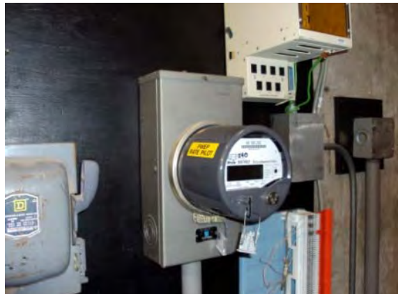
Photo #190: Electric meter at main electrical room
