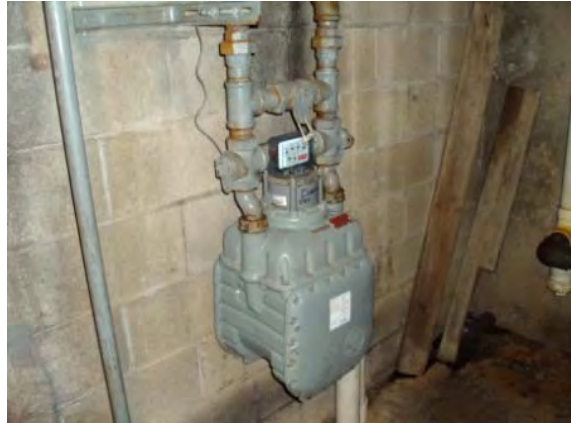
Photo #188: Gas metering at basement
