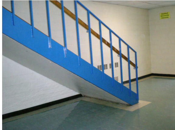
Photo #50: Non-compliant guardrail and handrail at stair
