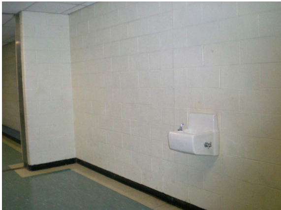
Photo #77: Projecting drinking fountain into path of travel. Also non-compliant due to twisting controls
