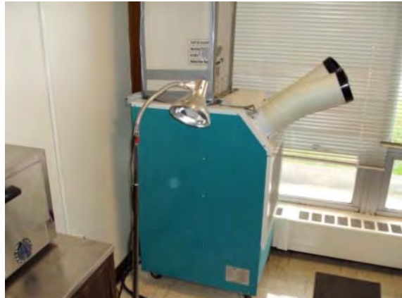
Photo #172: Portable AC unit at Nurses office
