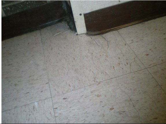
Photo #86: Heaving slab at connection to modular addition
