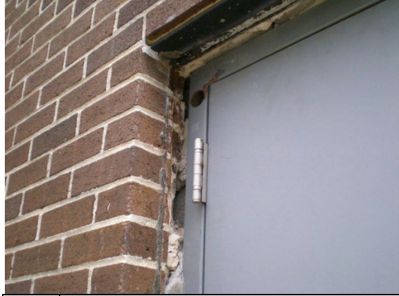
Photo #32: Exposed cavity at service door frame.
