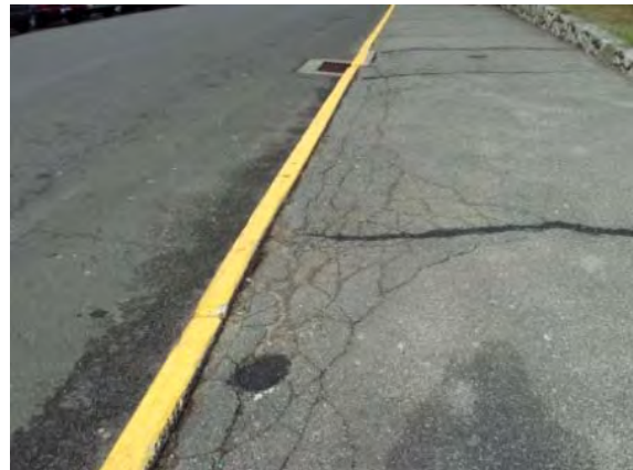
Photo #108: Asphalt deterioration and tripping hazard at the sidewalk
