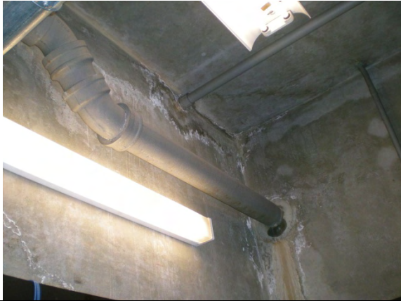
Photo #85: Moisture infiltration over main telephone equipment in basement
