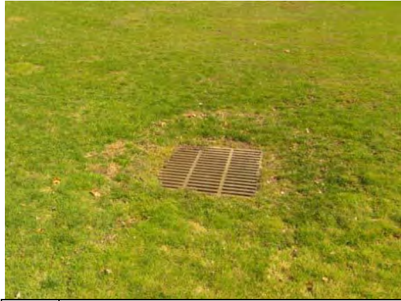
Photo #152: Landscape drainage inlet at play fields
