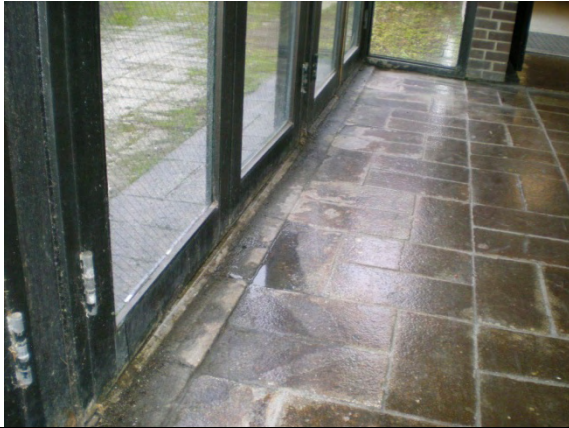
Photo #55: Water infiltration at north side entrance
