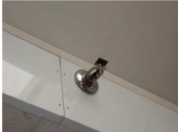
Photo #212: Sprinkler head
