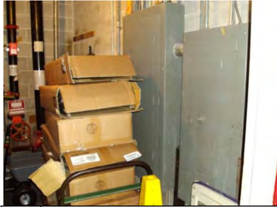
Photo #1340 : Blocked circuit breaker panels at fire suppression room
