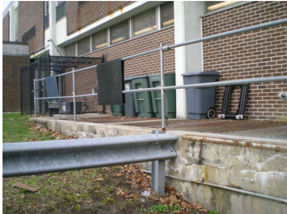
Photo #28: Spalled areas at loading dock
