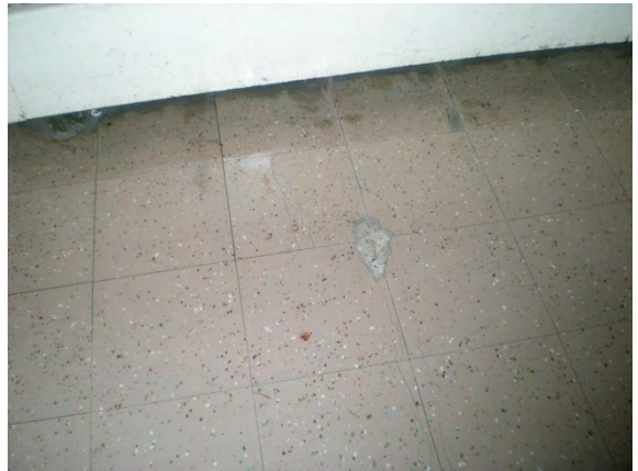
Photo #76: Suspect asbestos tile condition in classroom
