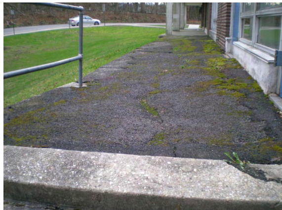
Photo #24: Asphalt overlay and open railing at sidewalk connection to fire exit balcony
