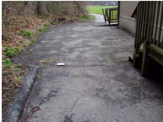
Photo #105: Asphalt condition at sidewalk adjacent to modular building
