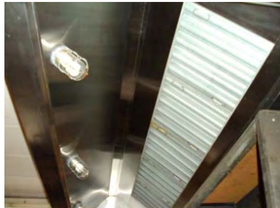
Photo #142: Exhaust hood without Ansul fire suppression
