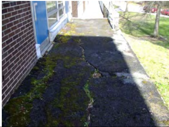
Photo #115: Deteriorated asphalt on top of concrete sidewalk at rear of building
