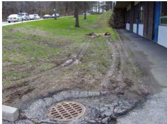
Photo #136: Barren landscaping and deterioration at drainage inlet - rear of building (northwest elevation)
