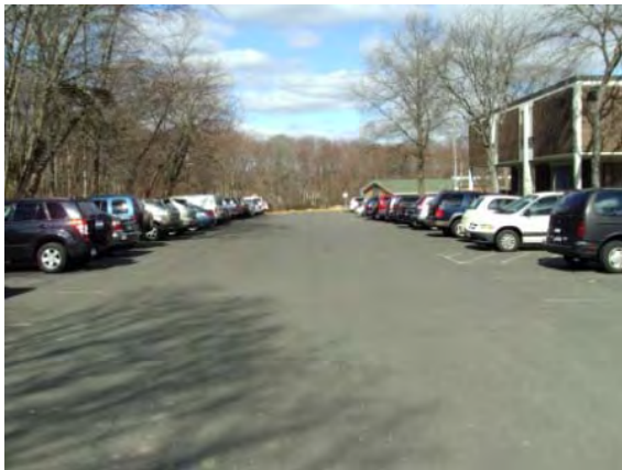
Photo #101: Worn pavement and striping at right side of building
