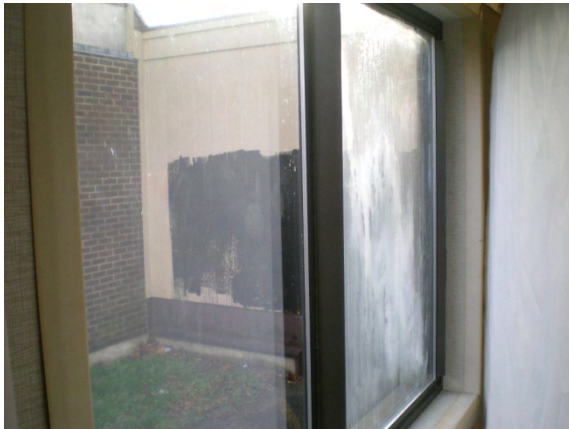
Photo #69: Broken seals at modular addition
