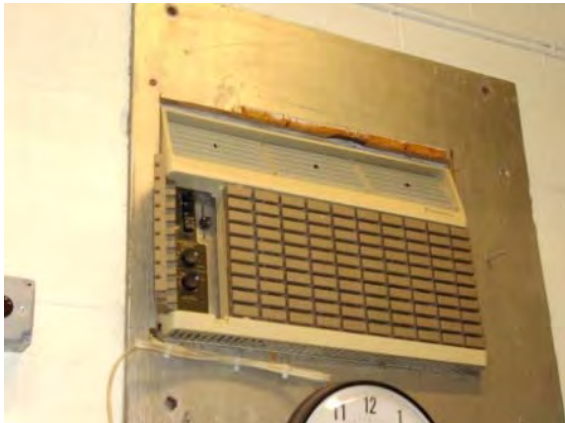
Photo #173: Through-wall AC unit at custodian office
