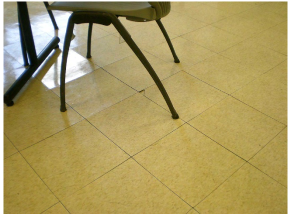
Photo #84: Moisture damaged flooring in lower level classroom
