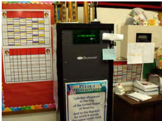
Photo #191: School PA system equipment at office
