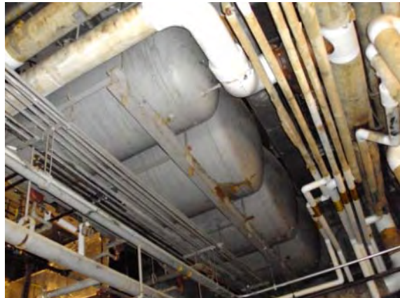
Photo #156: Boiler expansion tanks
