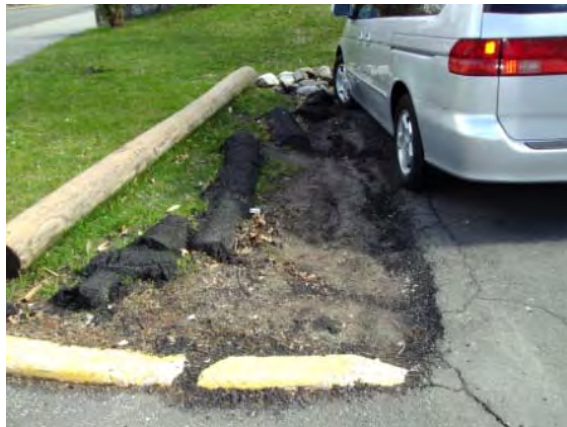
Photo #119: Displaced asphalt curbing at south parking lot
