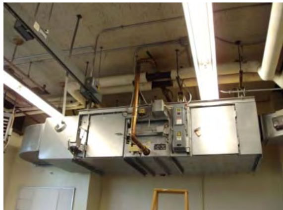
Photo #162: Air Handling Unit at classroom #82 (new unit)
