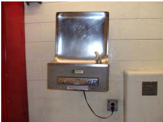
Photo #185: Common area drinking fountain at corridor missing GFCI outlet
