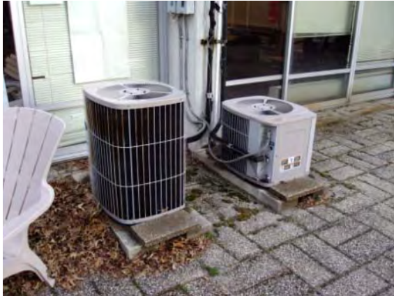
Photo #169: Pad-mount condensing units at courtyard
