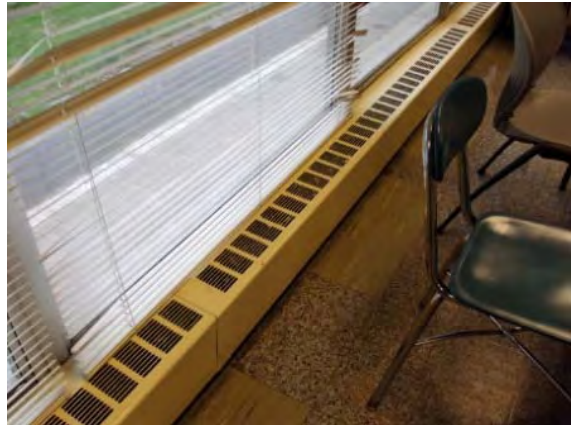
Photo #166: Perimeter baseboard radiant heat unit at classroom
