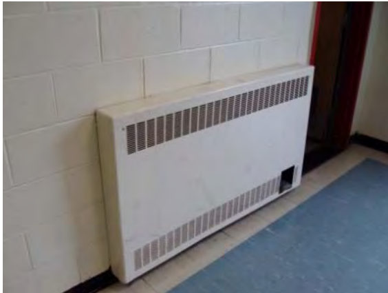
Photo #165: Wall-mounted cabinet radiant unit
