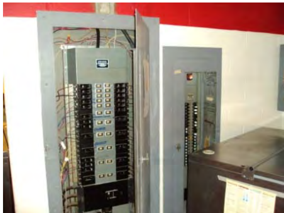
Photo #197: Original circuit breaker panels in kitchen
