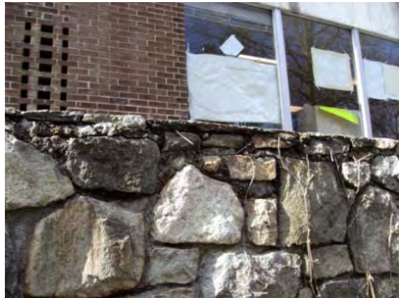
Photo #130: Deteriorated mortar at rear stone retaining wall
