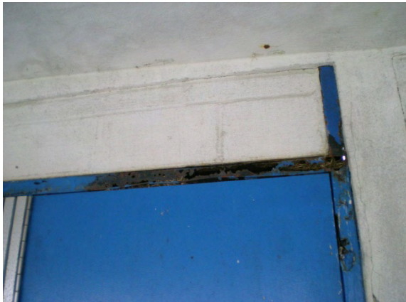
Photo #17: Rusted through door frame at west courtyard entrance
