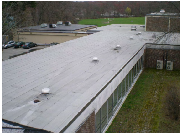
Photo #40: Roof overview of modular addition and partial roof around east courtyard
