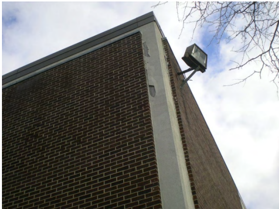
Photo #35: Condition of paint at concrete structural covering
