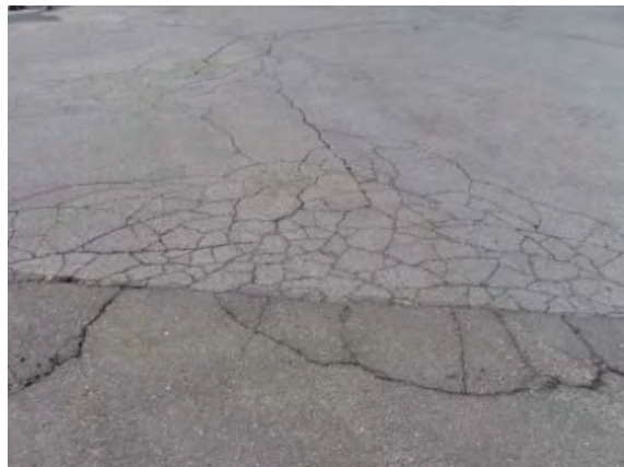
Photo #100: Alligator cracking at asphalt pavement rear of building
