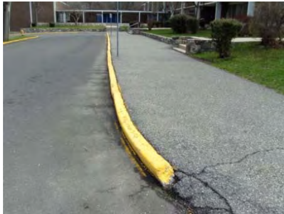
Photo #117: Shifting concrete curbing along front sidewalk
