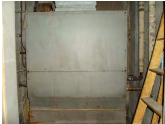
Photo #159: Air Handling Unit (AHU) at basement
