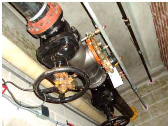
Photo #138: BFP for fire sprinkler system
