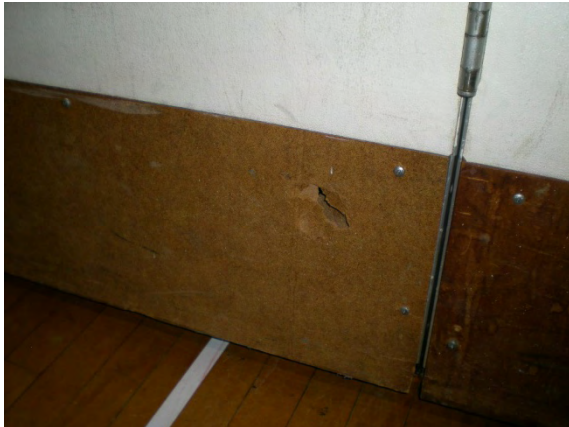
Photo #63: Condition of masonite at base of folding divider wall
