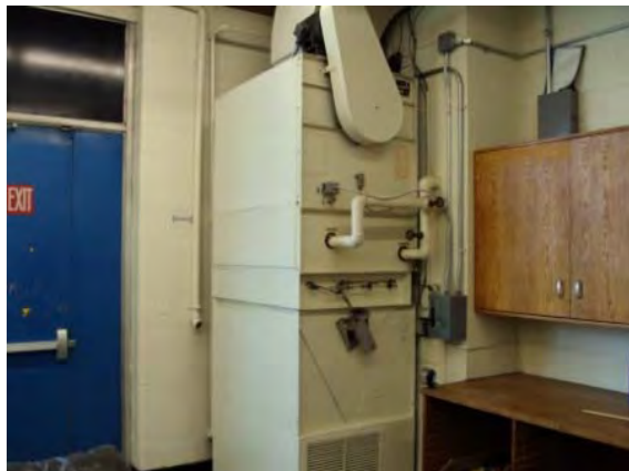
Photo #161: Air Handling Unit at classroom #80
