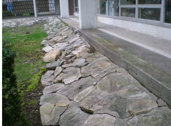
Photo #14: Loose stones with deteriorated mortar along front and side entrances
