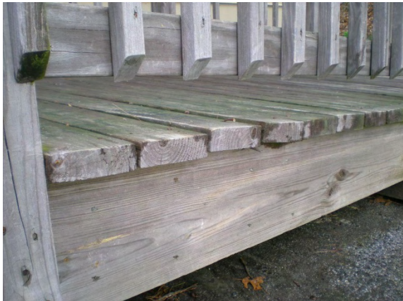
Photo #29: Warping floor boards at access ramp to modular addition
