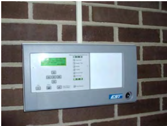
Photo #141: Annunciator panel at entry vestibule
