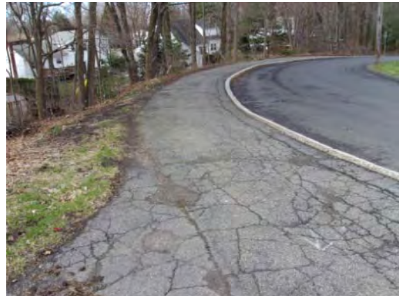
Photo #104: Asphalt condition at sidewalk leading to adjacent neighborhood (south elevation)
