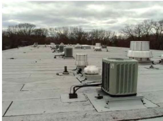
Photo #168: Rooftop condensing units and exhaust fans
