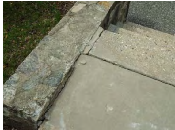
Photo #122: Deterioration at concrete steps at front elevation
