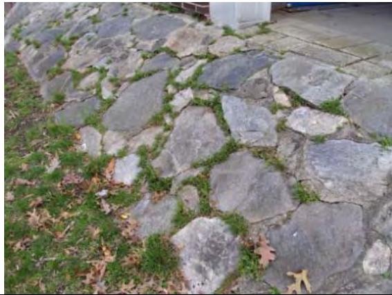
Photo #127: Vegetation growth at sloped stone masonry retaining wall (side elevation)
