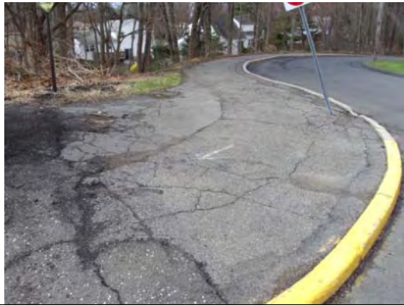
Photo #109: Asphalt deterioration at sidewalk leading to adjacent neighborhood (south elevation)
