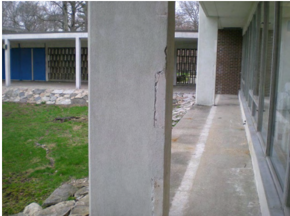
Photo #15: Damaged column from former concrete block wall attachment
