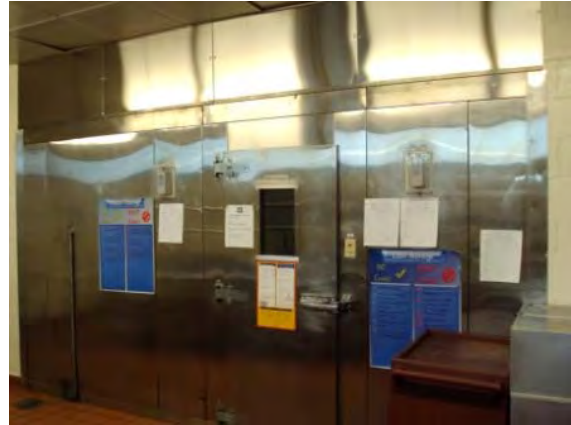
Photo #218: Walk-in refrigerator/freezer
