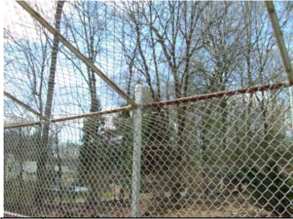
Photo #146: Loose fencing at backstop
