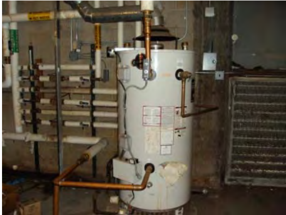
Photo #175: Domestic water heater at basement mechanical room
