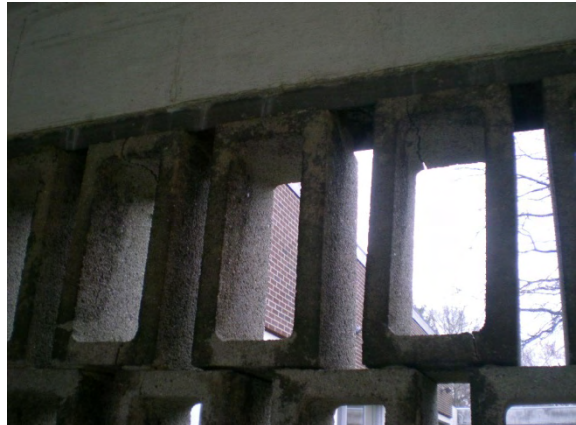
Photo #16: Damaged concrete screen wall at west courtyard
