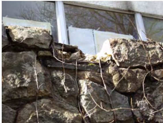
Photo #129: Deterioration at rear stone retaining wall
