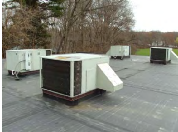
Photo #154: Rooftop package units for the modular classrooms
