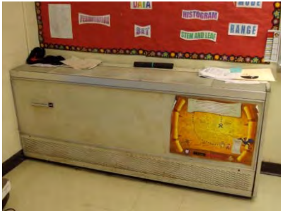
Photo #167: Original unit ventilator at classroom
