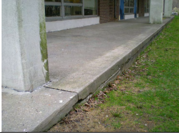
Photo #26: Damaged concrete slab at north elevation
