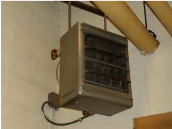
Photo #171: Unit heater at custodian office
