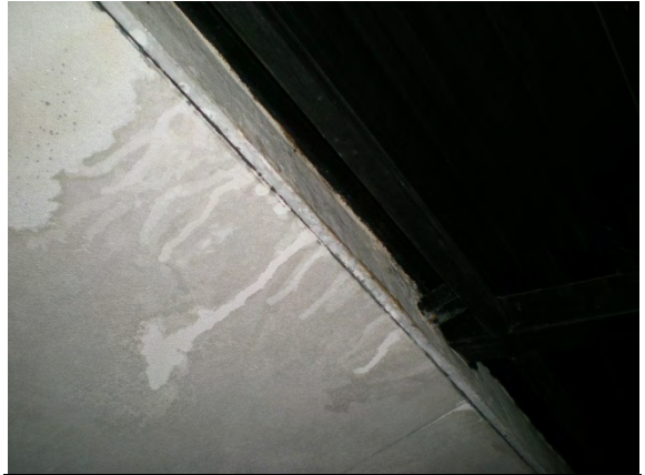
Photo #56: Evidence of water infiltration at ceiling of north side entrance
