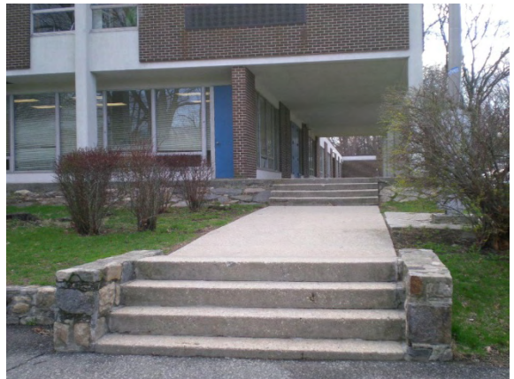
Photo #10: Exterior stairs with no railings and partial south elevation
