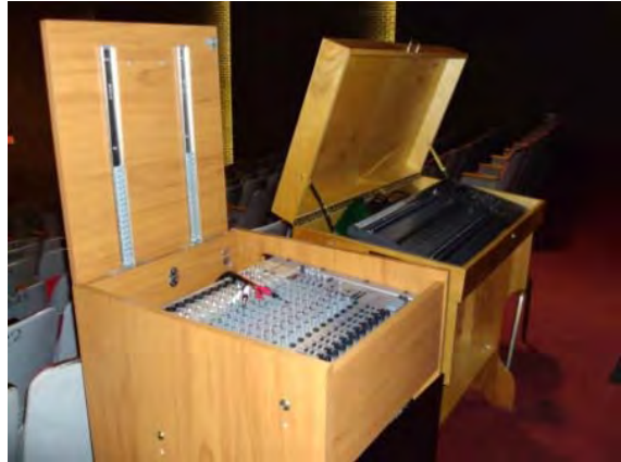
Photo #194: Auditorium audio controls
