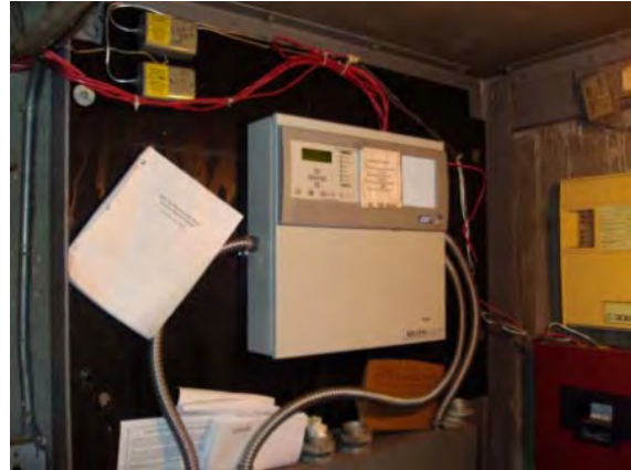
Photo #140: Central fire alarm panel at basement mechanical room
