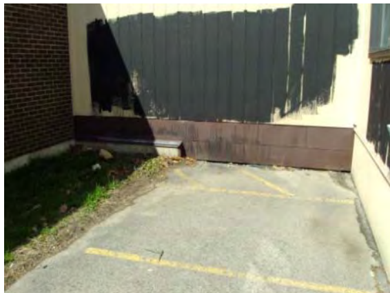
Photo #123: Inadequate drainage at rear of modular building (east elevation)
