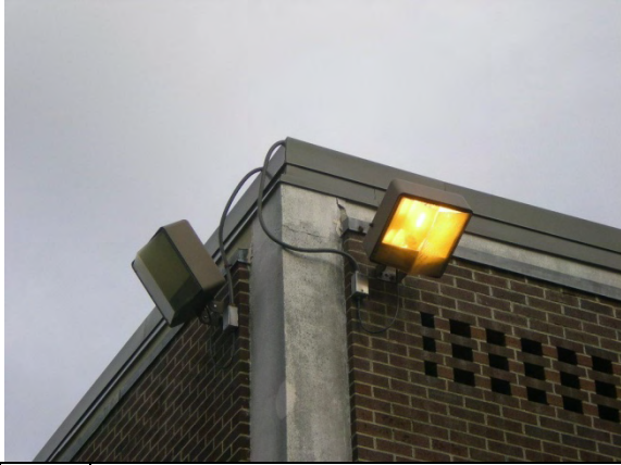
Photo #31: Cracked column cover at top of building
