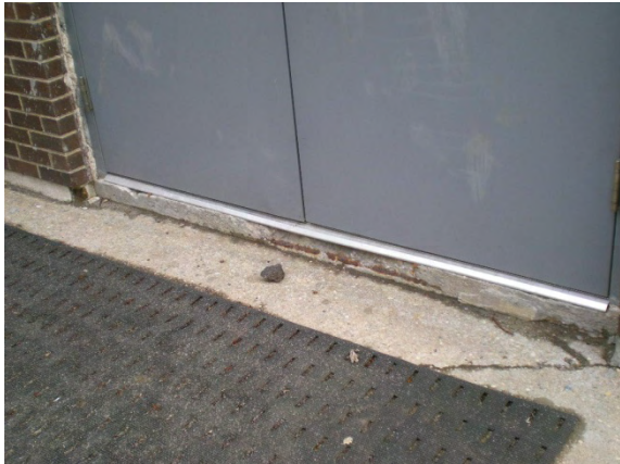
Photo #33: Corroded and spalled concrete door sill at service door with exposed rebar
