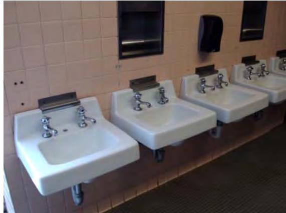
Photo #182: Girls common area restroom lavatory sinks with wall-bracket for added support
