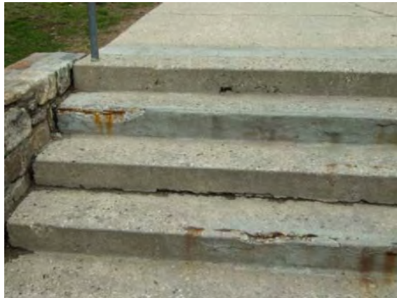
Photo #121: Deterioration at concrete steps at side elevation
