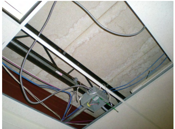
Photo #58: Exposed structure within classroom showing water stains
