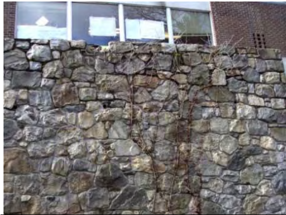
Photo #128: Deteriorated mortar and vine growth at rear stone retaining wall
