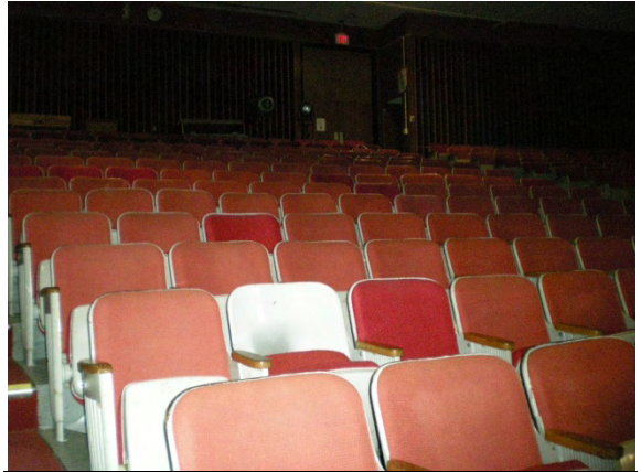
Photo #80: Condition of auditorium seating
