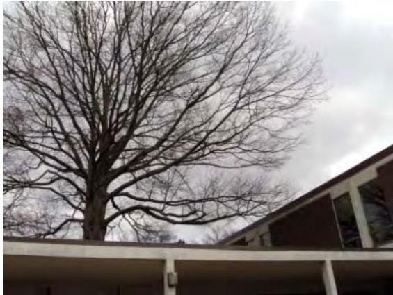
Photo #133: Tree overhanging roof surface at courtyard
