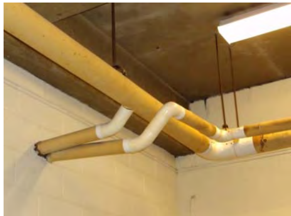
Photo #186: Suspect ACM at pipe covering at custodian office
