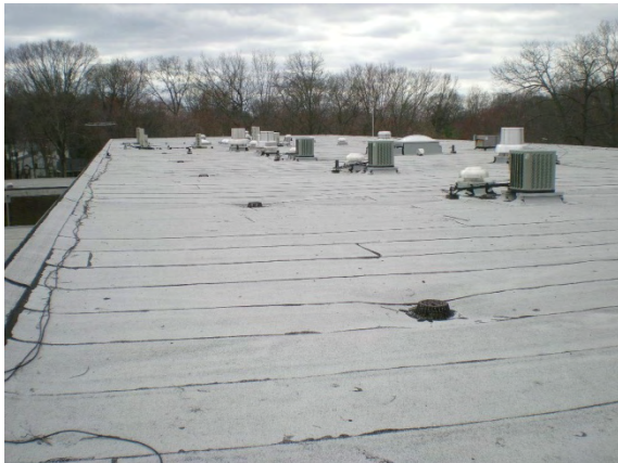
Photo #41: Roof overview of central building spine including main office and cafeteria
