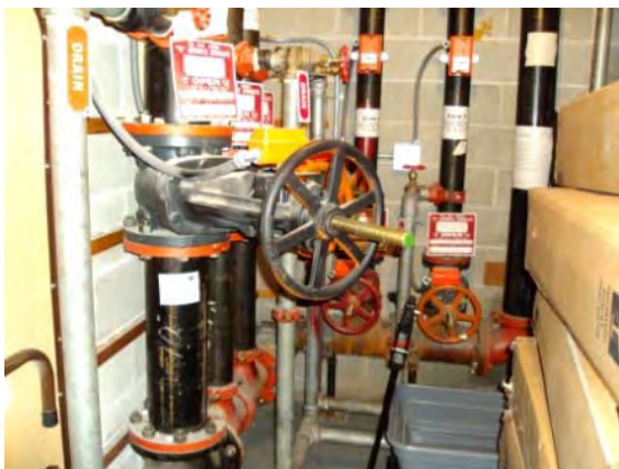
Photo #137: Fire suppression risers
