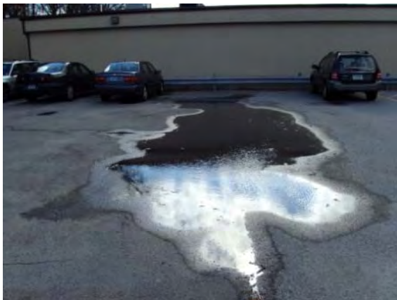
Photo #99: Ponding at asphalt pavement at rear parking lot
