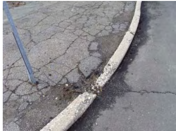
Photo #118: Deteriorated concrete curb at south elevation
