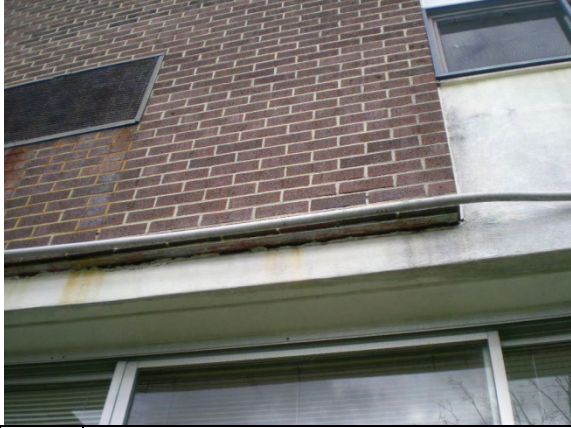
Photo #25: Rusting fan coil grille and rusting and deteriorating brick angle
