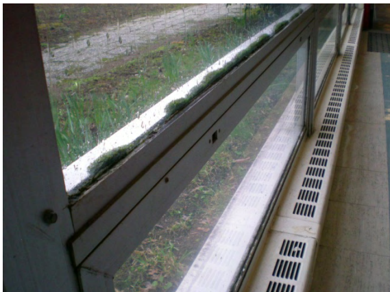
Photo #53: Condition of windows – showing moss growth
