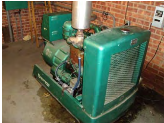
Photo #195: Emergency generator in basement
