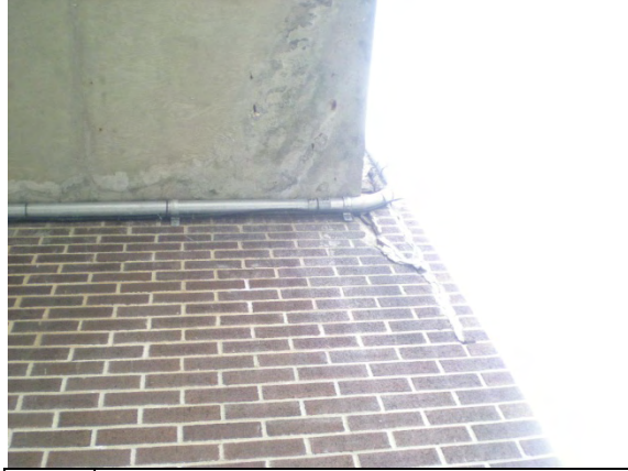
Photo #20: Spalling brick veneer under cantilevered fire exit balcony at north elevation
