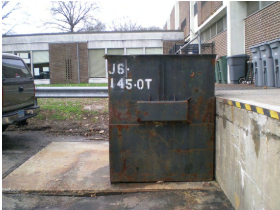
Photo #27: Loading dock area with no bumpers at dumpster and damaged concrete dock
