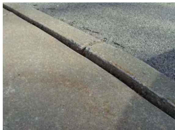
Photo #114: Tripping hazard at concrete sidewalk adjacent to rear drive lane
