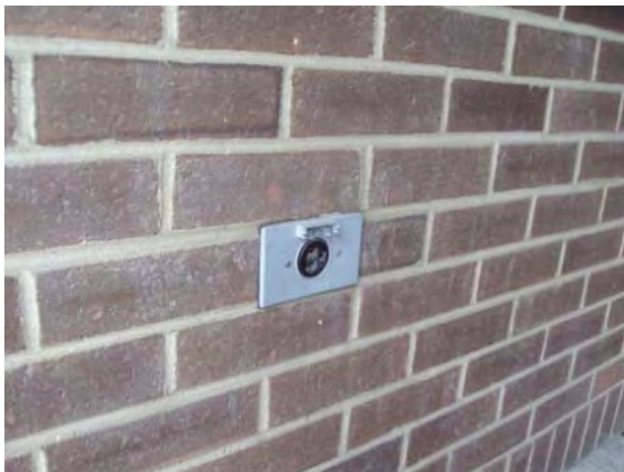
Photo #135: Exterior outlet missing GFCI and cover at main entrance
