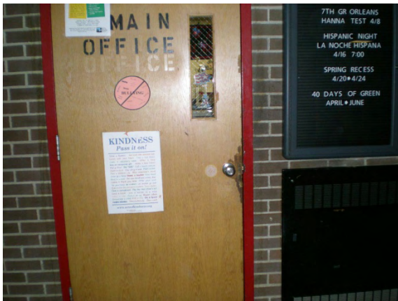
Photo #47: Main office entrance with knob handle hardware and damaged door
