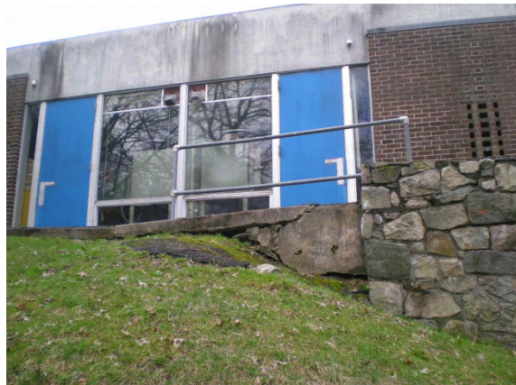
Photo #22: Damaged concrete sidewalk at connection to fire exit balcony
