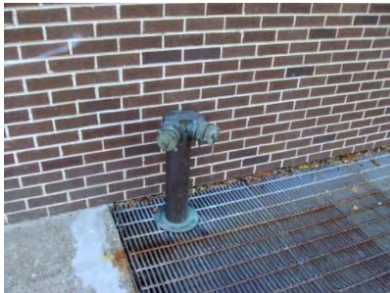
Photo #213: Siamese connection at rear of building
