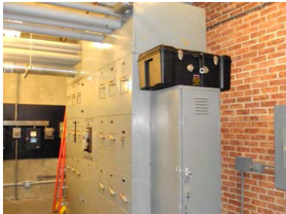
Photo #189: Main electrical switchgear in basement of building
