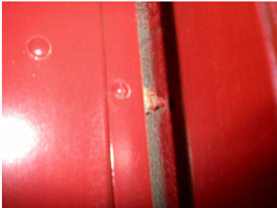
Photo #59: Loose bank of lockers – not securely attached into wall
