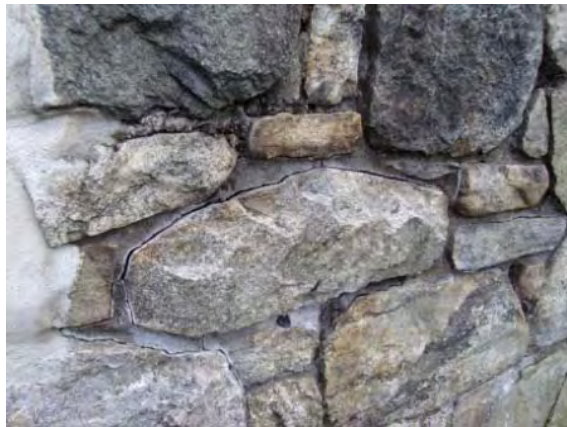
Photo #131: Cracking mortar at stone retaining wall at left side of building
