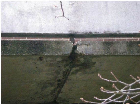
Photo #21: Corroded concrete and rusted through steel support at cantilevered balcony
