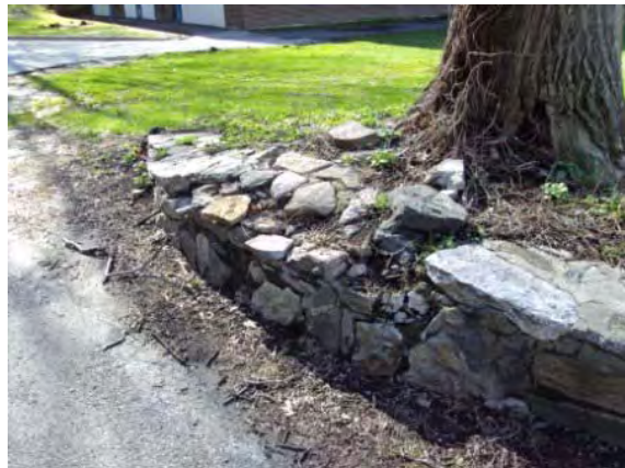
Photo #132: Deterioration at stone retaining wall along rear drive lane
