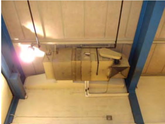
Photo #163: Air Handling Unit at gymnasium
