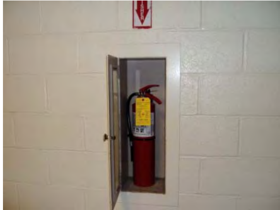
Photo #211: Cabinet-mount fire extinguisher
