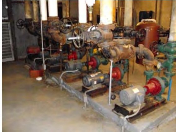
Photo #157: Hot water circulating pumps
