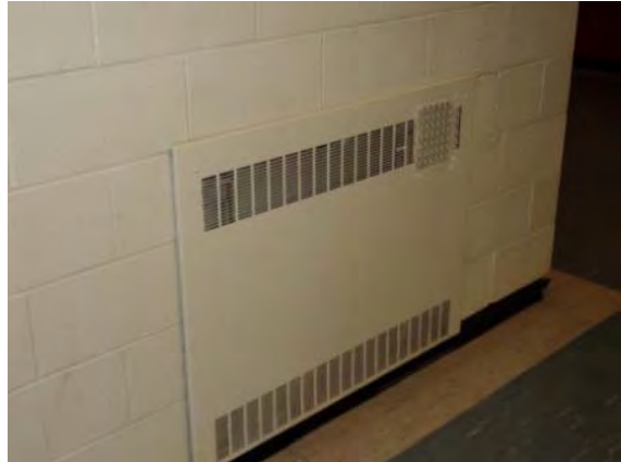
Photo #164: Recessed cabinet radiant unit
