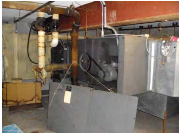
Photo #160: Air Handling Unit at loft above classroom #82
