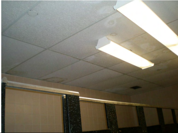
Photo #73: Water stains in student restroom
