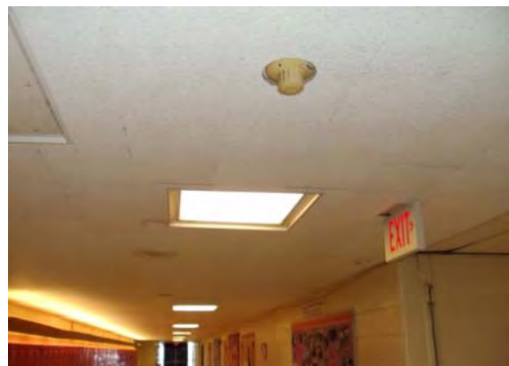
Photo #210: Smoke detector and illuminated exit sign
