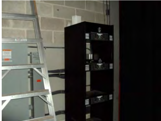
Photo #193: Auditorium lighting controls
