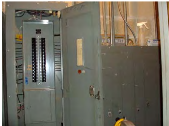
Photo #198: Original circuit breaker panels in electrical closet
