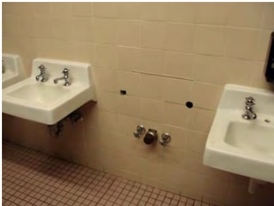
Photo #183: Girls common area restroom missing a lavatory sink
