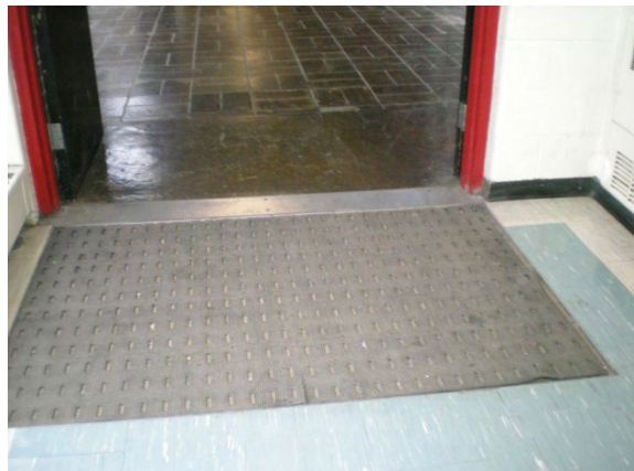
Photo #54: Curled recessed walk-off mat at north side entrance creating trip hazard
