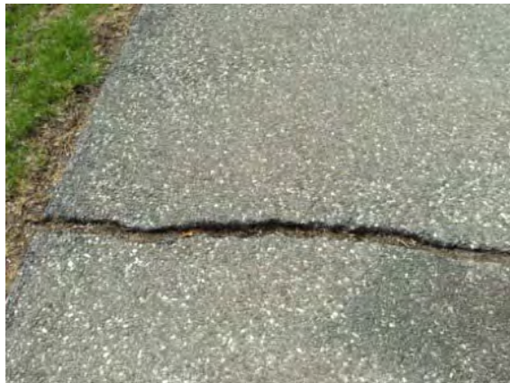
Photo #107: Settlement and cracking at asphalt sidewalk at left side of building
