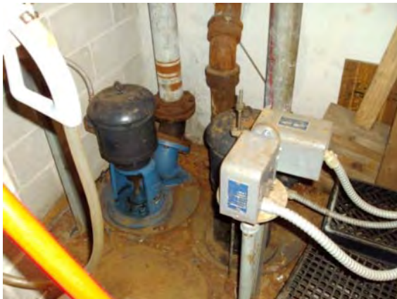
Photo #177: Dual sewage pump system at lower level
