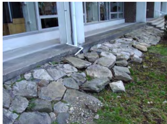
Photo #126: Loose stones and deteriorated mortar at sloped stone retaining wall (front elevation)
