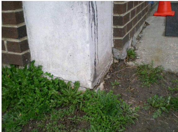
Photo #30: Cracked column base cover and foundation
