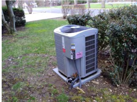
Photo #170: Pad-mount condensing unit at front of school
