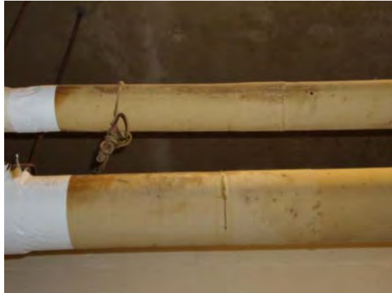
Photo #187: Damaged suspect ACM at pipe covering at custodian office
