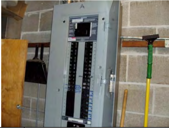
Photo #1339 : Replacement circuit breaker panel
