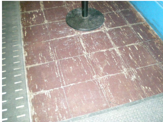
Photo #46: Condition of suspect asbestos tile flooring at main lobby
