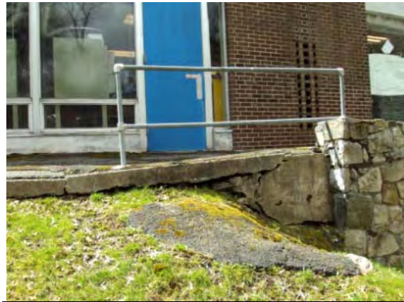
Photo #116: Collapsing concrete sidewalk at rear of building (adjacent to retaining wall)
