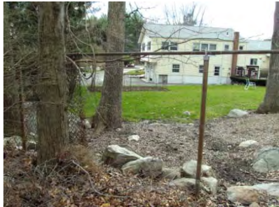
Photo #142: Damaged chain link fencing along perimeter at southeast elevation
