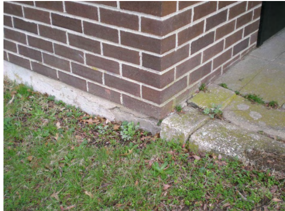
Photo #34: Damaged foundation at southwest corner
