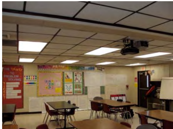
Photo #214: Modular classroom with sprinkler heads
