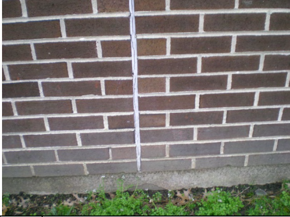
Photo #19: Deteriorated expansion joint
