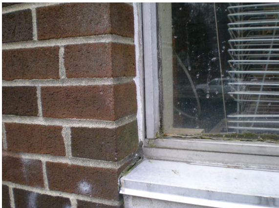
Photo #23: Deteriorated sealant
