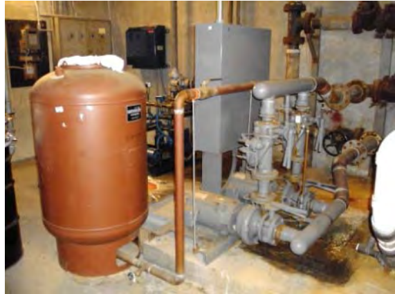
Photo #176: Domestic water booster system at basement mechanical room
