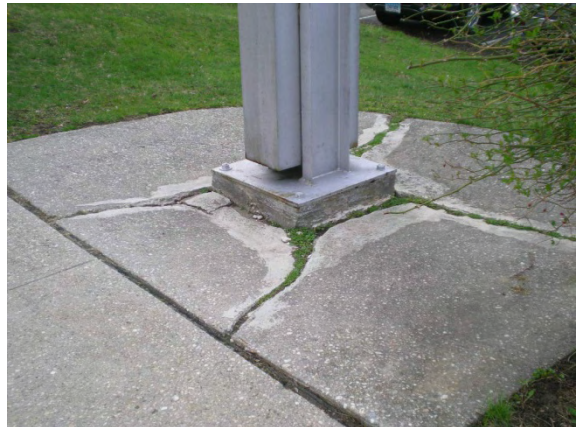
Photo #36: Condition of base at flag pole
