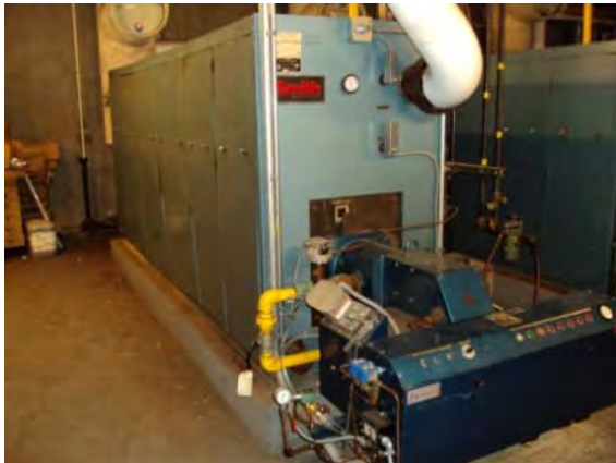
Photo #155: Hot water heating boilers (1 of 3) at basement mechanical room
