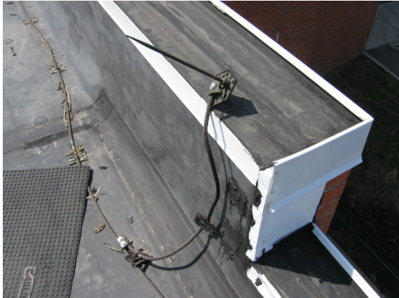
Photo #21: Several lightning arrestor spikes have delaminated from the roof
