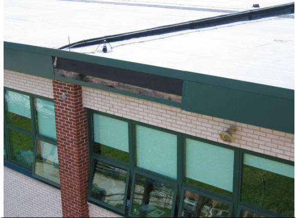
Photo #14: One section of roof edge fascia is missing, minor repairs are needed
