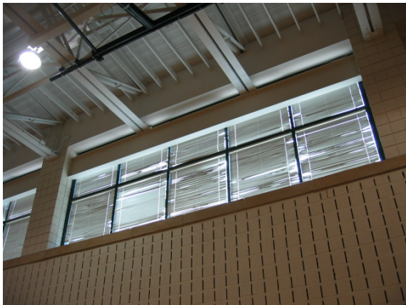
Photo #35: Detail of the damaged gymnasium window blinds
