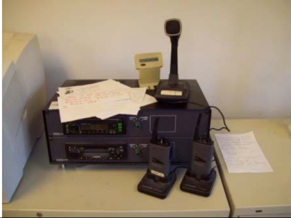
Photo #109: PA system in main office
