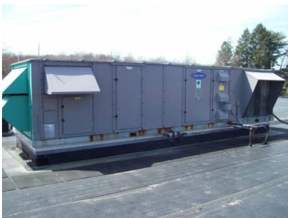
Photo #77: Rooftop Unit 3A
