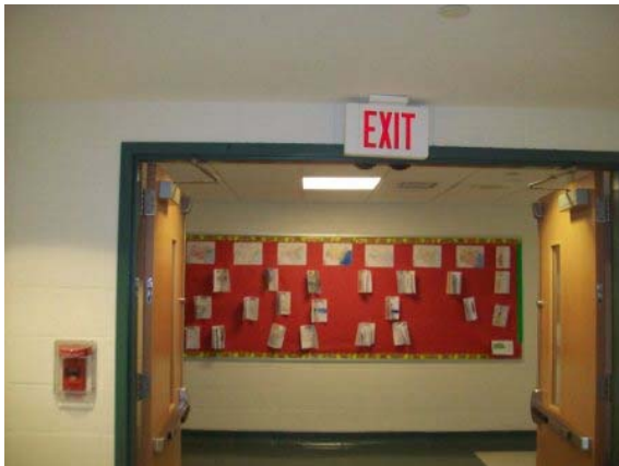
Photo #125: Emergency exit sign and pull station
