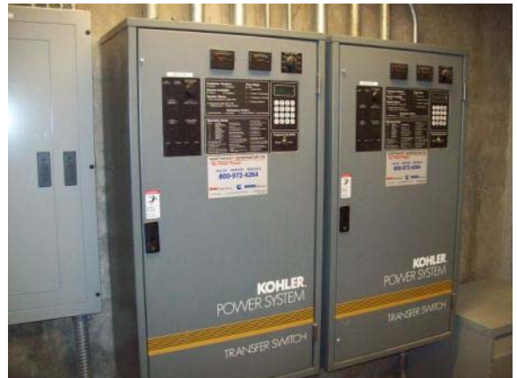
Photo #108: Transfer switches
