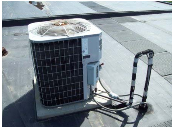
Photo #88: Condensing unit for AC-9
