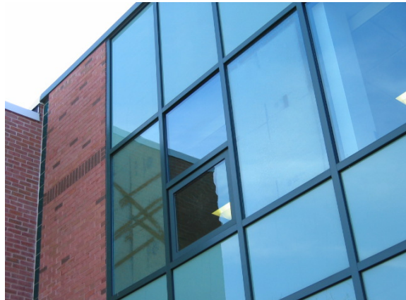
Photo #10: Two 2 nd floor windows were observed to be shattered
