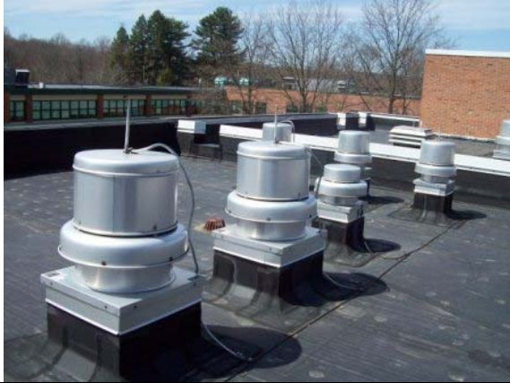
Photo #91: Roof-mounted exhaust fans
