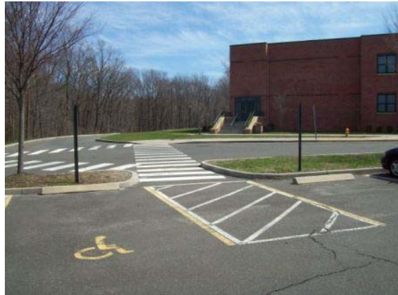
Photo #132: Accessible parking stalls with missing signage
