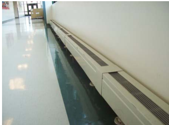
Photo #72: Baseboard-mounted finned tube radiant heat unit
