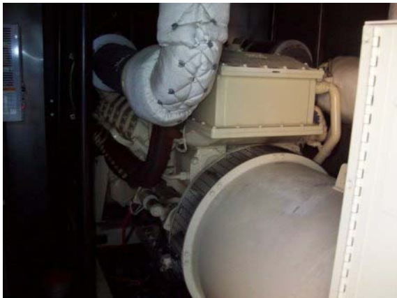
Photo #107: Emergency generator
