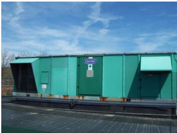
Photo #75: Rooftop Unit 2A
