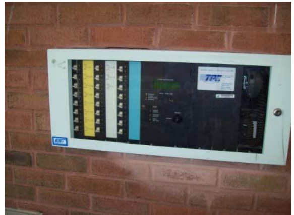
Photo #124: Fire alarm annunciator panel
