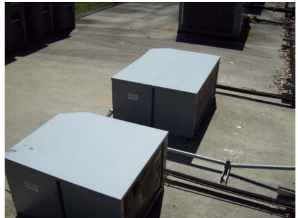
Photo #156: Compressors for walk-in units
