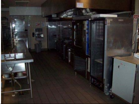
Photo #151: Commercial kitchen
