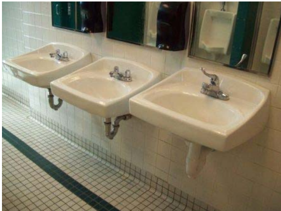
Photo #99: Typical restroom fixtures
