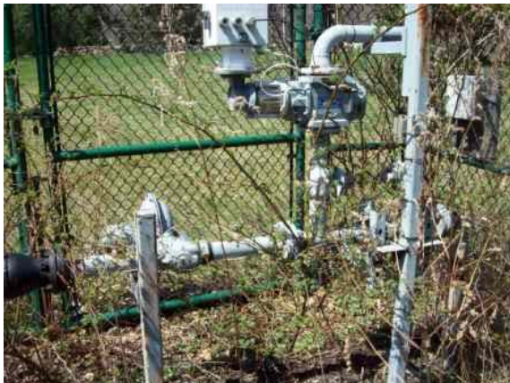
Photo #101: Gas meter and regulator
