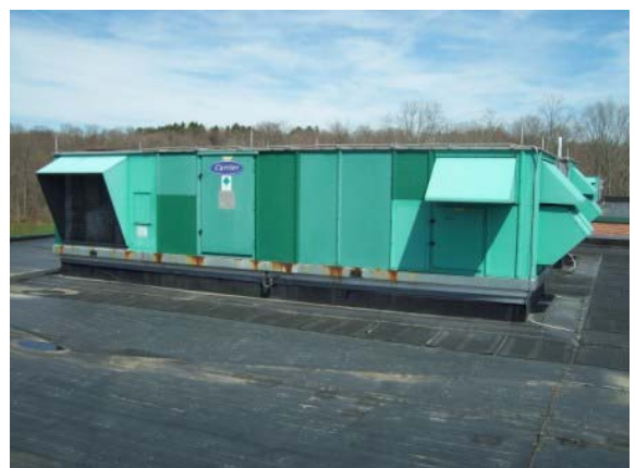
Photo #78: Rooftop Unit 3B
