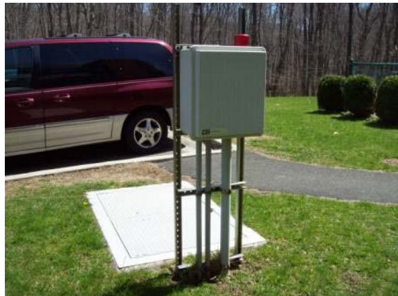
Photo #96: Lift station at east side of property
