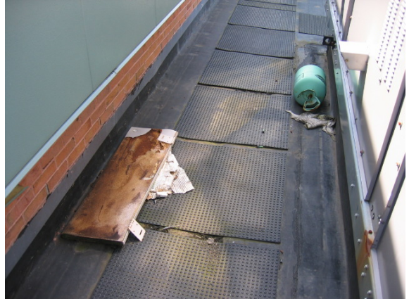
Photo #20: Isolated sections of roof debris were noted
