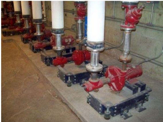
Photo #69: Hot water circulating pumps
