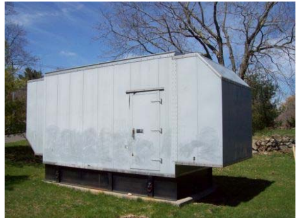
Photo #106: Emergency generator enclosure
