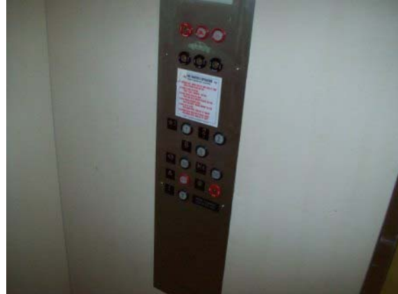
Photo #116: Cafeteria elevator control panel
