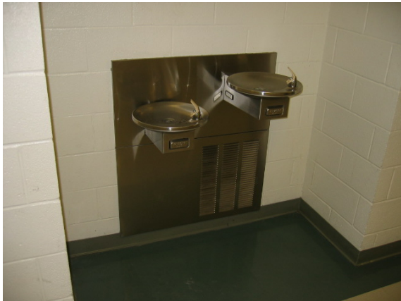
Photo #27: Handicapped-accessible water fountains are found throughout the corridors
