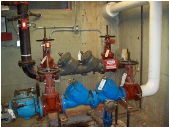
Photo #93: Domestic water service
