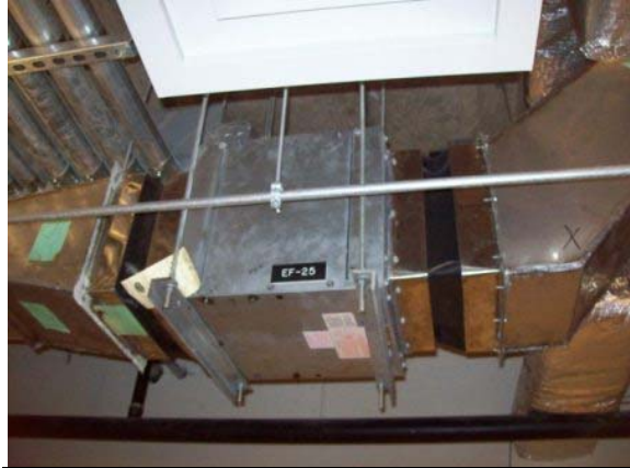
Photo #92: Ceiling-mounted exhaust fan
