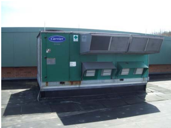
Photo #83: Rooftop Unit 6
