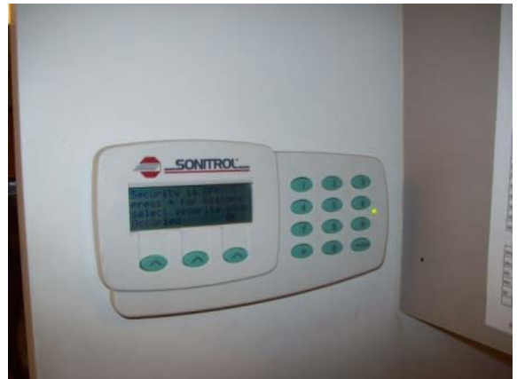
Photo #126: Security interface panel
