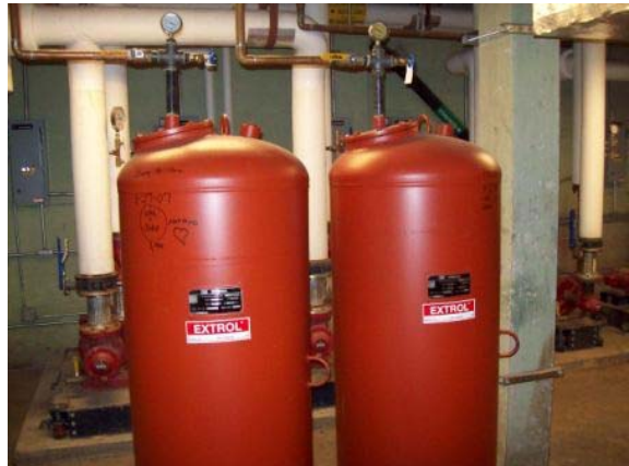
Photo #70: Expansion tanks
