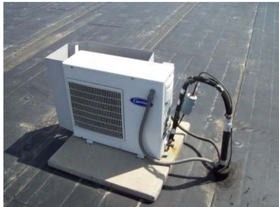
Photo #90: Condensing unit for wall-mounted AC
