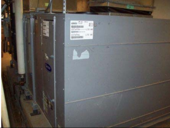
Photo #85: AC-7 serving cafeteria
