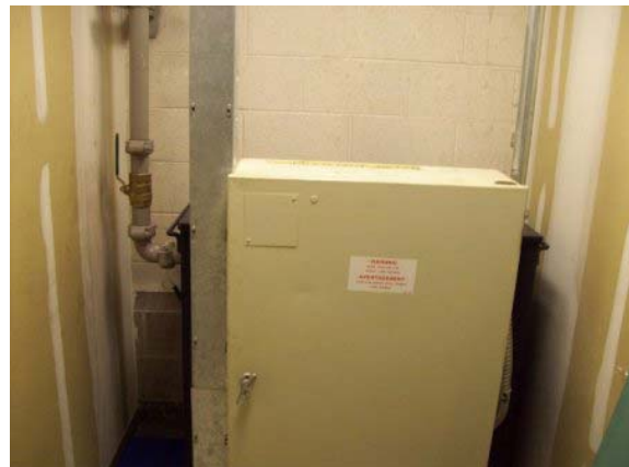
Photo #118: Bus entrance elevator hydraulic equipment
