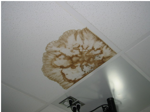
Photo #57: A few isolated stained acoustic ceiling tiles were noted
