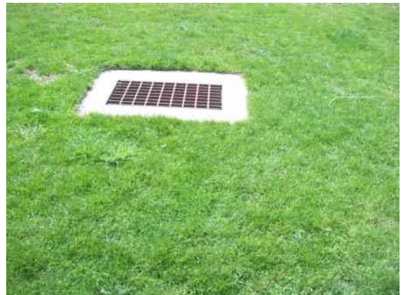
Photo #138: Typical catch basin
