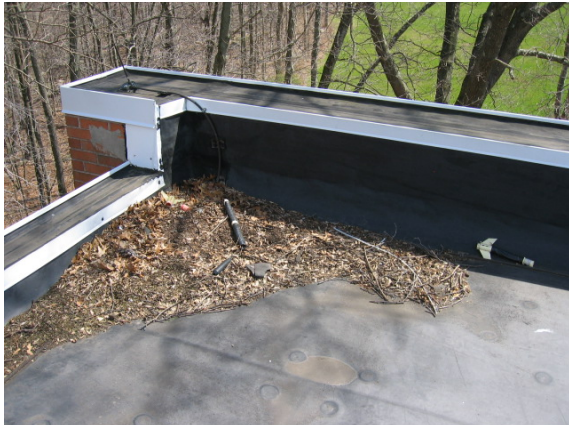
Photo #23: Fallen organic matter exists in some roof corners
