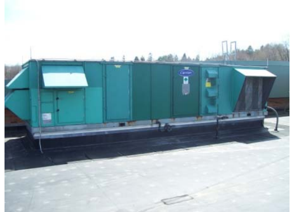
Photo #74: Rooftop Unit 1B
