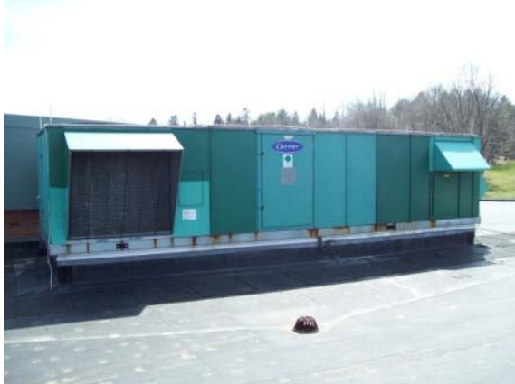
Photo #73: Rooftop Unit 1A
