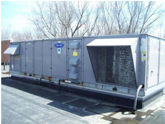
Photo #81: Rooftop Unit 5A
