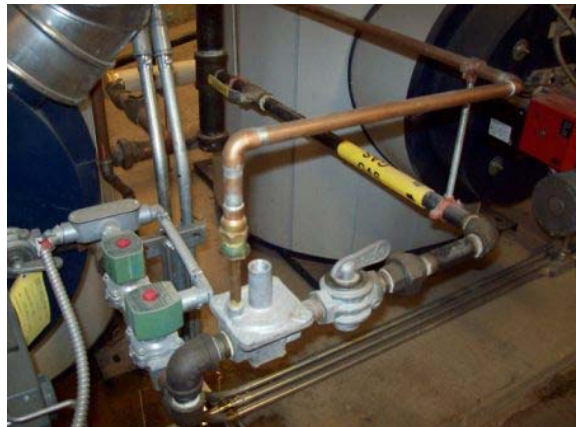
Photo #102: Gas feed for domestic water boiler
