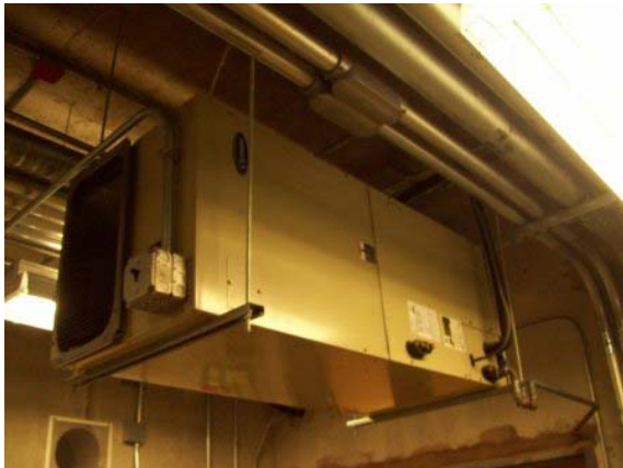
Photo #87: AC-9 serving electrical room
