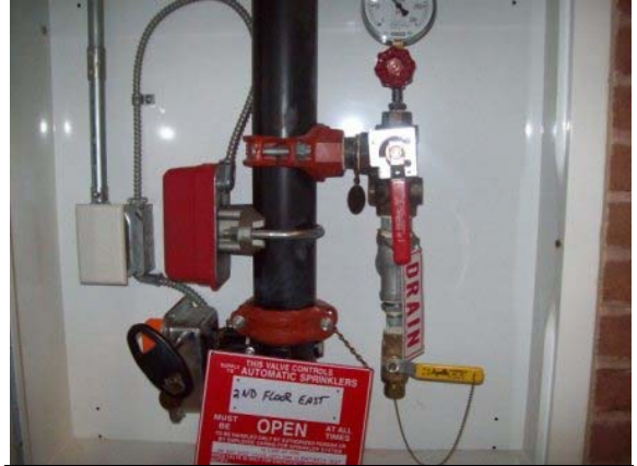
Photo #122: Sprinkler stand pipe and test valves
