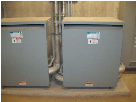
Photo #105: Step down transformers
