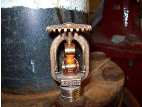
Photo #121: Typical sprinkler head
