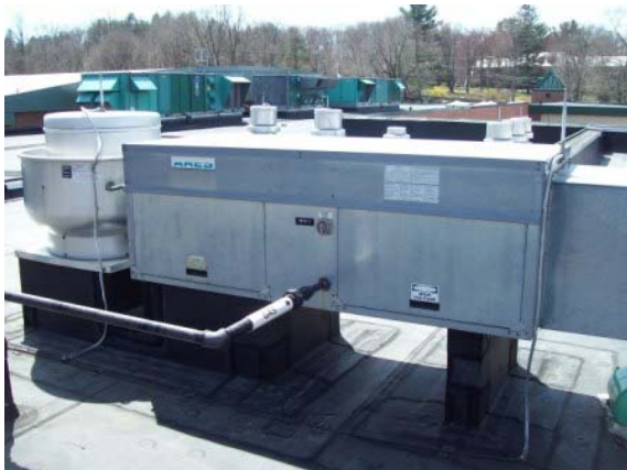
Photo #89: Make-up air unit for kitchen
