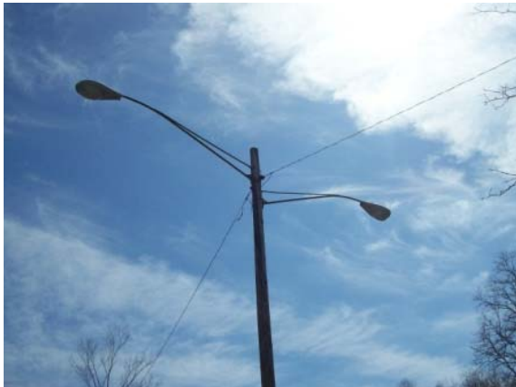
Photo #141: Typical site light standard
