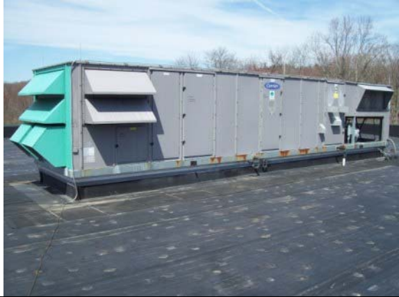
Photo #80: Rooftop Unit 4B
