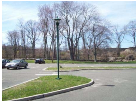
Photo #142: Pole mounted site lighting
