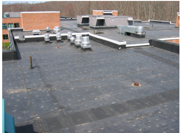
Photo #16: Most areas of the school are covered with a fully adhered EPDM
