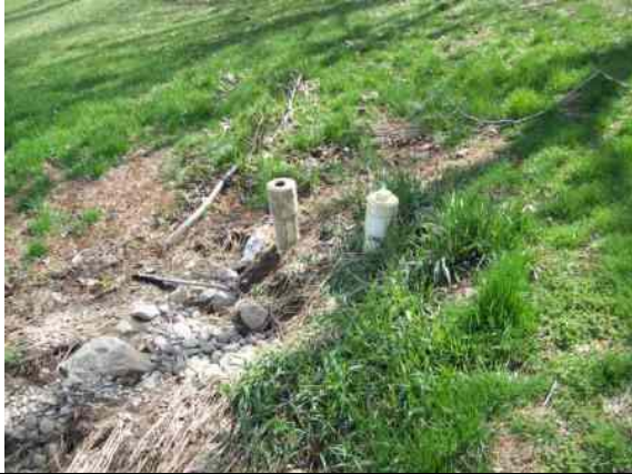
Photo #97: Septic system cleanouts
