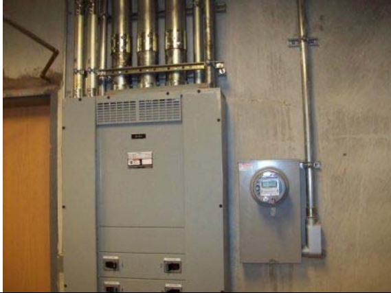
Photo #103: Electric meter
