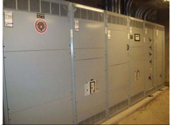
Photo #104: Main switchgear
