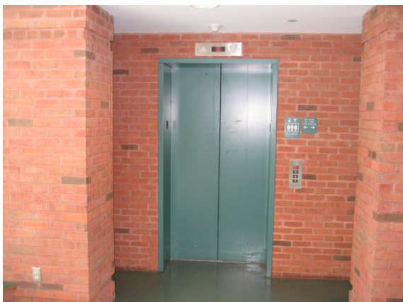
Photo #65: 2-stop hydraulic elevator near the main office
