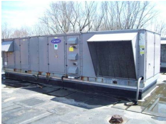
Photo #82: Rooftop Unit 5B
