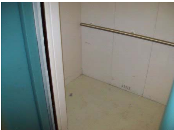
Photo #119: Bus entrance elevator cab interior
