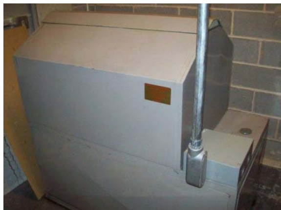
Photo #114: Cafeteria elevator hydraulic equipment
