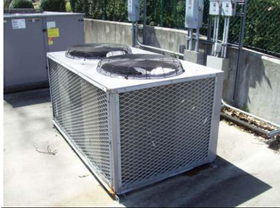
Photo #86: Condensing units for AC-7
