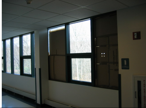
Photo #56: Inside view of two corridor windows that have shattered and been covered with cardboard
