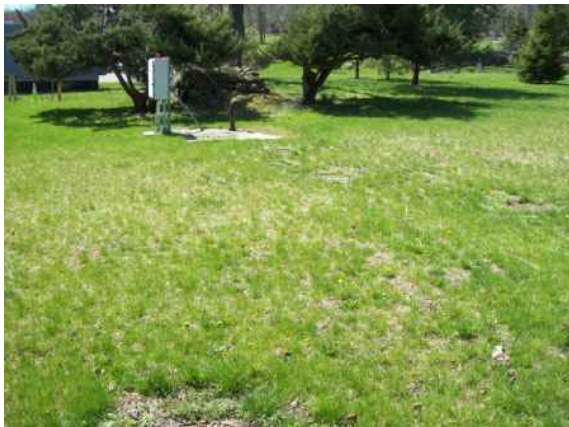
Photo #95: Septic system holding tanks and lift station at west side of property
