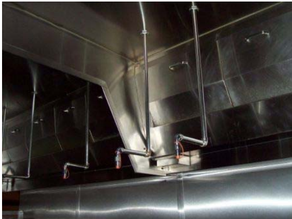
Photo #153: Ansil system in exhaust hood
