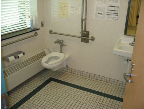
Photo #43: A full ADA accessible, single user toilet room exists in the nurse's office
