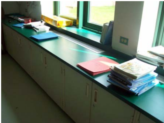
Photo #71: Cabinet-mounted finned tube radiant heat unit
