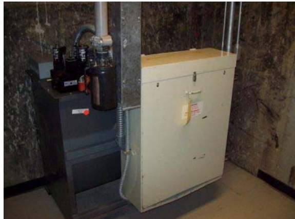
Photo #112: Main elevator hydraulic equipment
