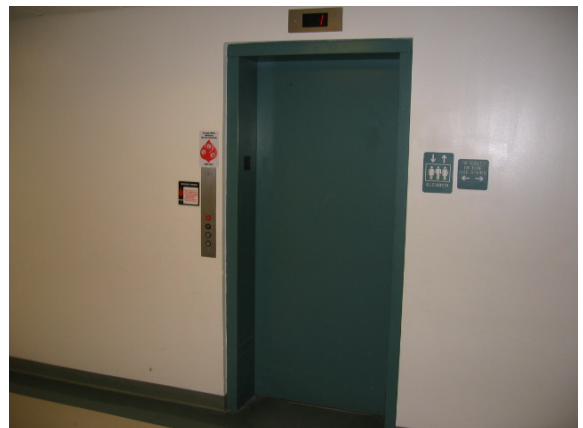
Photo #64: 3-stop hydraulic elevator at cafeteria
