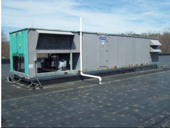
Photo #79: Rooftop Unit 4A
