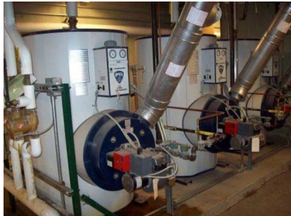
Photo #94: Domestic water boilers
