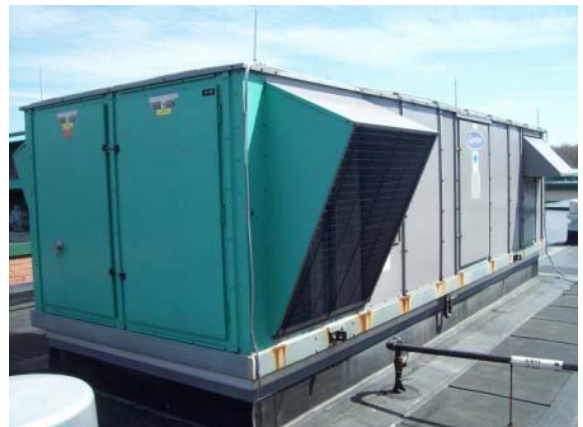
Photo #76: Rooftop Unit 2B
