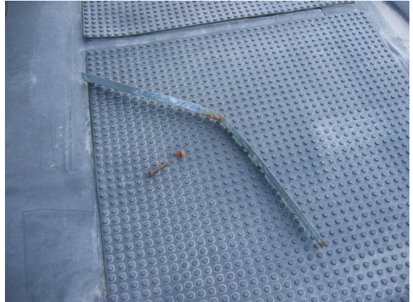
Photo #22: Roof debris of metal straps, screws and nails were observed
