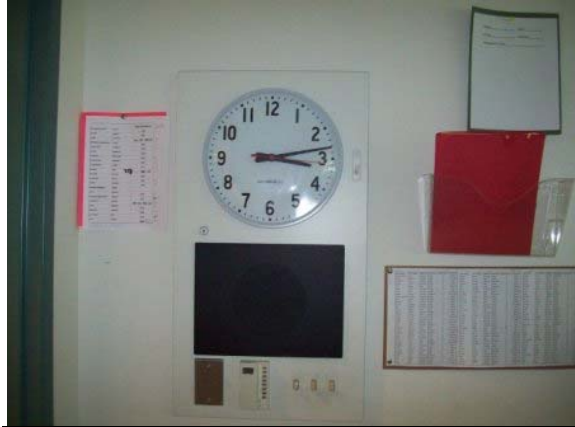
Photo #110: PA panel in classroom
