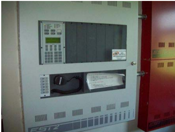
Photo #123: Fire alarm control panel
