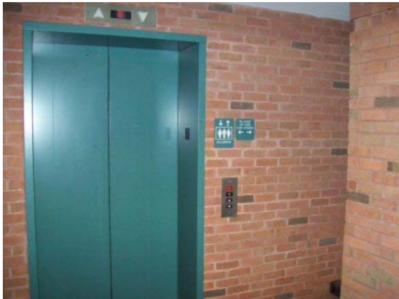
Photo #111: Main elevator
