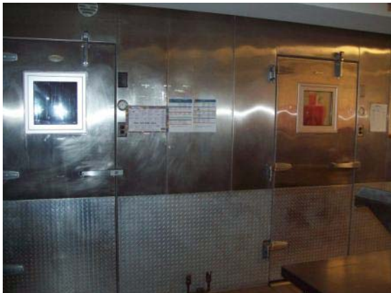
Photo #155: Walk-in cooler and freezer
