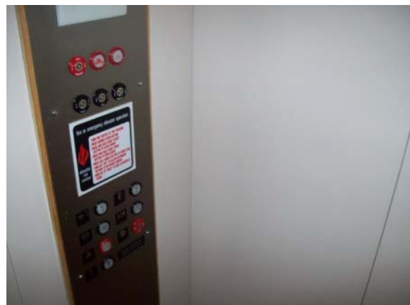
Photo #120: Bus entrance elevator control panel
