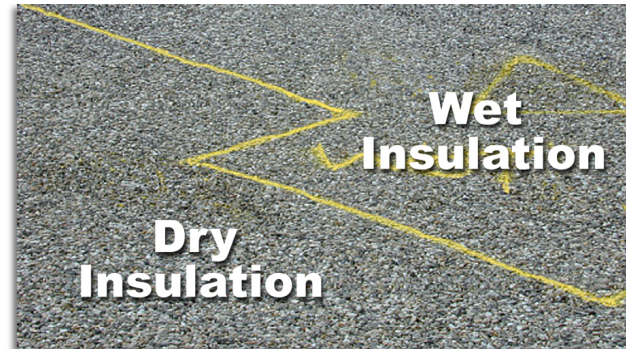
Control image, wet sections marked for removal
