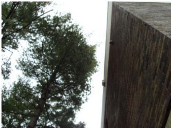
Photo #113: Overgrown trees at rear of building
