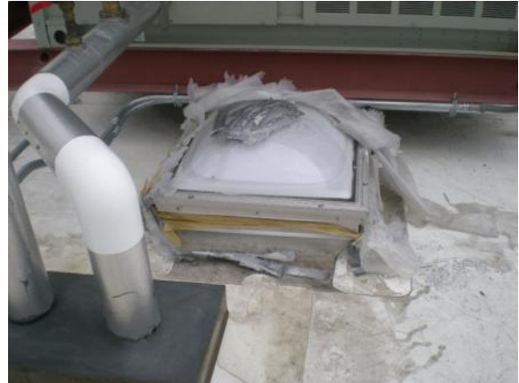
Photo #20: Broken skylight
