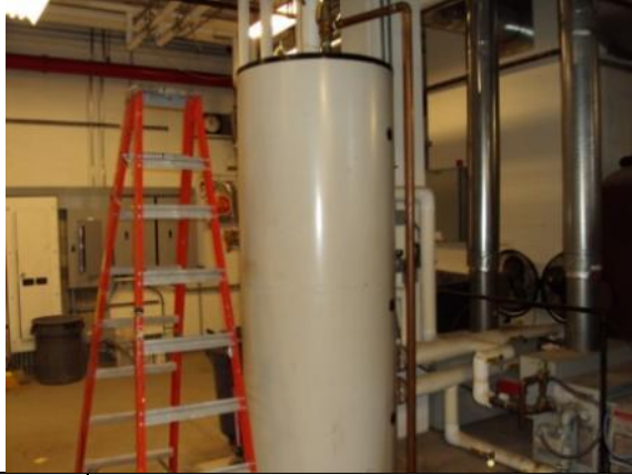
Photo #151: Domestic hot water storage tank
