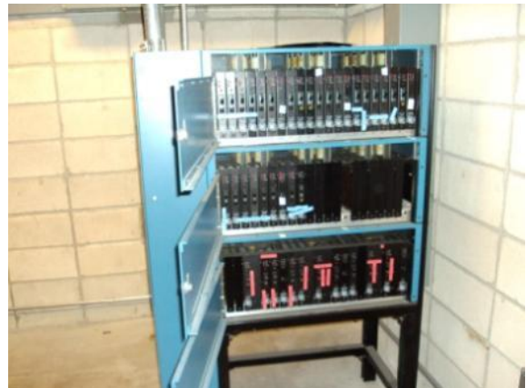
Photo #172: Auditorium lighting controls in auditorium mechanical room
