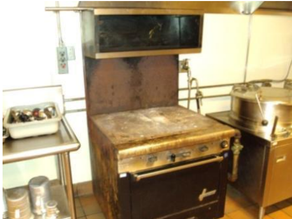
Photo #195: Kitchen gas range
