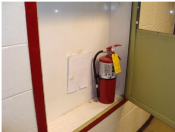
Photo #185: Cabinet-mounted fire extinguisher
