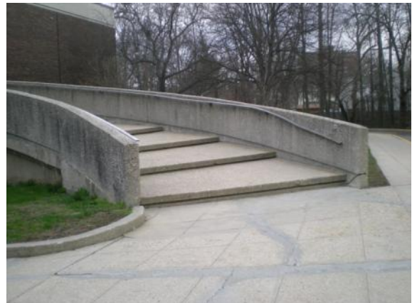
Photo #6: Front entrance – main stair with damaged/loose stair rail and spalled concrete at base of stair
