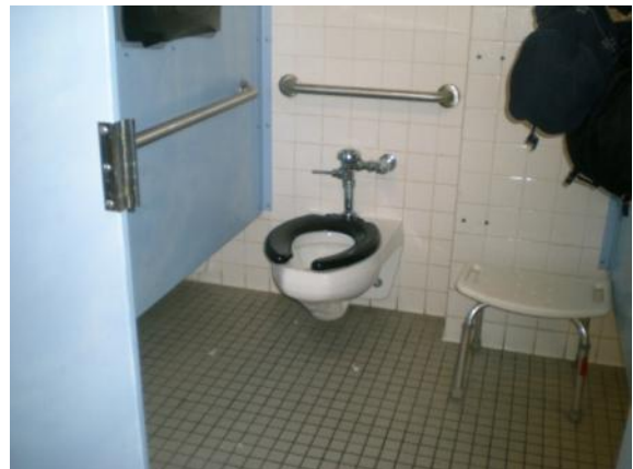
Photo #36: Grab bars mounted too high and not compliant in length at restroom for 110
