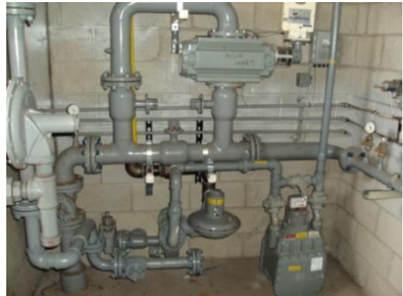
Photo #162: Gas metering
