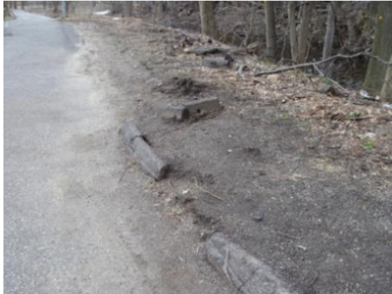
Photo #103: Deteriorating, missing and displaced asphalt curbing at east elevation
