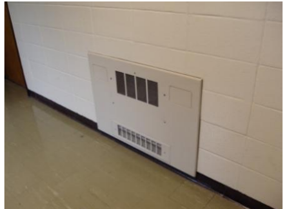
Photo #132: Recessed cabinet radiant unit
