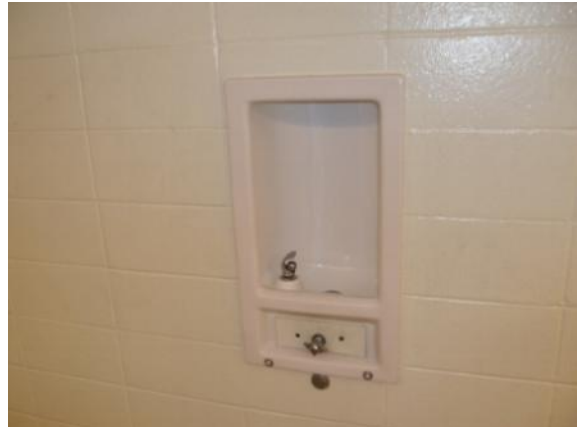
Photo #154: Original common area drinking fountain
