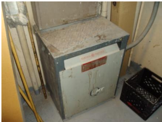
Photo #167: Step-down transformer at electrical closet
