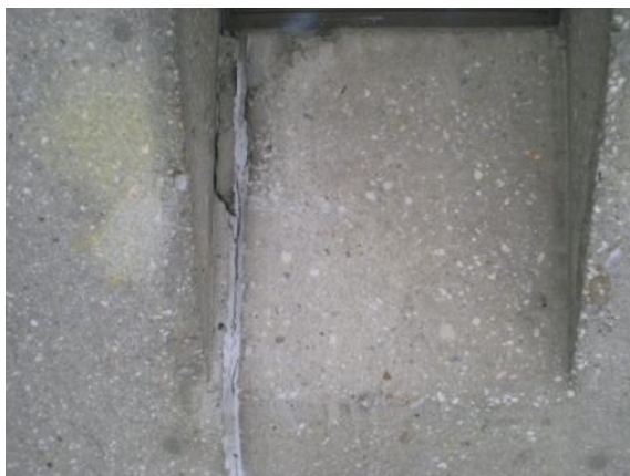
Photo #11: Condition of control joints under windows
