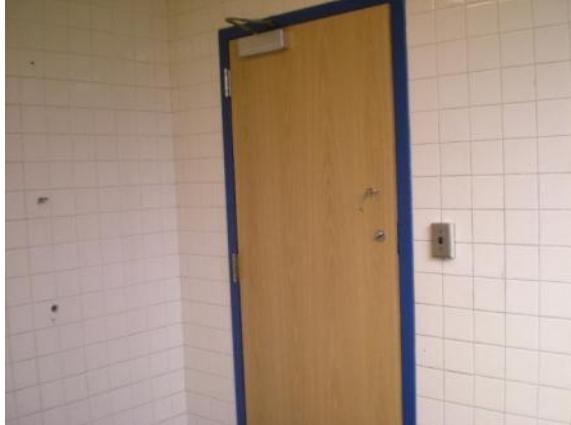
Photo #55: No pull side hardware in restroom
