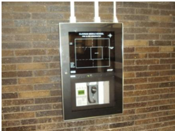
Photo #191: Annunciator panel at lobby
