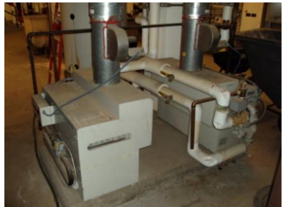
Photo #150: Domestic hot water boilers
