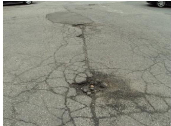
Photo #76: Asphalt deterioration at rear parking lot
