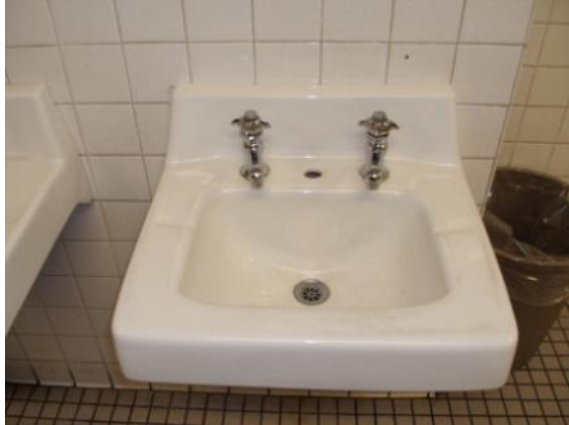
Photo #157: Common area restroom lavatory sink with single hot and cold faucet
