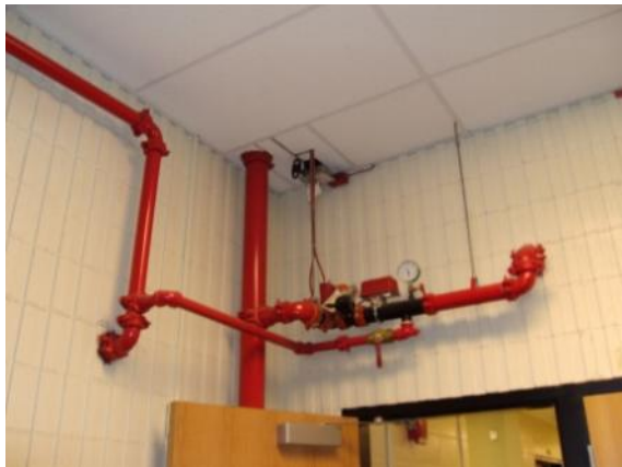
Photo #189: Fire standpipe at stairwell
