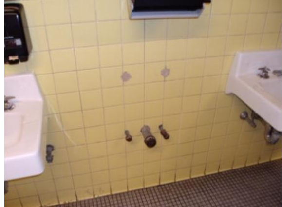
Photo #158: Boys locker room missing a lavatory sink
