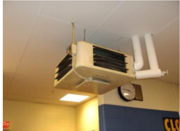
Photo #146: Ceiling-mounted unit heater at kitchen
