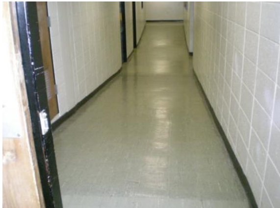
Photo #59: Interior ramp with no handrails
