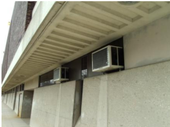
Photo #147: Through-wall air conditioning units for classroom 110
