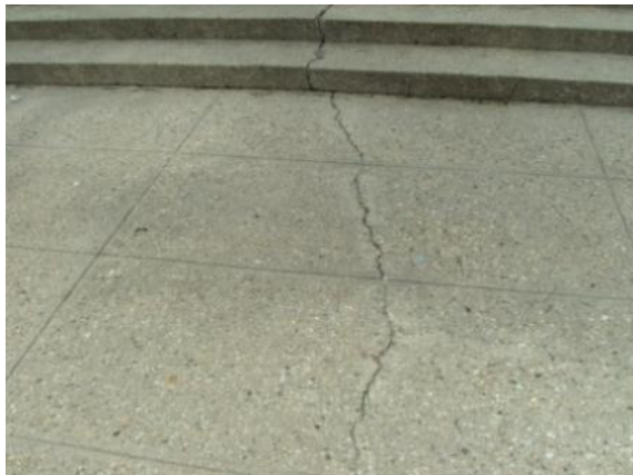
Photo #99: Cracking at front concrete steps/sidewalk
