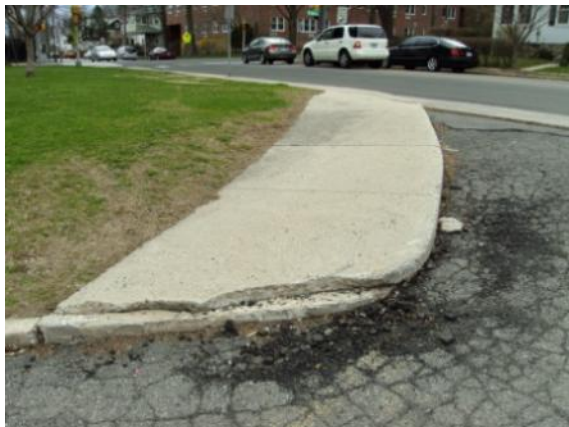
Photo #93: Deterioration at concrete sidewalk and curbing at west elevation
