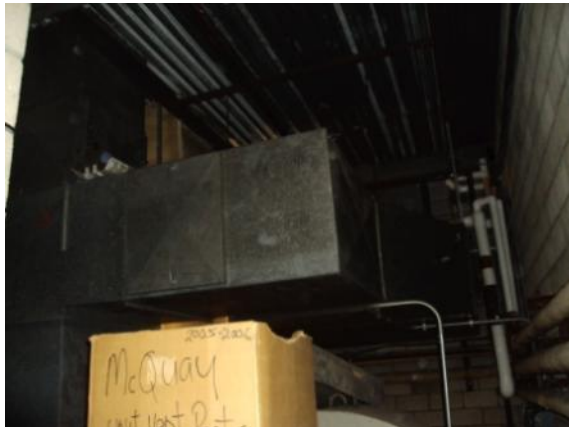
Photo #135: Air handling unit (AHU-16)
