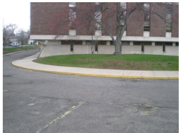
Photo #12: Severely faded ADA designated parking at front with no curb cut near stalls
