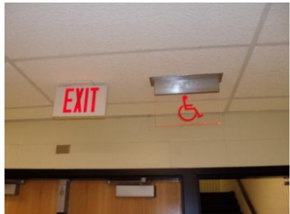
Photo #186: Illuminated exit sign and ADA sign at corridor
