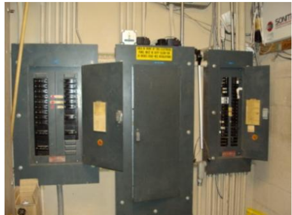
Photo #166: Original circuit breaker panels in electrical closet
