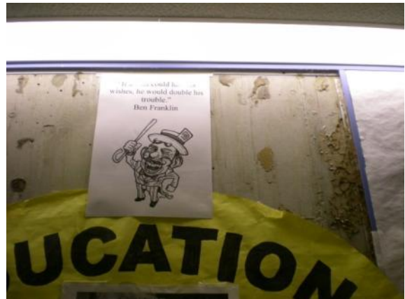
Photo #46: Moisture reported to penetrate wall and damaging wall finishes
