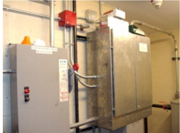
Photo #176: Elevator controls
