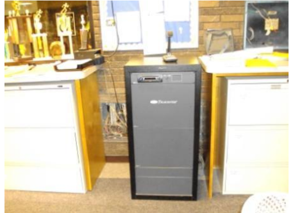
Photo #170: School PA system equipment at office
