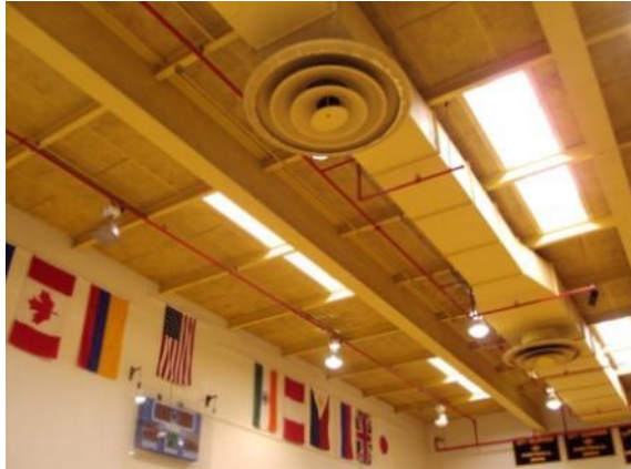
Photo #145: Gym with ceiling-mounted HVAC ducts and diffusers
