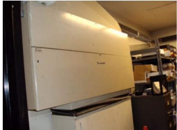
Photo #130: Original unit ventilator serving lobby
