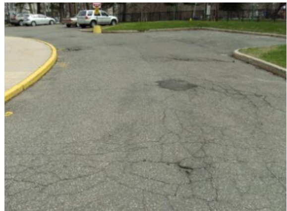
Photo #84: Asphalt condition at front parking area and drive lane
