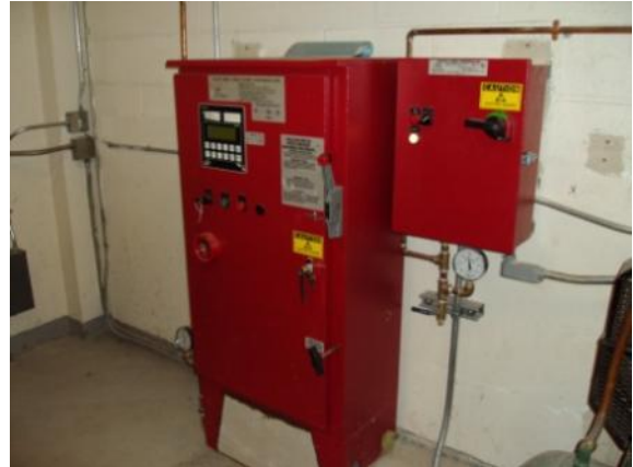
Photo #182: Fire pump controller
