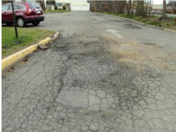
Photo #79: Asphalt deterioration and condition at northwest corner parking area
