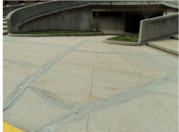
Photo #92: Cracking at concrete sidewalks at front elevation
