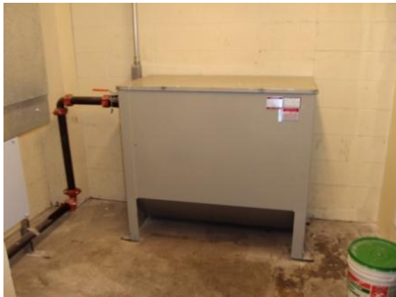
Photo #177: Elevator hydraulic machinery
