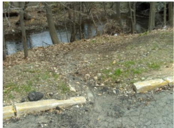
Photo #108: Drainage area requiring stone riprap at east elevation
