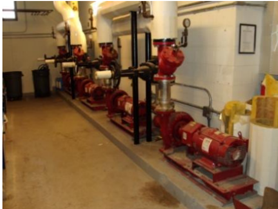
Photo #129: Hot water circulating pumps
