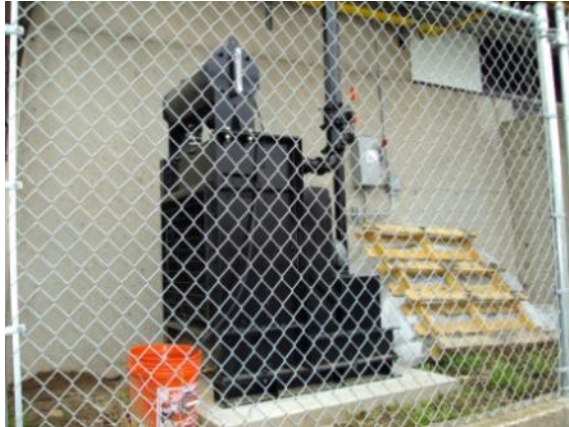
Photo #169: Chain link fence enclosures the generator cooling system at the rear of the building
