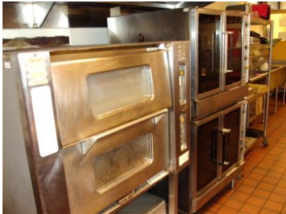
Photo #197: Kitchen gas ovens
