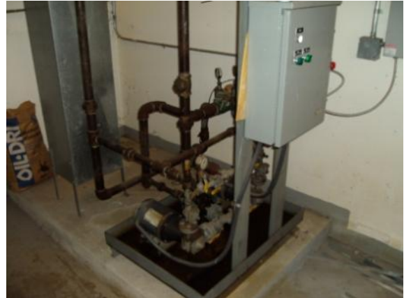
Photo #128: Oil pump set for boilers
