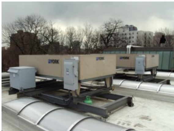
Photo #143: Rooftop condensers for auditorium
