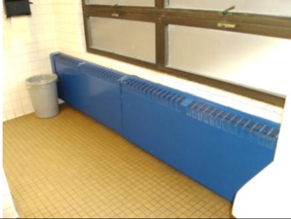
Photo #133: Wall-mounted cabinet radiant unit at restroom
