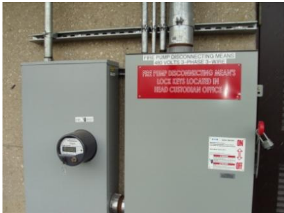
Photo #165: Fire pump meter at rear of building
