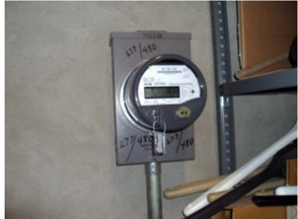
Photo #164: Electric meter at main electrical room
