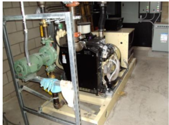
Photo #168: Emergency generator in locked room at rear loading dock area
