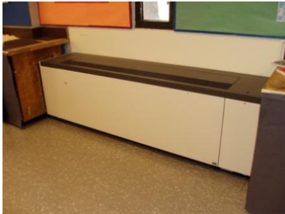
Photo #131: Replacement unit ventilator at classroom
