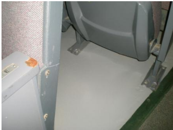
Photo #27: Broken chair backs in auditorium
