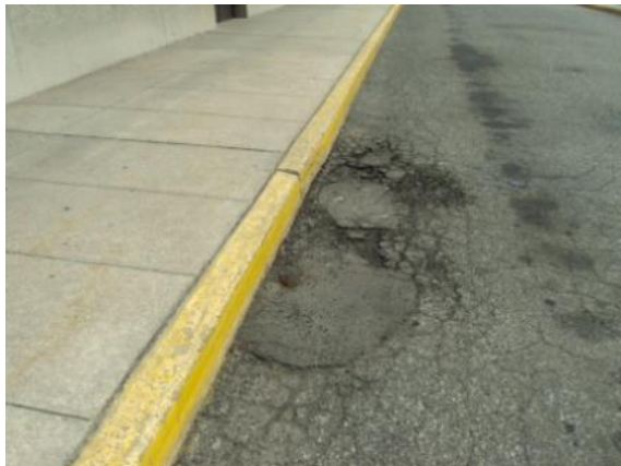
Photo #81: Asphalt deterioration at west drive lane
