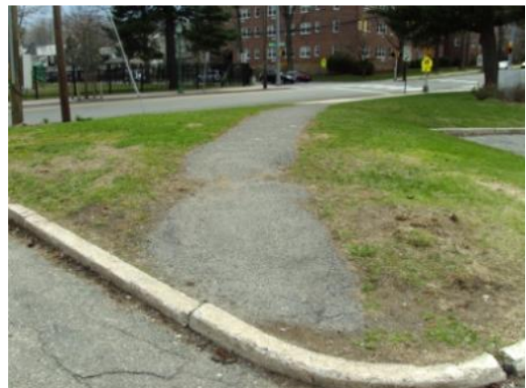
Photo #96: Asphalt sidewalk condition at front elevation
