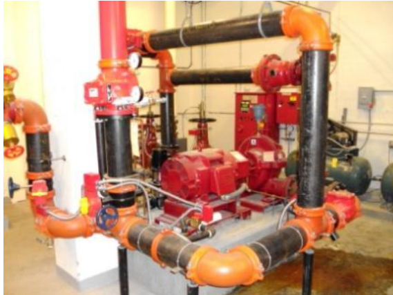
Photo #181: Main fire suppression system at basement mechanical room with fire pump
