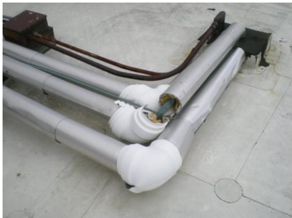
Photo #149: Damaged refrigerant line insulation and rusting electrical conduit at roof
