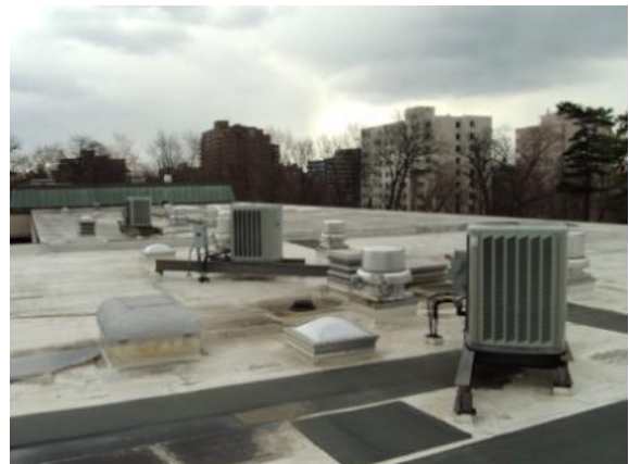
Photo #144: Rooftop condensers for offices/teachers lounge areas
