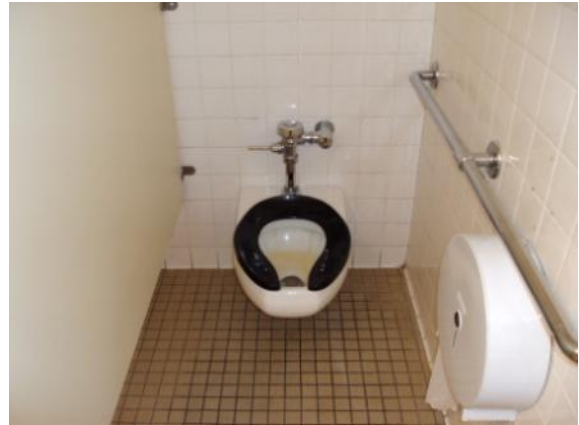
Photo #160: Wall-mounted toilet at restroom
