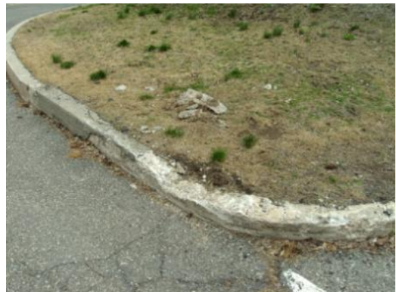
Photo #102: Deteriorating concrete curbing at rear of building
