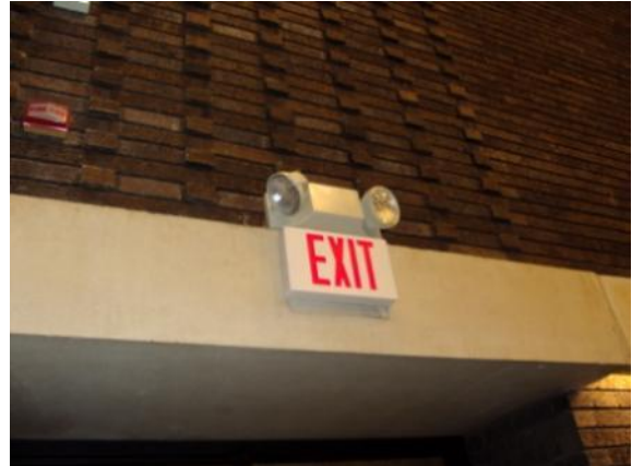
Photo #188: Illuminated exit sign and emergency lights at auditorium
