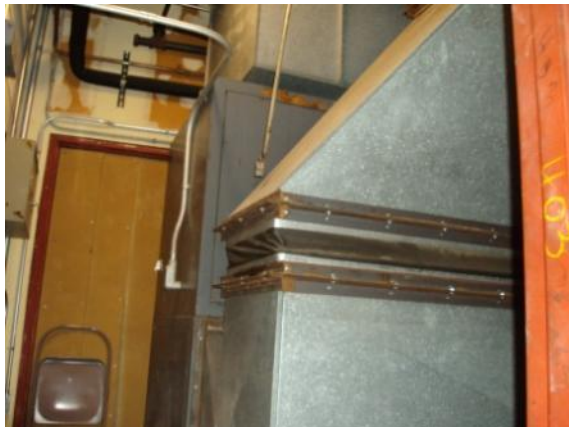
Photo #137: Air handling unit (AHU-18)
