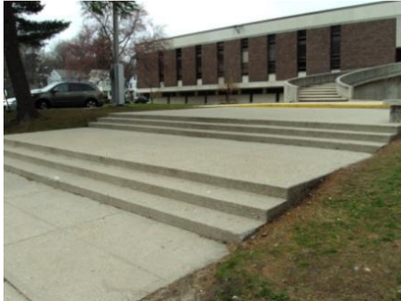
Photo #97: Concrete steps at front elevation (note missing handrails)
