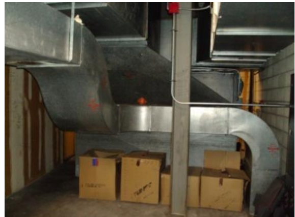
Photo #138: Air handling unit (AHU-19)
