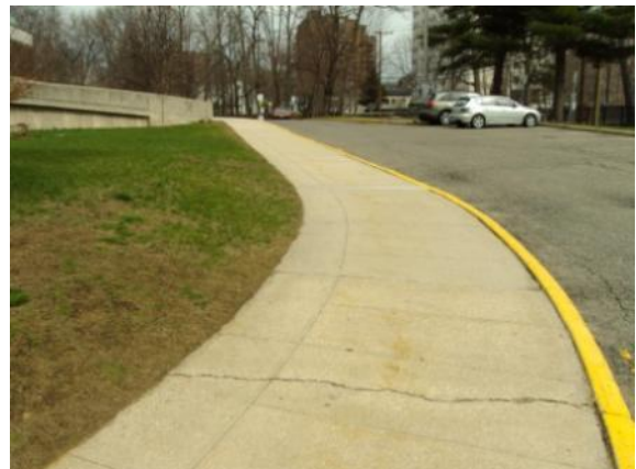
Photo #90: Concrete sidewalk at front of building (note cracking)
