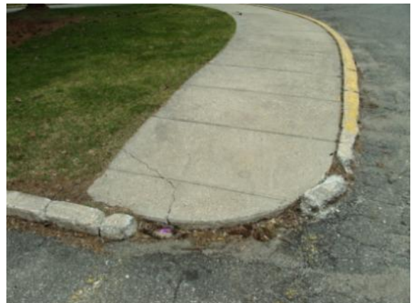
Photo #94: Tripping hazard and deterioration at concrete sidewalk and curbing at rear of building
