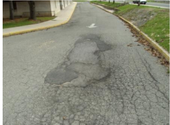
Photo #80: Asphalt condition at rear of west drive lane
