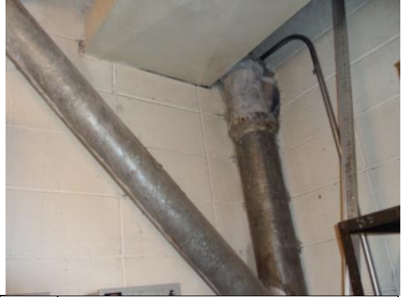
Photo #152: 4-inch galvanized steel piping
