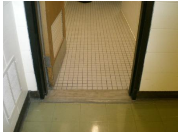
Photo #34: High threshold at restroom for 110
