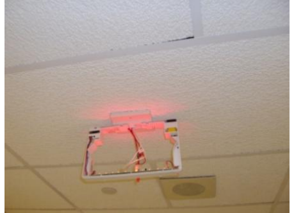
Photo #194: Damaged exit sign at ground floor corridor
