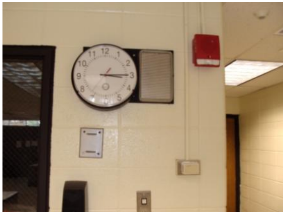
Photo #171: PA system call button and speaker in classroom, with adjacent clock, thermostat and strobe alarm
