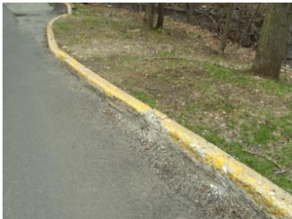
Photo #101: Deteriorating concrete curbing along east drive lane
