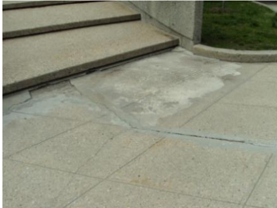
Photo #91: Concrete sidewalk front elevation with repair area that is cracking and deteriorating
