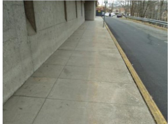
Photo #86: Concrete sidewalk and curbing along right side of building
