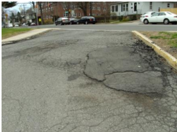
Photo #83: Asphalt deterioration entering from Powell Place
