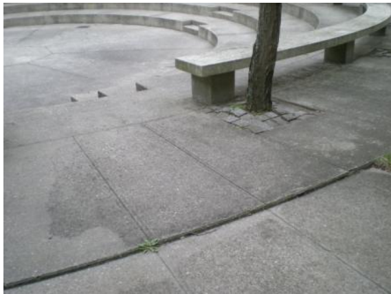
Photo #45: Vertical displacement at courtyard creating tripping hazards
