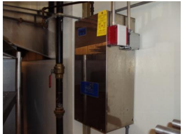
Photo #184: Ansul system for kitchen hood
