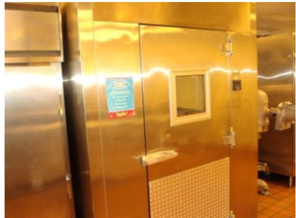
Photo #202: Roll-in refrigeration unit at kitchen
