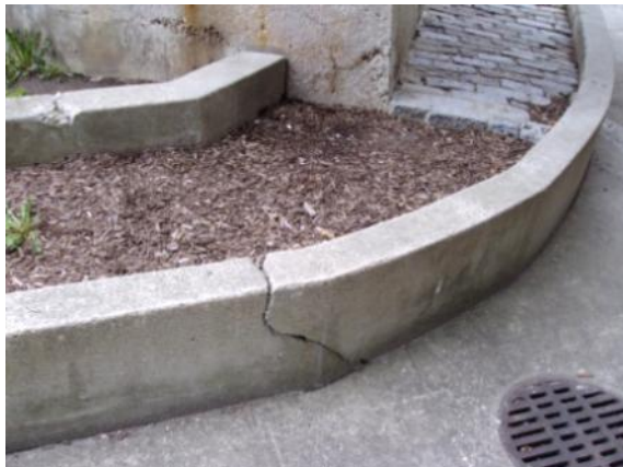
Photo #111: Cracking/shifting of concrete retaining wall at front elevation
