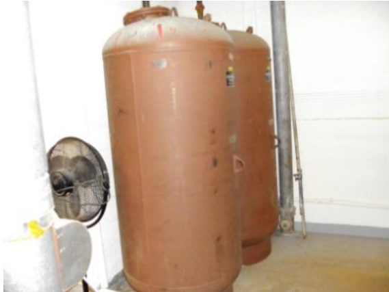
Photo #127: Boiler expansion tanks
