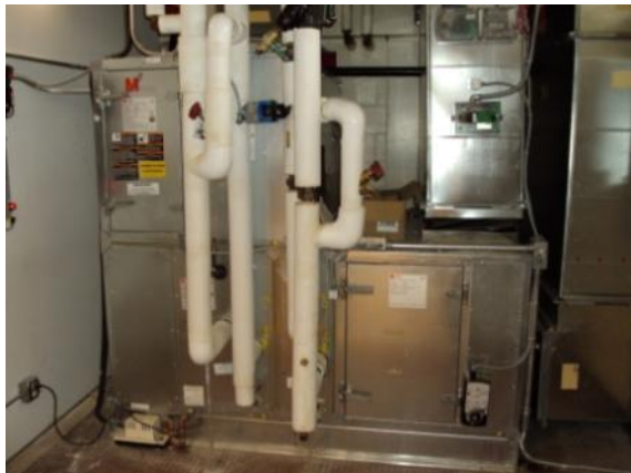
Photo #141: Air handling unit (AHU-1)
