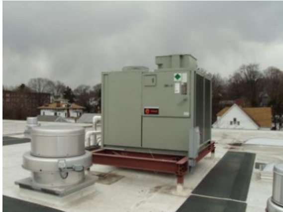
Photo #139: Rooftop air-cooled liquid chiller
