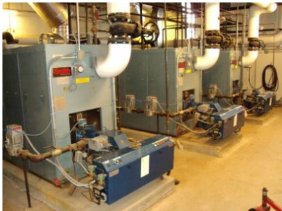
Photo #125: Three hot water heating boilers
