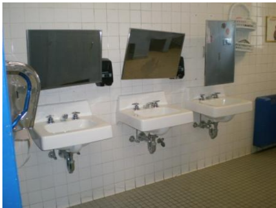
Photo #35: Non-insulated drain lines in restroom for 110
