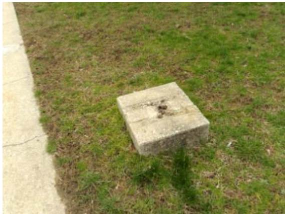
Photo #123: Abandoned concrete base adjacent to front sidewalk
