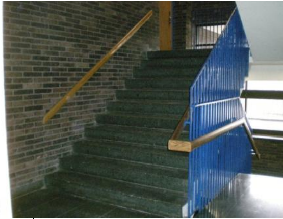
Photo #31: Stair with no railing extensions
