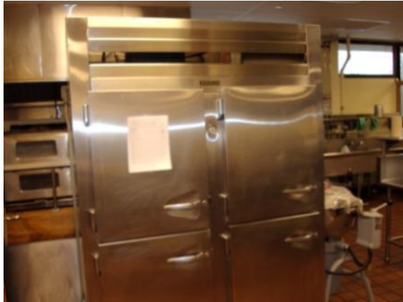
Photo #199: Refrigeration unit in kitchen
