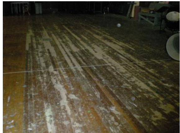
Photo #28: Worn stage in auditorium
