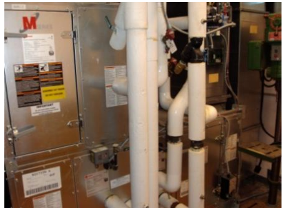
Photo #142: Air handling unit (AHU-2)
