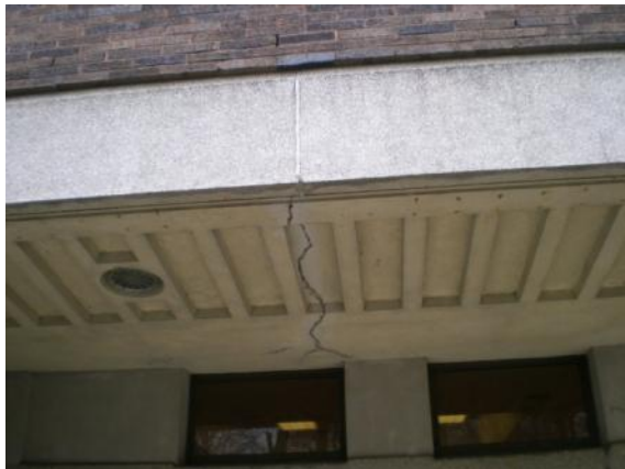
Photo #15: Cracks at soffit
