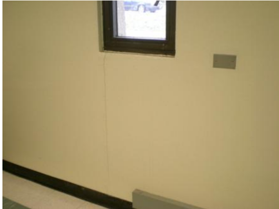
Photo #43: Crack at wall under window
