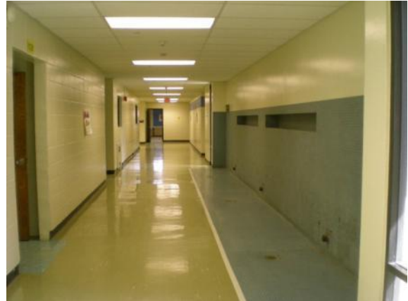
Photo #38: Lower level (ground) corridor with ceramic tile at former sink area
