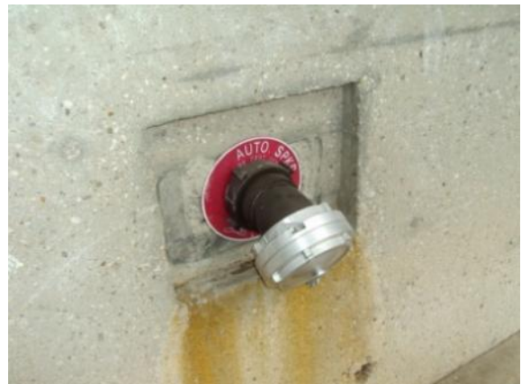
Photo #192: Fire house connection at building exterior wall
