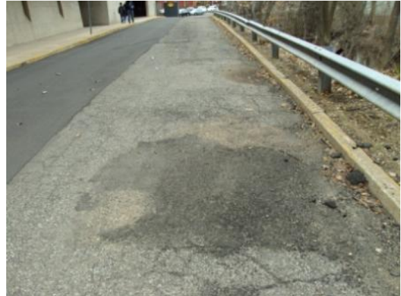
Photo #74: Asphalt condition along right side of east drive lane
