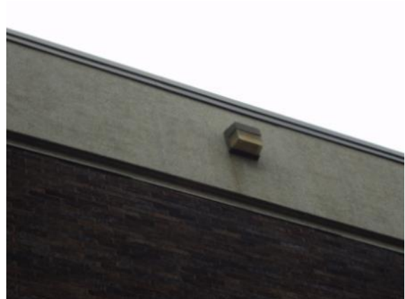
Photo #122: Building-mounted light fixture
