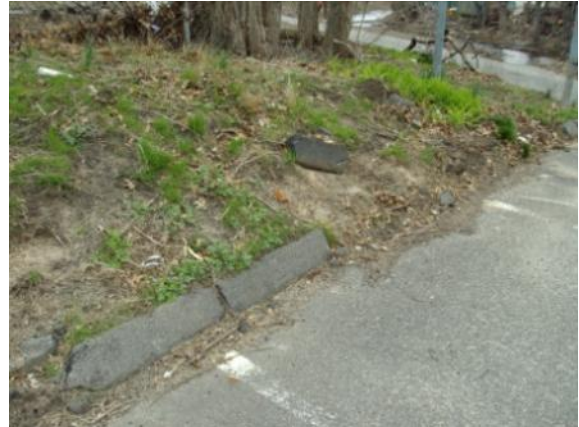
Photo #104: Deteriorating, missing and displaced asphalt curbing at rear parking lot
