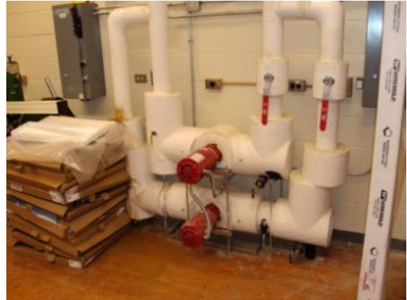
Photo #140: Chiller circulating pumps
