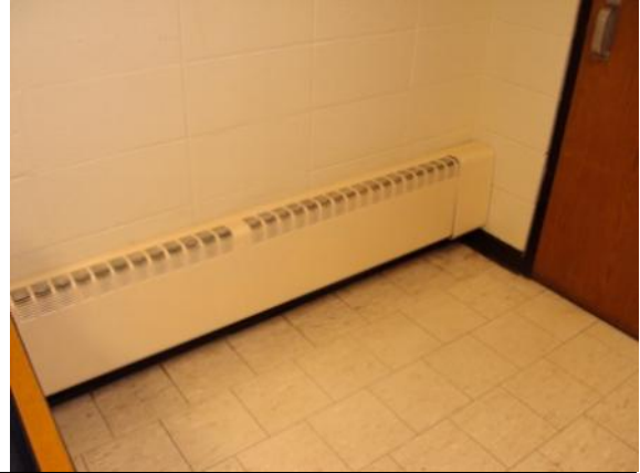
Photo #134: Baseboard-mounted cabinet radiant unit at restroom
