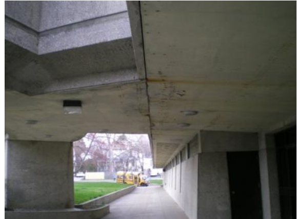
Photo #8: Exposed rebar, spalling and water infiltration evidence under main stair connection to main entrance
