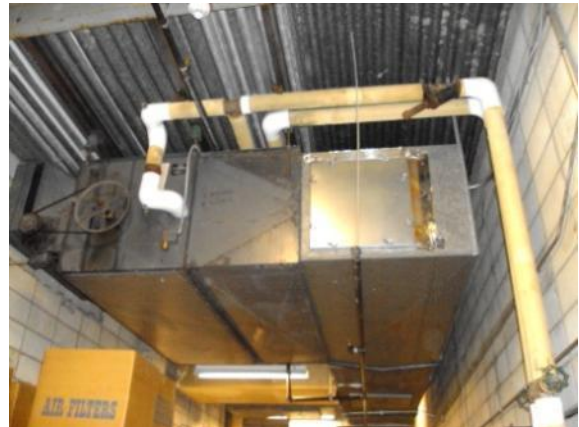
Photo #136: Air handling unit (AHU-17)
