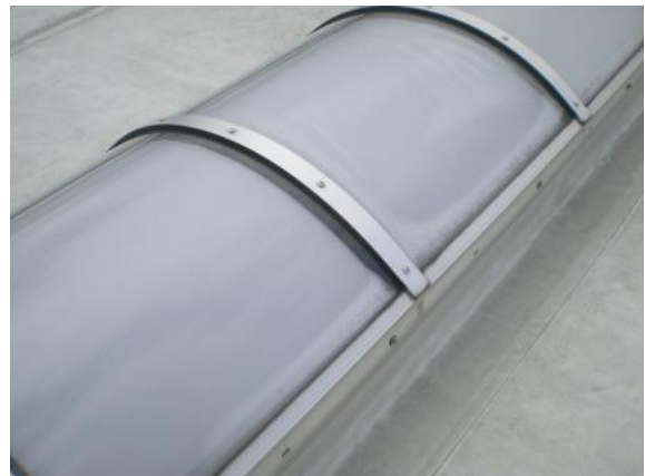
Photo #18: Broken seals on barrel type skylights
