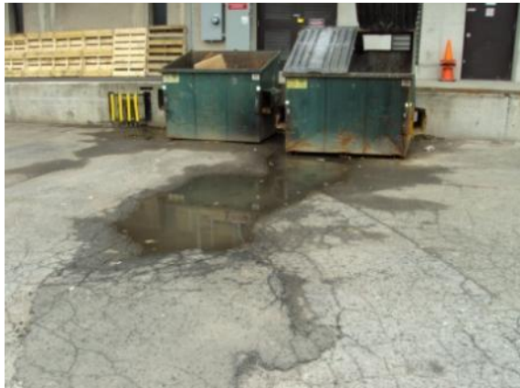
Photo #71: Ponding at asphalt pavement – adjacent to rear loading dock
