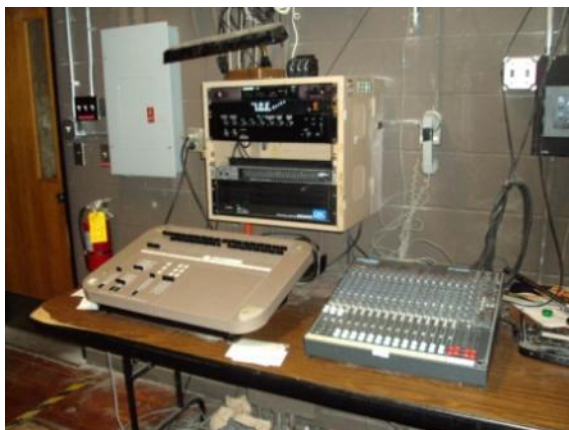
Photo #173: Auditorium audio and light controls at stage
