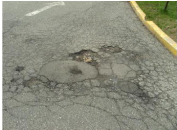
Photo #72: Asphalt deterioration entering east drive lane
