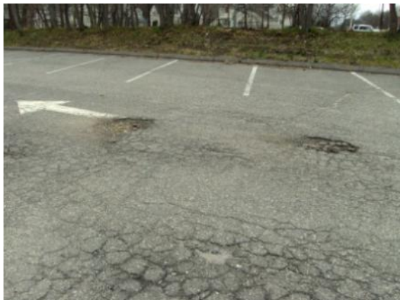
Photo #77: Asphalt deterioration at rear parking lot
