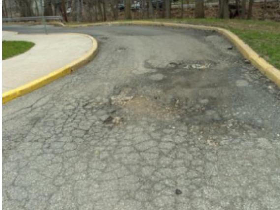
Photo #73: Asphalt deterioration entering east drive lane
