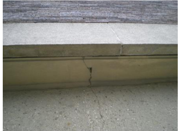
Photo #14: Cracks at fascia and soffit
