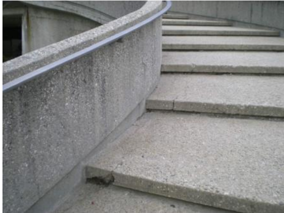
Photo #7: Cracked stair treads at front entrance main stair
