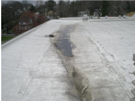
Photo #19: Ponding on roof - tapered insulation does not promote proper drainage
