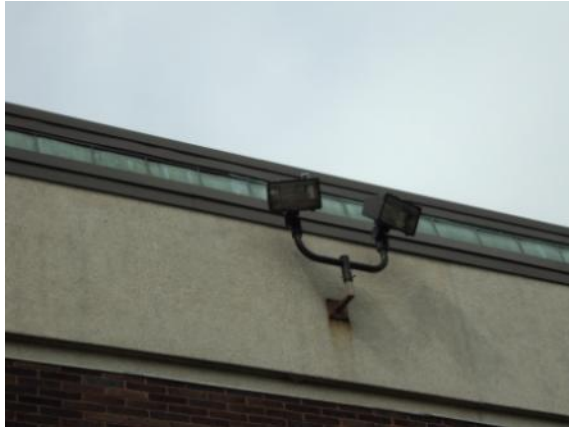
Photo #121: Building-mounted light fixture
