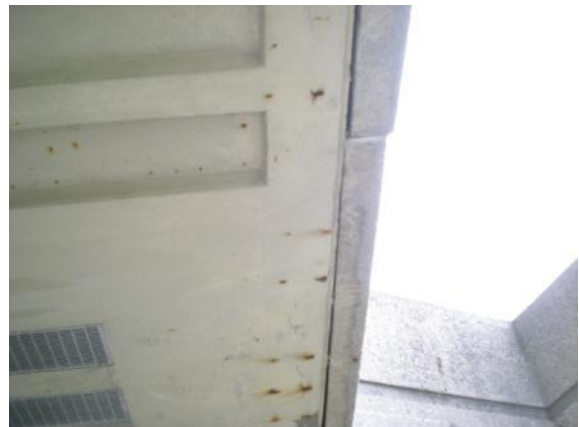
Photo #10: Exposed rebar at soffit and horizontally shifted precast concrete panel at front
