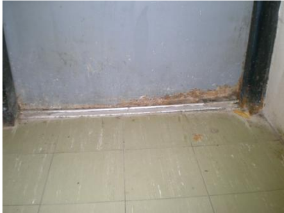
Photo #61: Rusted service doors and frame with evidence of water infiltration near music rooms
