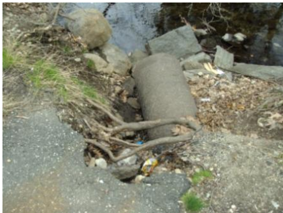
Photo #107: Drainage swale requiring stone riprap at east elevation
