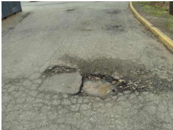
Photo #75: Asphalt deterioration at the rear of the east drive lane
