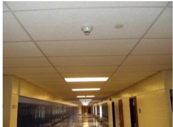
Photo #190: Smoke detector and recess sprinkler head at corridor
