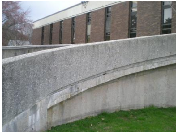
Photo #5: Front entrance – main stair showing water evidence penetrating concrete
