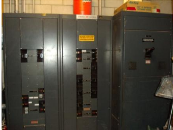
Photo #163: Main electrical switchgear (adjacent to the custodial break room)
