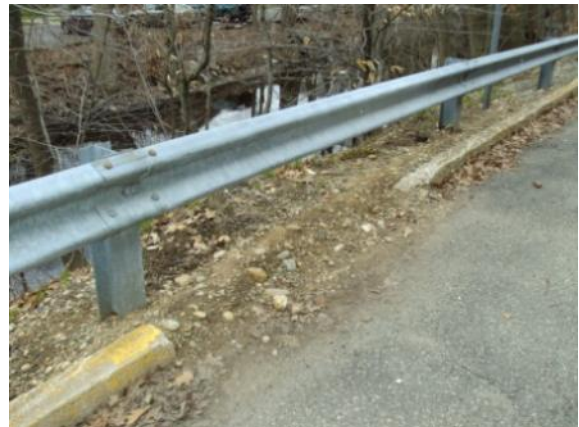
Photo #100: Deteriorating/missing section of concrete curbing along east drive lane
