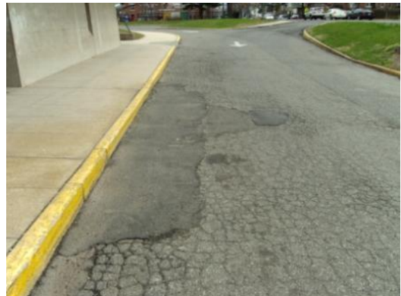
Photo #82: Asphalt deterioration at west drive lane
