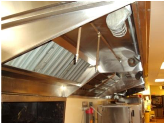
Photo #183: Exhaust hood with fire suppression
