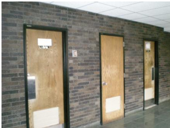
Photo #29: Common area restrooms with high thresholds
