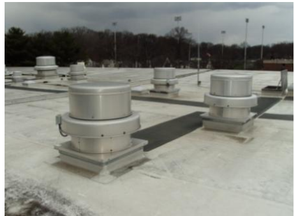
Photo #148: Rooftop exhaust fans, with larger fan for kitchen
