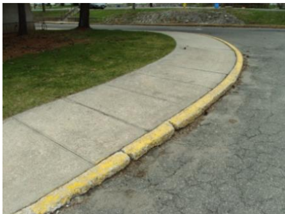
Photo #95: Settlement of concrete sidewalk and deteriorating curbing at rear of building
