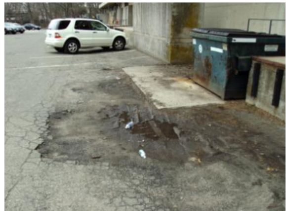
Photo #78: Asphalt deterioration adjacent to rear dumpster
