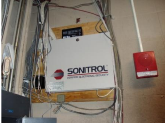
Photo #193: Security alarm panel in electrical closet by main office
