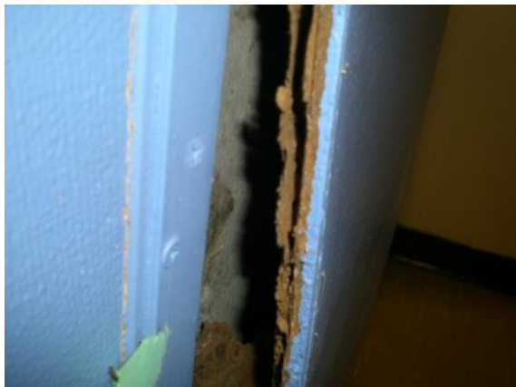
Photo #47: Moisture reported to penetrate wall and damaging wall finishes
