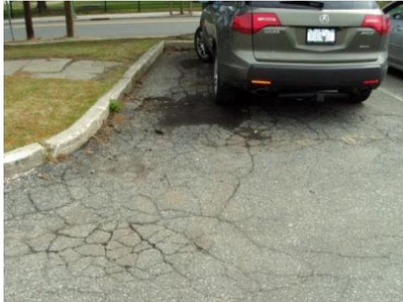
Photo #85: Asphalt deterioration at front parking area
