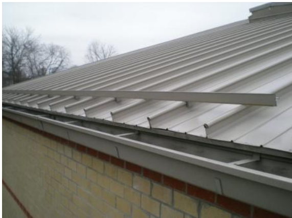
Photo #87: Ice dam does not seem to prevent snow and ice from sheeting
