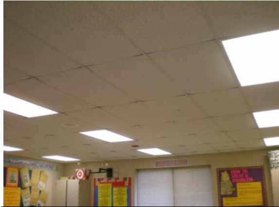
Photo #116: Bulging and cupping acoustic tile
