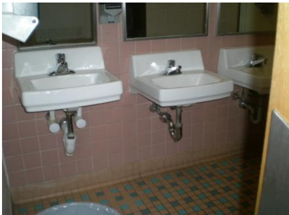
Photo #119: Missing drain pipe insulation
