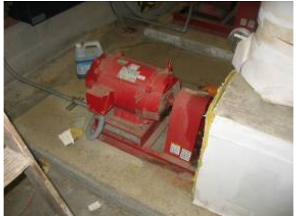
Photo #28: View of water circulation pumps.
