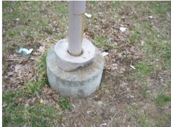
Photo #4: View of damaged base of pole mounted lighting fixture.
