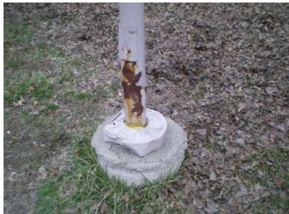
Photo #66: Moderate to severely damaged light pole
