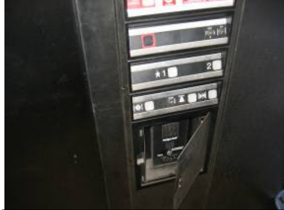
Photo #50: View of passenger elevator cab control panel.
