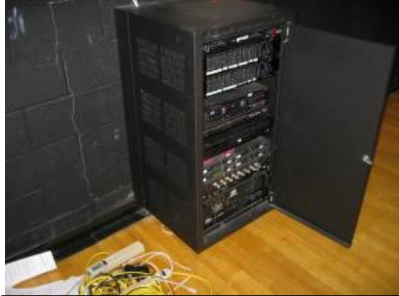
Photo #62: View of auditorium sound system.
