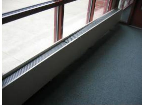
Photo #32: View of fin tube radiators.
