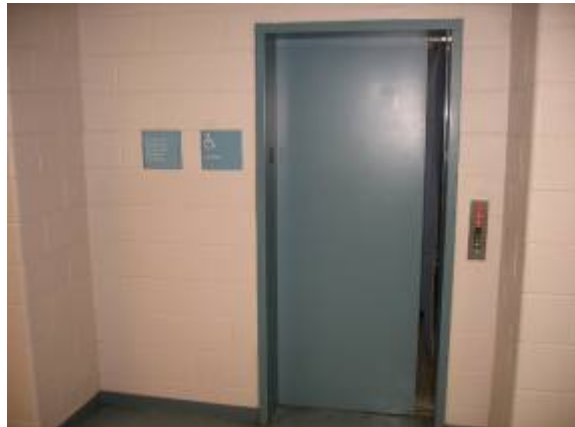
Photo #48: View of passenger elevator doors.
