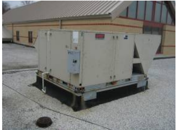
Photo #34: View of RTU-1.
