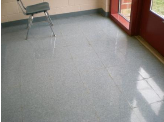
Photo #115: Deteriorated edges of vinyl tile from moisture
