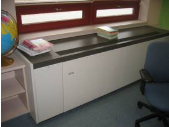
Photo #31: View of fan coil unit.
