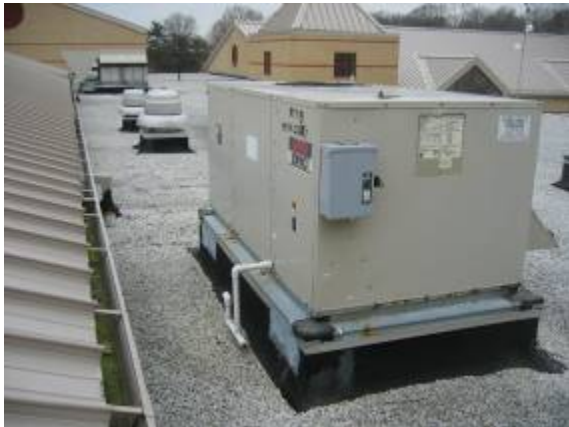
Photo #41: View of RTU-8.
