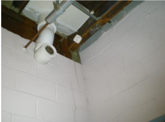
Photo #127: Cracking through block and exposed structure
