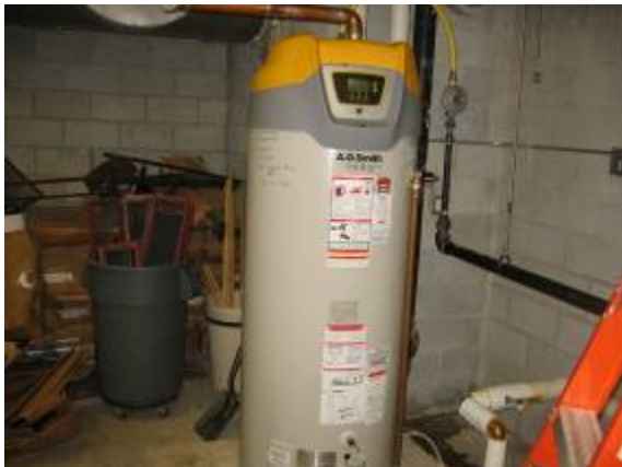
Photo #45: View of domestic hot water heater.
