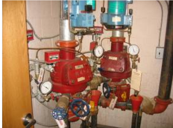
Photo #56: View of sprinkler valves.
