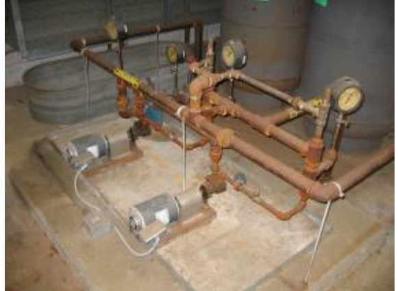
Photo #26: View of fuel oil circulation pumps.
