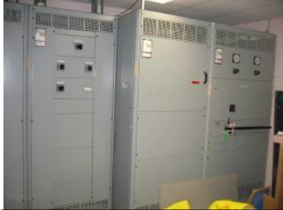
Photo #44: View of main electrical switchgear.
