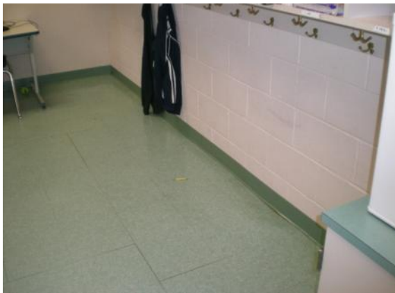
Photo #131: Separated vinyl tile and dip in slab at 2 nd floor classroom
