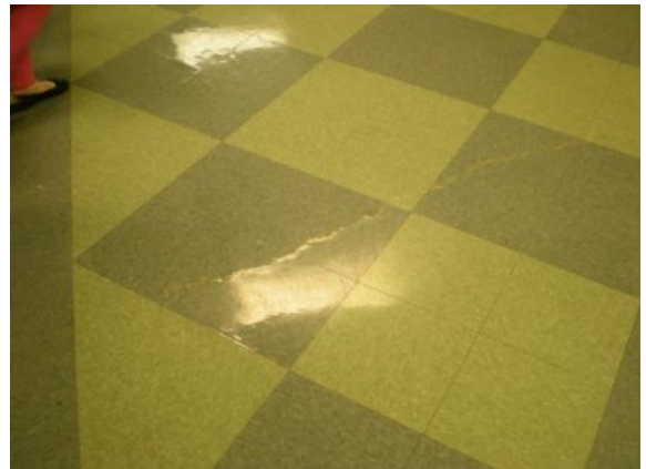
Photo #130: Cracking slab under vinyl tile flooring finish
