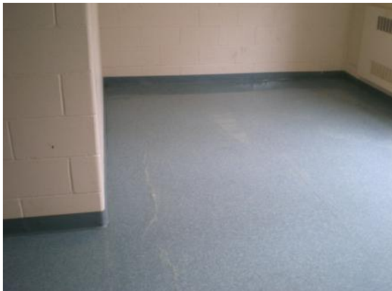
Photo #129: Cracking slab under flooring finish
