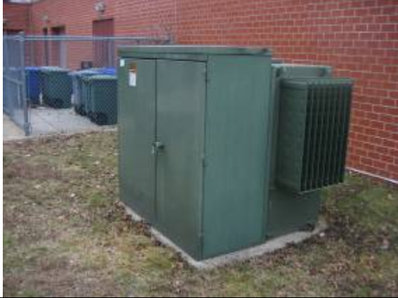
Photo #43: View of pad mounted electrical transformer.
