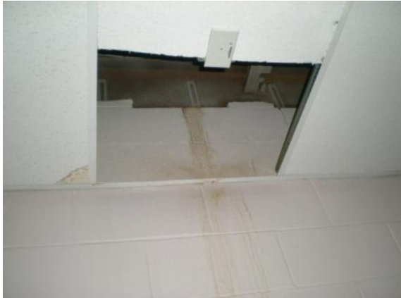
Photo #91: Active leak in side area off main lobby
