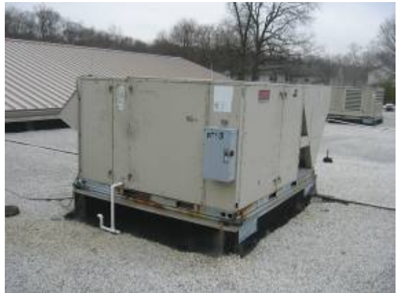
Photo #36: View of RTU-3.
