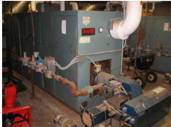
Photo #24: View of Boiler No. 2.
