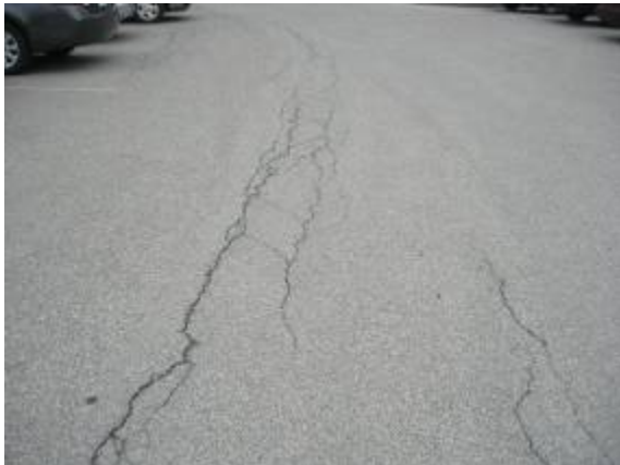
Photo #17: View of deteriorated asphalt parking lot.
