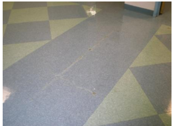
Photo #132: Cracking slab under vinyl tile flooring finish
