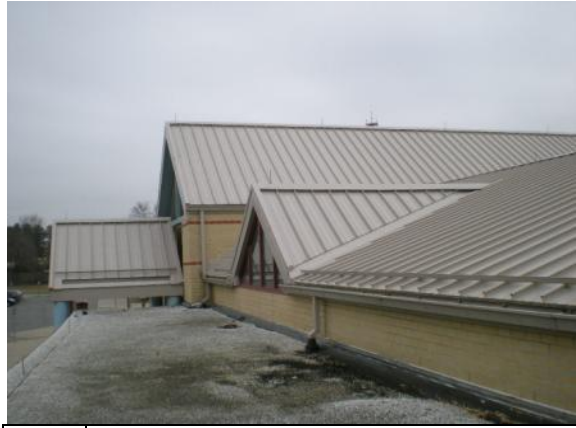
Photo #86: Roof over covered walkway with evident of ponding
