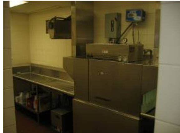
Photo #52: View of dishwashing station.
