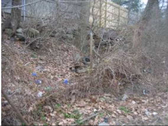
Photo #13: View of damaged chain link fencing system.
