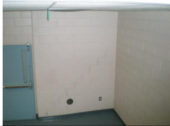
Photo #122: Stair step cracking
