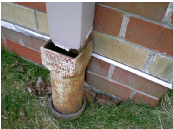
Photo #77: Condition of downspout
