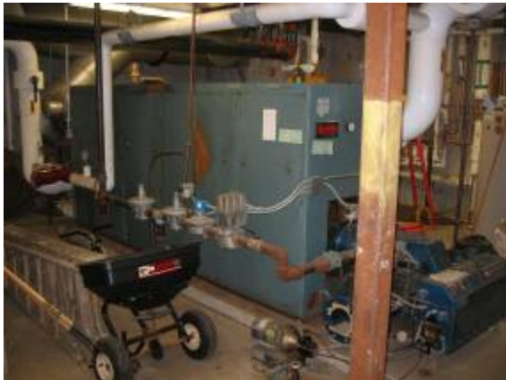
Photo #23: View of Boiler No. 1.
