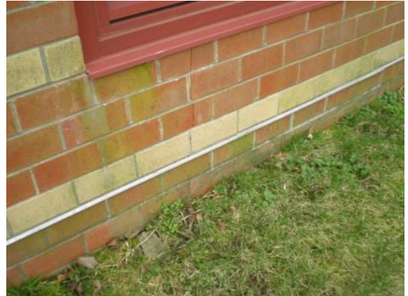
Photo #128: Cracking at brick veneer
