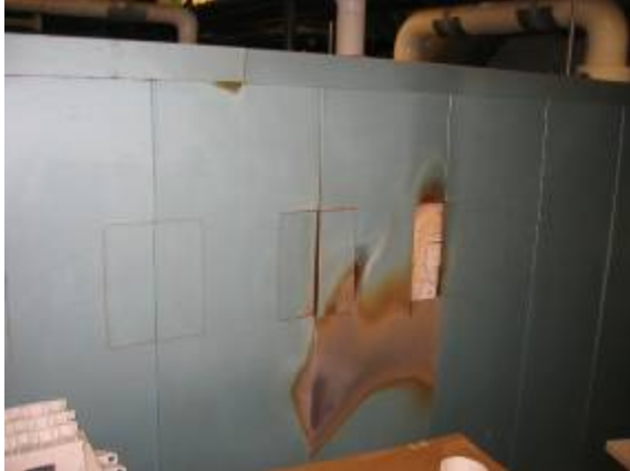
Photo #25: View of damaged portion of Boiler No. 1.
