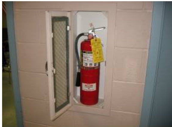
Photo #58: View of fire extinguisher.
