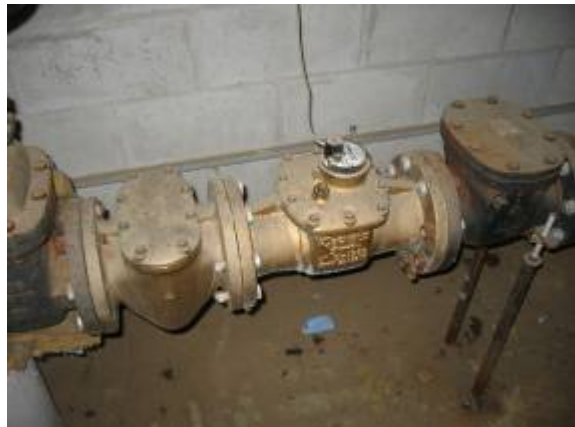
Photo #46: View of water metering equipment.
