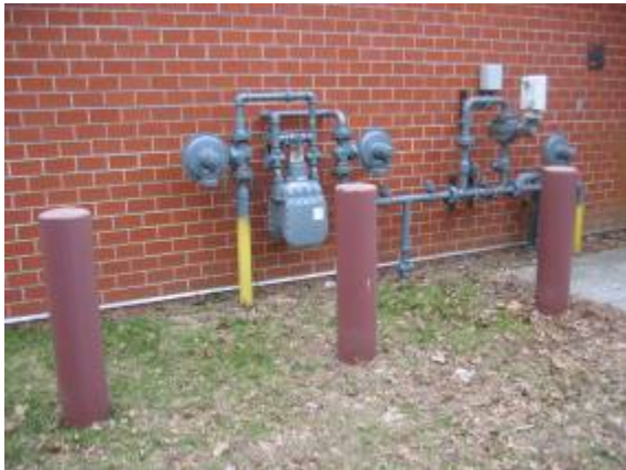
Photo #47: View of natural gas metering equipment.
