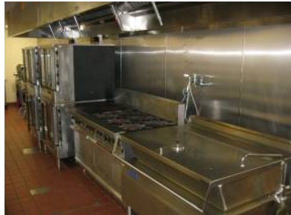
Photo #54: View of commercial kitchen equipment.
