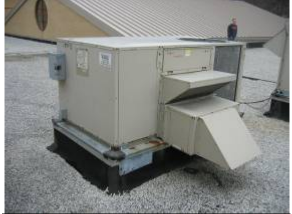
Photo #38: View of RTU-5.
