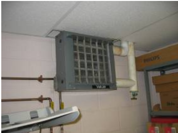
Photo #29: View of auxiliary heater.
