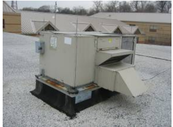
Photo #40: View of RTU-7.
