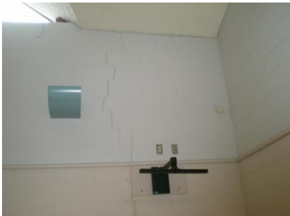
Photo #125: Cracking in concrete masonry units
