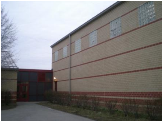
Photo #71: Rear elevation of gymnasium with vandalized glass block units
