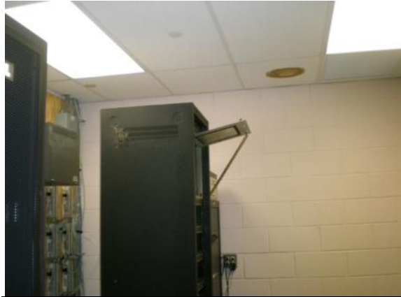
Photo #104: Leak in Media Center server room
