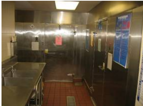
Photo #53: View of commercial kitchen equipment.
