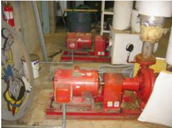
Photo #27: View of water circulation pumps.
