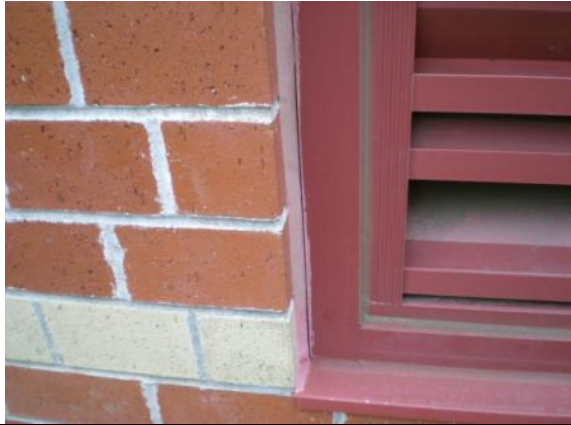
Photo #74: Separation of window sealant
