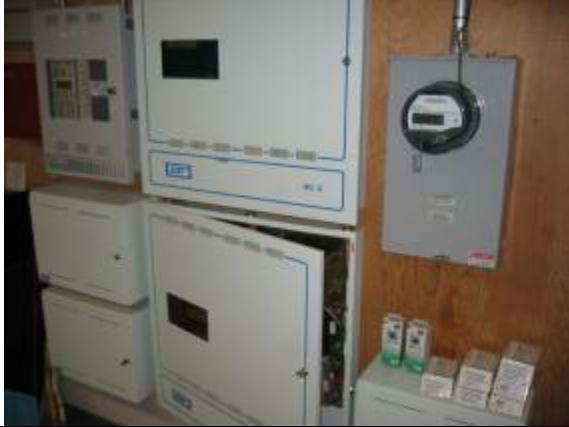
Photo #61: View of fire control panel.
