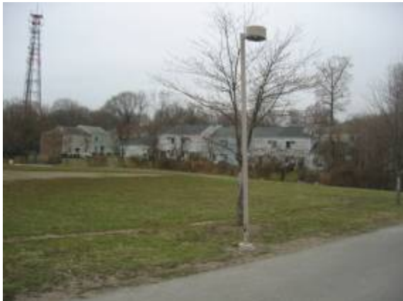
Photo #5: View of damaged pole mounted lighting fixture.
