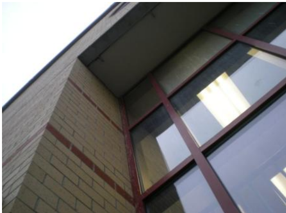
Photo #75: Area of birds infiltrating open joints at rear
