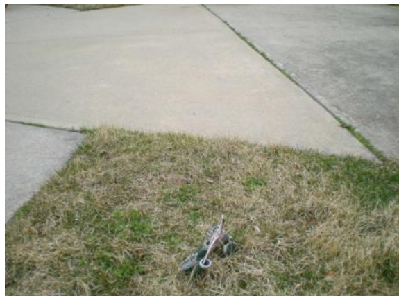
Photo #64: Damaged electrical receptacles in courtyard
