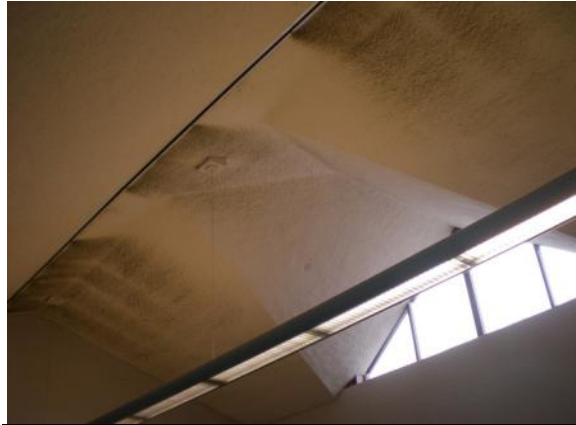
Photo #98: Dirt from diffuser at ceiling
