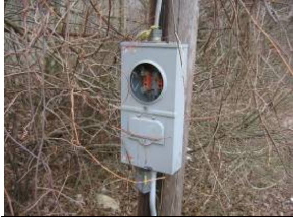
Photo #14: View of abandoned electrical service metering equipment.
