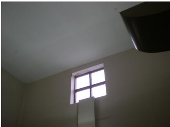
Photo #107: Active leak at high window in FRC3
