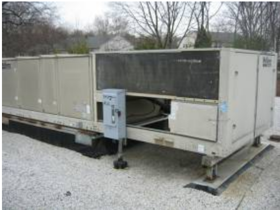
Photo #35: View of RTU-2.
