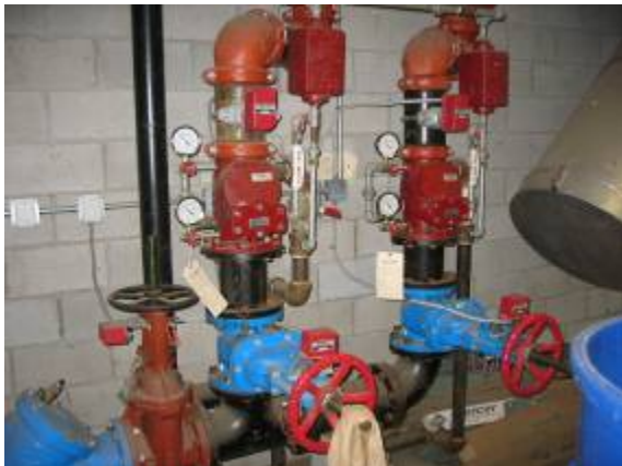
Photo #57: View of sprinkler valves.
