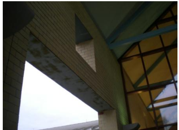
Photo #82: Exposed metal structure/soffit at main entrance
