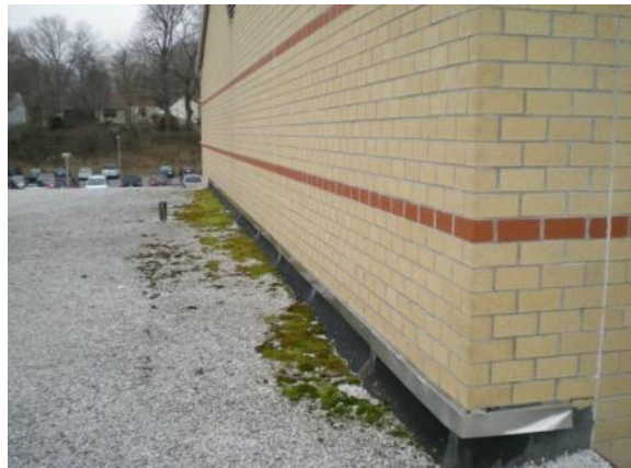
Photo #88: Moss build up against gymnasium at roof
