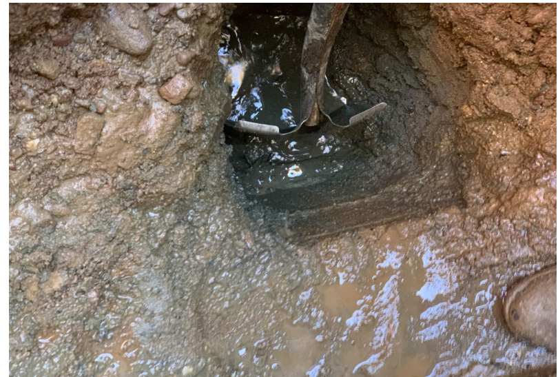
Photo # 4: Hand dug to expose 20-inch deep footing and no perimeter drain.
