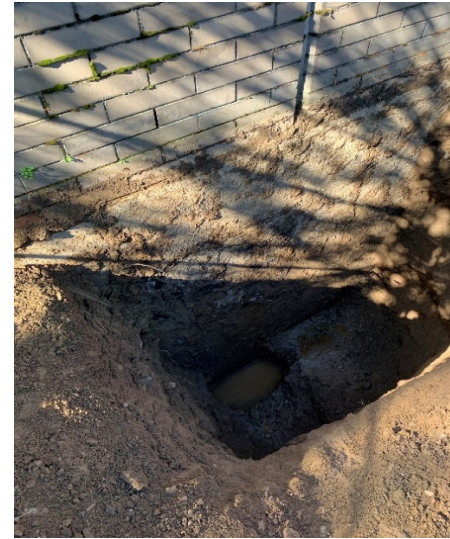
Photo # 3: Compromised water proofing and groundwater over footing.
