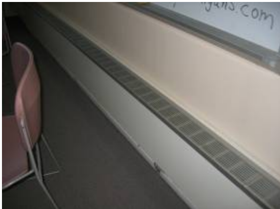
Photo #45: View of fin tube radiators.
