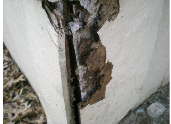
Photo #104: Suspect termite damage at north modular addition
