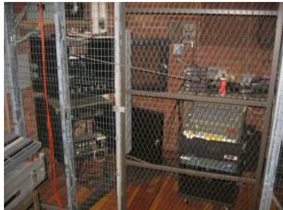
Photo #64: View of sound and lighting control equipment.
