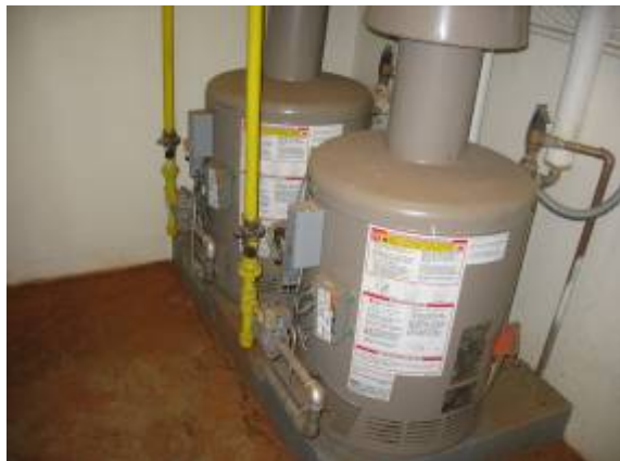
Photo #48: View of domestic hot water heaters.
