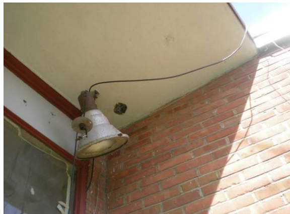
Photo #102: Damaged security light
