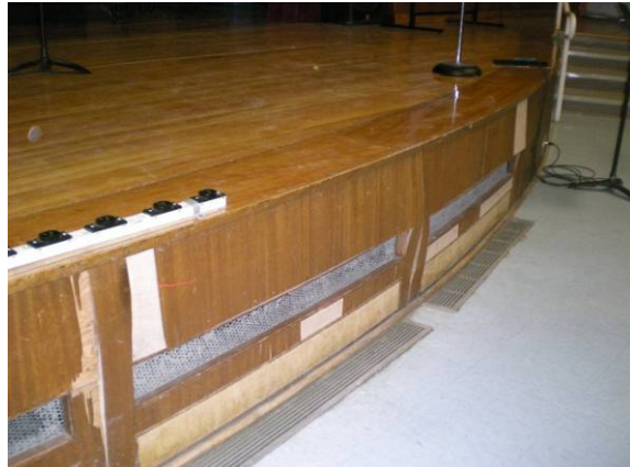
Photo #112: Condition of thin veneer wood panels in Auditorium stage
