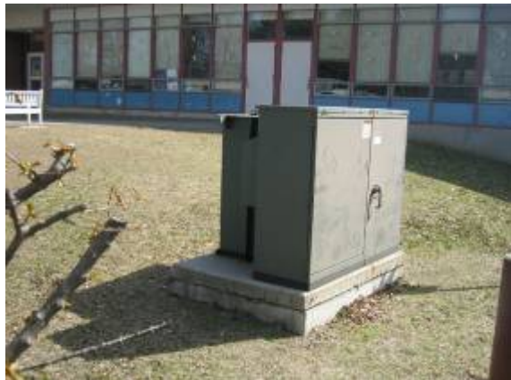
Photo #46: View of pad mounted electrical transformer.
