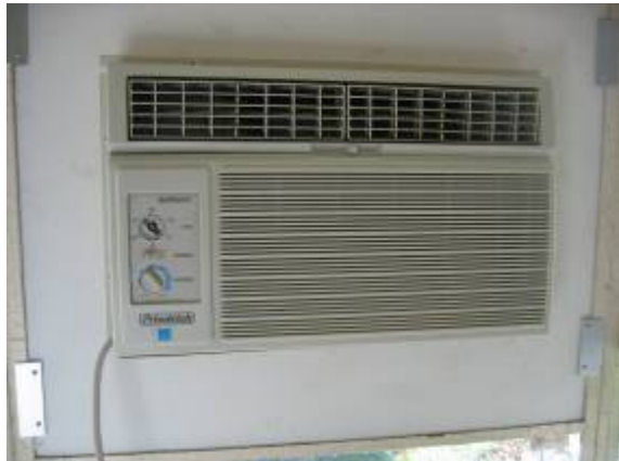
Photo #42: View of window mounted air conditioning unit.
