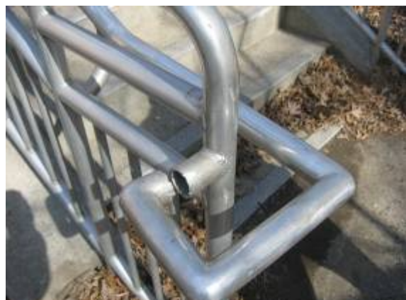
Photo #12: View of damaged handrails on stairs at the end of the 200 corridor.
