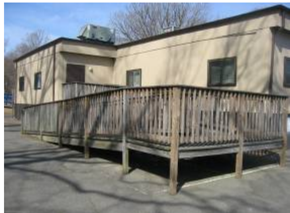
Photo #6: View of wood framed ramp, which is located at the end of the 100 corridor.
