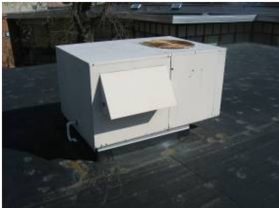
Photo #39: View of RTU 100-3.
