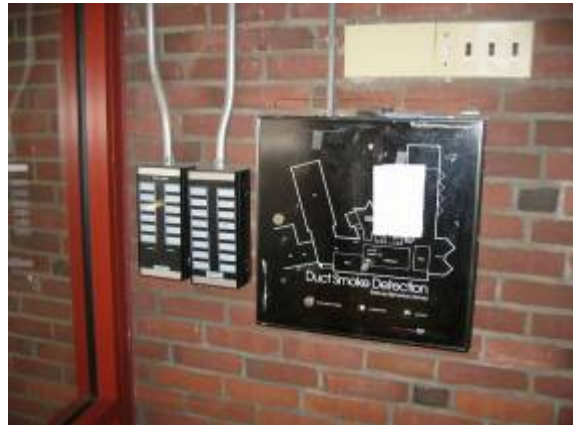
Photo #62: View of fire annunciator panel.
