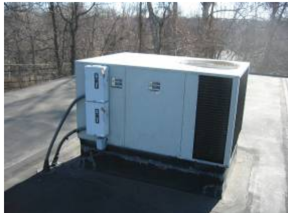
Photo #34: View of RTU 500-3.
