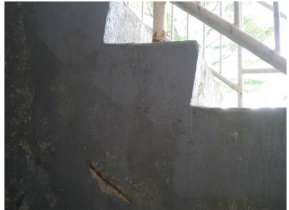
Photo #108: Railing and stair condition at loading dock
