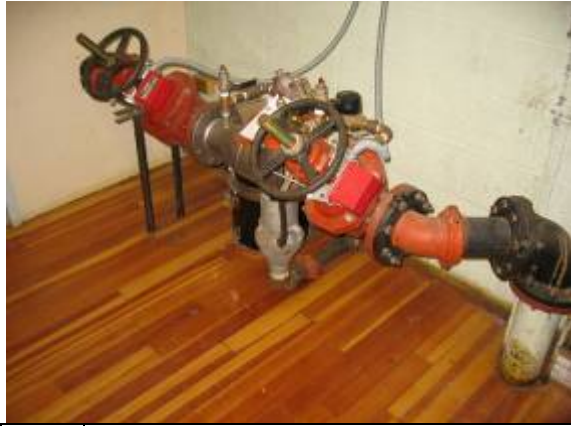
Photo #50: View of water metering equipment.
