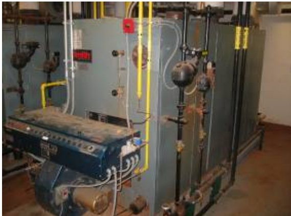
Photo #23: View of Boiler No.1.
