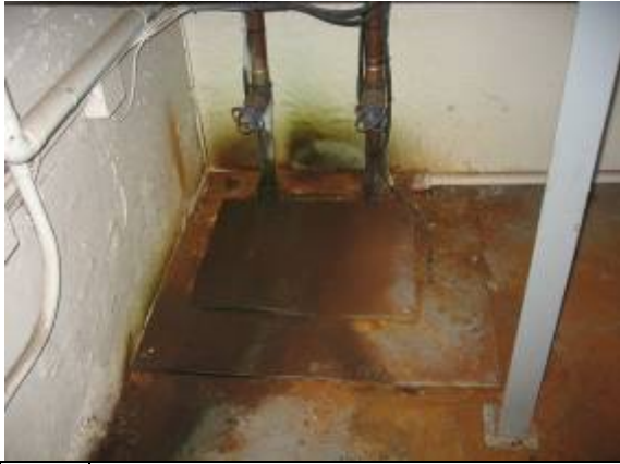
Photo #49: View of sump pump.
