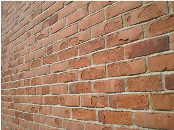
Photo #105: Soft brick at 500 wing
