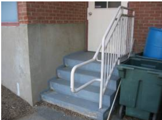
Photo #9: View of cast in place concrete steps, which are located at the receiving dock.
