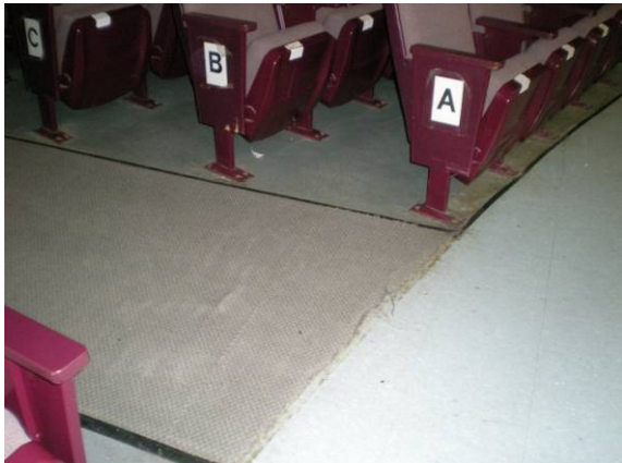
Photo #113: Condition of carpet at auditorium
