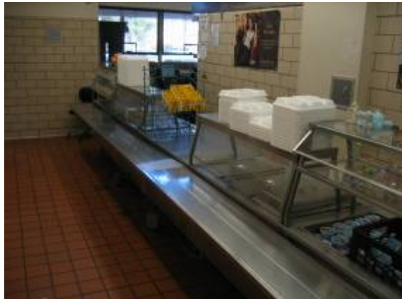
Photo #56: View of commercial kitchen equipment.
