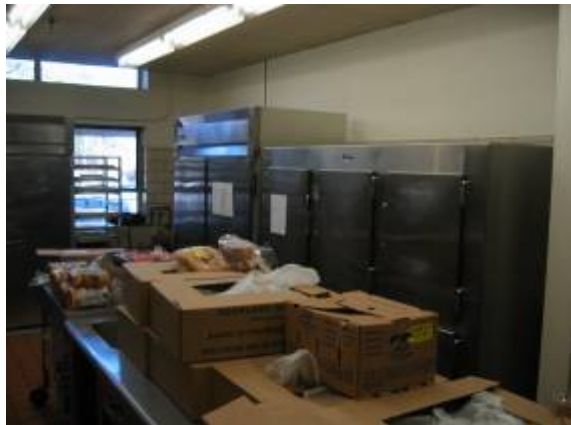
Photo #58: View of commercial kitchen equipment.
