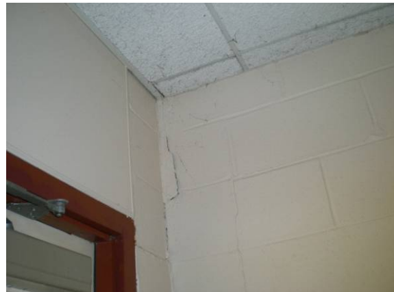
Photo #124: Settlement cracking in corridor at far northwest corner
