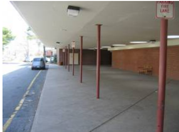
Photo #14: View of concrete paved sidewalks, which are located at the main entrance.
