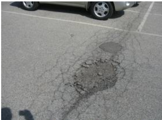
Photo #17: View of deteriorated asphalt pavement.
