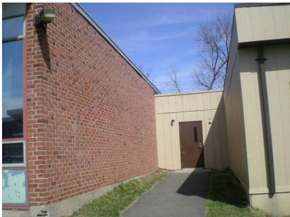
Photo #77: Link between 500 wing and north end modular addition note damaged corner
