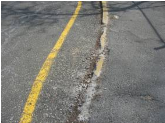
Photo #15: View of deteriorated concrete curbing along the main entry drive.
