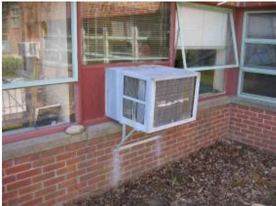
Photo #43: View of window mounted air conditioning unit.
