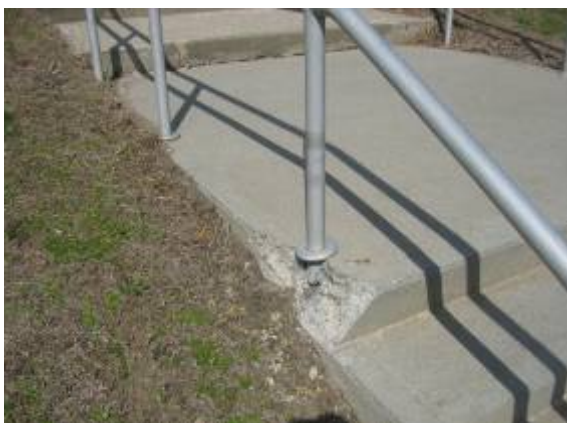
Photo #11: View of damaged handrail connection on stairs at the end of the 400 corridor.
