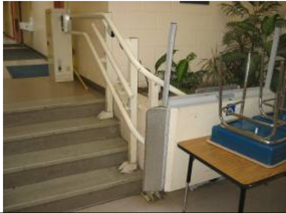
Photo #52: View of wheel chair lift, which is located within the 300/500 corridors.
