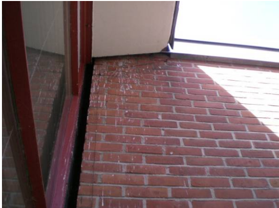
Photo #99: Gap at junction between 200 wing and main office section – evidence of birds
