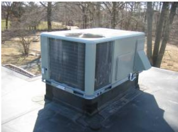
Photo #35: View of RTU 100-7.
