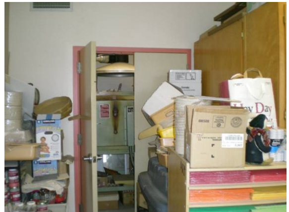
Photo #136: Kiln in art room – non-functional
