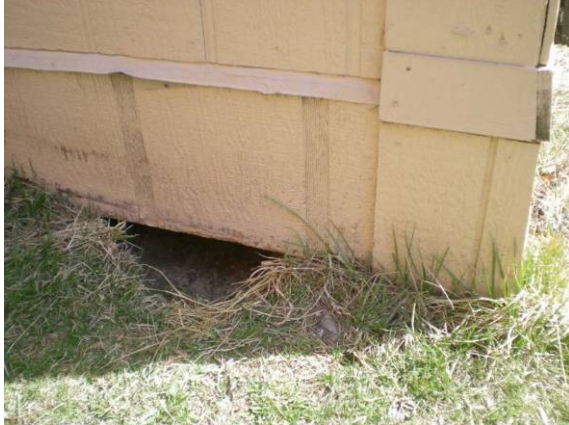
Photo #103: Evidence of burrowing animals under north modular addition
