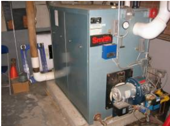
Photo #25: View of Boiler No.3.
