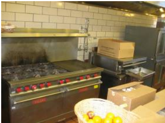
Photo #57: View of commercial kitchen equipment.
