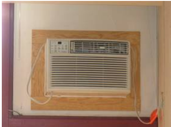
Photo #44: View of window mounted air conditioning unit.
