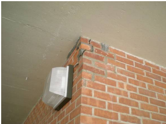
Photo #93: Dislodged brick veneer near from entrance
