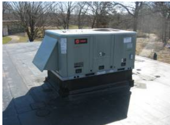
Photo #36: View of RTU 100-6.
