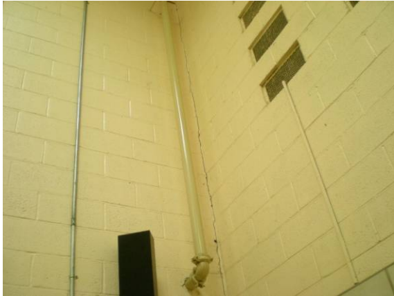
Photo #133: Settlement crack in cafeteria
