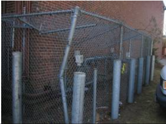
Photo #51: View of natural gas metering equipment.
