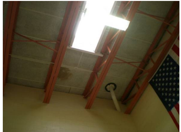
Photo #132: Reportedly inactive roof leak in cafeteria
