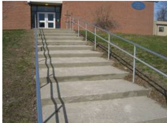
Photo #8: View of cast in place concrete steps, which are located at the end of the 400 corridor.
