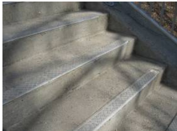
Photo #10: View of cast in place concrete steps at the end of the 200 corridor, whose metal tread noses are becoming dislodged.
