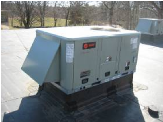
Photo #37: View of RTU 100-5.
