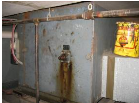
Photo #30: View of make-up air unit, which serves the cafeteria.
