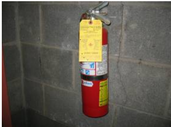
Photo #63: View of fire extinguisher.
