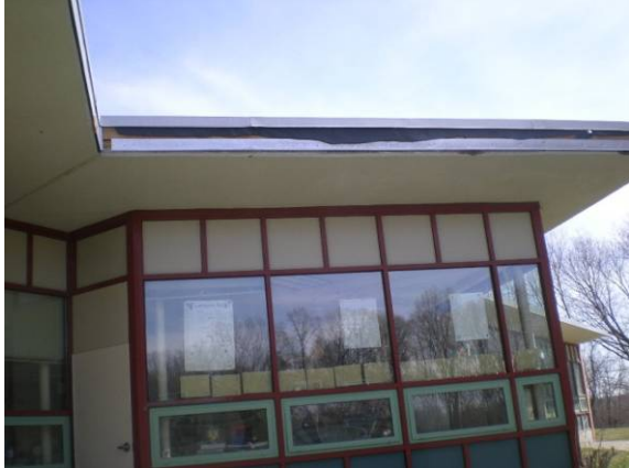
Photo #97: Missing fascia panels
