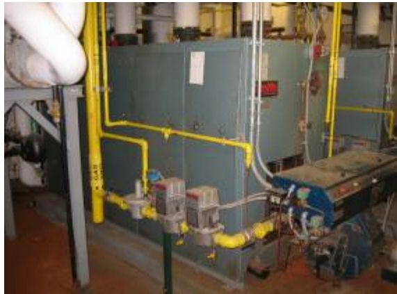
Photo #24: View of Boiler No.2.
