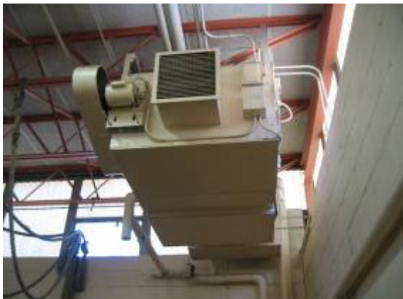
Photo #29: View of make-up air unit, which is located in small gymnasium.
