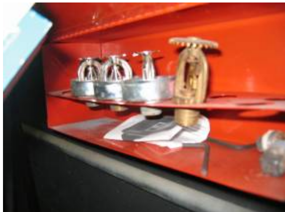
Photo #60: View of spare sprinkler heads.
