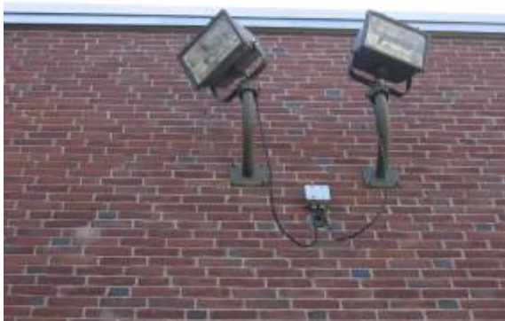
Photo #3: View of building mounted site lighting fixtures.
