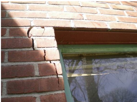
Photo #101: Settlement cracking at brick veneer
