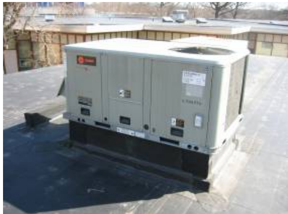
Photo #40: View of RTU 100-2.
