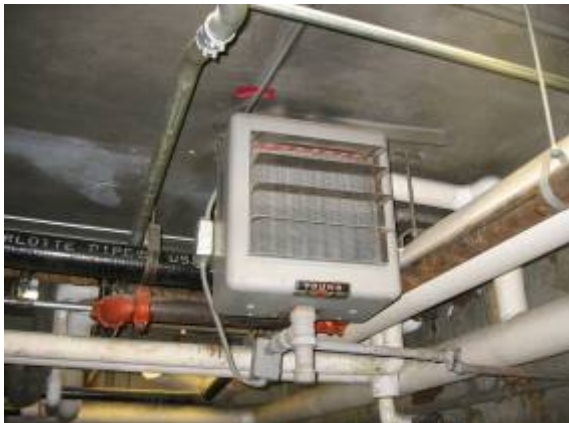
Photo #27: View of auxiliary heaters.
