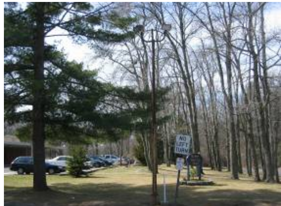
Photo #4: View of pole mounted site lighting fixtures.
