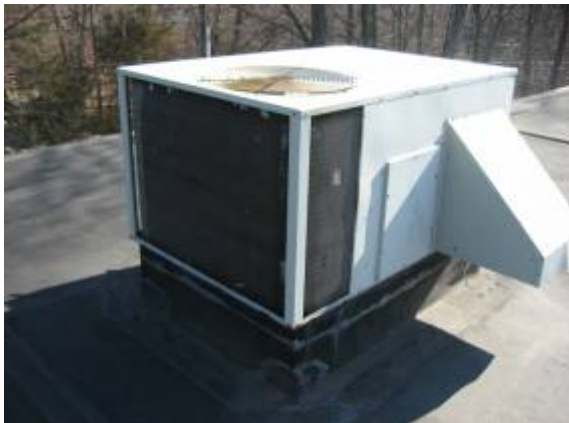
Photo #33: View of RTU 500-2.
