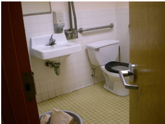
Photo #125: ADA restroom at junction between K classroom and south modular wing
