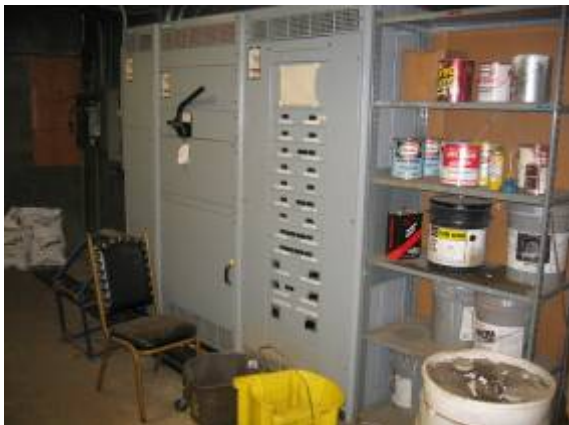
Photo #47: View of main electrical switchgear.
