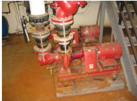
Photo #26: View of hot steam distribution pumps.
