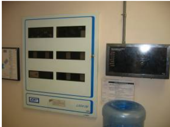
Photo #61: View of fire control panel.
