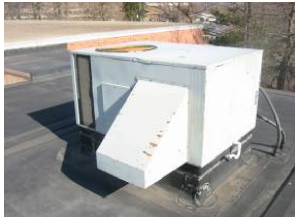
Photo #32: View of RTU 500-1.
