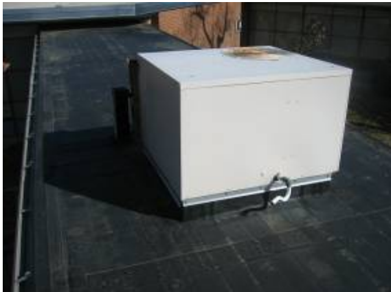
Photo #41: View of RTU 100-1.
