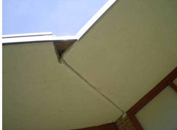
Photo #98: Spalled concrete soffit panel
