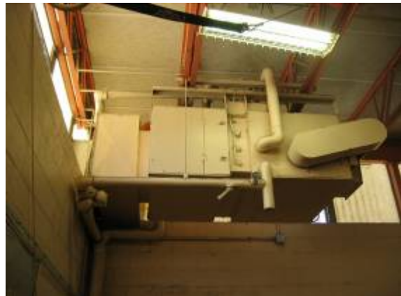
Photo #28: View of make-up air unit, which is located in small gymnasium.
