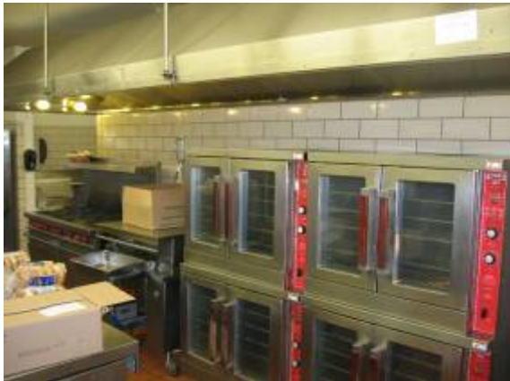
Photo #55: View of commercial kitchen equipment.
