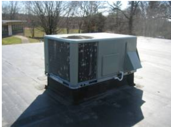
Photo #38: View of RTU 100-4.
