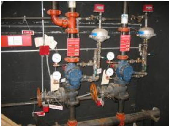
Photo #59: View of main sprinkler valves.
