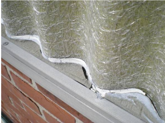
Photo #91: Common condition at gym clerestory – broken seals
