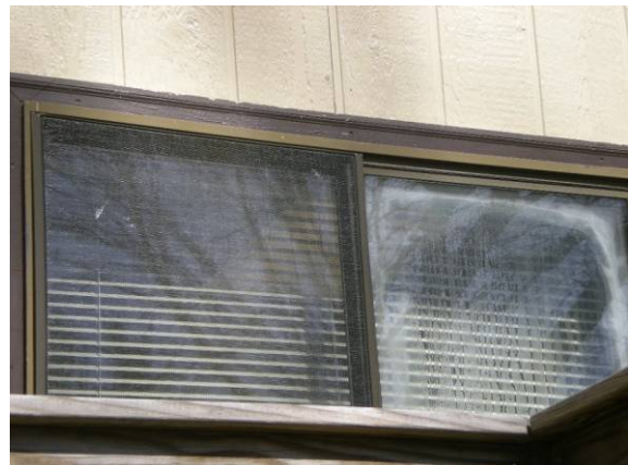
Photo #96: Broken seals at windows on south modular addition
