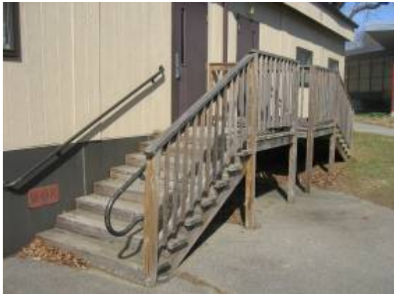
Photo #7: View of wood framed steps, which are provided at a majority of the modular classrooms.
