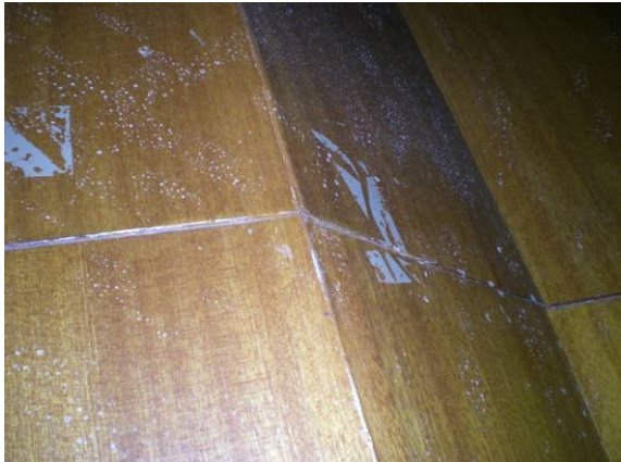
Photo #111: Condition of thin veneer wood panels in Auditorium
