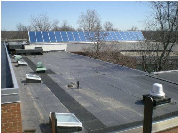
Photo #83: Roof over main office area and view of Media Center skylight
