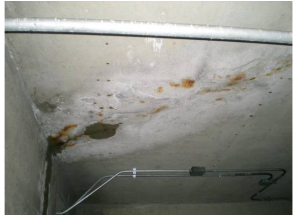
Photo #106: Crack and water infiltration of raised concrete landing at basement access
