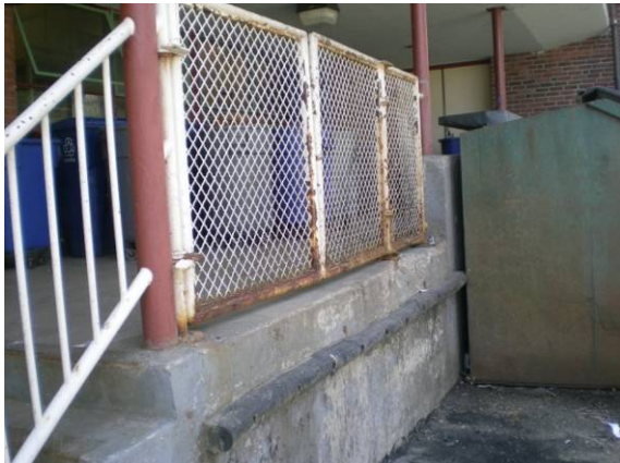
Photo #107: Loading dock gate and bumper condition
