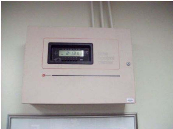
Photo #129: Security interface panel
