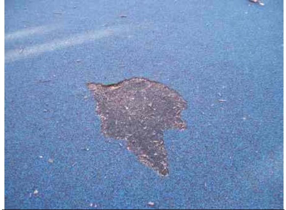
Photo #44: Damage to rubber playground surface
