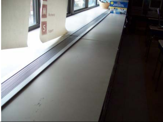
Photo #103: Perimeter finned-tube heating unit for classroom
