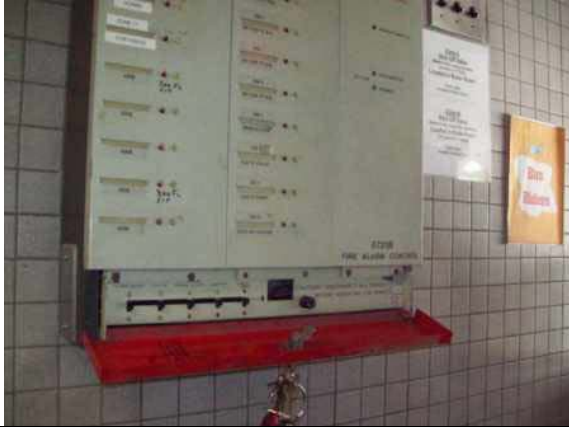
Photo #127: Fire alarm annunciator panel
