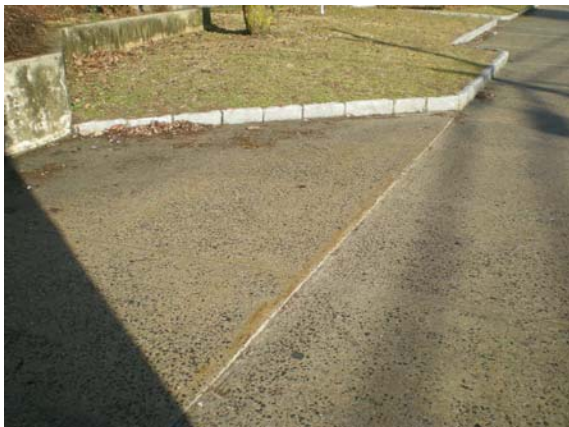
Photo #41: Tripping hazard near main entrance
