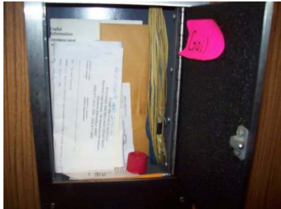
Photo #124: Missing elevator communication equipment
