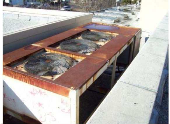
Photo #98: Air-cooled condensing unit for AC-5
