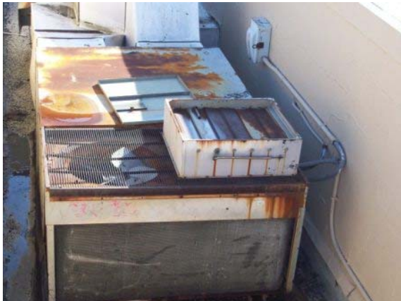
Photo #99: Packaged rooftop unit (AC-6)
