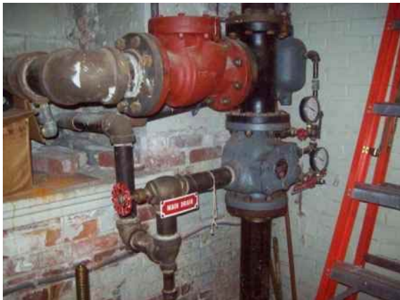
Photo #131: Fire sprinkler riser
