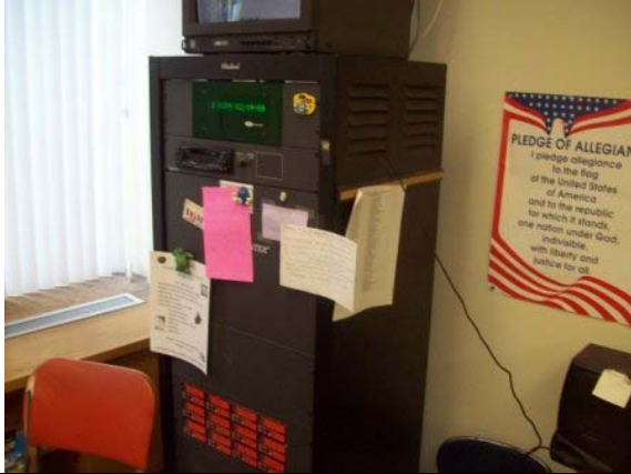
Photo #133: PA system control unit
