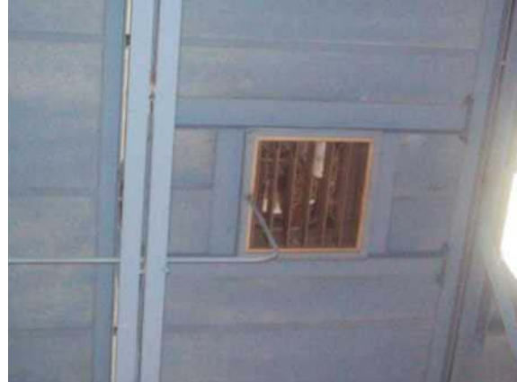
Photo #110: Exhaust fan for gymnasium (1 of 2)
