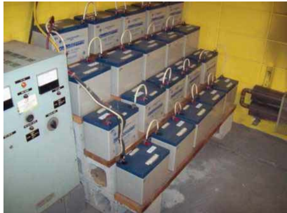
Photo #118: Emergency battery back-up system
