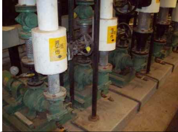
Photo #86: Hot water circulating pumps
