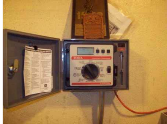
Photo #50: Irrigation controls for soccer field
