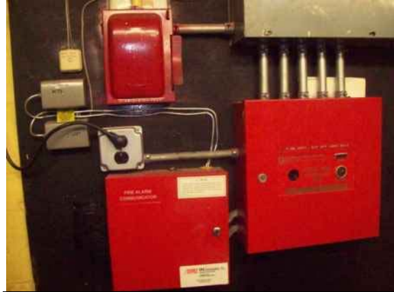
Photo #128: Fire alarm communicator panel
