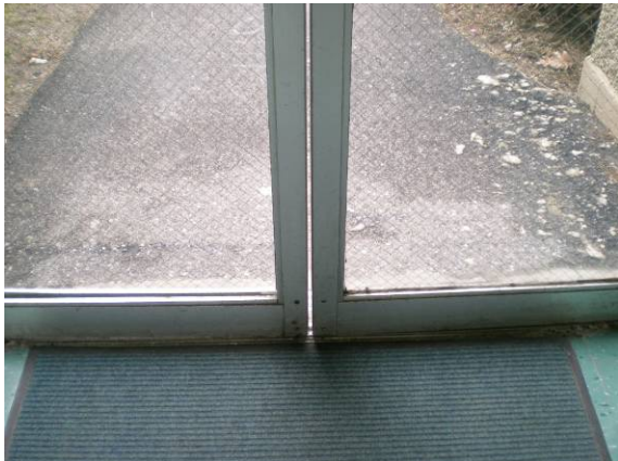
Photo #71: No weather stripping at door
