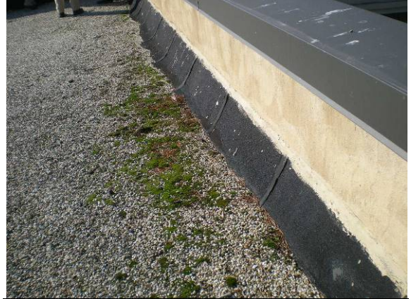
Photo #32: Moss build up
