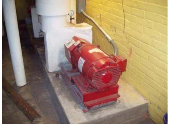
Photo #92: Chiller water circulating pump
