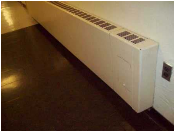
Photo #107: Wall-mounted finned-tube heating unit for corridor
