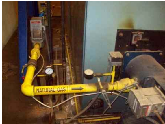
Photo #115: Natural gas distribution in boiler room
