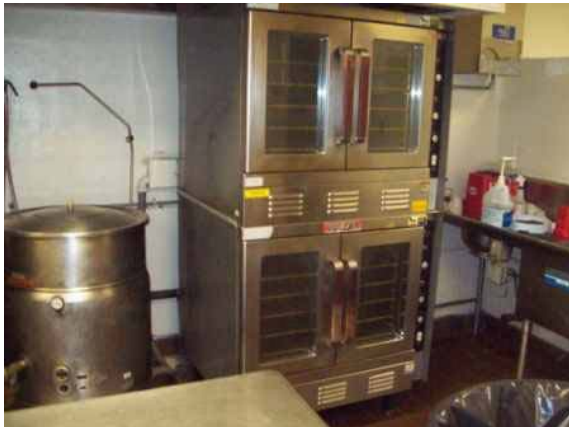
Photo #135: Convection ovens and steamer in kitchen
