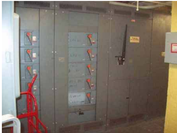
Photo #117: Electrical switchgear
