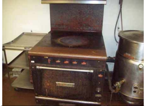
Photo #134: Gas range in kitchen
