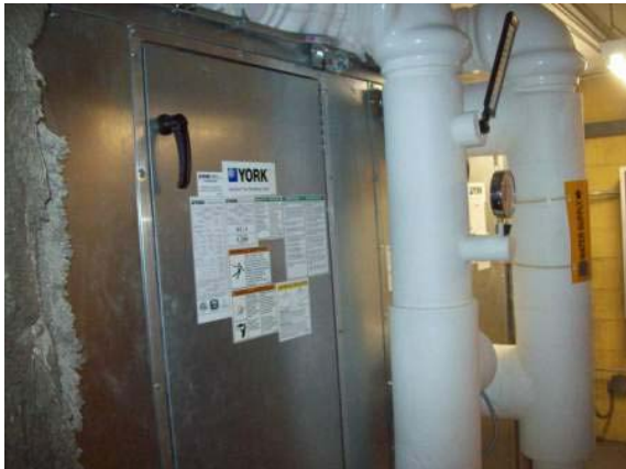
Photo #93: Air handling unit (AC-1)
