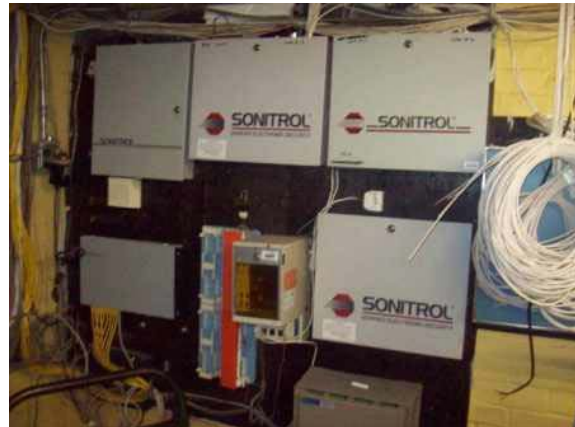
Photo #130: Security control panel
