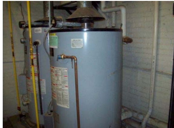
Photo #112: Domestic water heaters
