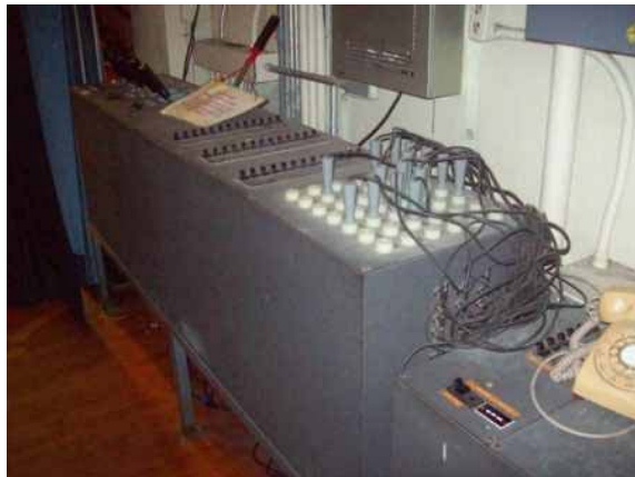
Photo #119: Auditorium lighting controls
