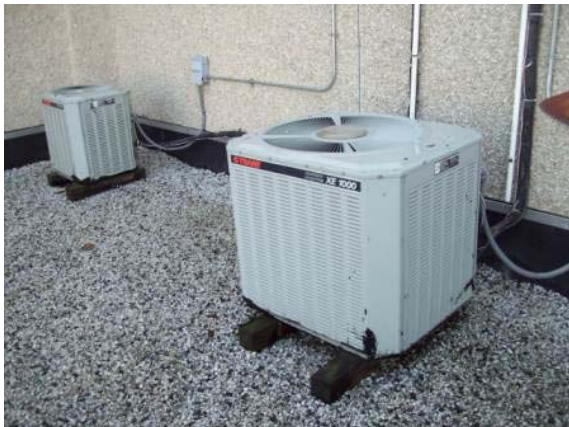
Photo #101: Split system condensing units for media center computer rooms
