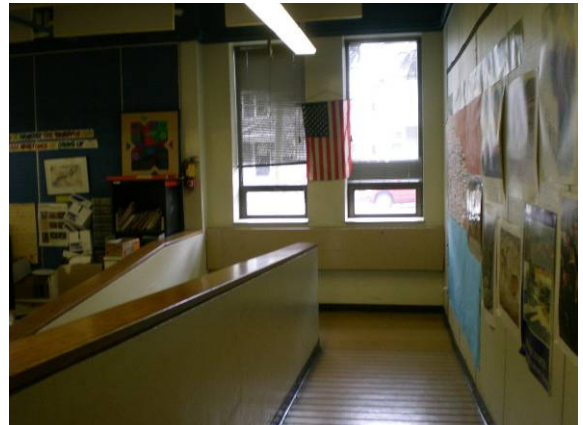
Photo #72: Ramp access to art rooms – no railings
