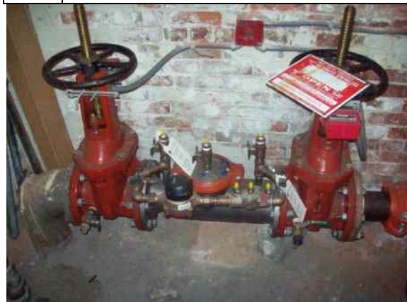
Photo #132: Fire sprinkler backflow preventer
