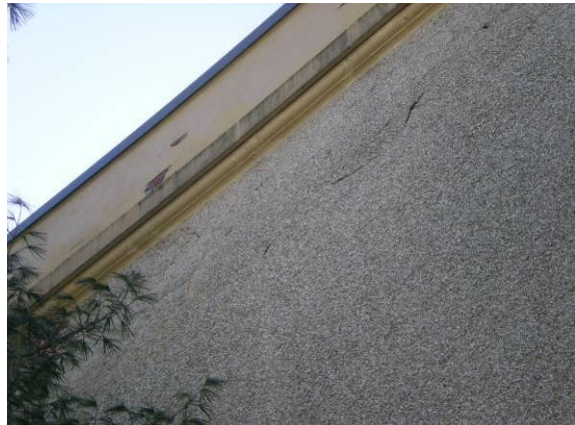
Photo #24: Spalling at cornice and peeling of heavy skim coat
