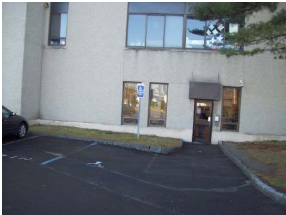
Photo #51: Area of drainage issue in north parking lot
