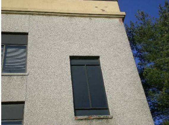
Photo #25: Spalling of heavy skim coat at window sill, elevation and cornice
