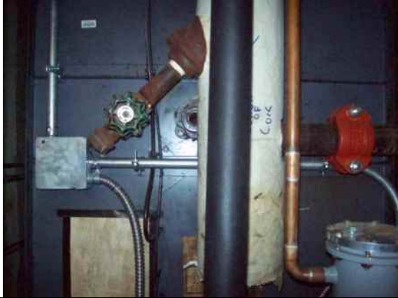
Photo #97: Air handling unit (AC-5)
