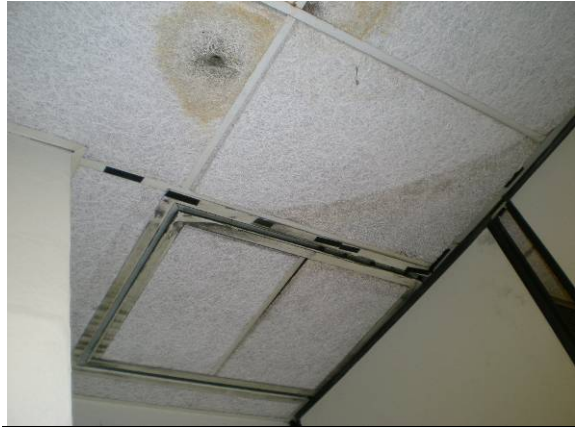
Photo #74: Suspect mold at ceiling in room off cafeteria
