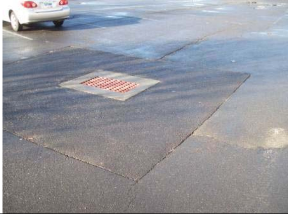
Photo #38: Catch basin for municipal storm drainage
