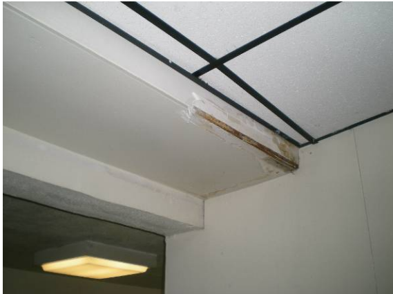
Photo #81: Roof leak at juncture between building and modular wing
