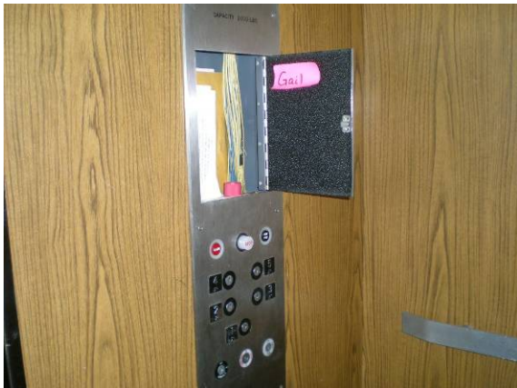
Photo #57: Elevator with no emergency communication
