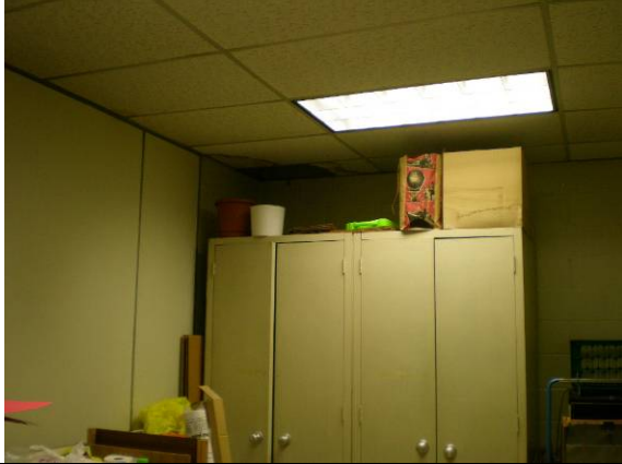
Photo #67: Roof leak off storage area off classroom B1
