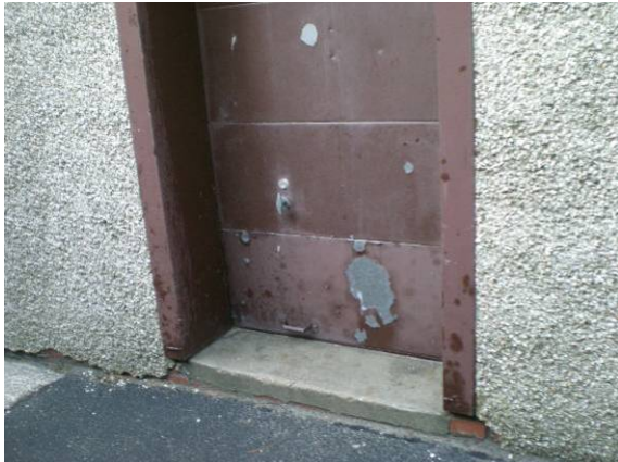
Photo #21: Condition of small roll up door
