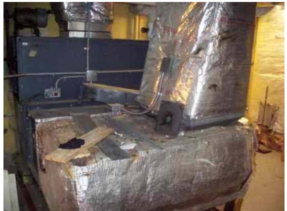
Photo #96: Air handling unit (AC-4)
