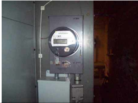
Photo #116: Electric meter
