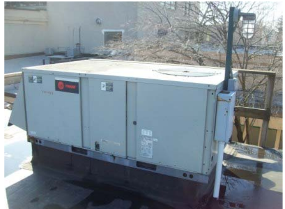
Photo #100: Packaged rooftop unit for modular classroom (1 of 2)
