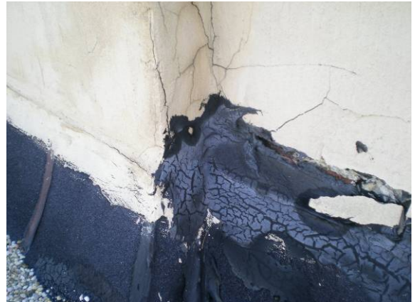
Photo #34: Cracked roofing compound and coating at parapet
