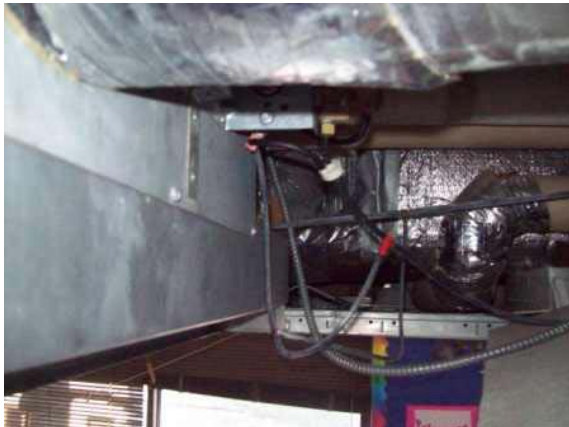
Photo #105: Air distribution for classroom air conditioning
