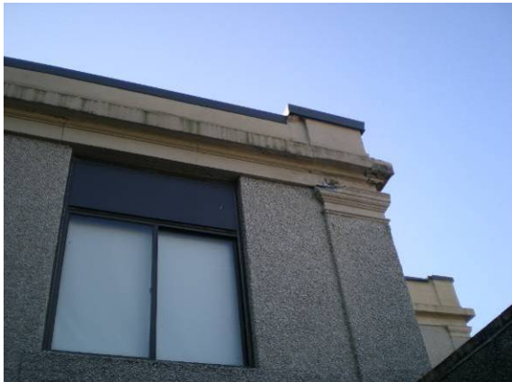
Photo #23: Spalling at cornice
