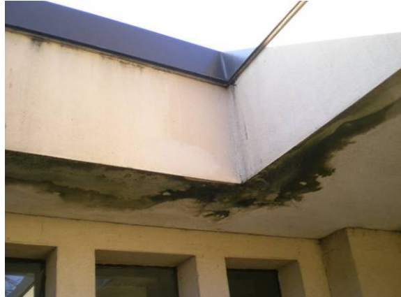
Photo #20: Mildew on soffit at north facing corridor elevation
