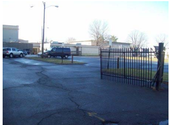
Photo #48: Damaged gate at north entrance
