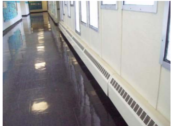
Photo #106: Baseboard finned-tube heating units in corridor
