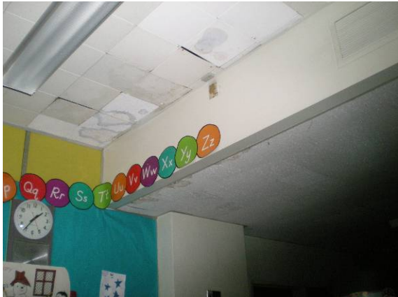
Photo #69: Evidence of leaks
