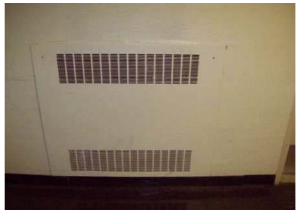
Photo #108: Recessed convection unit for restroom
