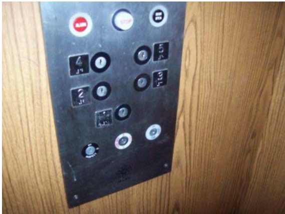
Photo #123: Elevator control panel
