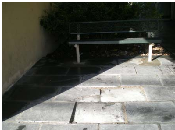
Photo #42: Tripping hazard near main entrance
