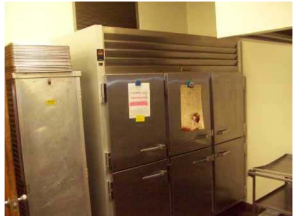
Photo #136: Refrigeration units in kitchen
