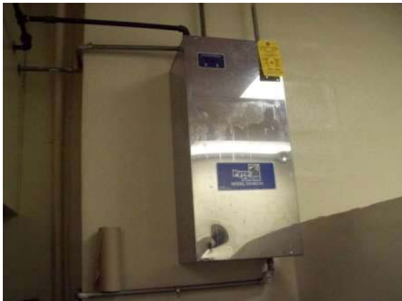
Photo #137: Dry chemical fire protection system in kitchen
