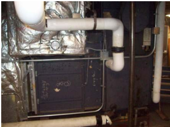
Photo #95: Air handling unit (AC-3)
