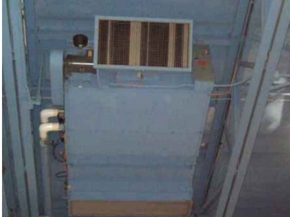
Photo #109: Make-up air unit for gymnasium (1 of 4)
