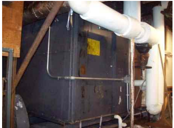
Photo #94: Air handling unit (AC-2)
