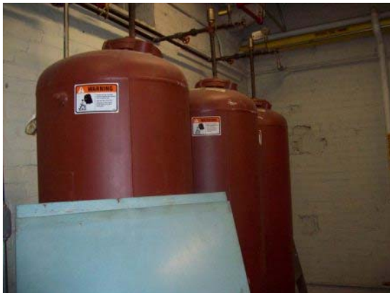
Photo #89: Hot water loop expansion tanks
