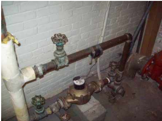
Photo #111: Domestic water meter
