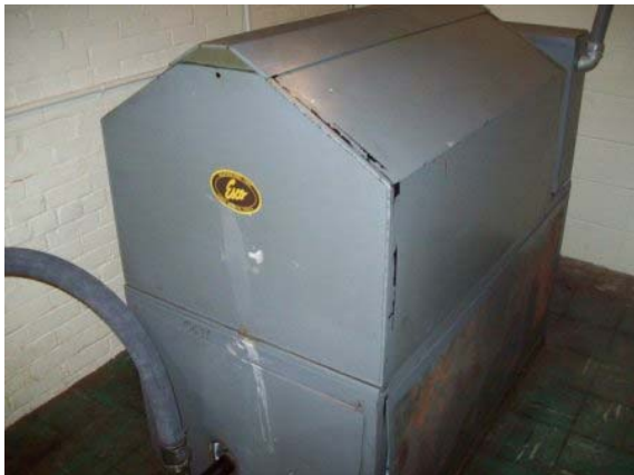
Photo #125: Hydraulic elevator equipment
