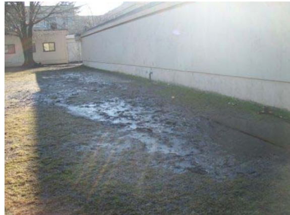
Photo #52: Ponding at adjacent to building near building at soccer field
