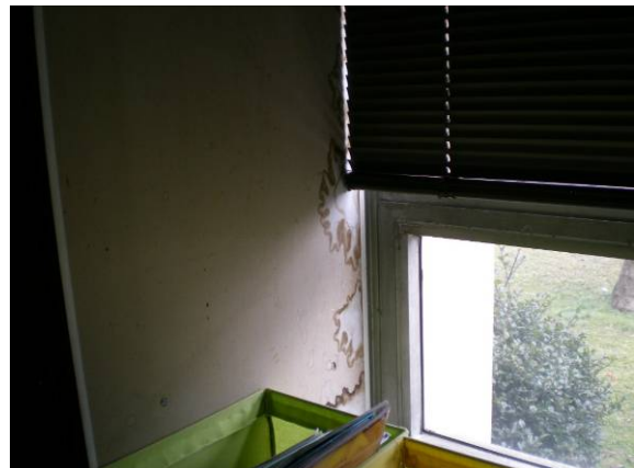
Photo #66: Evidence of water staining due to broken window sealant
