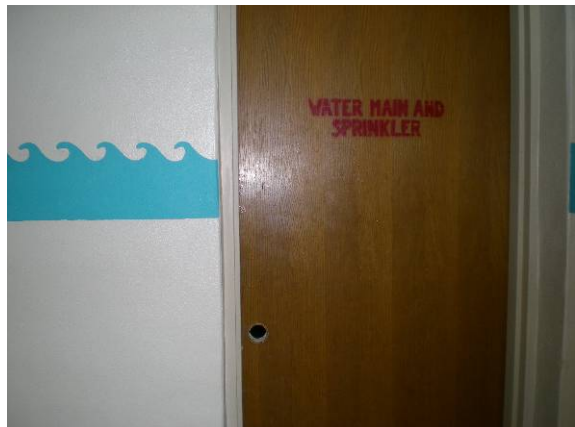
Photo #78: Life safety issue – missing door hardware at sprinkler room
