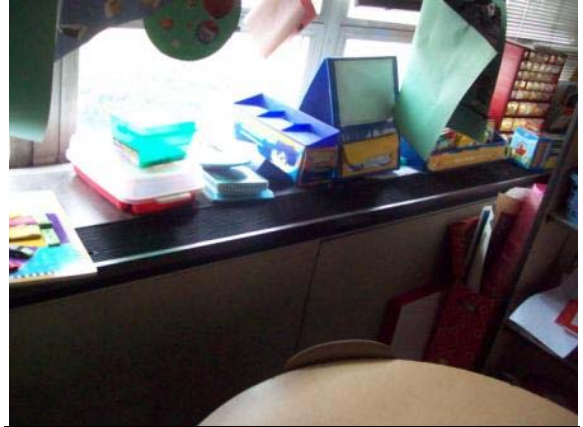
Photo #104: Unit ventilator for classroom
