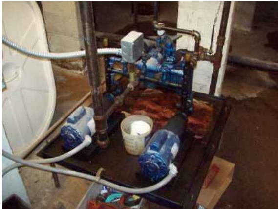
Photo #87: Fuel oil pump set
