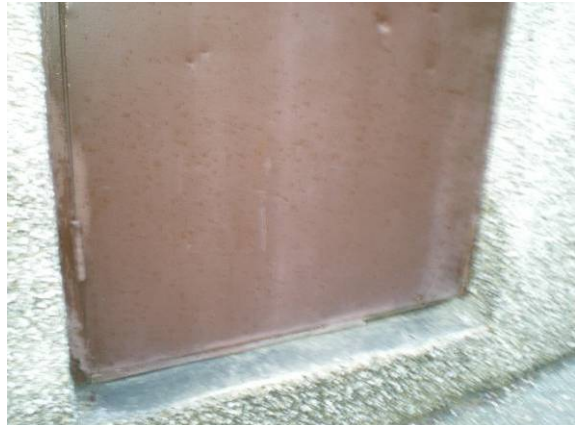
Photo #22: Service door condition
