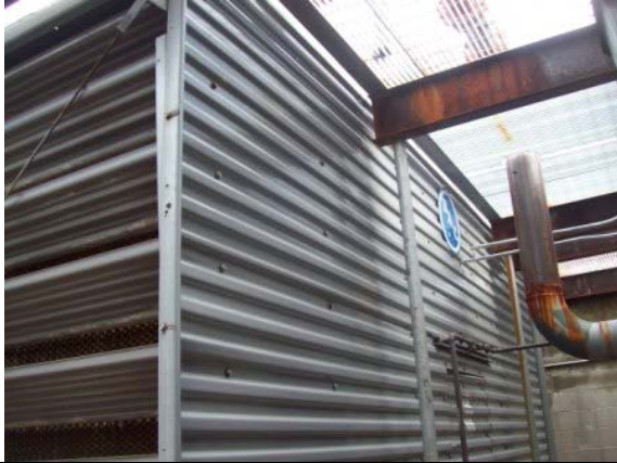
Photo #91: Cooling tower
