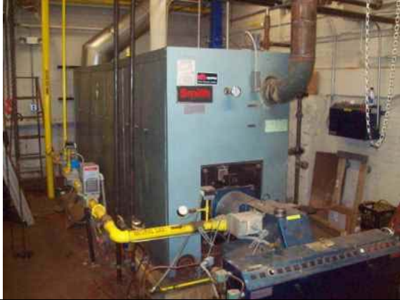
Photo #85: Boiler (1 of 3)
