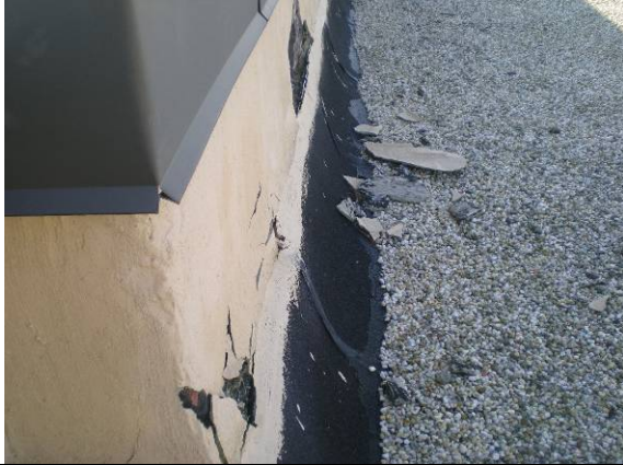
Photo #31: Spalling at parapet
