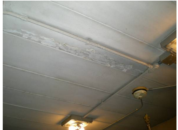
Photo #82: Leaking evidence at area north of gymnasium
