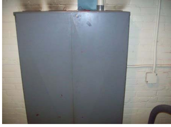
Photo #126: Elevator control unit
