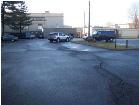
Photo #39: Alligator cracking in north parking lot
