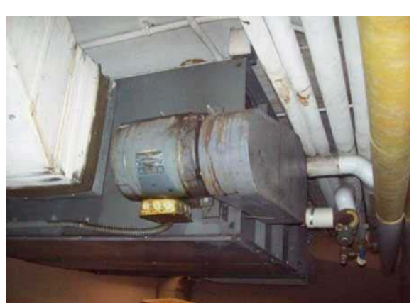
Photo #102: Fan coil unit for gym offices
