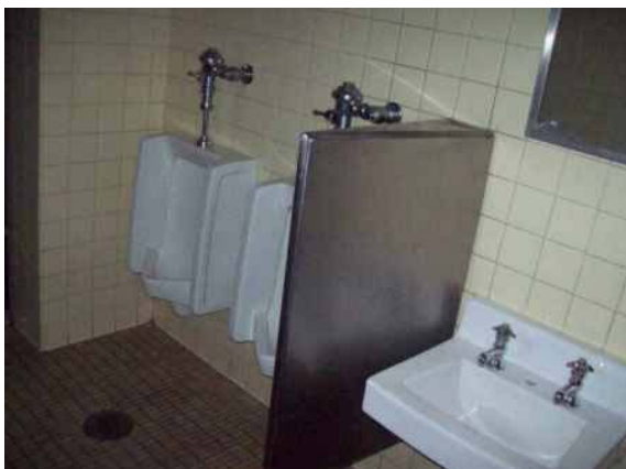
Photo #113: Typical lavatory and urinal plumbing fixtures
