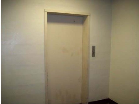
Photo #121: Elevator cab door
