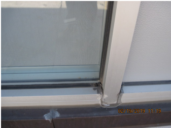
Possible non-roof sources of water infiltration
