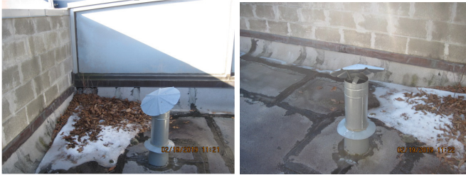
Broken vent caps
