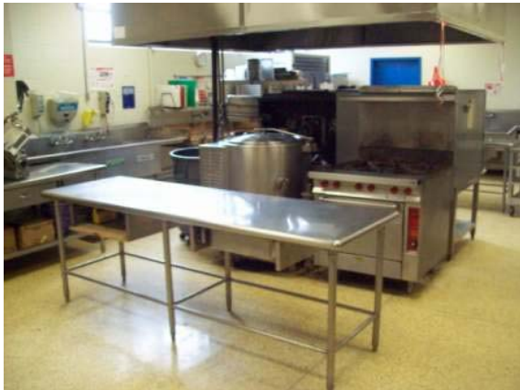
Photo #117: Kitchen equipment
