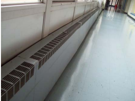
Photo #85: Typical finned-tube radiant heat unit
