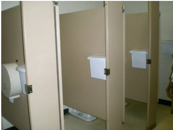
Photo #57: Common restroom
