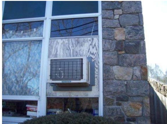
Photo #90: Typical window air conditioning unit
