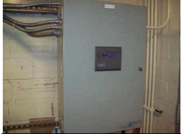
Photo #80: Boiler control unit
