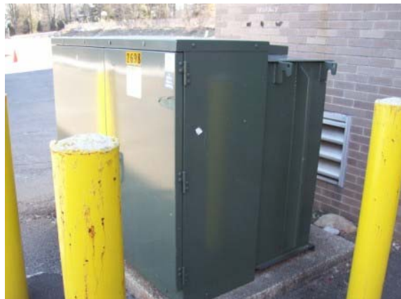
Photo #102: Electrical transformer
