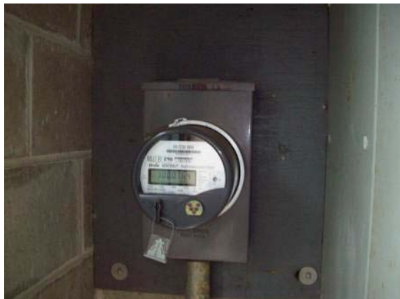
Photo #101: Electric meter
