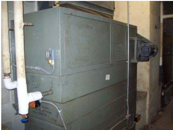
Photo #87: Air handling unit (1 of 3)
