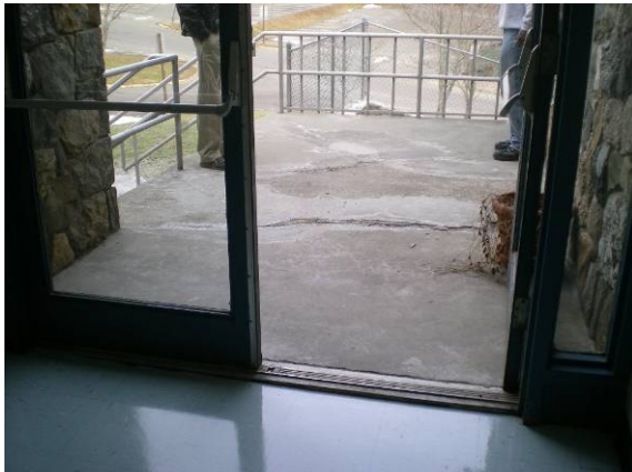
Photo #23: Side entrance with low guardrail and cracked landing
