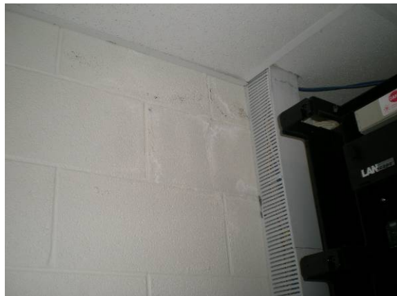
Photo #66: Suspect mold in Media Center server room
