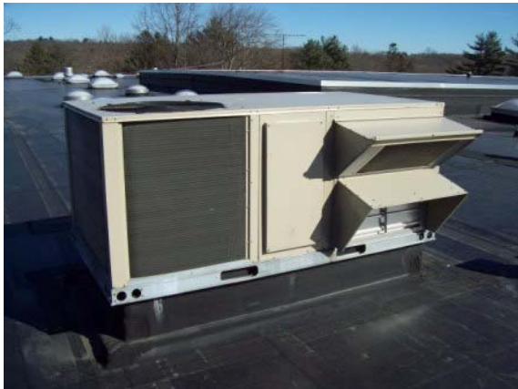
Photo #89: Typical rooftop unit
