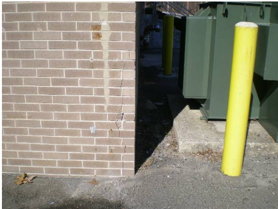
Photo #75: Cracking at southeast corner near transformer
