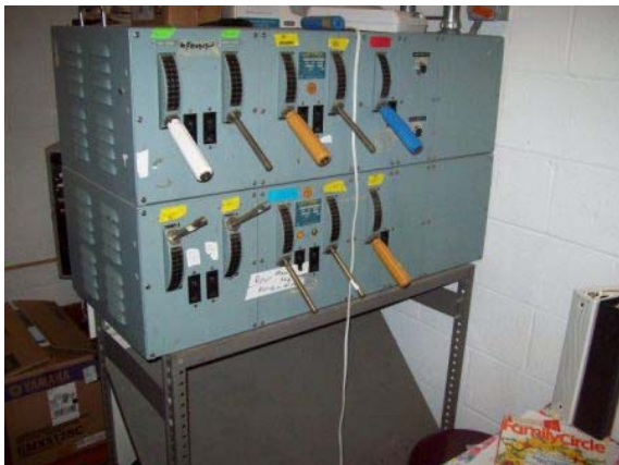
Photo #107: Lighting controls for auditorium
