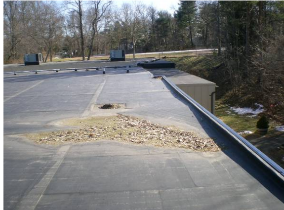
Photo #20: Evidence of ponding on original school building
