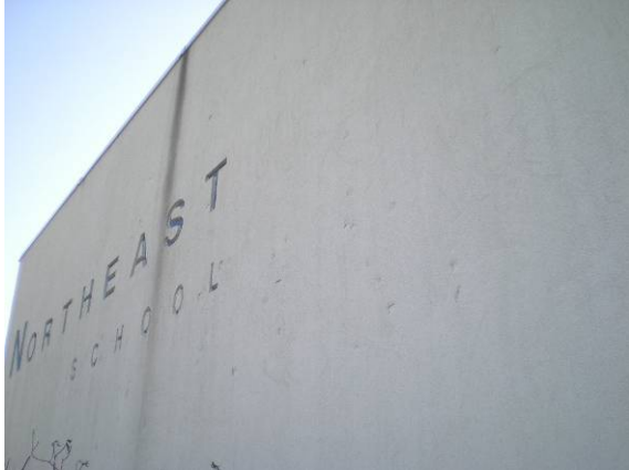
Photo #55: Damage to EIFS at Media Center
