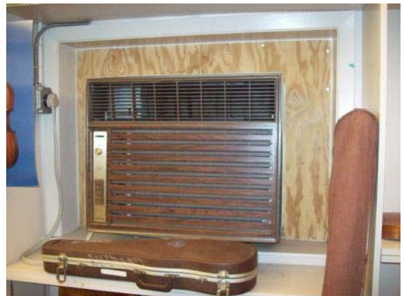
Photo #126: Air conditioning unit for annex building
