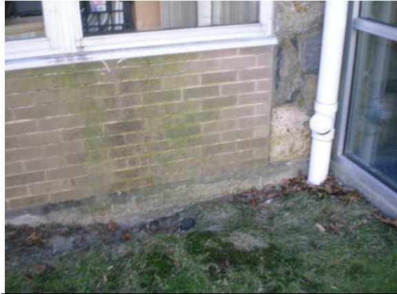
Photo #38: Erosion at front elevation of building
