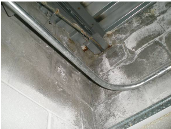
Photo #65: Evidence of roof leak at Media Center storage room
