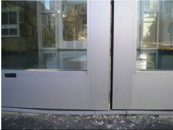
Photo #25: Storefront doors not set properly. Threshold bent from non level substrate
