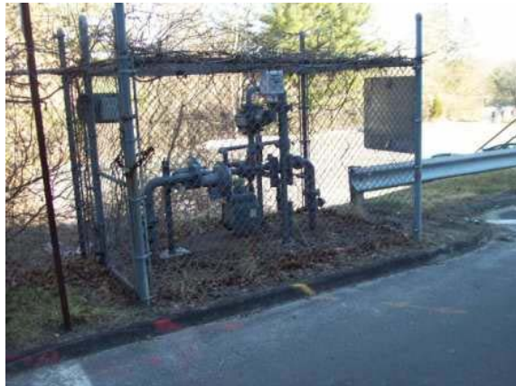
Photo #99: Gas meter and regulator
