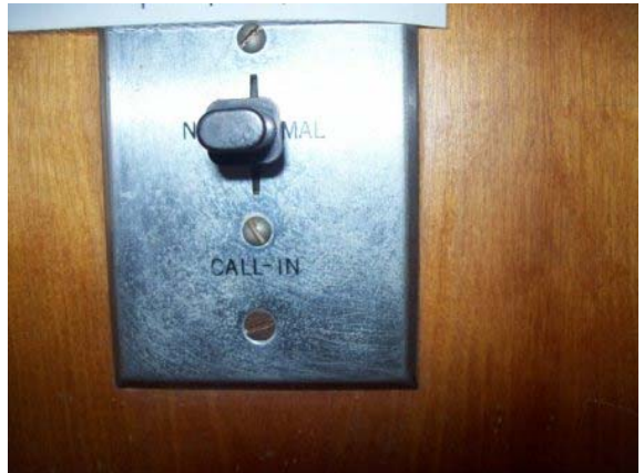
Photo #106: Typical PA call panel in classroom
