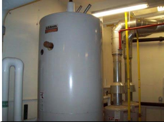
Photo #92: Domestic hot water storage tank
