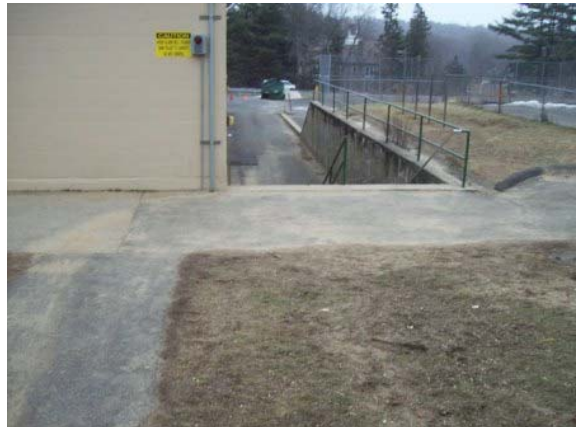
Photo #40: Area of reported drainage problems at south side of building
