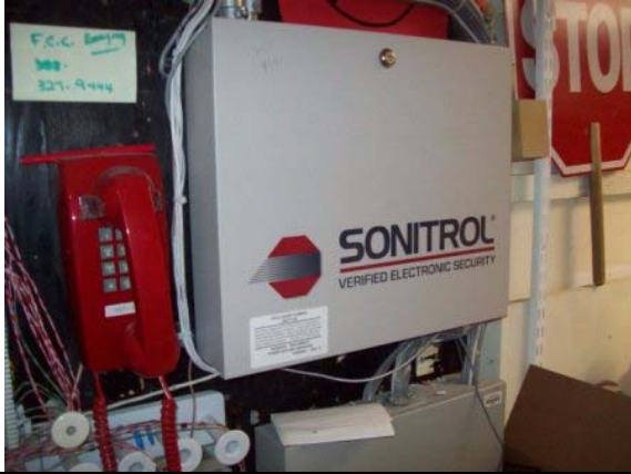
Photo #115: Security panel
