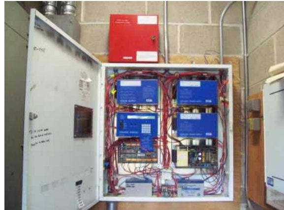
Photo #110: Fire alarm battery panel
