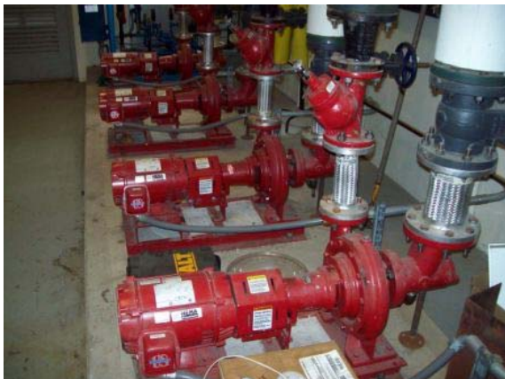
Photo #83: Hot water circulating pumps
