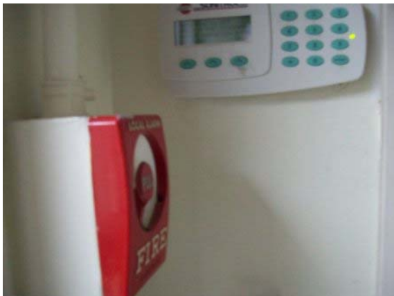
Photo #131: Fire alarm pull station and security key pad for annex building
