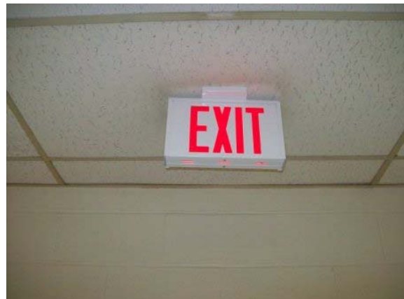
Photo #114: Typical illuminated exit sign
