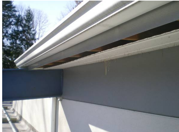
Photo #16: Missing soffit panel at Media Center
