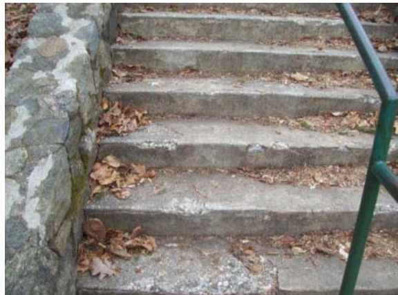
Photo #36: Damage to concrete steps
