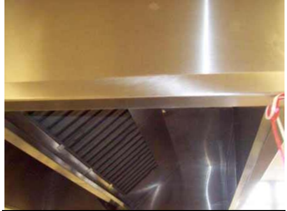
Photo #116: Kitchen exhaust hood without fire protection
