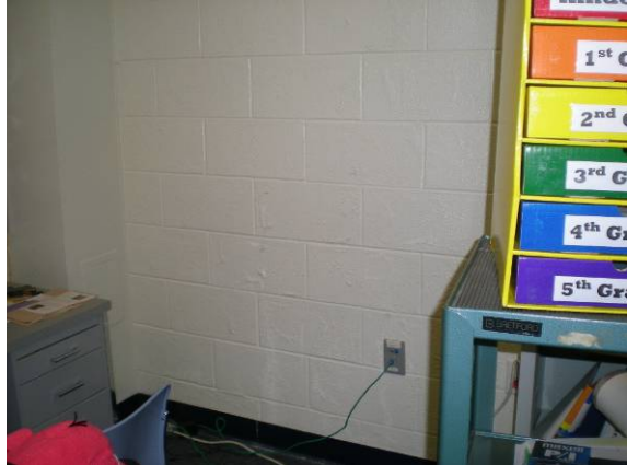
Photo #67: Water infiltration at Media Center office
