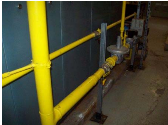
Photo #100: Gas lines in boiler room
