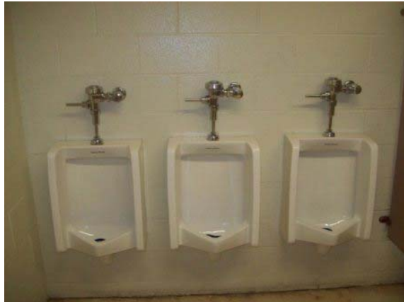
Photo #97: Typical urinal fixtures
