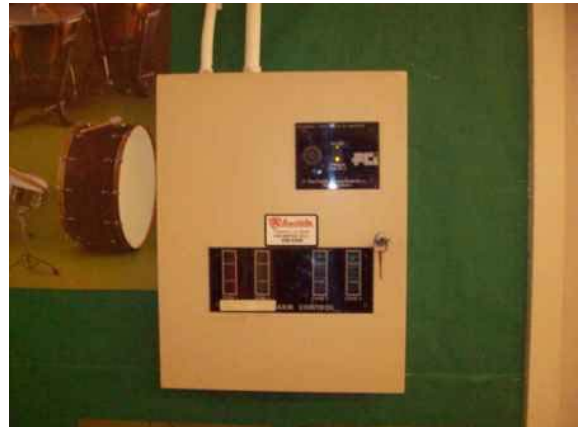
Photo #130: Fire alarm annunciator panel for annex building
