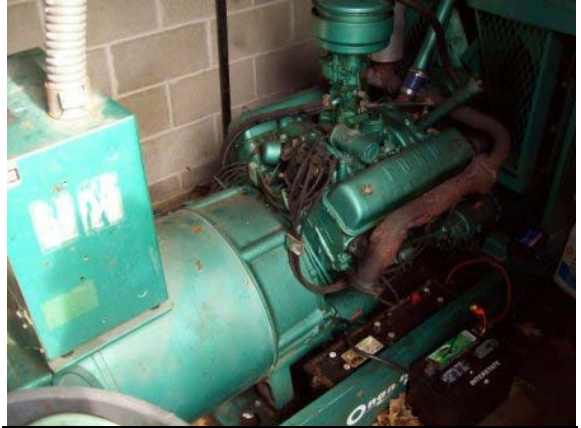
Photo #104: Emergency generator
