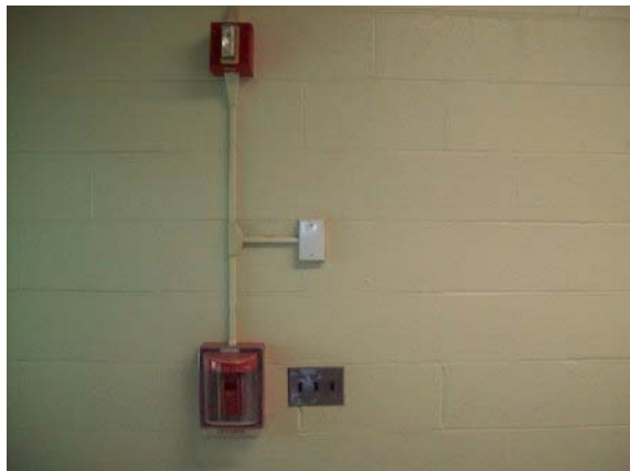
Photo #113: Fire alarm pull station and alarm horn with strobe light
