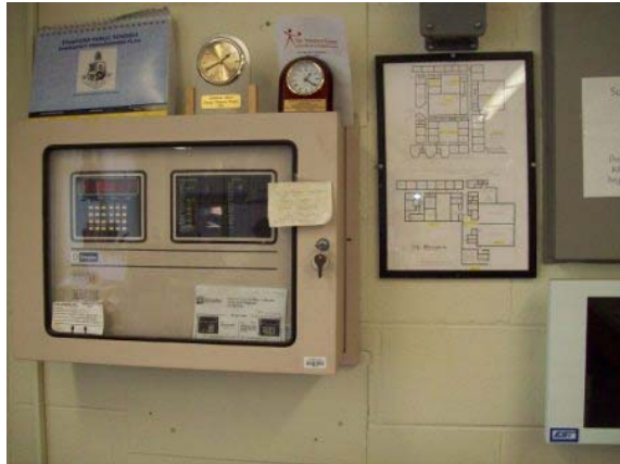
Photo #109: Fire alarm annunciator panel
