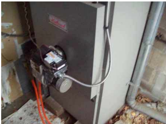
Photo #125: Furnace for annex building
