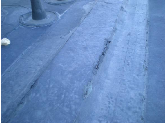
Photo #19: Cracking at single ply membrane over modular section
