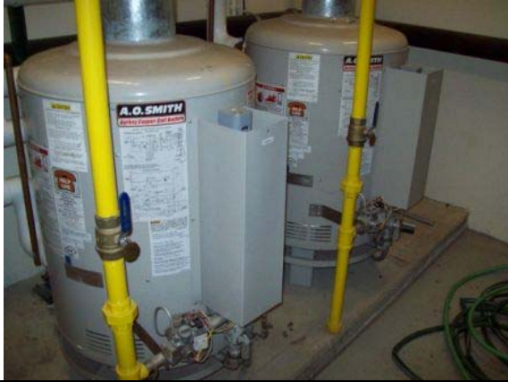
Photo #91: Domestic water boilers
