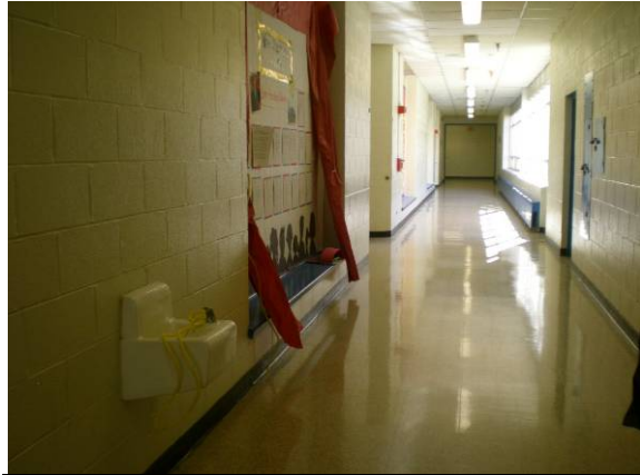
Photo #50: Corridor with protruding drinking fountain
