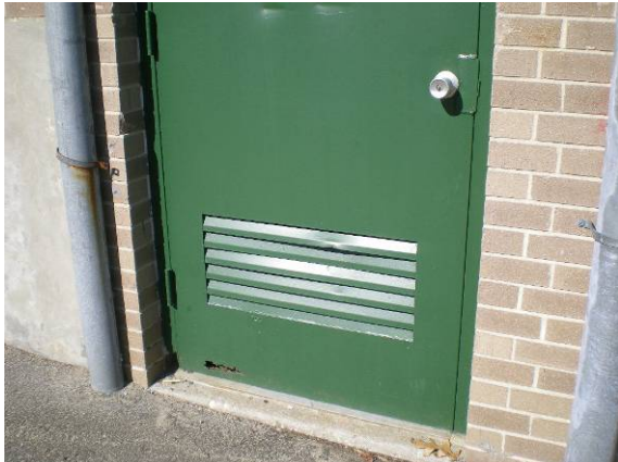
Photo #21: Service door condition
