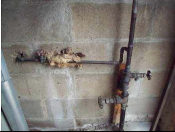
Photo #127: Incoming water service for annex building
