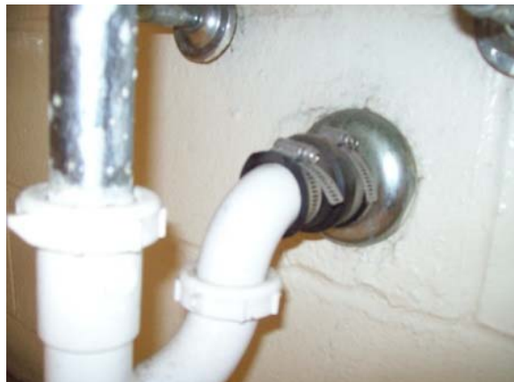
Photo #96: Prior repairs to drain lines
