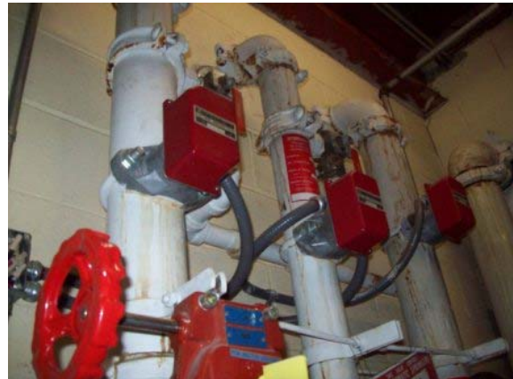
Photo #112: Fire sprinkler risers
