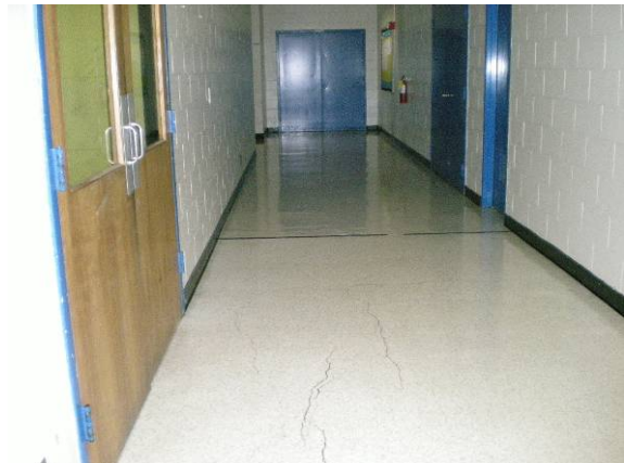
Photo #52: Cracks in corridor flooring finish
