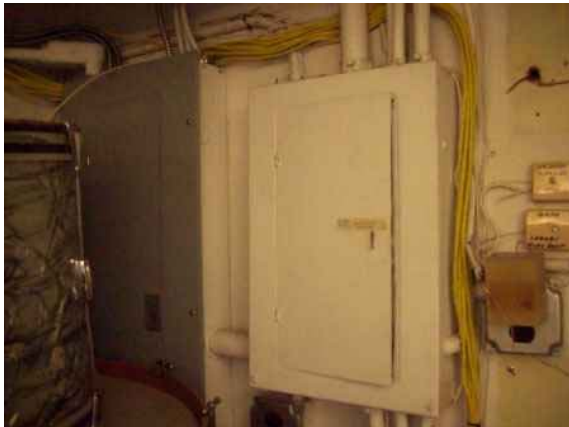
Photo #129: Main breaker panel for annex building
