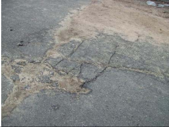
Photo #31: Asphalt damage in service drive
