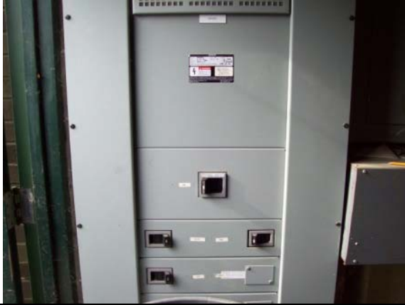
Photo #103: Main breaker panel
