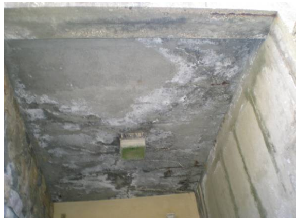
Photo #24: Underside of cracked landing on side entrance
