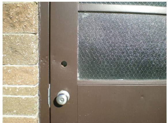
Photo #132: Missing locking device at Annex building
