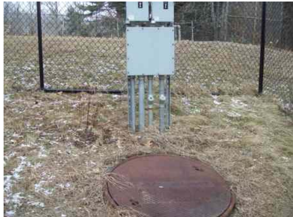
Photo #94: Sanitary waste force main pumping station
