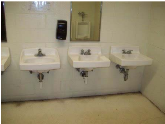
Photo #95: Typical restroom fixtures
