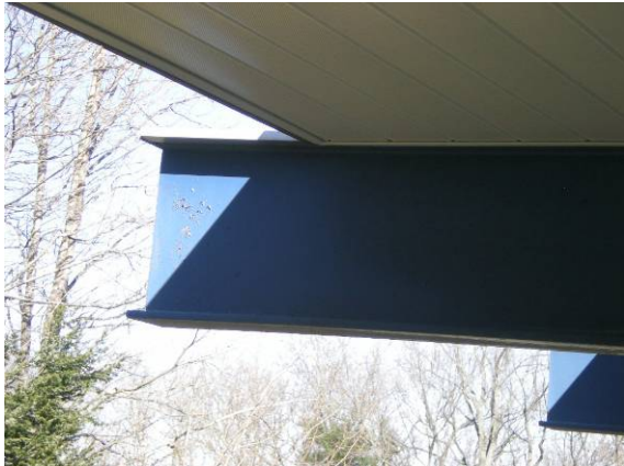
Photo #15: Exposed structure of Media Center with isolated rust
