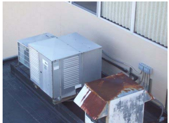
Photo #120: Walk in refrigeration compressor units
