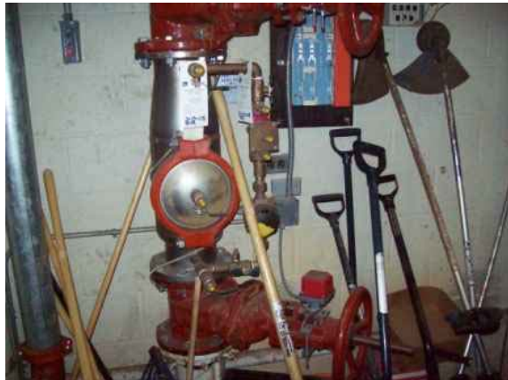
Photo #111: Backflow preventer for sprinkler system
