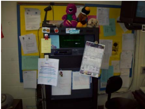
Photo #105: PA system in main office
