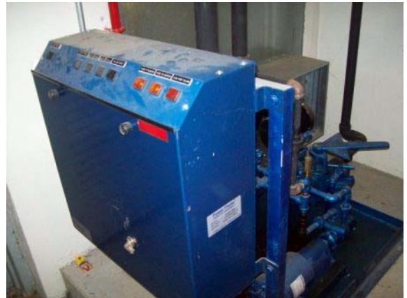
Photo #82: Fuel oil pump set
