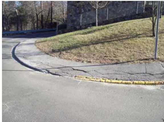
Photo #34: Asphalt damage at asphalt walking path
