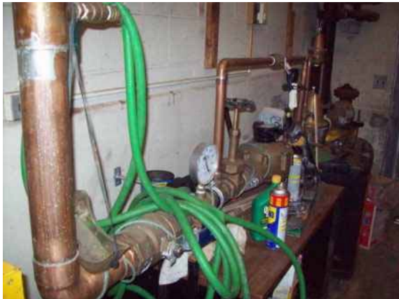
Photo #93: Domestic water service connection
