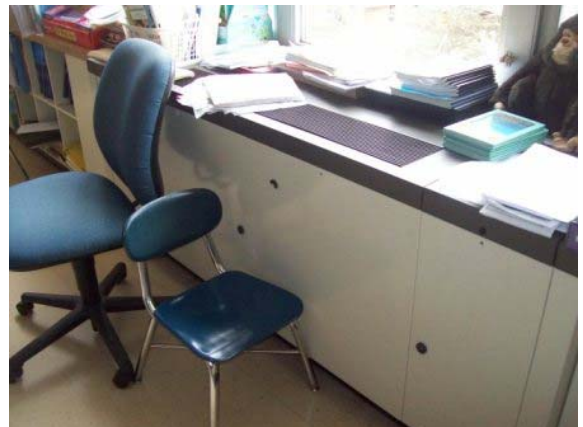
Photo #84: Typical unit ventilator
