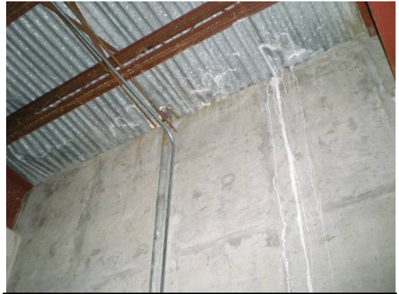
Photo #74: Water infiltration at subterranean wall in storage area at front of building
