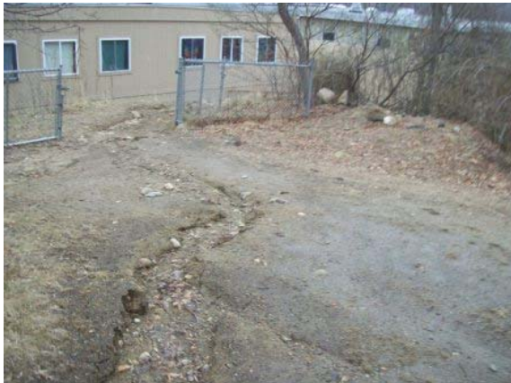
Photo #39: Erosion at south side of building, from baseball fields
