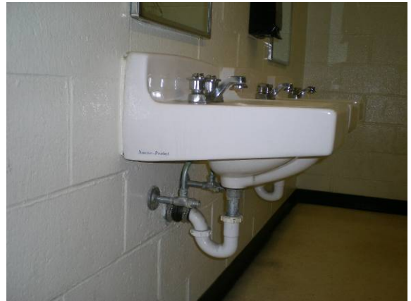
Photo #58: Common restroom
