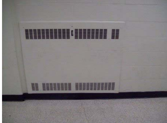
Photo #86: Typical convection unit
