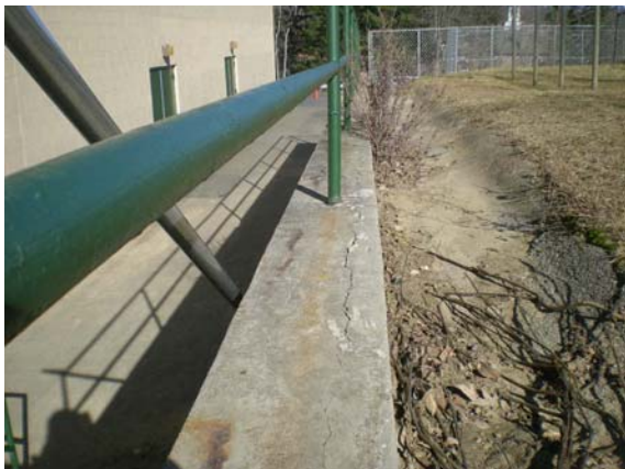
Photo #41: Cracking along top of retaining wall
