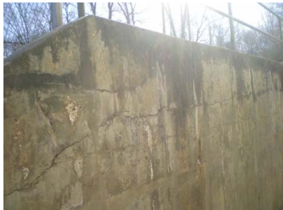
Photo #42: Cracking along face of retaining wall
