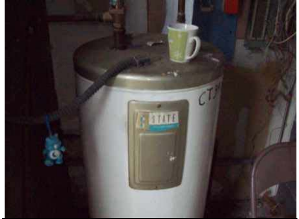
Photo #128: Domestic water heater for annex building
