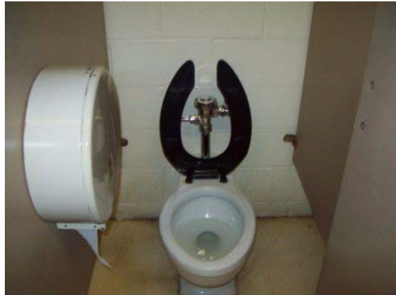
Photo #98: Typical toilet fixture
