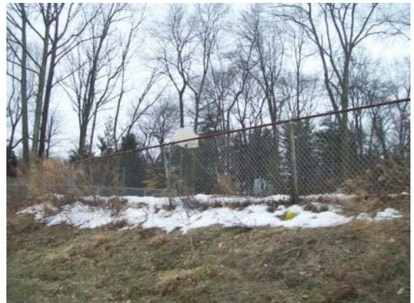
Photo #48: Damaged site fencing
