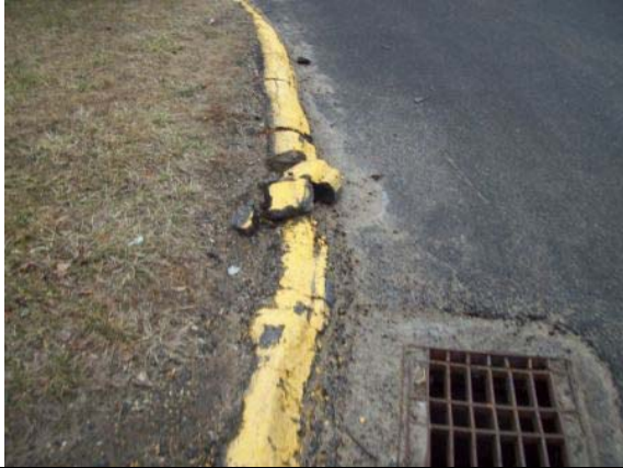
Photo #37: Damage to asphalt curbing
