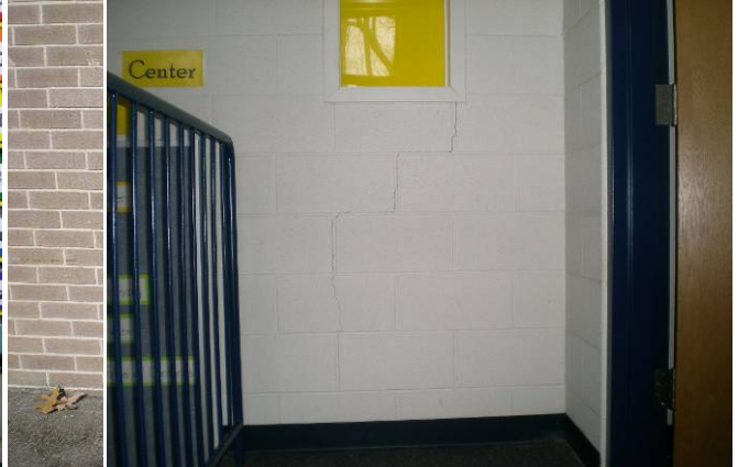
Photo #68: Settlement cracking in Media Center
