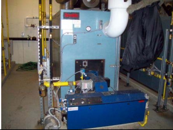
Photo #79: Boiler (1 of 2)
