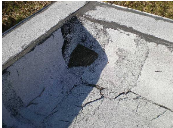
Photo #18: Cracked built up roofing and parapet wall topped with built up membrane
