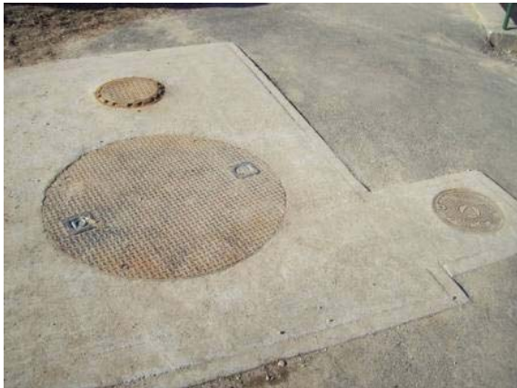
Photo #81: Fuel oil underground storage tank
