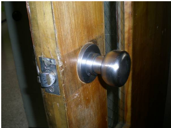
Photo #59: Classroom door hardware with no locking mechanism from interior
