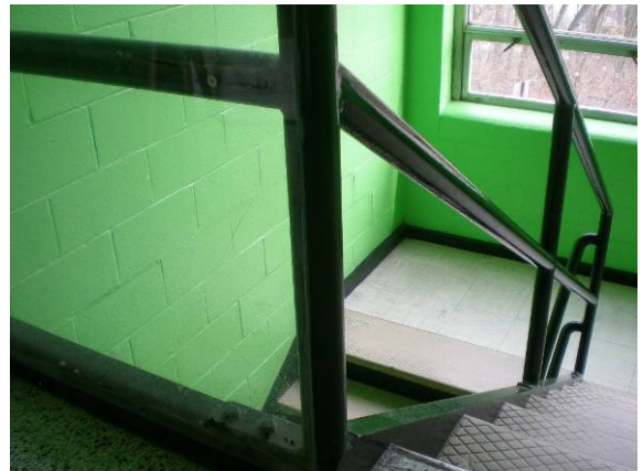
Photo #60: Stairwell with acrylic at top landing but no protection along stair portion of railing
