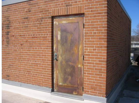
Photo #26: Several of the outdoor common and roof access doors are rusted
