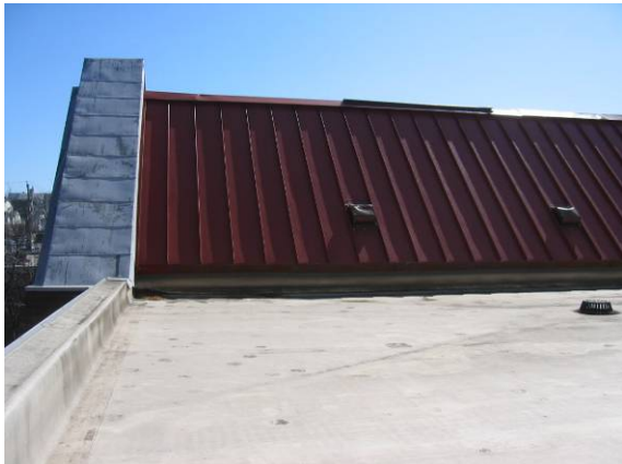
Photo #27: Detail of the pitched, standing seam metal roof above the office lobby
