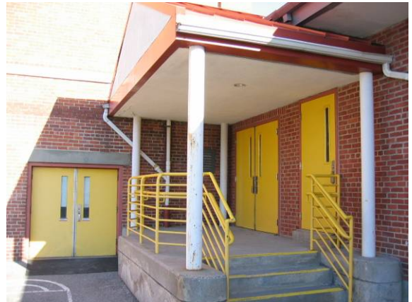
Photo #4: Secondary common entrances exist on all façades. note peeling paint
