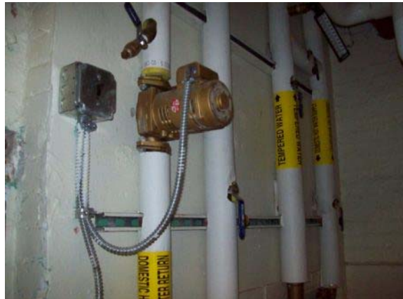
Photo #94: Domestic water circulating pump
