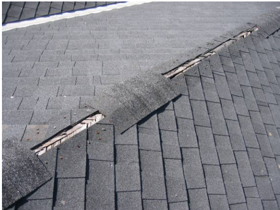
Photo #33: Detail of the damaged or missing roof shingles along the hip ridges
