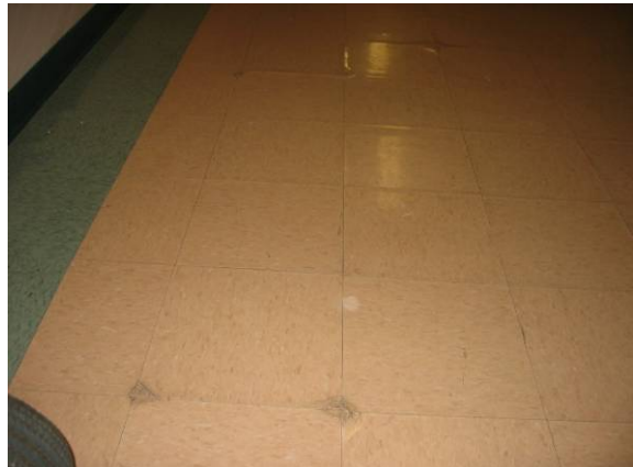
Photo #52: Detail view of several isolated sections of damaged VCT floor tiles
