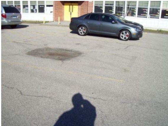
Photo #123: Damaged area in staff parking lot
