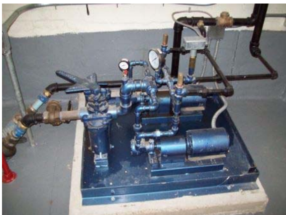
Photo #77: Fuel oil pump set
