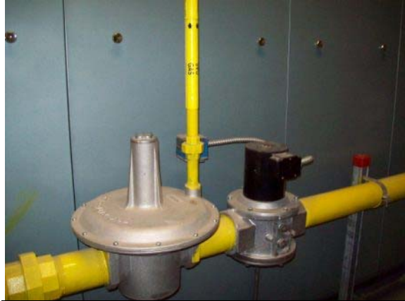
Photo #98: Natural gas regulator and distribution lines for boilers
