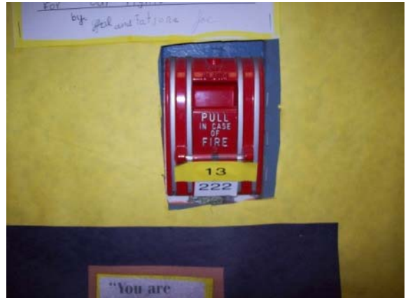
Photo #118: Fire alarm pull station
