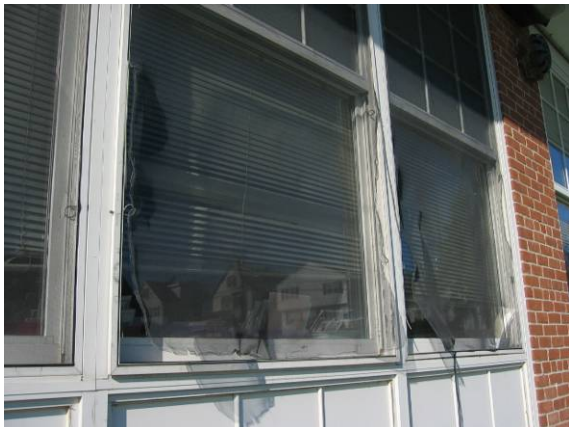
Photo #17: Detail of the widespread damaged window screens
