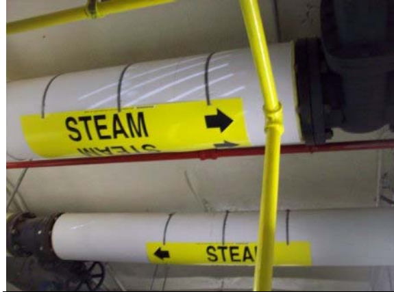
Photo #74: Steam distribution lines
