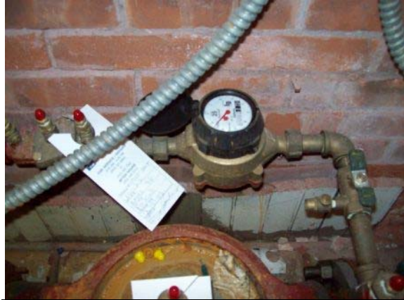
Photo #92: Domestic water meter
