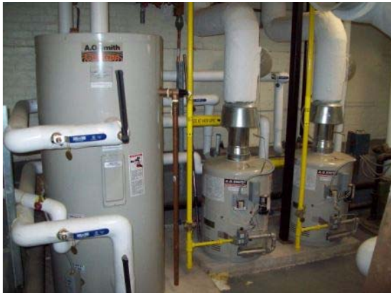
Photo #93: Domestic water boilers and storage tank
