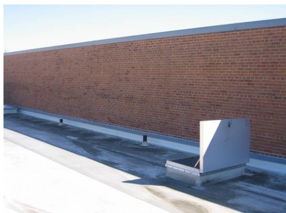
Photo #30: Access to the upper gymnasium flat roof would be improved with a fixed roof ladder secured to the brick wall
