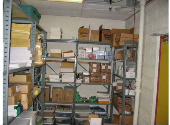
Photo #68: View of the school supply closet - stained/missing ceilings tiles were noted
