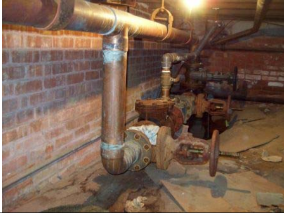
Photo #91: Domestic water service line
