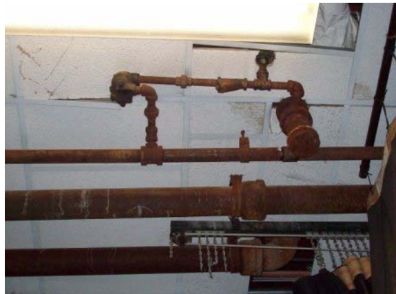
Photo #96: Corroded sanitary waste lines
