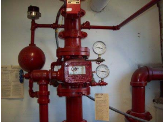
Photo #109: Wet pipe sprinkler riser
