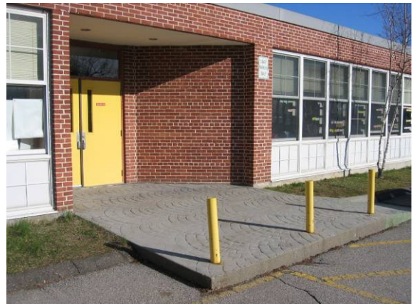
Photo #6: View of the common entrance to the kindergarten wing - no ADA ramp exists
