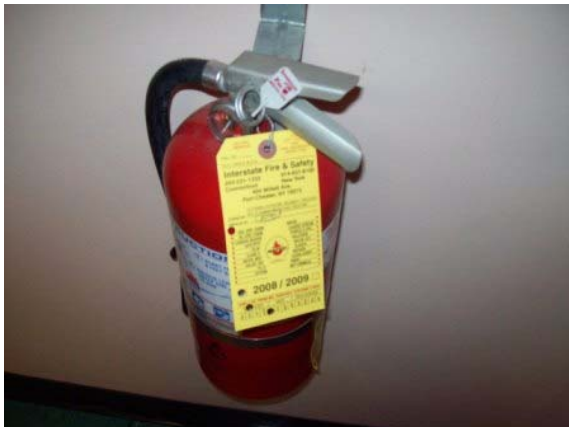
Photo #119: Fire extinguisher
