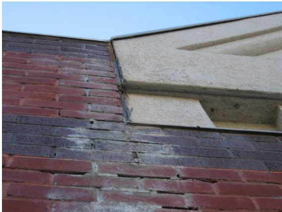
Photo #3: Detail of the efflorescence and worn brick mortar joints at main entrance
