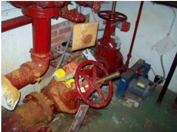
Photo #111: Dry-pipe sprinkler riser and compressor
