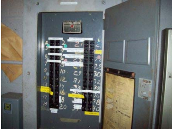
Photo #103: Breaker panel for stage lighting control
