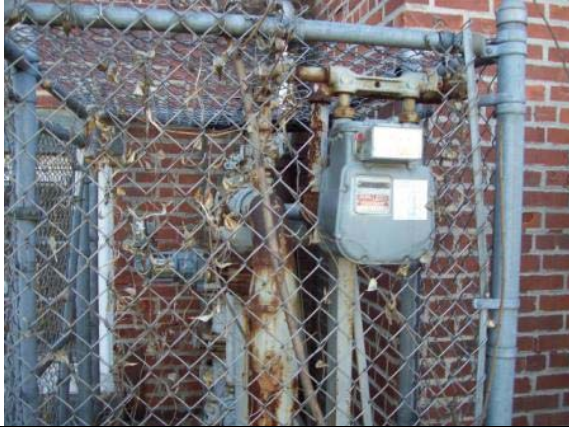
Photo #97: Natural gas meter
