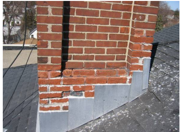
Photo #34: The brick chimney exhibited a few isolated open mortar joints
