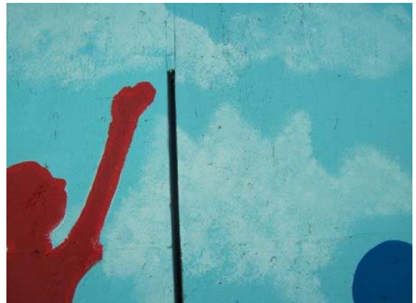
Photo #138: Expansion joint missing sealant (south retaining wall)
