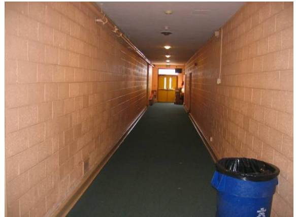
Photo #46: View of the egress corridor near the auditorium. A clogged or leaking roof drain exists within the CMU wall.
