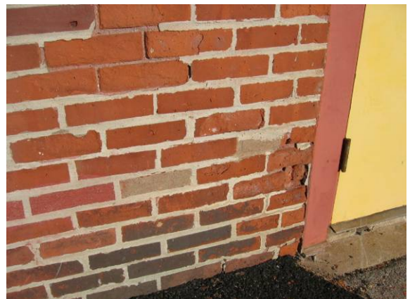
Photo #12: Detail of the isolated brick step cracks and open mortar joints
