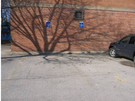
Photo #7: View of the two on-site ADA parking stalls - striping is faded and no access aisle exists
