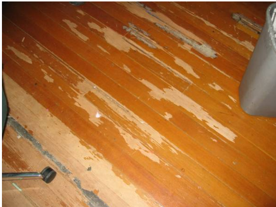
Photo #45: Detailed view of the deteriorated auditorium stage wood planks
