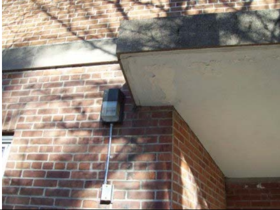
Photo #145: Exterior building-mounted lighting
