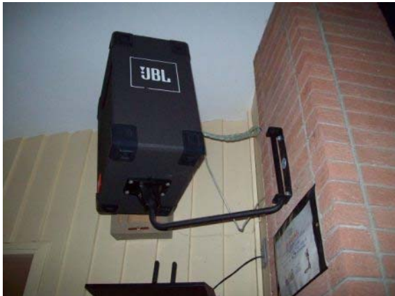
Photo #105: Auditorium sound system
