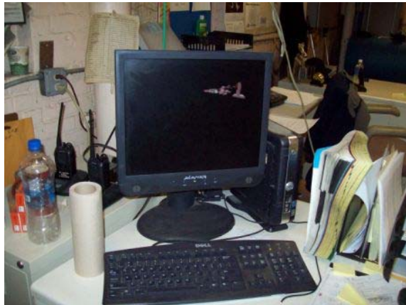
Photo #87: HVAC control terminal
