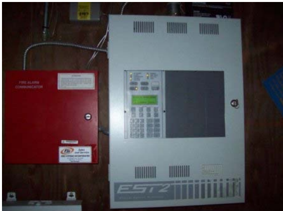
Photo #113: Fire alarm control panel
