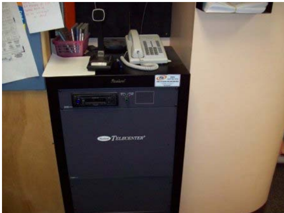
Photo #107: Public address system control unit
