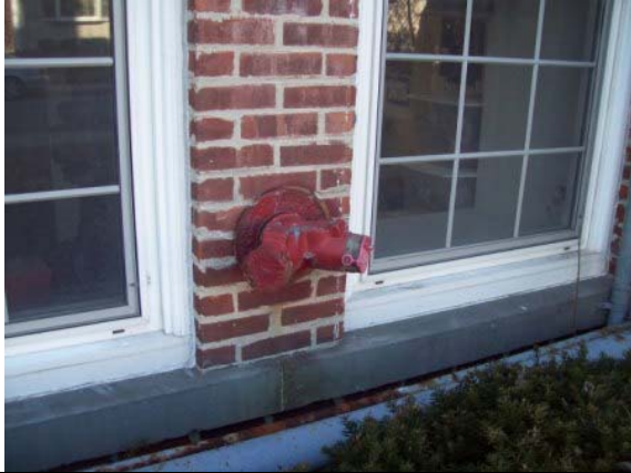
Photo #115: Fire department Siamese connection on building exterior
