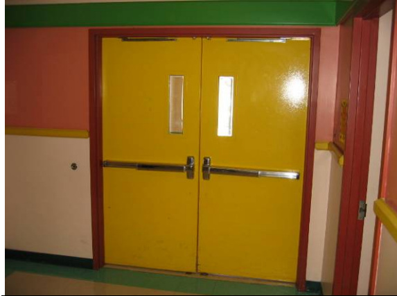
Photo #56: Several of the interior corridor/stairwells fire doors do not close properly
