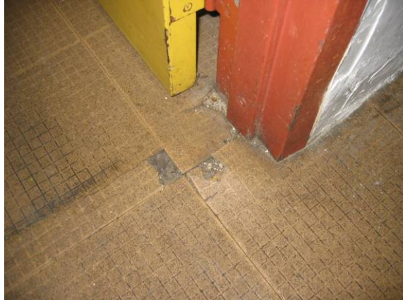
Photo #49: Detail view of the deteriorated and lifting kitchen floor tiles
