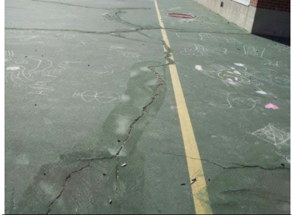
Photo #128: Cracking in paved area
