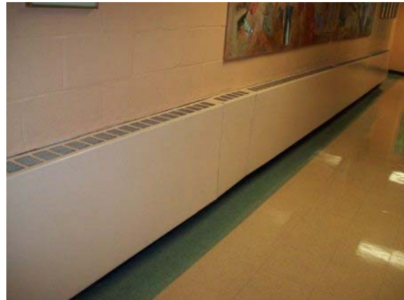
Photo #76: Typical radiant heat unit
