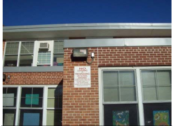
Photo #146: Exterior building-mounted lighting
