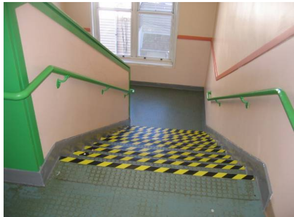
Photo #54: The two interior wood stairwells within the 3-story portion appear out of level/plumb and with soft spots
