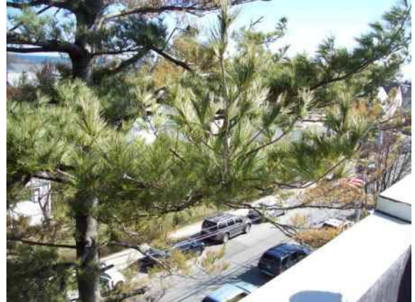
Photo #134: Tree growing close to school building
