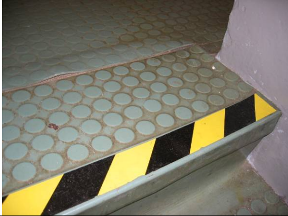
Photo #55: Several sections of the textured vinyl floor material are lifting on the landings
