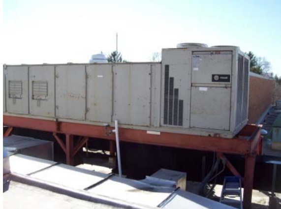
Photo #79: Rooftop air conditioning unit for media center area
