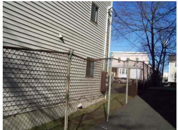
Photo #144: Damaged fence at north property line
