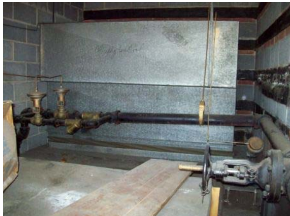
Photo #83: Make-up air unit for gymnasium/cafeteria
