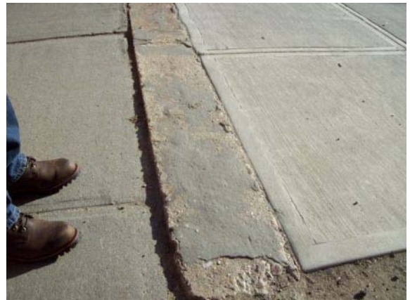
Photo #132: Tripping hazard near front entrance
