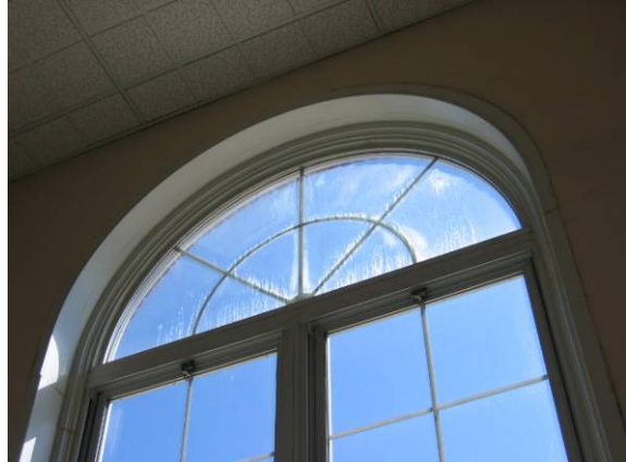
Photo #20: Several of the stairwell and classroom windows were failed with fogging
