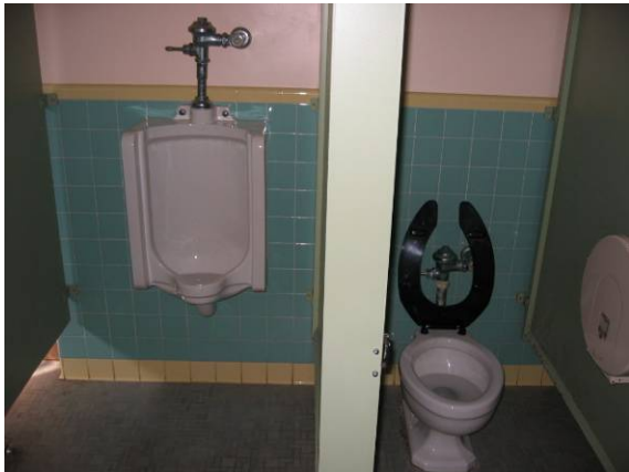
Photo #63: Neither of the multi-user toilet rooms near the auditorium provide ADA access
