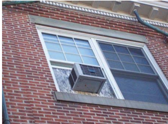
Photo #86: Typical window air conditioning unit note plywood installation
