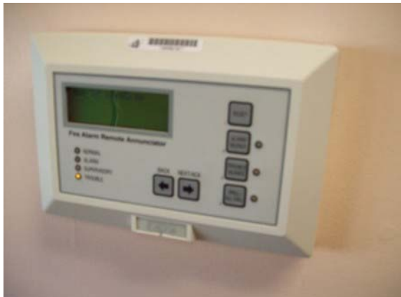
Photo #114: Fire alarm annunciator panel
