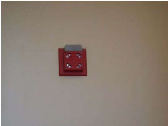
Photo #117: Fire alarm horn with strobe light
