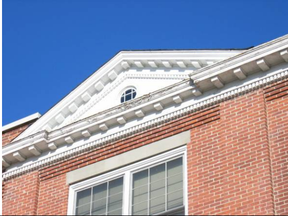
Photo #13: Detail of the rear façade roof dormer with deteriorated wood trim
