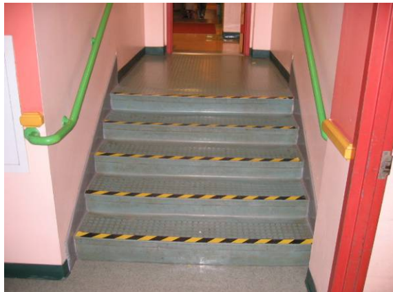
Photo #53: Several short stair runs exist connecting the two main building sections - no wheelchair lifts exist
