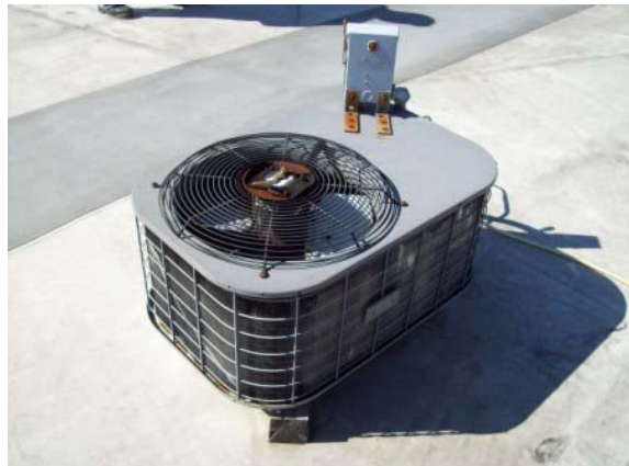
Photo #84: Split condensing unit for Classroom 1
