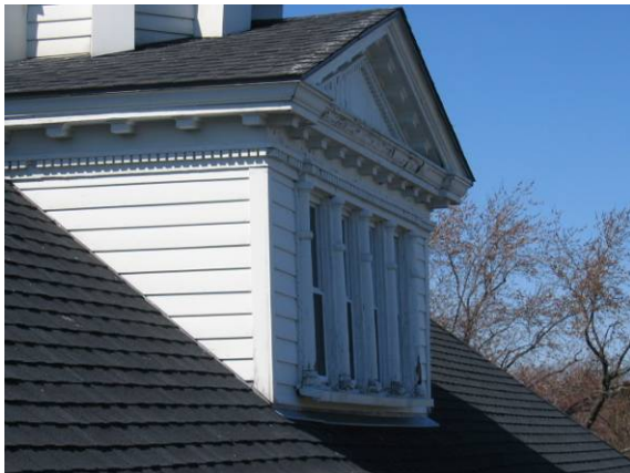
Photo #35: Close-up views of the front and rear wood dormers revealed peeling paint and deteriorated wood trim
