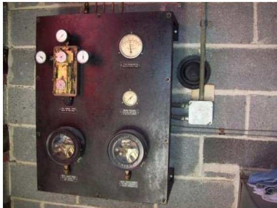
Photo #89: Pneumatic control panel
