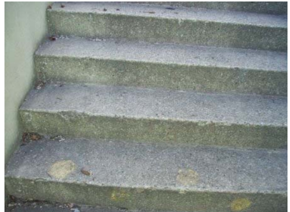
Photo #130: Damage at concrete steps
