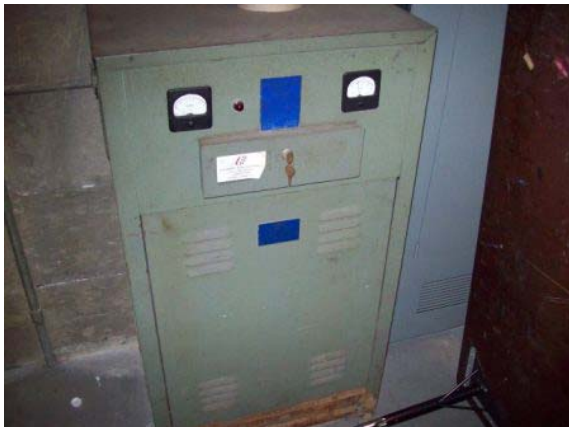
Photo #101: Battery backup system
