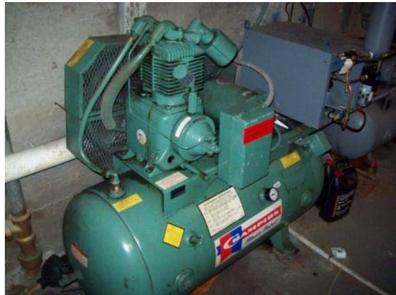
Photo #88: Compressor for pneumatic controls
