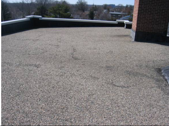
Photo #37: Two flat gravel surfaced built-up roof (BUR) sections also exist at the 3-story portion at the east and west ends
