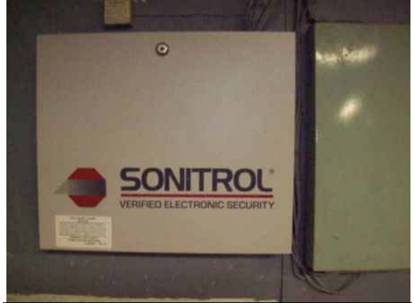
Photo #116: Security control panel
