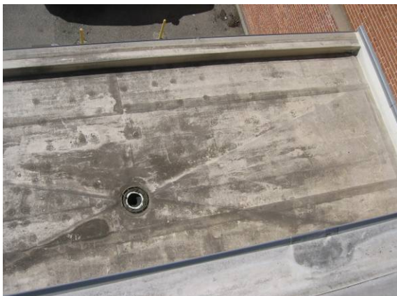
Photo #23: Several of the flat roof drain strainers were observed to be missing
