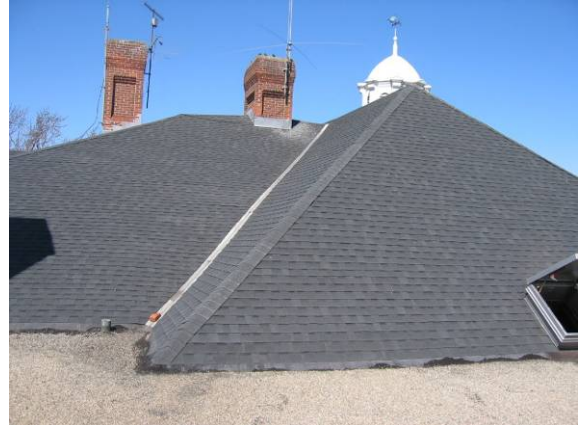
Photo #32: View of the pitched asphalt shingle roof over the original 3-story portion
