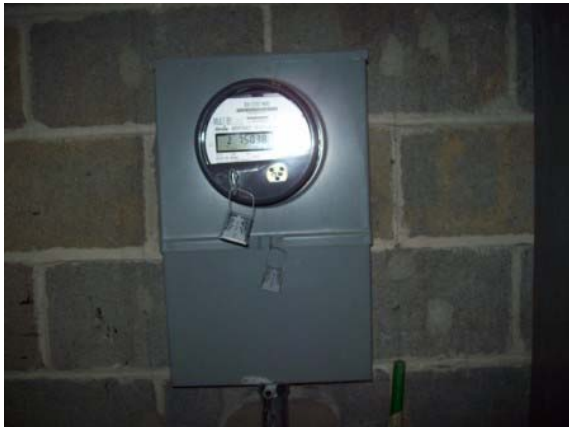
Photo #99: Electric meter
