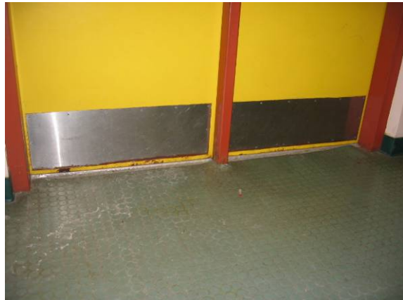
Photo #58: Detail view of the rusted and delaminating exterior doors
