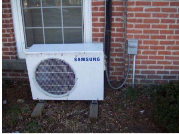
Photo #85: Ductless split system for Classroom 16
