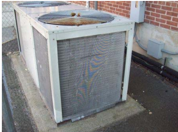
Photo #81: Split condenser for auditorium (1 of 2)
