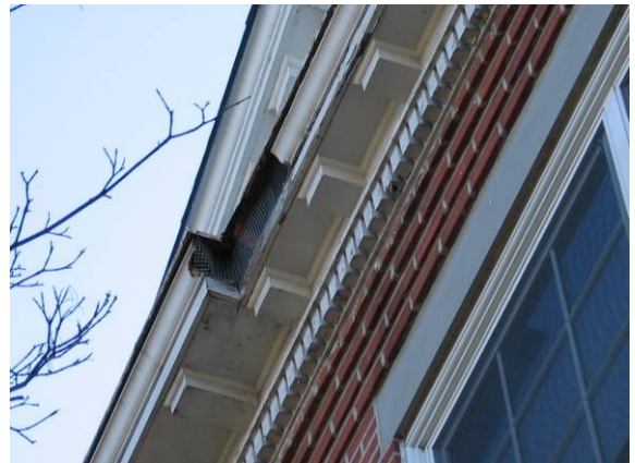
Photo #10: Detail of deteriorated wood soffits and eaves at the 3-story portion
