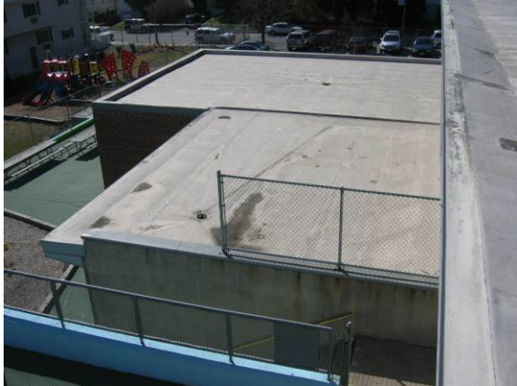
Photo #25: A short length of chain link fence was installed but has been unsuccessful
