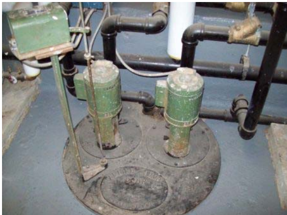
Photo #95: Sump pump
