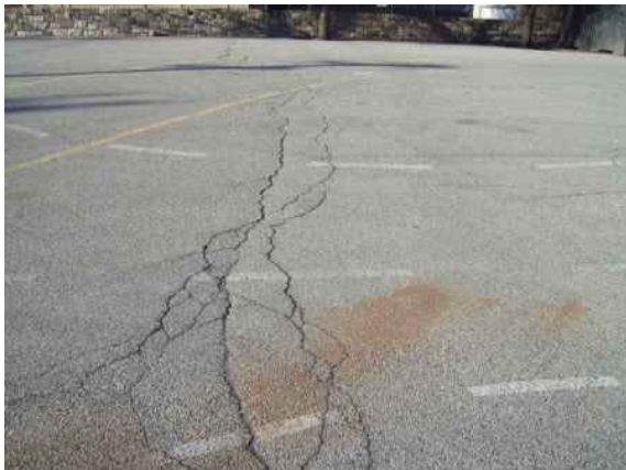
Photo #125: Damage in northwest paved area
