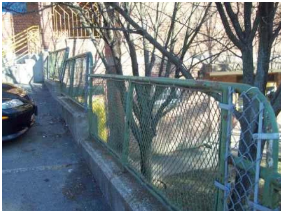
Photo #143: Damaged fence at west retaining wall
