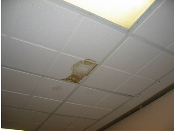
Photo #43: Isolated sections of the suspended acoustic ceilings were stained
