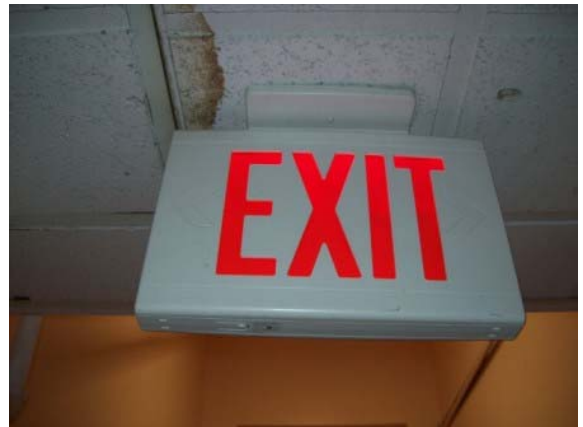
Photo #120: Exit light
