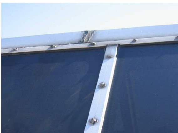
Photo #29: One occasional leak was reported in the media center skylight system
