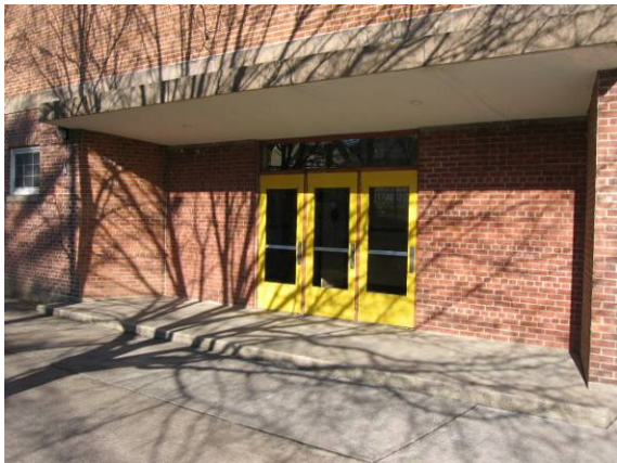
Photo #5: View of the common entrance to the auditorium - no ADA ramp exists
