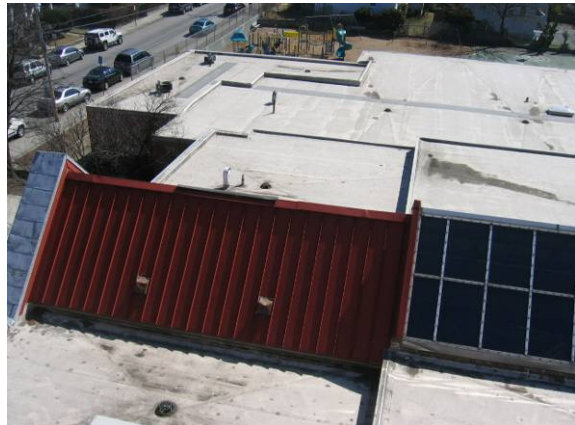
Photo #22: Overview of the EPDM roofs towards the front - the pitched metal roof is over the office lobby entrance
