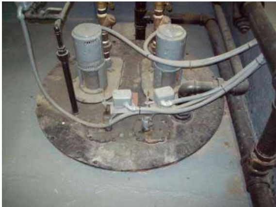
Photo #75: Condensate pumps
