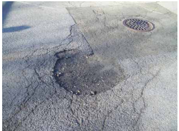
Photo #126: Damage in northwest paved area
