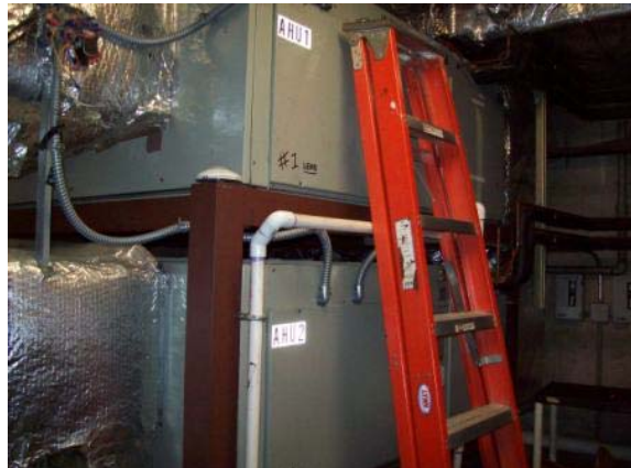
Photo #82: Fan coil units for auditorium
