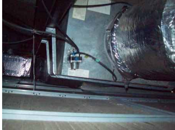
Photo #80: Typical VAV terminal
