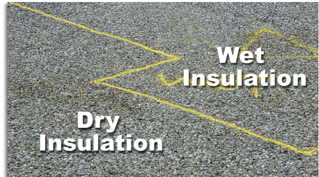
Control image, wet sections marked for removal
