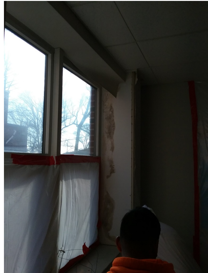
Wall covering was removed on the 2 nd floor hallway to identify leaks and mold growth.
