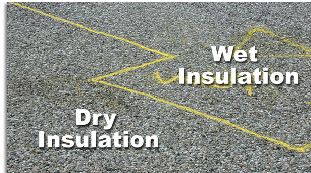
Control image, wet sections marked for removal
