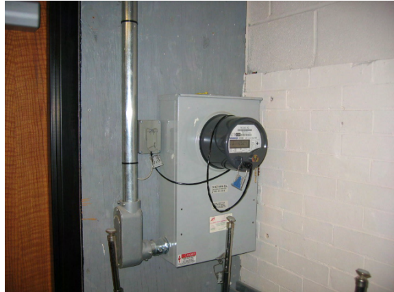
Photo #40: View of electrical metering equipment.
