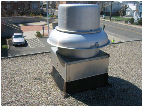
Photo #33: View of exhaust fan.
