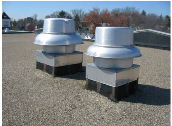
Photo #34: View of exhaust fans.
