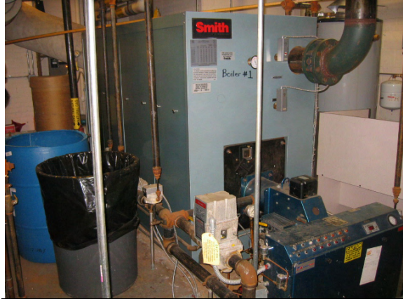
Photo #20: View of Boiler No. 1.
