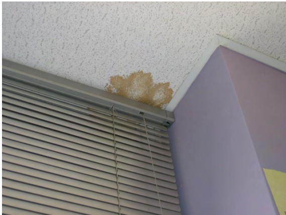
Photo #105: A few isolated stained ceiling tiles were noted along corridors and within rooms.
