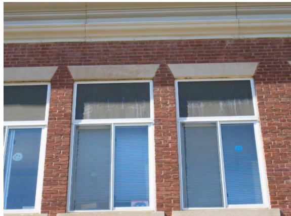
Photo #72: Detail view of the typical upper floor windows with deteriorated masonite transoms.
