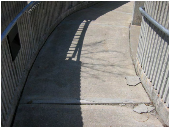
Photo #63: Several sections of deteriorated, spalled and/or settled concrete exist at the ramp.
