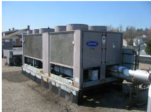
Photo #24: View of chiller.
