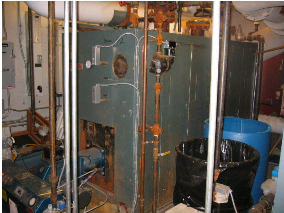
Photo #21: View of Boiler No. 2.
