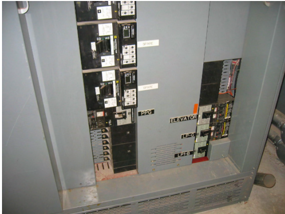
Photo #41: View of missing safety covers on main electrical panels.
