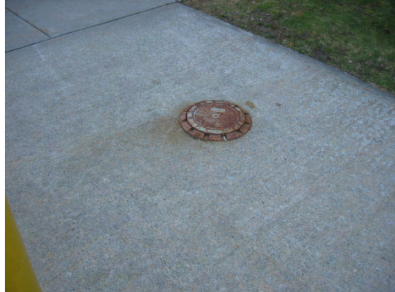
Photo #56: View of underground fuel oil tank fill port.
