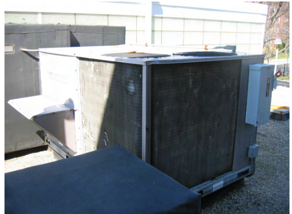
Photo #28: View of RTU-4.
