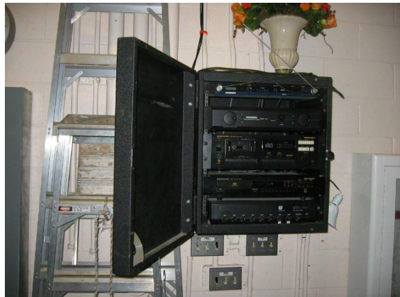
Photo #54: View of auditorium sound system.
