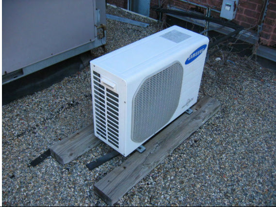
Photo #31: View of data center split DX unit.
