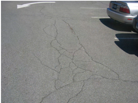
Photo #3: View of open pavement cracks.
