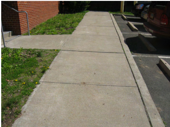
Photo #9: View of cast in place concrete sidewalks, which are adjacent to the front parking lot.
