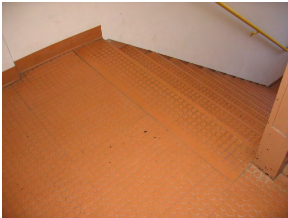
Photo #89: Nearly all of the stairwell textured rubber flooring at landings and treads is lifting.
