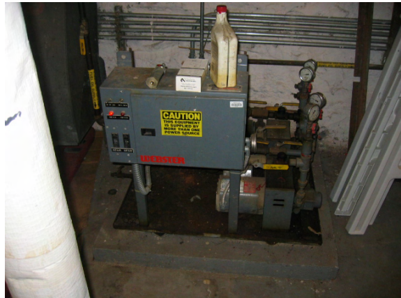
Photo #22: View of fuel oil pumps.
