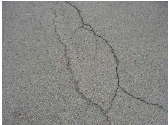
Photo #4: View of open pavement cracks.
