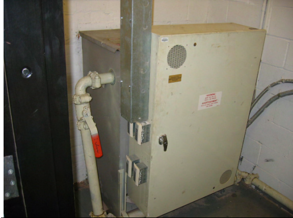
Photo #50: View of passenger elevator equipment.
