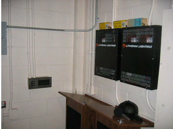
Photo #55: View of auditorium lighting control system.
