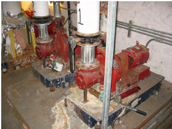
Photo #23: View of water circulation pumps.
