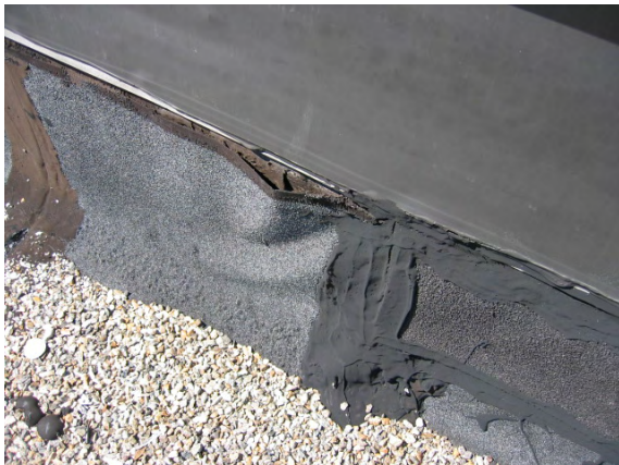
Photo #77: Detail of the isolated deteriorated mastic and base flashings along parapets.
