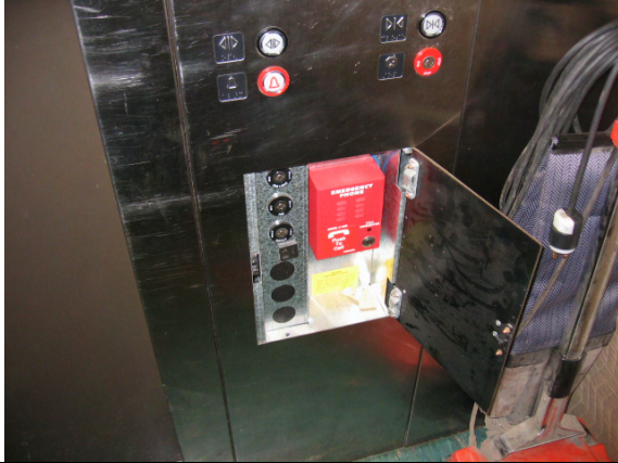
Photo #49: View of passenger elevator control panel.
