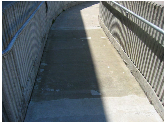
Photo #12: View of cast in place concrete ramp, which is located at the main entrance.
