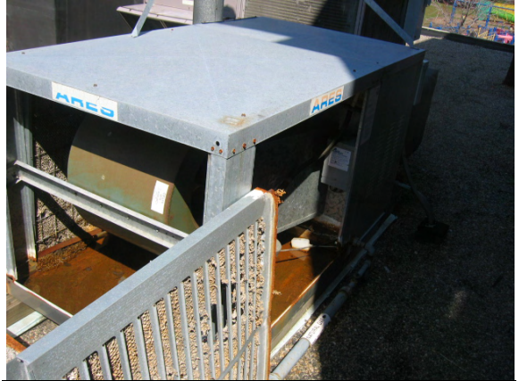
Photo #32: View of auxiliary heating unit for kitchen.
