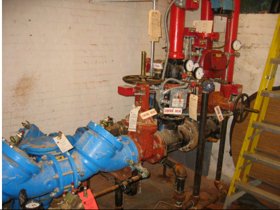
Photo #43: View of fire sprinkler valving.
