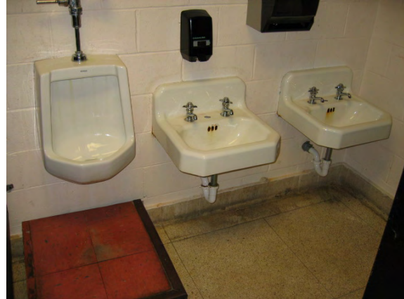
Photo #110: The toilet rooms near the gym/cafeteria have not been renovated to comply with ADA.
