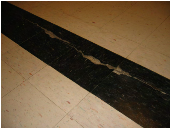
Photo #87: Isolated section of the corridor and classroom VCT flooring are cracked.
