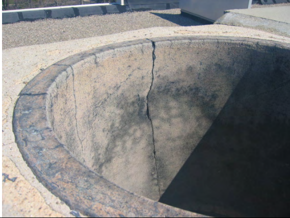
Photo #79: Detail of the cracking within the concrete and tile main boiler chimney.
