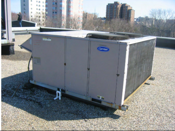
Photo #25: View of RTU-1.
