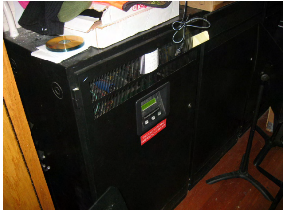
Photo #42: View of back-up battery systems.
