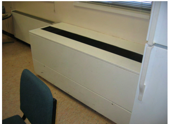
Photo #36: View of typical fan coil unit.
