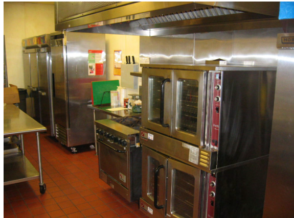
Photo #52: View of commercial kitchen equipment.
