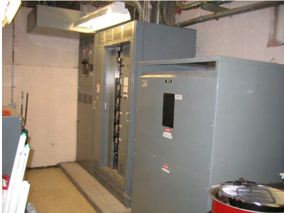
Photo #39: View of main electrical switchgear.
