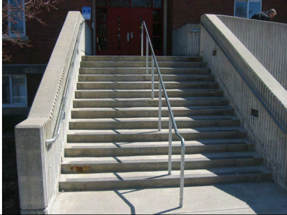
Photo #13: View of cast in place concrete steps at the main entrance.
