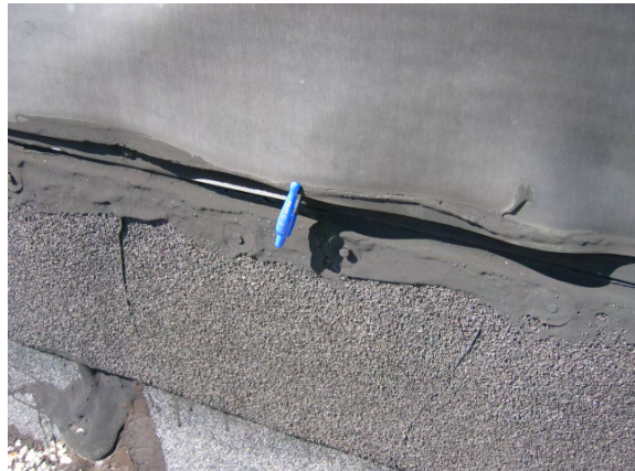
Photo #76: Isolated sections of the inboard parapet EPDM are loose and require repair.
