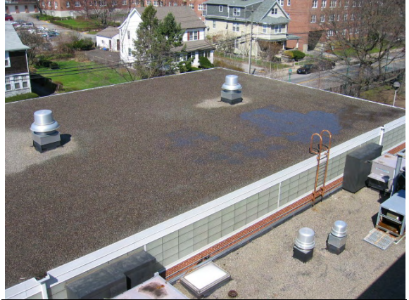
Photo #80: Overview of the flat GSBUR gymnasium roof. Note ponding. Additional drains are required.
