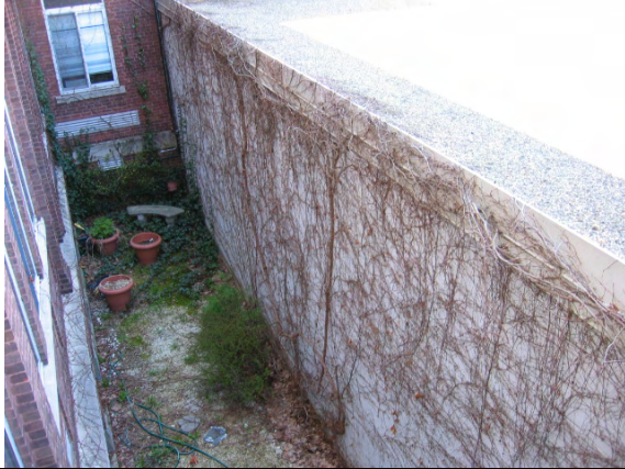
Photo #73: View of an inner courtyard and rear gymnasium wall. Note vine growth.
