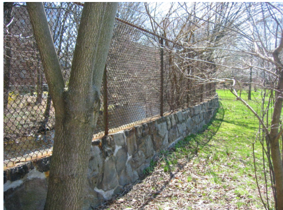
Photo #18: View of wet set stone retaining wall and chain link fencing system.
