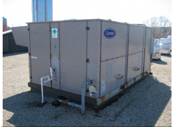
Photo #26: View of RTU-2.
