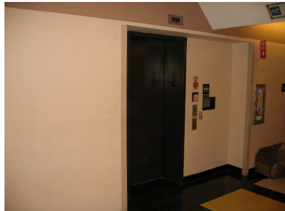
Photo #112: The school is equipped with a single passenger elevator.
