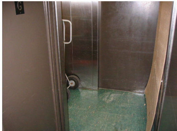
Photo #48: View of hydraulic passenger elevator cab.
