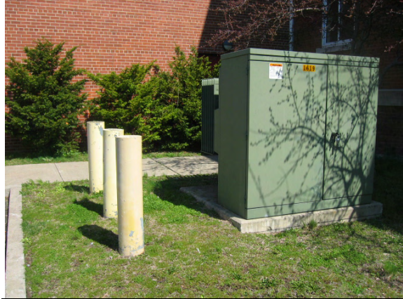
Photo #38: View of pad-mounted electrical transformer.
