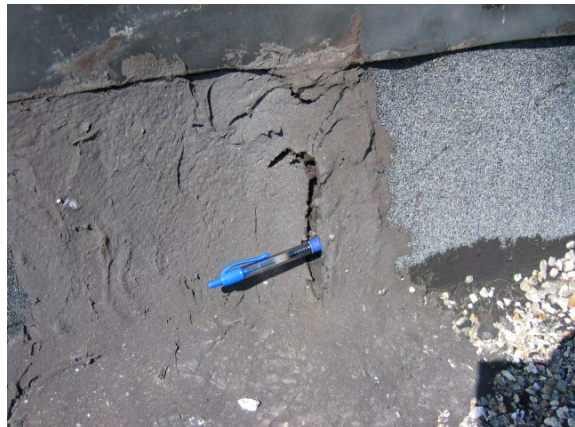
Photo #78: Detail of failed and dry/brittle mastic along parapet inboard surfaces.
