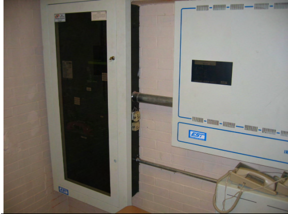
Photo #44: View of fire control panel.
