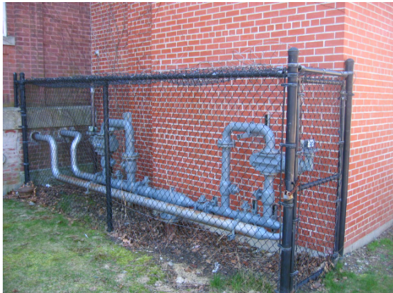
Photo #57: View of gas metering equipment.
