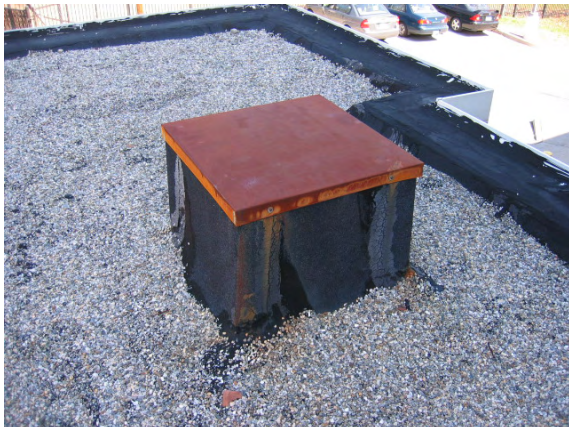
Photo #81: A few of the rooftop metals are rusted requiring routine maintenance and repainting.
