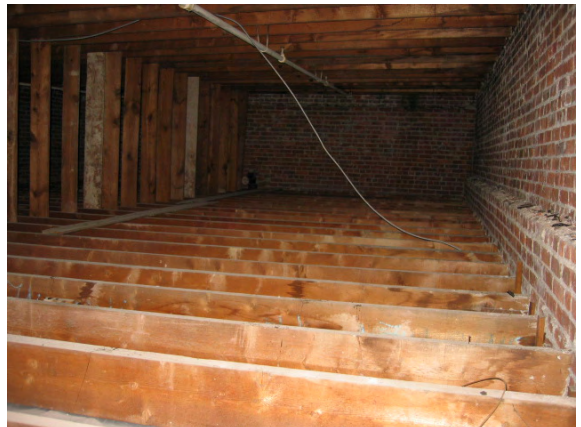
Photo #82: View of the wood framed attic space under the main flat roof system.
