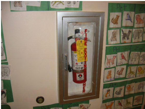
Photo #47: View of self contained fire extinguisher.
