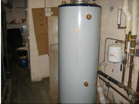
Photo #37: View of domestic hot water heater.
