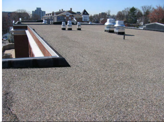
Photo #74: Overview of the gravel surfaced built-up roof (GSBUR) main roof system.
