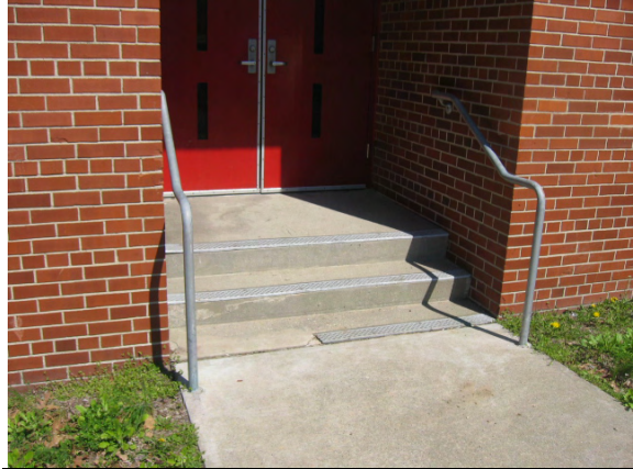
Photo #14: View of cast in place concrete steps at the auxiliary entrance to the Auditorium.
